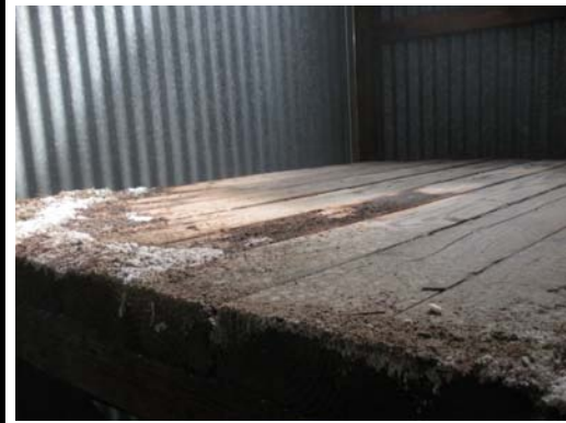
Photo 17 Facing Southeast Project Site Second Addition Soil Sample 8 Area Acid Vessel Wooden Platform Acid Crystals on Top
