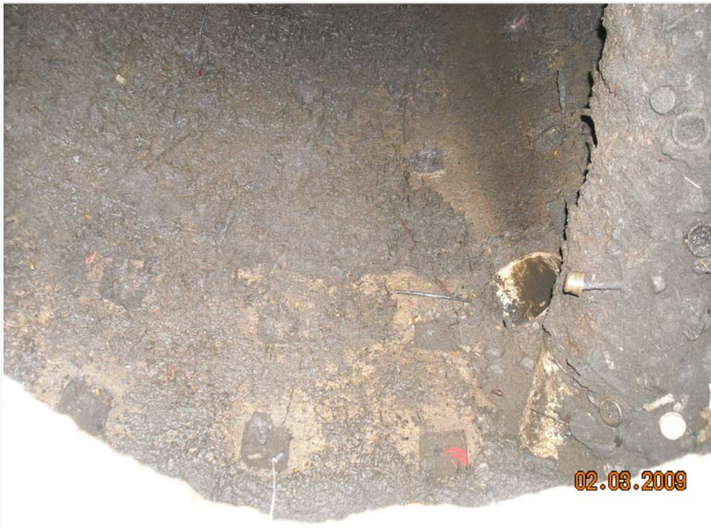
Photo 5. Smaller pipe, possibly from north catchbasin; visible on right side of photograph.
