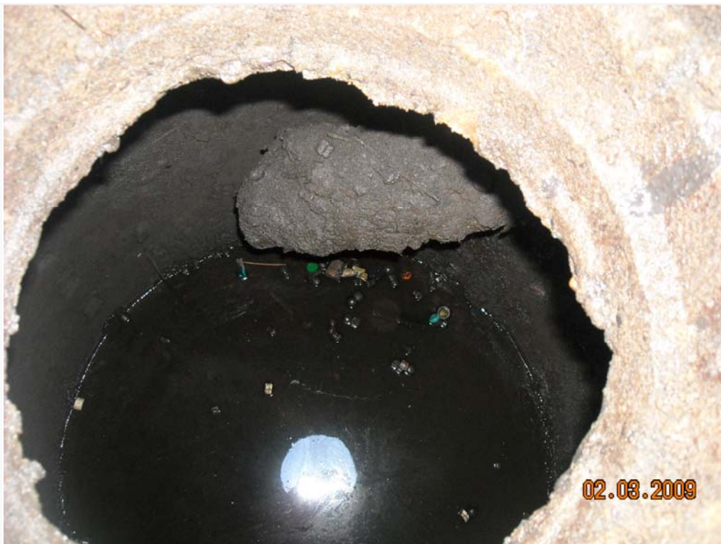
Photo 4. View inside drywell. Note sheen and debris in water. Pipe appears to be extending from east-adjacent catch basin.
