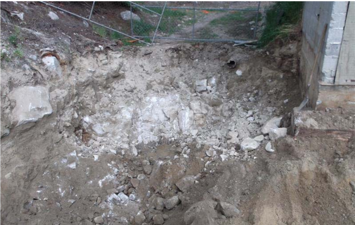
South to north view of northern corner of southern vehicle maintenance facility excavation.
