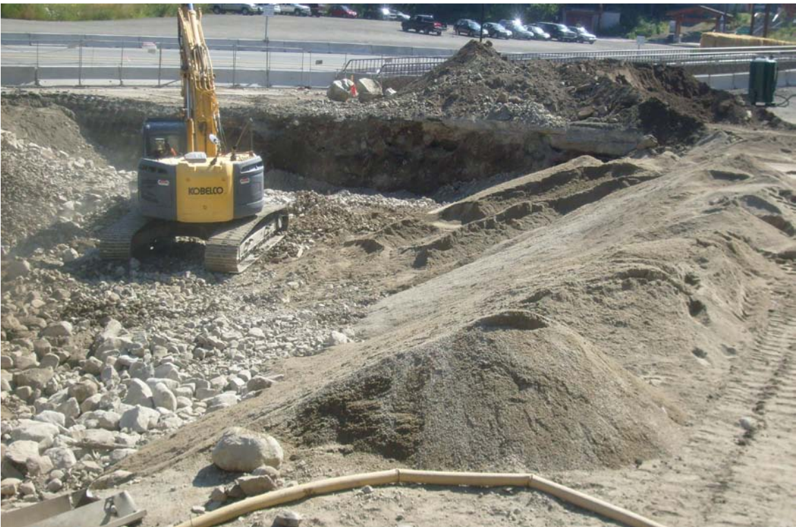
Northwest to southeast view of backfilling the southern part of the southern Mini Mart area excavation with cobbles and boulders.
