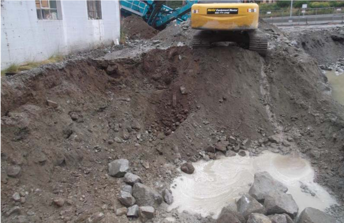
West to east view of northern end of southern Mini Mart area excavation, along the former maintenance building.
