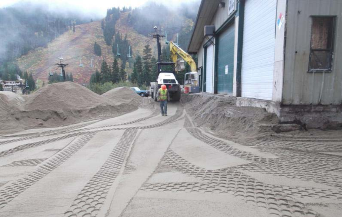
West to east view of backfilling of eastern part of northern vehicle maintenance facility excavation.
