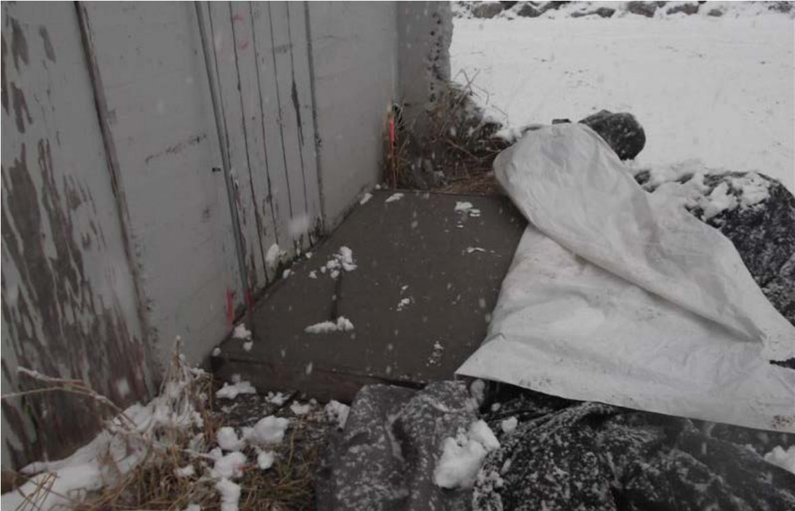
East to west view of concrete surface cap along northeast side of former maintenance building.
