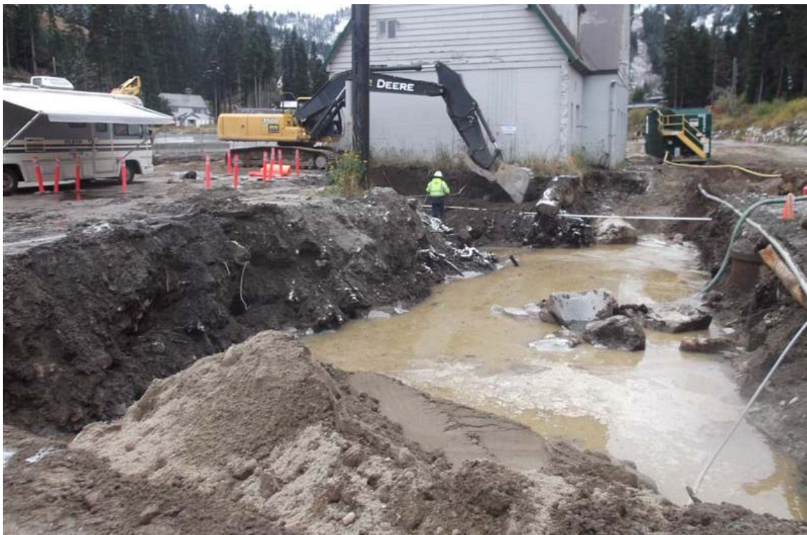
North to south view of groundwater extraction and initial backfilling in the northern part of the northern Mini Mart area excavation.
