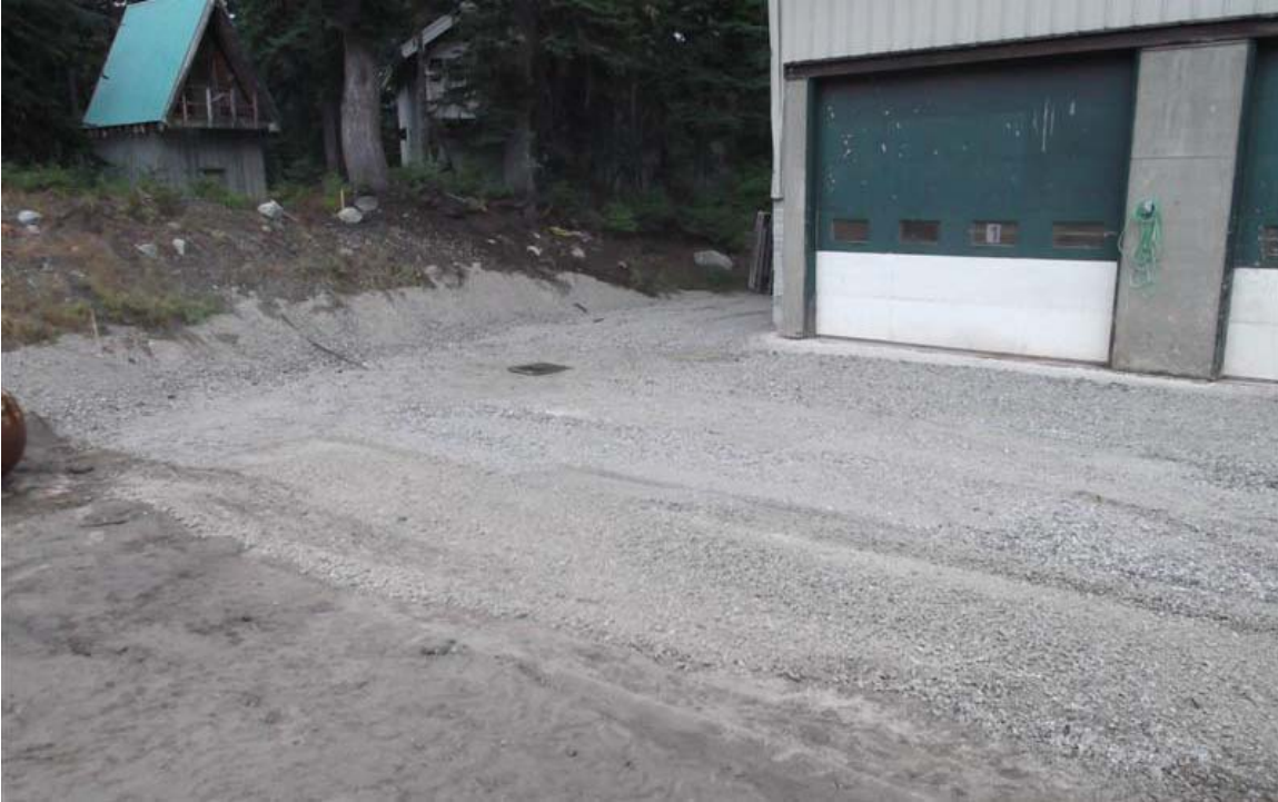
Southeast to northwest view of southern vehicle maintenance facility excavation area after backfilling.
