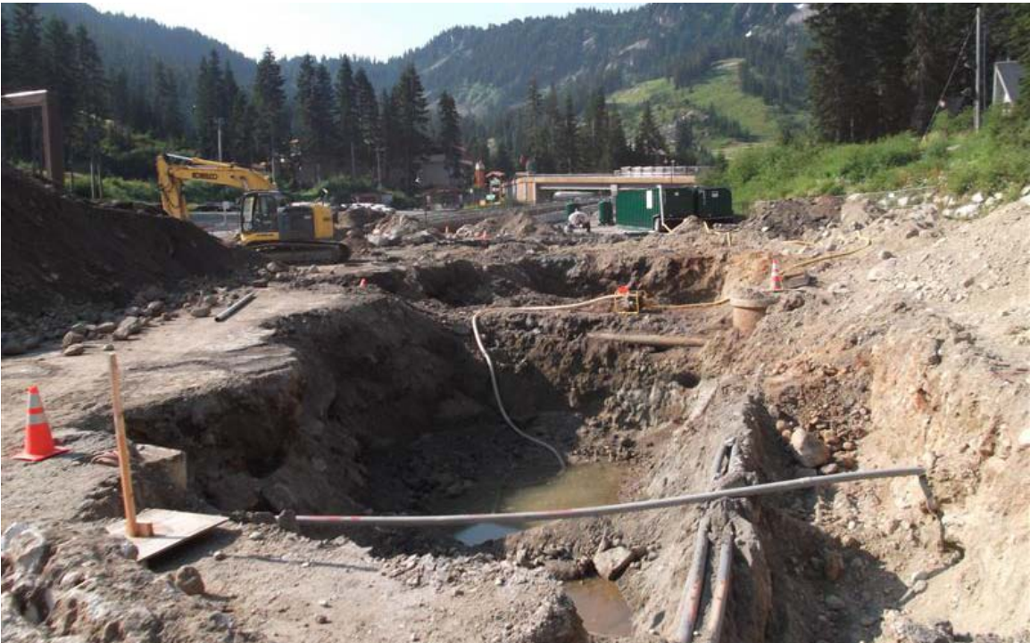
North to south view of southern Mini Mart area excavation after digging around several underground utilities. Groundwater extraction is being conducted at nearest excavation area.
