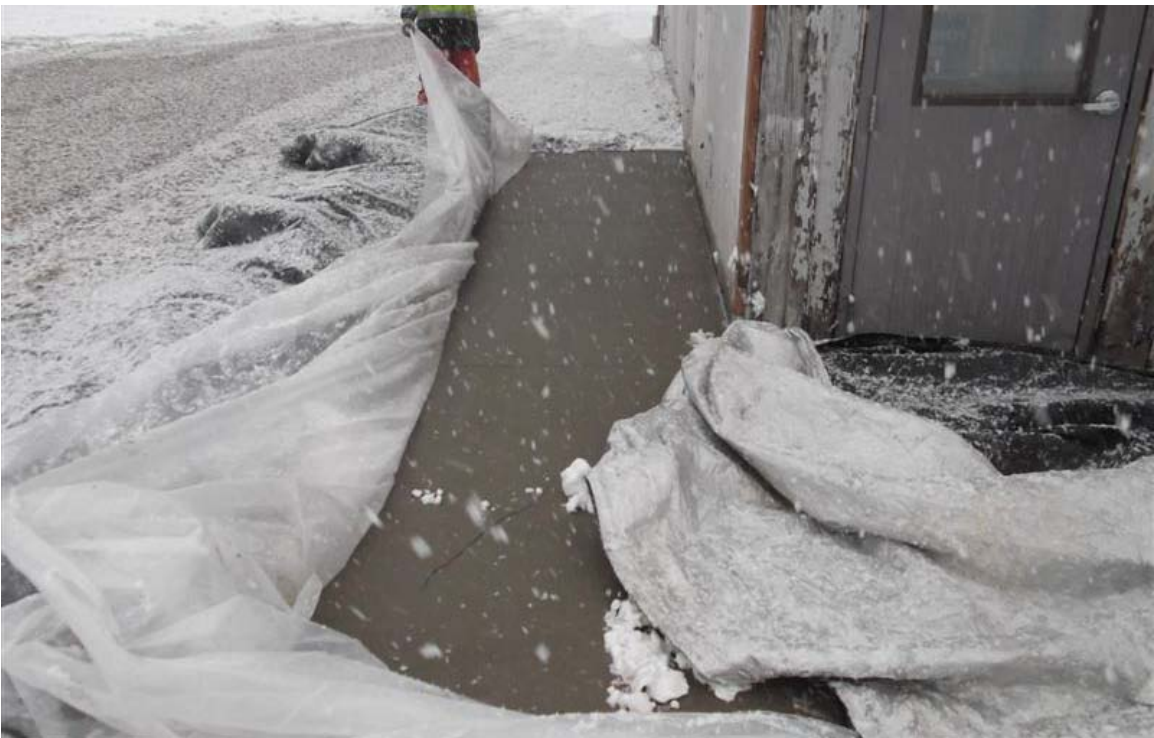
Western part of concrete surface cap near southeast corner of former maintenance building.
