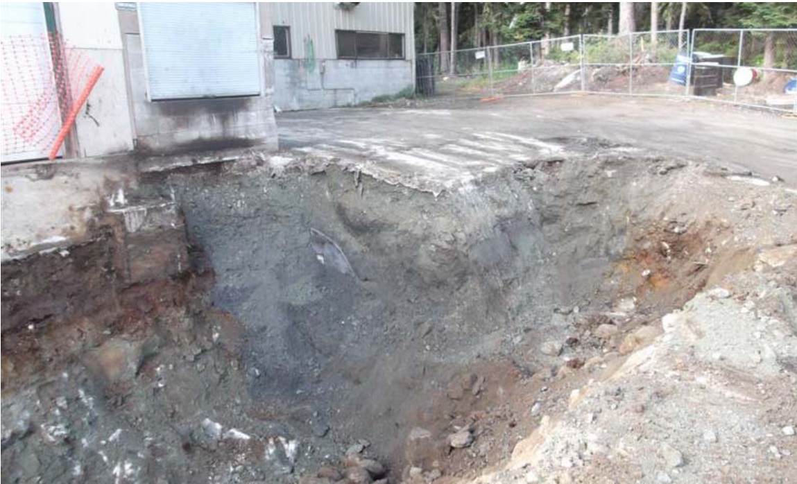
East to west view of gray-stained soil beneath fuel dispensing area and along the northeast corner of UST area at northern vehicle maintenance facility excavation. East end of gasoline UST is partially exposed.
