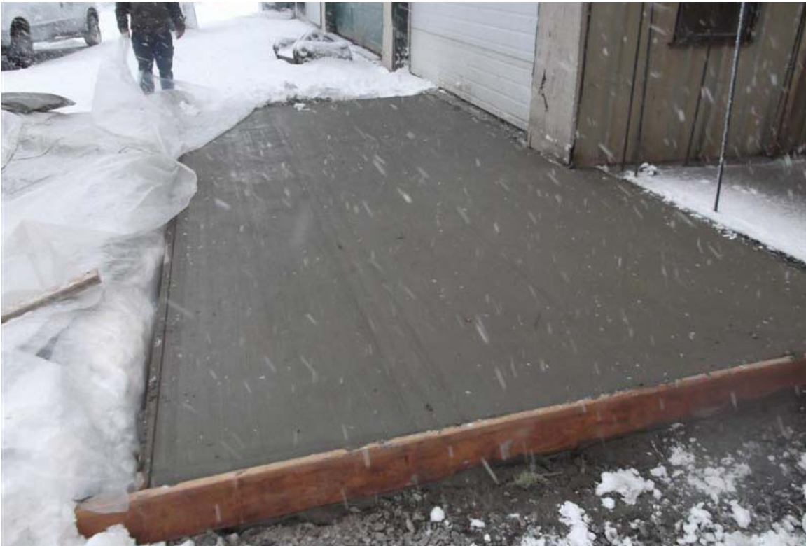
West to east view of northern portion of concrete surface cap along north side of vehicle maintenance building.
