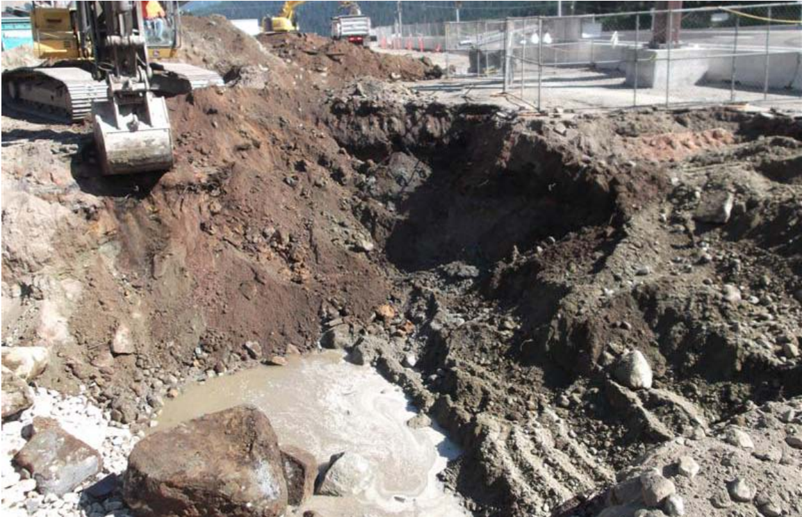
Southwest to northeast view of southeastern part of southern Mini Mart area excavation.
