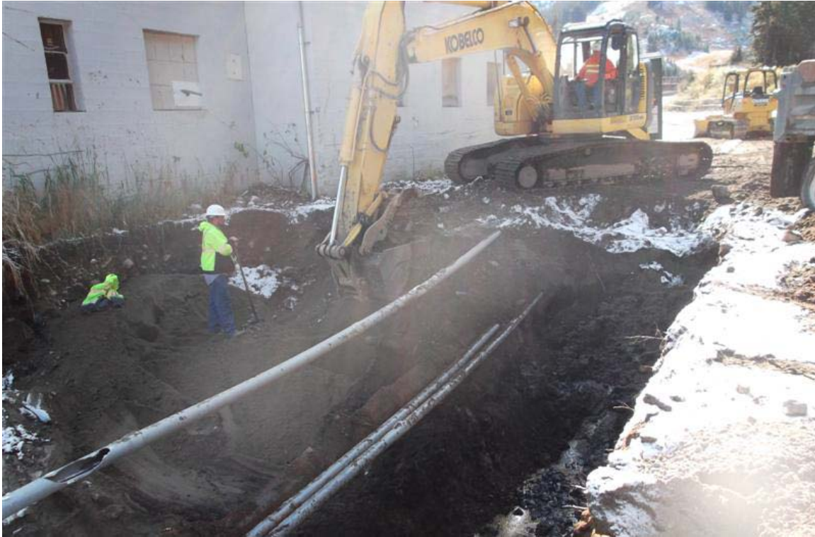
North to south view of southwestern part of northern Mini Mart area excavation.
