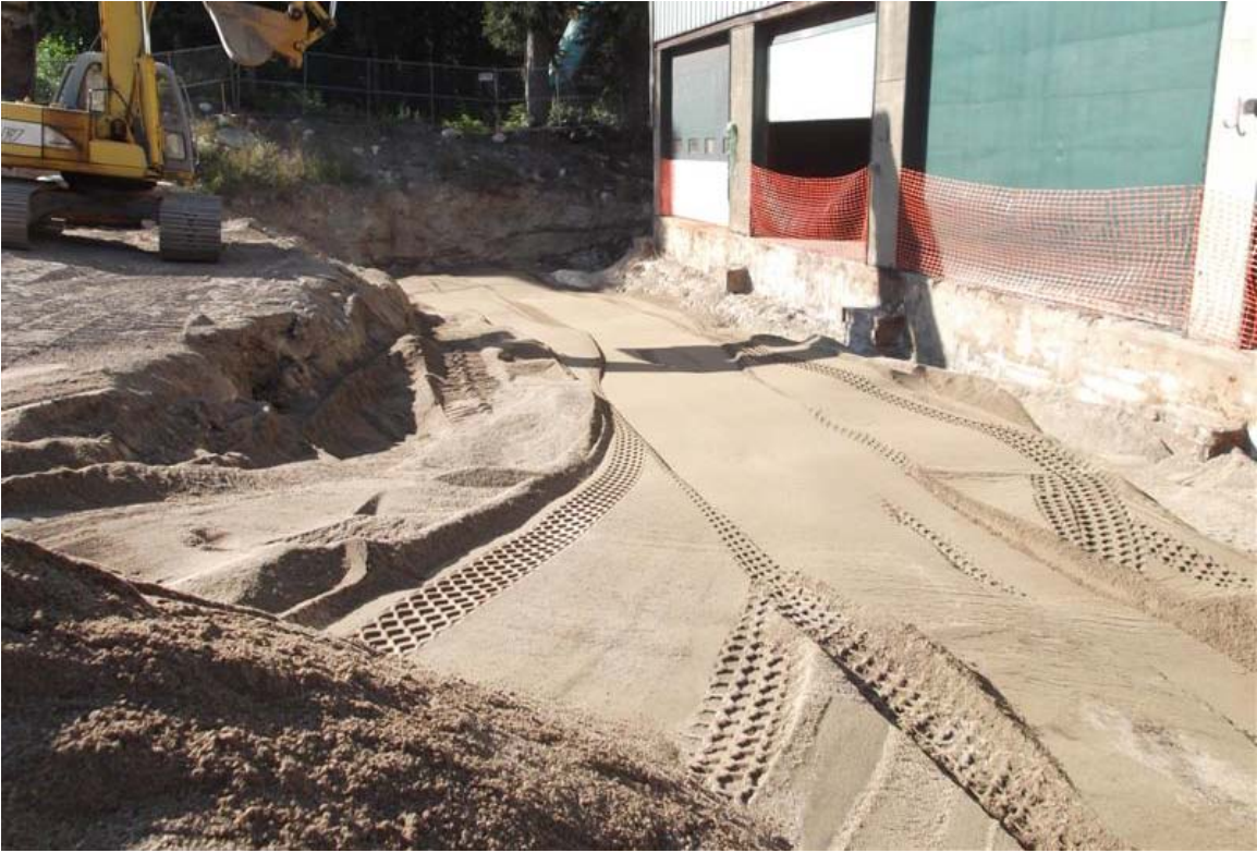
East to west view of backfilling of southern vehicle maintenance facility excavation.
