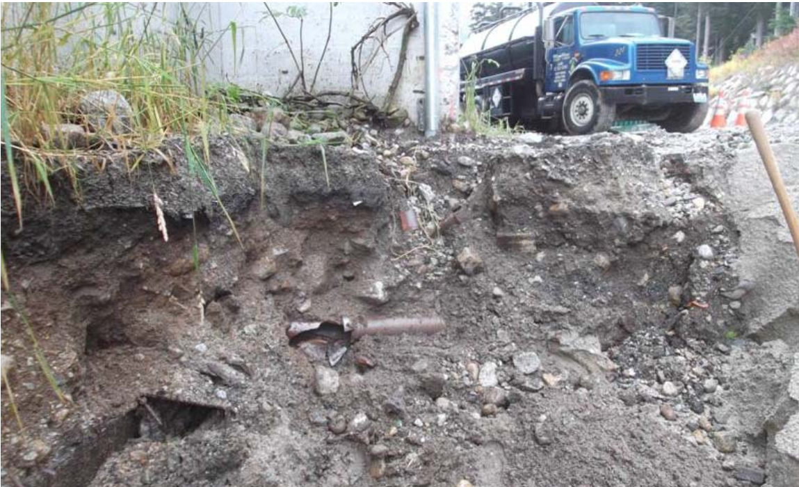
Northeast to southwest view of drain pipe that appeared to be the source of the impacted soil at the northern Mini Mart area excavation.
