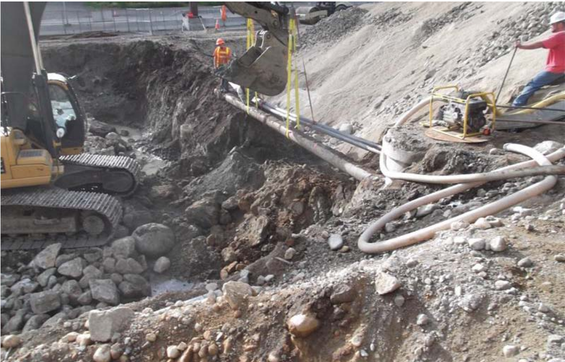
Northwest to southeast view of excavation of soil beneath a sewer line and electrical conduits.
