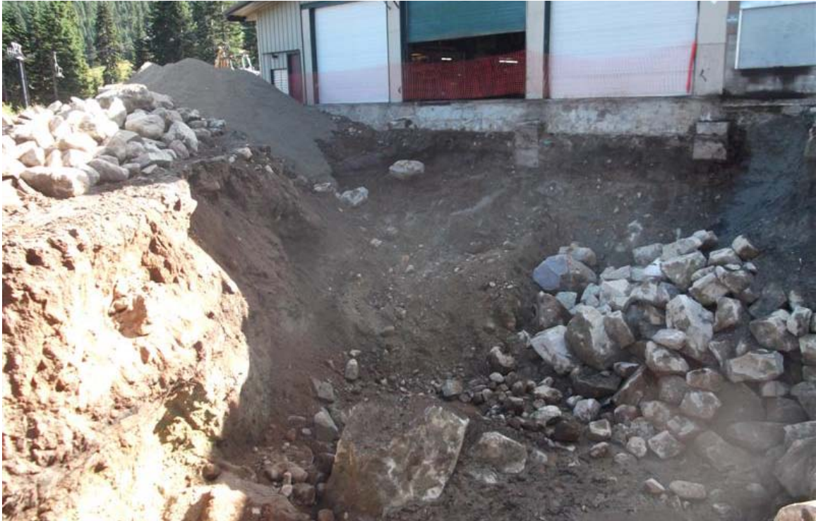
North to south view of eastern part of northern vehicle maintenance facility excavation.
