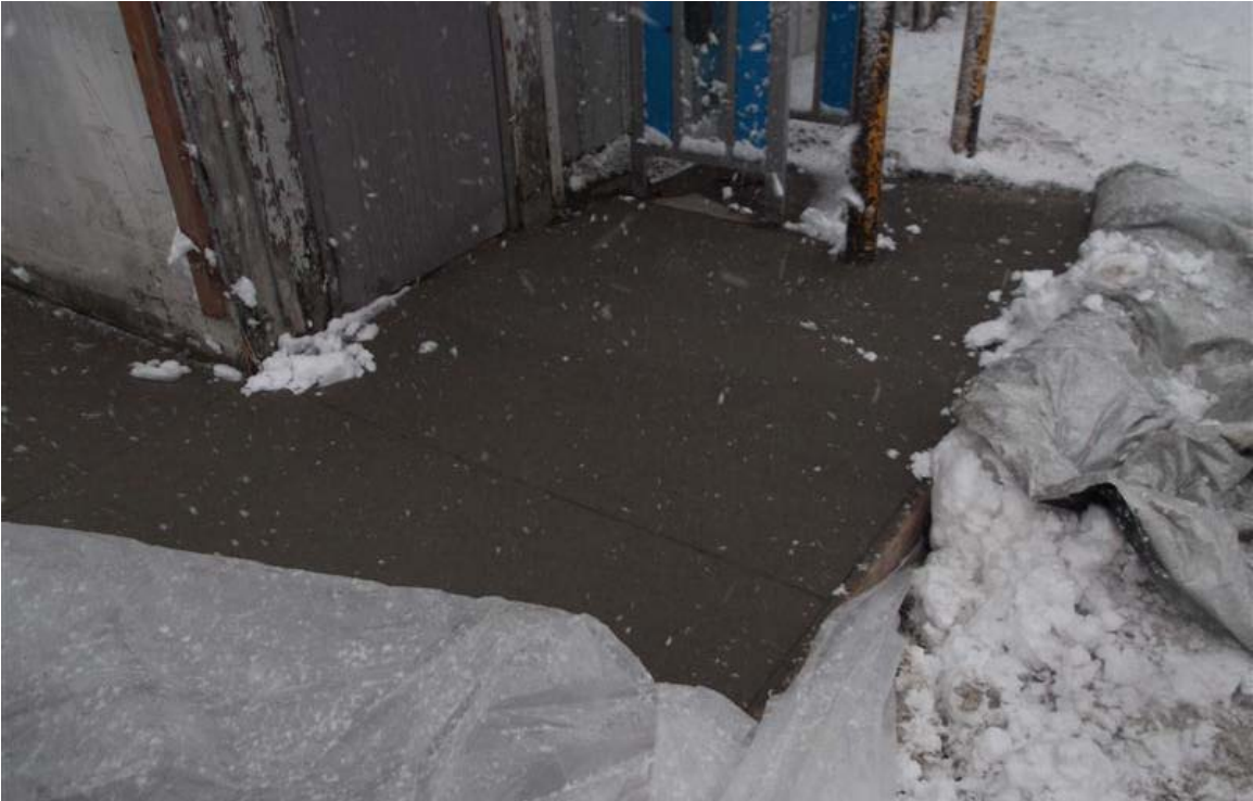
Eastern part of concrete surface cap near southeast corner of former maintenance building.
