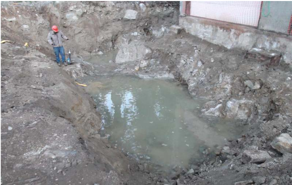
Extraction of groundwater from western and central parts of southern vehicle maintenance facility excavation.
