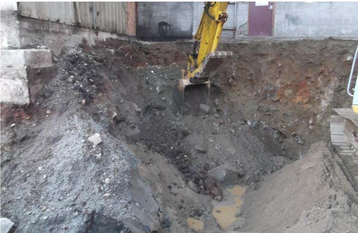
North to south view of excavation beneath former fuel dispensing shed adjacent to vehicle maintenance building.
