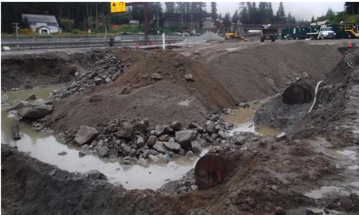
North to south view of northern part of southern Mini Mart area excavation. The central part of excavation is partially backfilled, and the 550-gallon USTs are on the right side of the photo.
