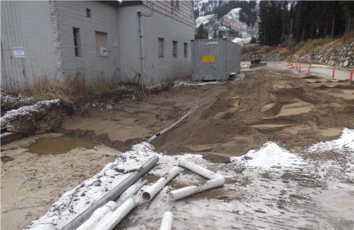
North to south view of backfilling of southwestern part of northern Mini Mart area excavation.
