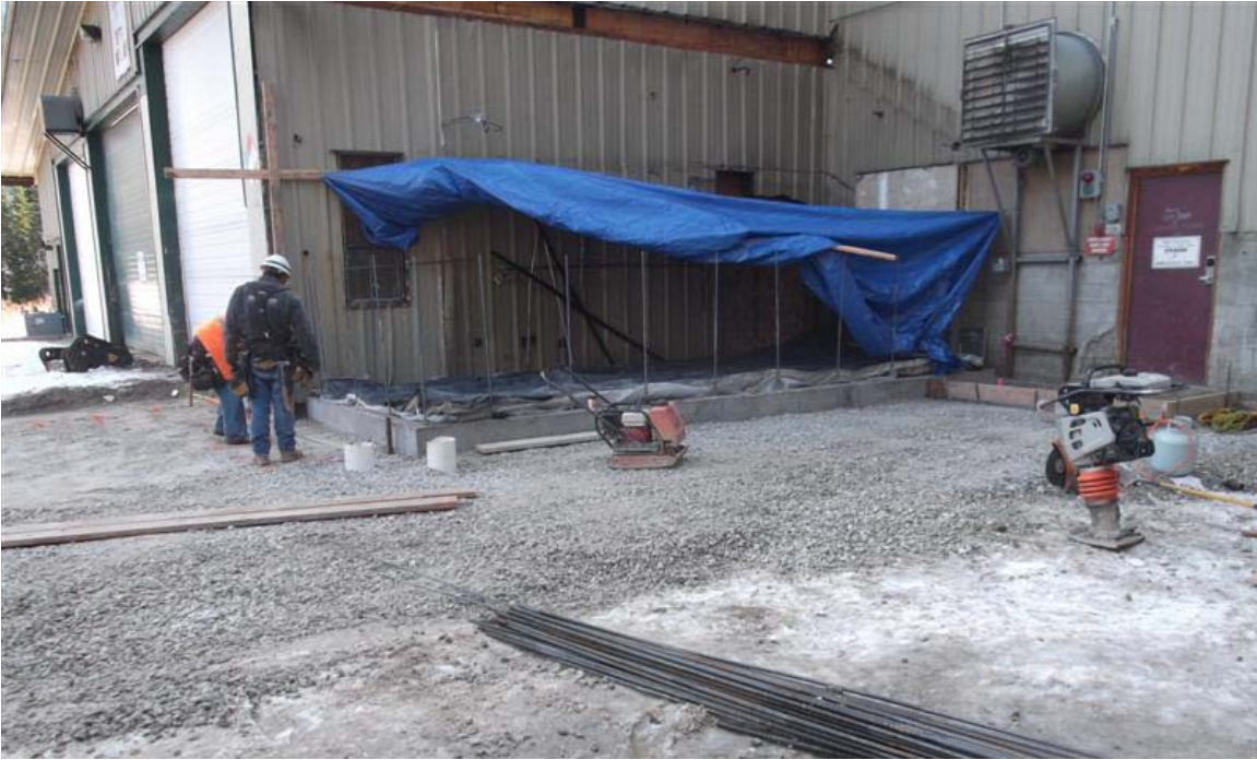
Construction of forms for concrete surface cap along north side of vehicle maintenance building, prior to rebuilding of shed.
