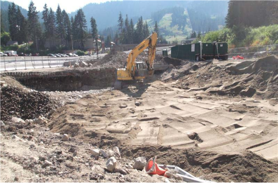
North to south view of backfilling of southern part of southern Mini Mart area excavation with finer-grained material.
