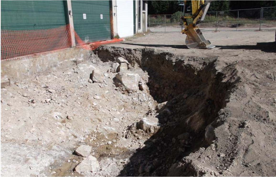
West to east view of eastern portion of southern vehicle maintenance facility excavation.
