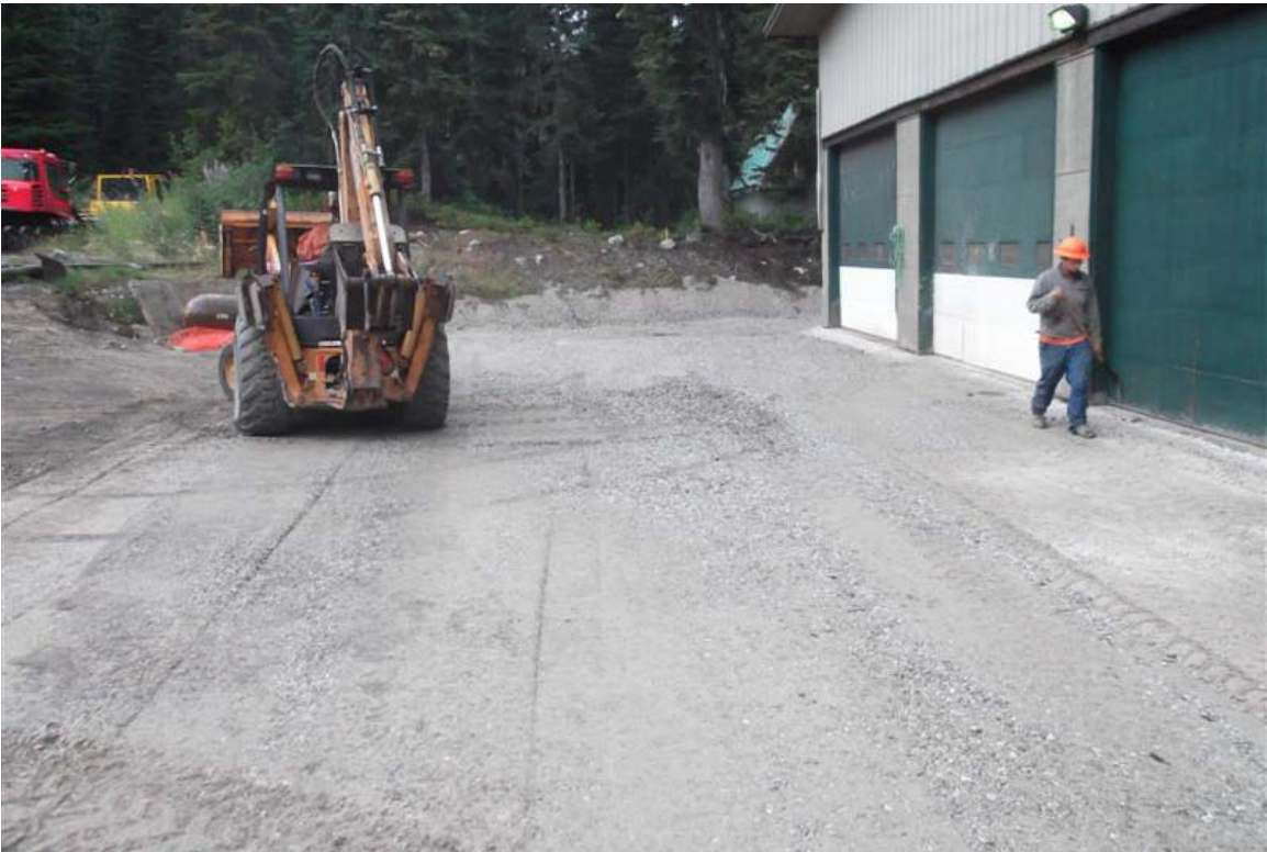
East to west view of southern vehicle maintenance excavation area after backfilling.
