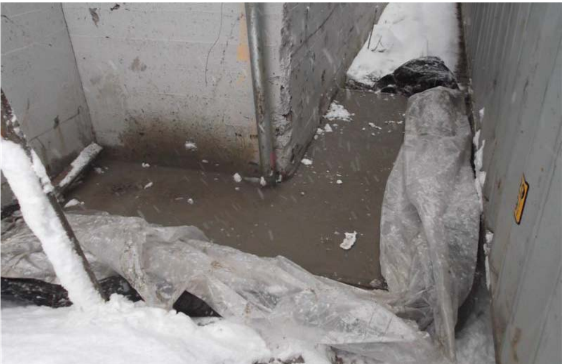
Concrete surface cap that wraps around the northern corner of the former maintenance building.
