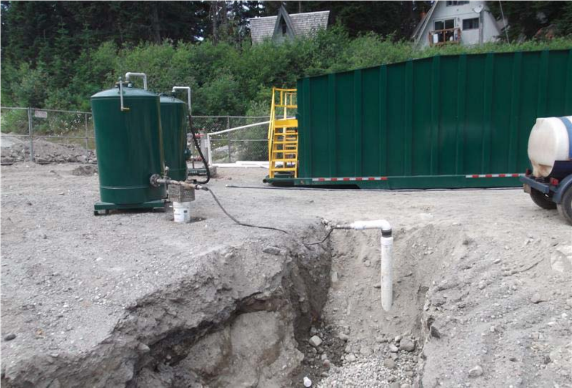
Groundwater treatment system and reinfiltration trench.
