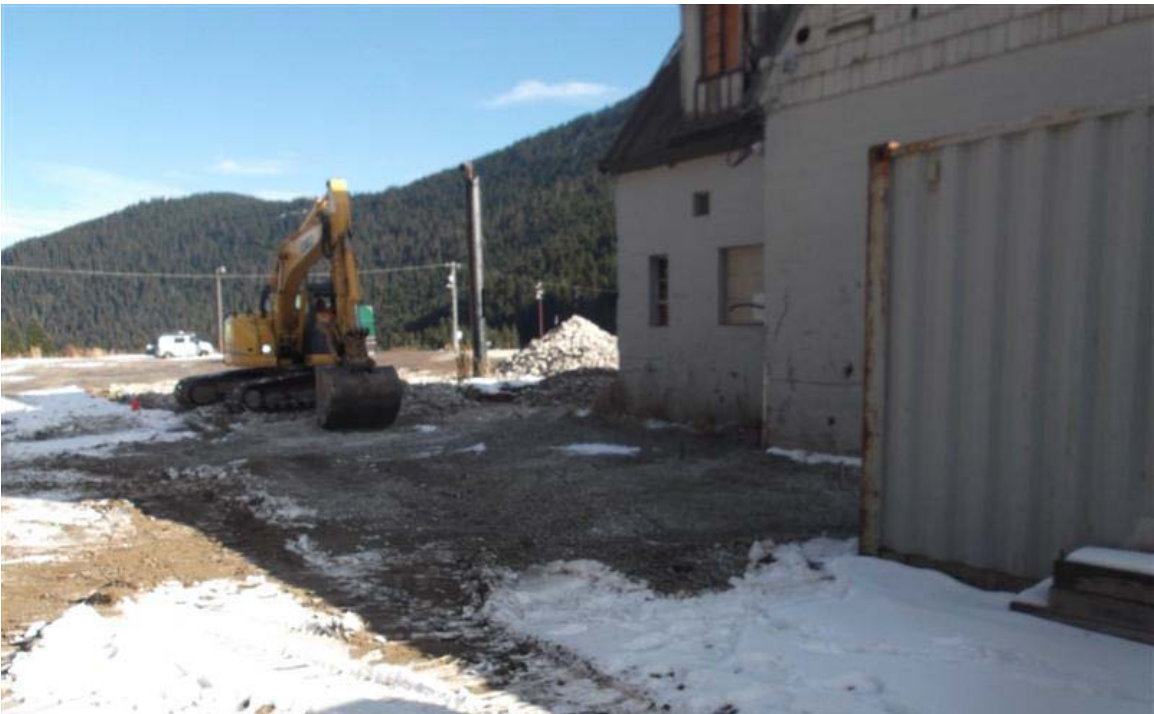
Southwest to northeast view of final backfilling of northern Mini Mart area excavation.
