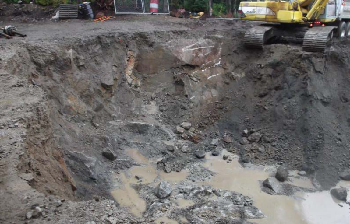
Southeast to northwest view of bedrock along western sidewall of northern vehicle maintenance facility excavation.
