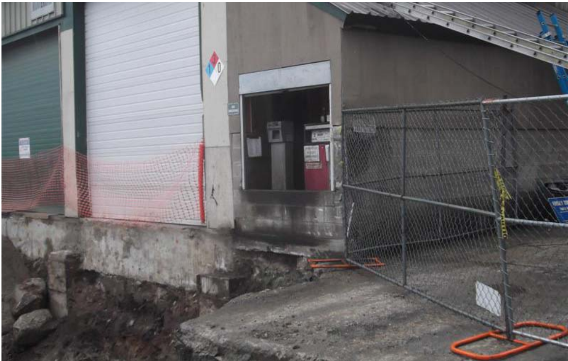
North to south view of fuel dispensing shed that was demolished in order to remove the USTs and the associated impacted soil.
