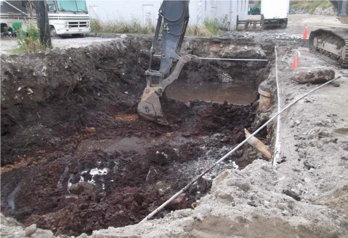
North to south view of northern and central portions of northern Mini Mart area excavation.
