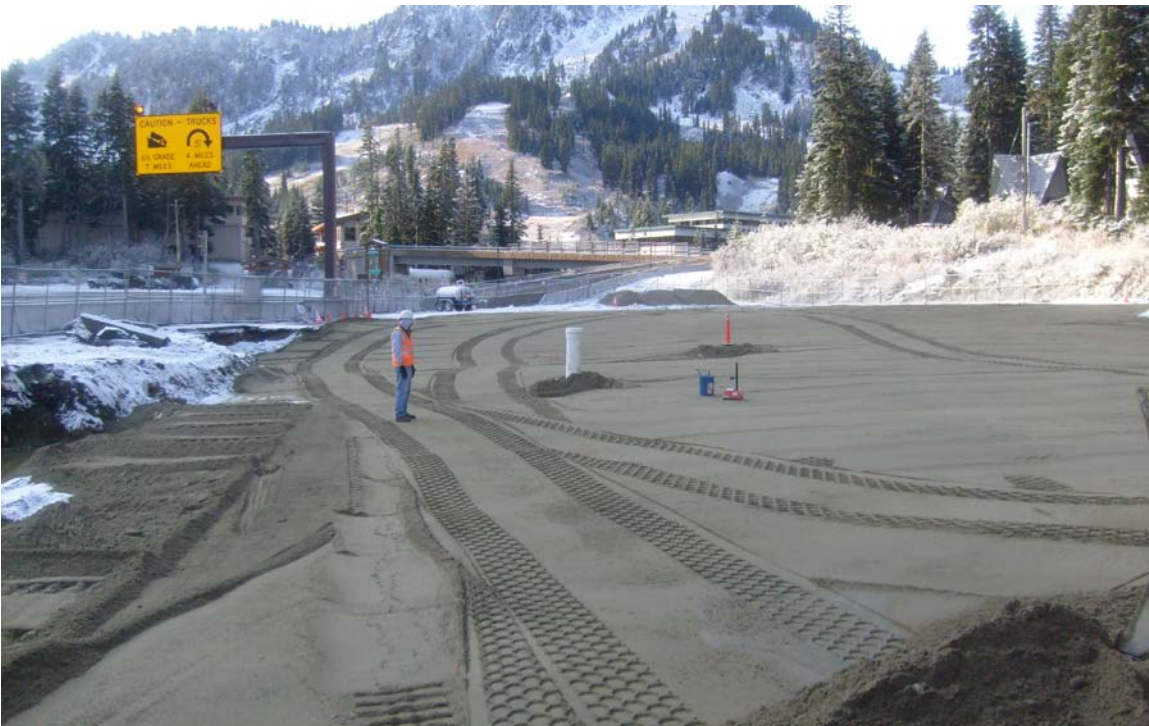
Northeast to southwest view of backfilling of southern Mini Mart area excavation. PVC pipe is for the installation of monitoring well SMW-4.
