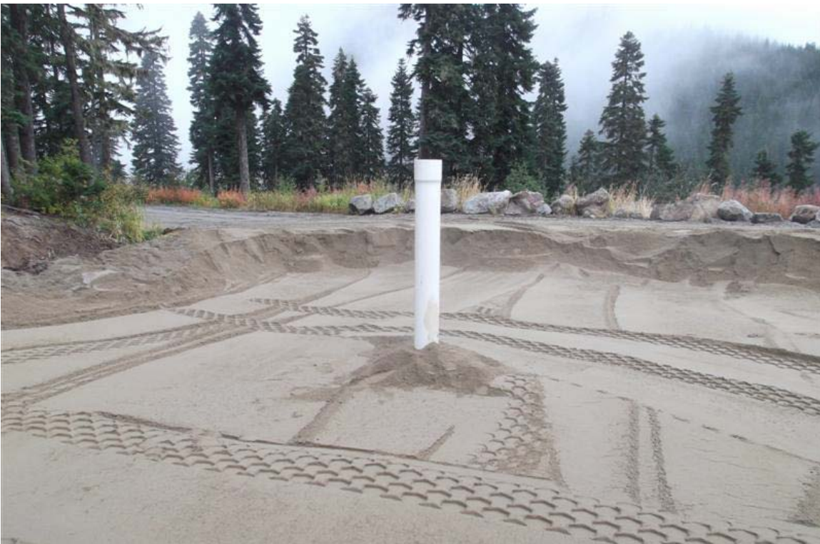
South to north view of backfilling of northern part of northern vehicle maintenance facility excavation. PVC pipe was used for the installation of monitoring well VMW-4.
