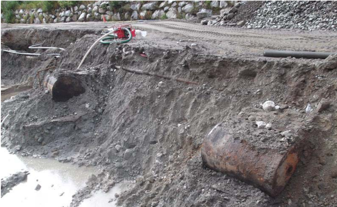
Northeast to southwest view of two 550-gallon USTs that were discovered in the northern part of the southern Mini Mart area excavation.
