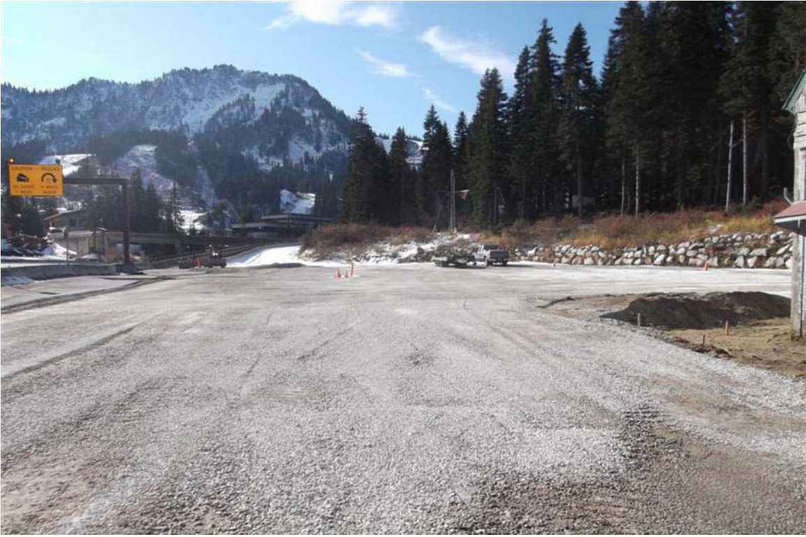
Northeast to southwest view of backfilled southern Mini Mart area excavation, prior to installation of concrete surface cap near south corner of former maintenance building.
