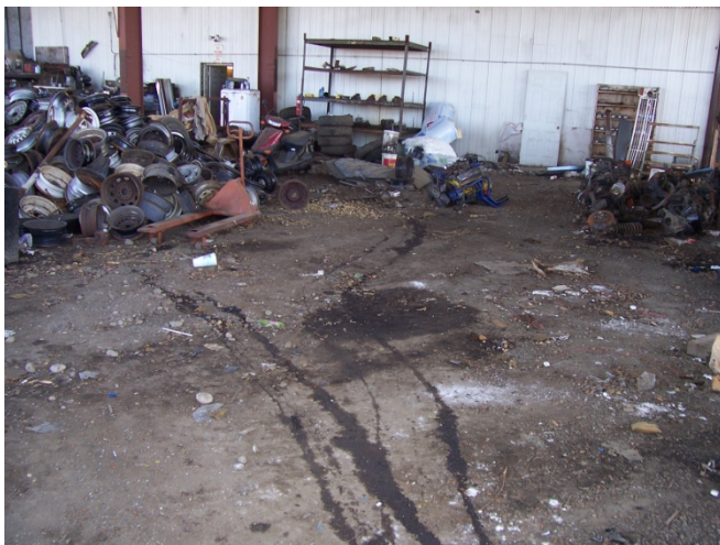
Photograph 5. Surface staining beneath former canopy
