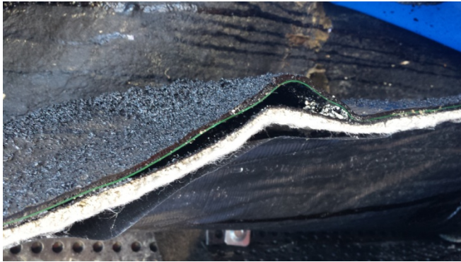
Photograph 19. Cross-sectional cut of sidewall vapor barrier. From bottom: black waterproofing, Voltex DSCR (gray-white layer), green VI-20 detailing fabric, and black Liquid Boot.
