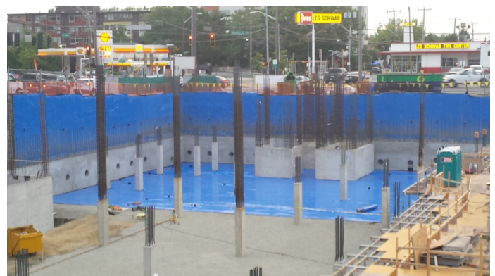
Photograph 24. Vapor barrier installation complete, with blue protective fabric installed to protect the barrier.
