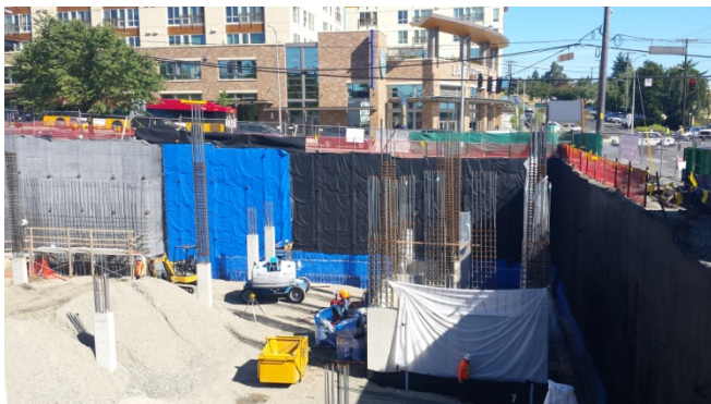
Photograph 17. Completed Liquid Boot on the upper level of the sidewall with blue protective fabric applied.
