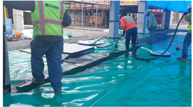
Photograph 20. Application of horizontal Liquid Boot layer over the detailing VI-20 fabric. Liquid Boot was sprayed between overlapping layers of fabric.
