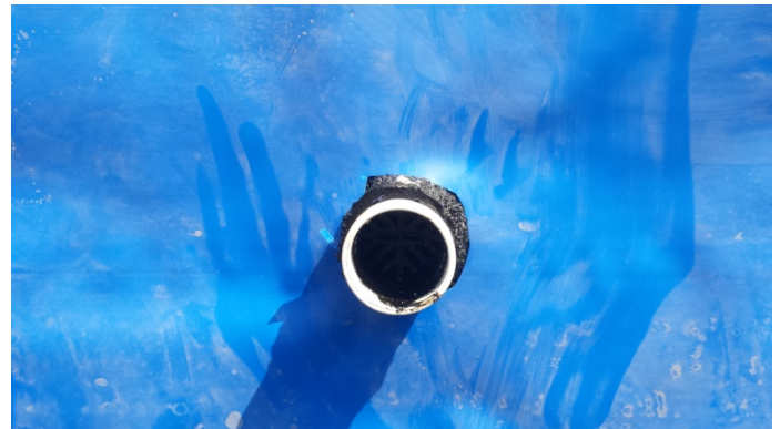
Photograph 16. Detail of piping through the vapor barrier, with Liquid Boot surrounding the piping.
