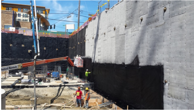
Photograph 13. Application of Liquid Boot vapor barrier on the eastern sidewall along the basement level. Not visible beneath the Liquid Boot is waterproofing Voltex DSCR and green detailing fabric (VI-20).
