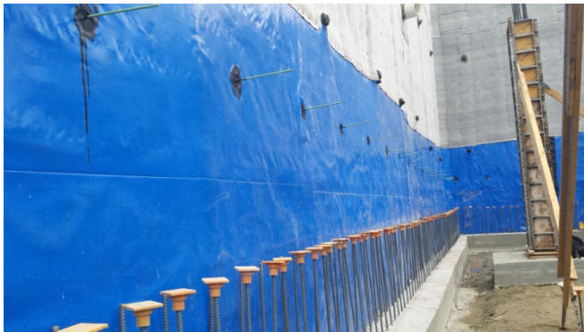
Photograph 15. Close up of detailing around intrusions through the vapor barrier on the northern sidewall, with blue protective fabric applied over the Liquid Boot to protect the Liquid Boot during concrete application.
