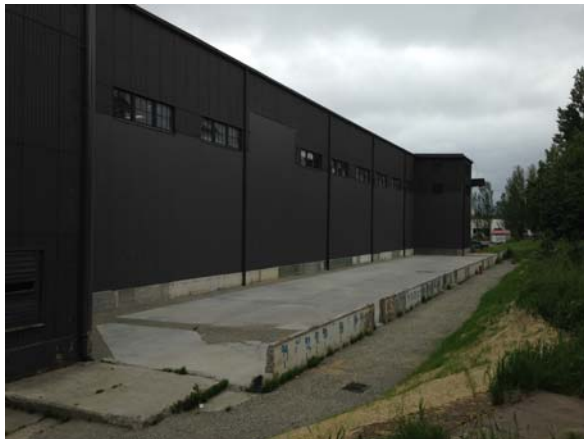
Final reconstruction of the south wall of Arena Sports after south shed (annex) removed.
