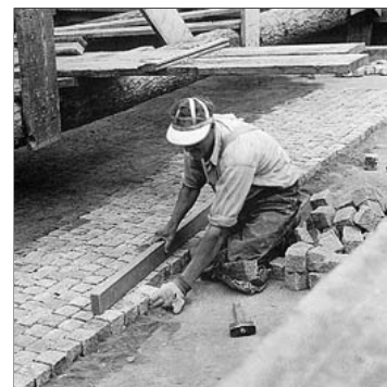
Laying granite blocks as part of runway, shop and storehouse construction, Sand Point, 1930 Courtesy United States Navy
