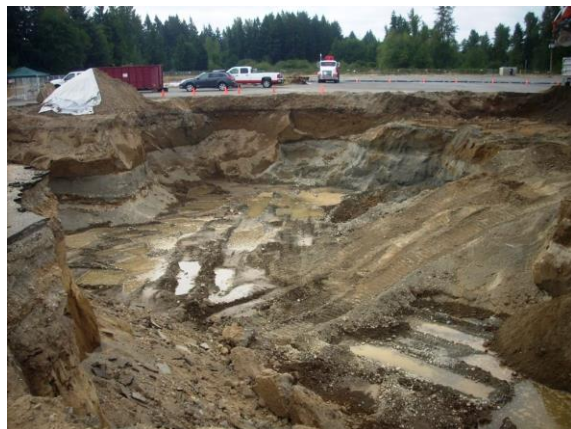
Photo #10: Excavation to depth of groundwater, some soils retained for reuse if not contaminated.
