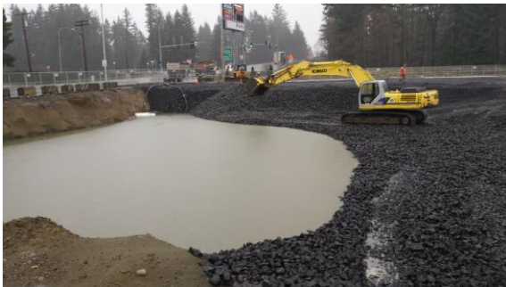
Photo #21: Casting spalls into water table
