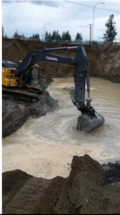
Photo #73: Scraping of overcompacted aquatard till at approximately 20 feet bgs. Removing top 6 inches with flat edged excavator bucket prior to spalls.
