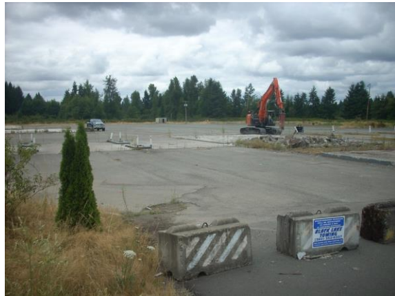
Photo #2: Looking southwest from UST area, store foundation in center by excavator.
