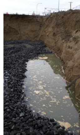
Photo #16: Rotary pump area for pump and treat system.
