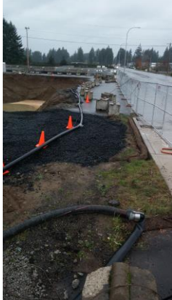
Photo #17: Pump inlet pipe background, discharge line foreground.
