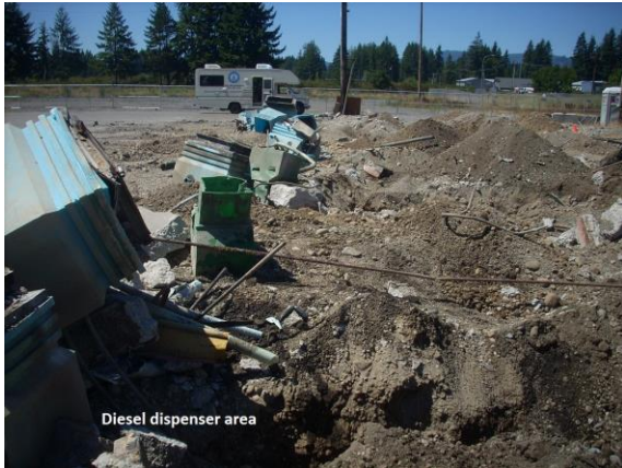
Photo #7: Diesel Dispenser containment and line exposure.
