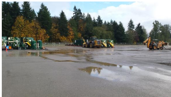
Photo #18: Groundwater treatment system, Carbon vessels and 6 pretreatment Baker Tanks on left, 3 post treatment, clean discharge tanks.
