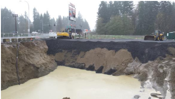
Photo #15: Backfill on eastern half of site. Looking East-northeast. Water level above spalls
