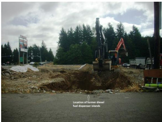
Photo #9: Removal of deeper soils beneath the dispenser islands to find lateral and vertical extents.
