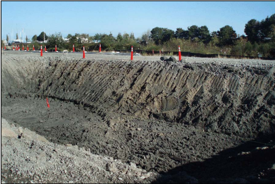
Figure 9. Overview of "Asphalt Warehouse" excavation location, depth at eleven feet below surface; view to the northeast.
