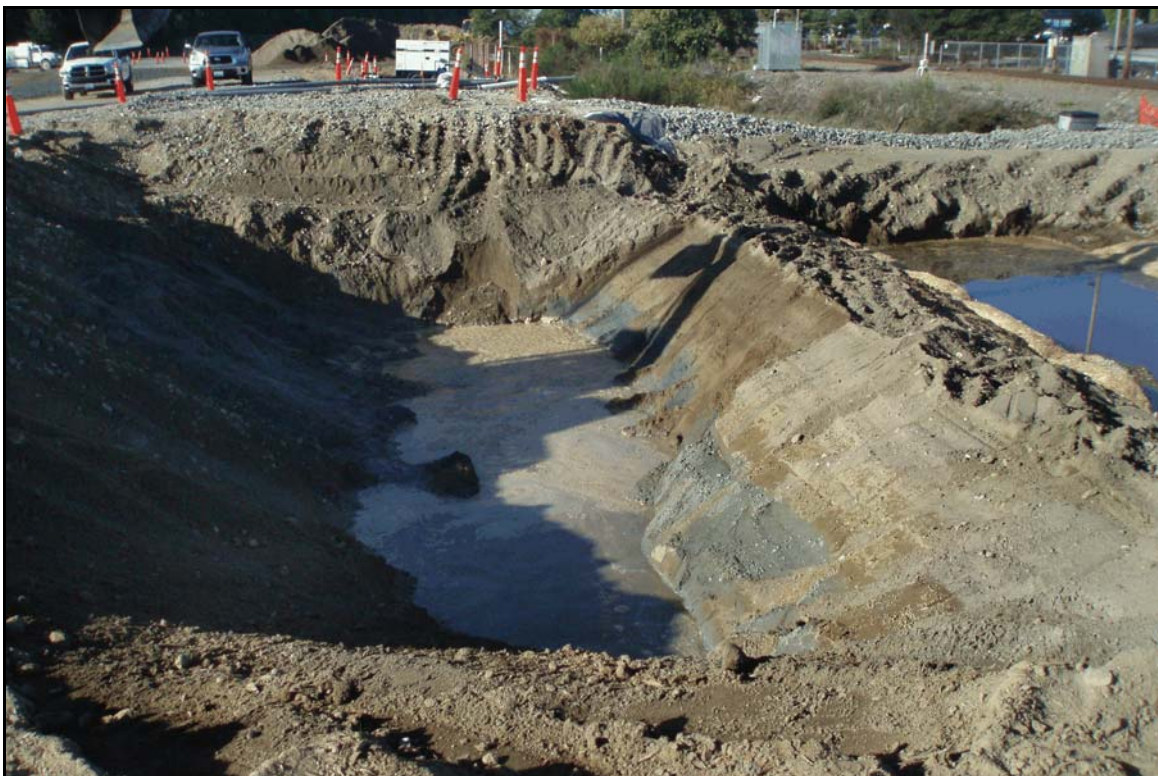
Figure 8. Overview of excavation at location B-9, depth at twelve feet below surface; view to the southwest.
