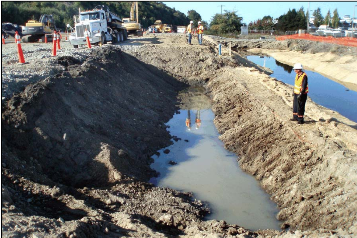
Figure 7. Overview of excavation at location B-8, depth at nine feet below surface; view to the south.
