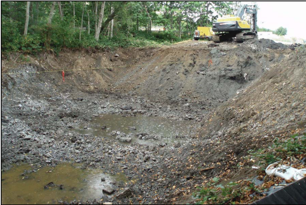
Figure 5. Overview of excavation at location B-1, depth at eleven feet below surface; view to the southwest.
