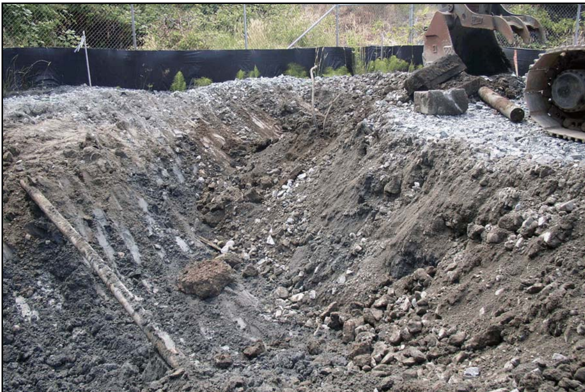
Figure 4. Overview of excavation at location B-19, depth at six feet below surface.
