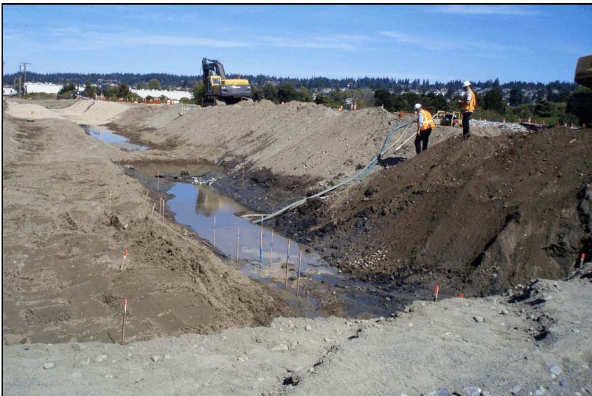
Figure 10. Overview of excavated Willow Creek, depth at twelve feet below surface; view to the northeast.
