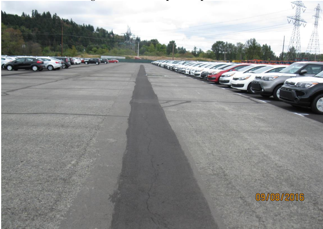
Photo 6: New Vehicle and Track Hoes Storage Area and the Asphalt Cap- from the north
