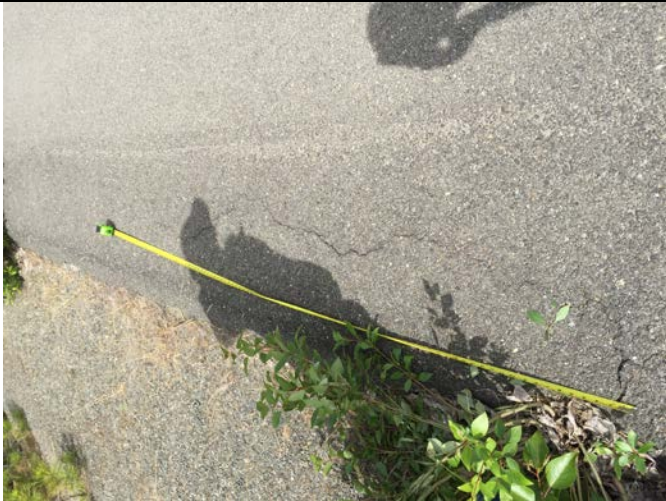
Photo 9: Crack parallel to northern edge of asphalt cap.
