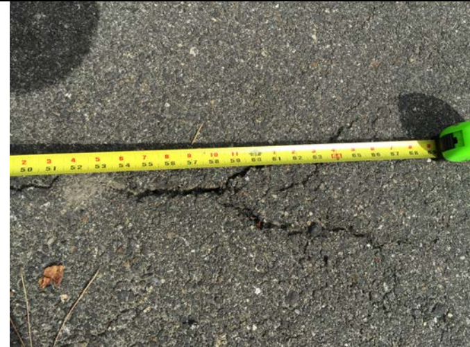
Photo 6: Close-up view of crack in northeastern corner of asphalt cap.
