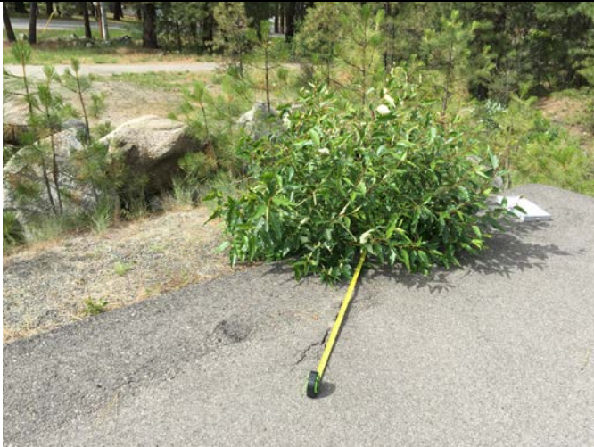
Photo 5: Crack in northeastern corner of asphalt cap. Cracks developing and elongating as a result of root expansion.
