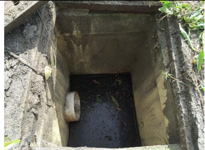
Photo 10: View of inside catch basing located on asphalt cap. Approximately 8" of water in vault.
