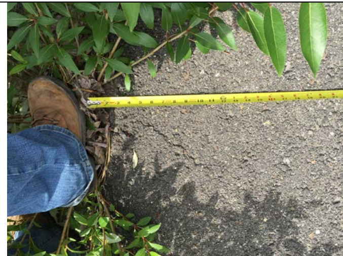
Photo 8: Crack developing in southeastern corner of asphalt cap.
