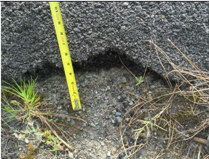
Photo 7: Close-up view of deteriorating eastern edge of asphalt cap at stairs down to MW-1.
