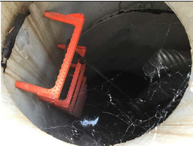
Photo 11: View inside grit chamber at cap.
