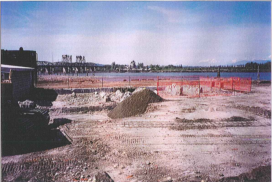
Area 7-2A Debris Removed to Concrete Slab and Initial Backfill (Looking North)
