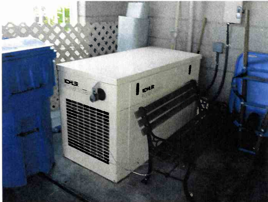
NATURAL GAS-POWERED EMERGENCY GENERATOR LOCATED NEAR THE NORTHWEST CORNER OF THE BUILDING. PHOTOGRAPH TAKEN FACING NORTHEAST.
