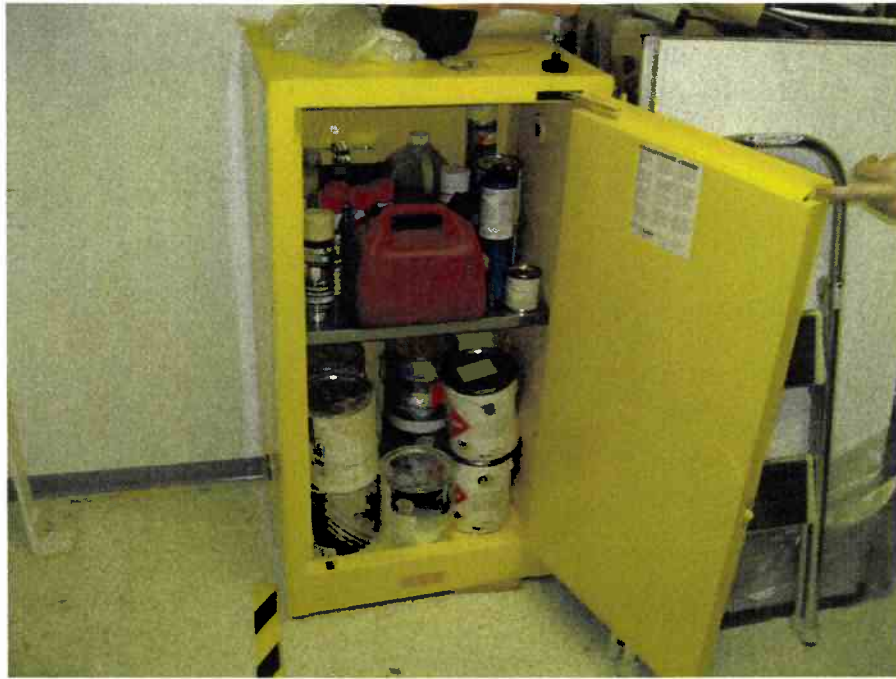
CHEMICAL STORAGE CABINET LOCATED IN THE SECOND-STORY MAINTENANCE ROOM. PHOTOGRAPH TAKEN FACING WEST.
