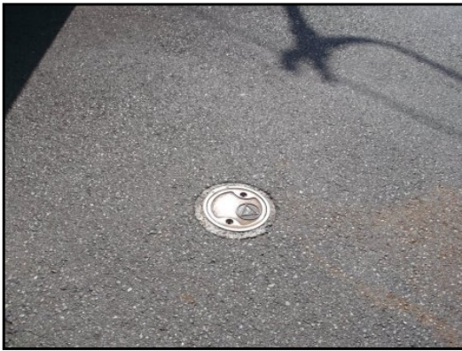
15 : Groundwater monitoring well
