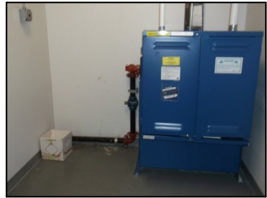
16 : Hydraulic elevator equipment
