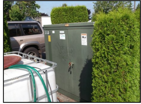
14 : Electrical transformer and remediation tote
