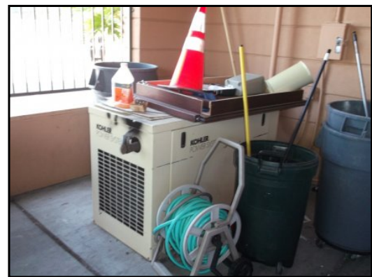
12 : Natural gas-fired emergency generator
