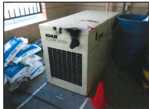
18 : Natural gas-fired emergency generator
