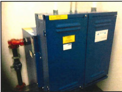
27 : Hydraulic elevator equipment
