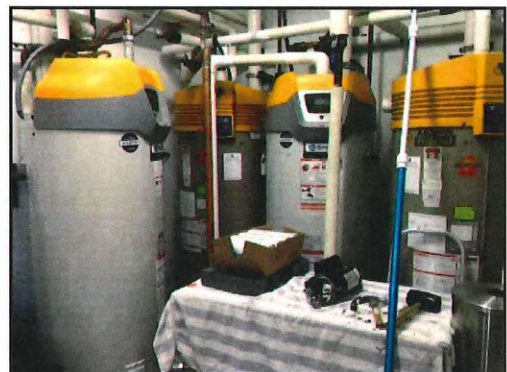
6 : Natural gas-fired water heaters
