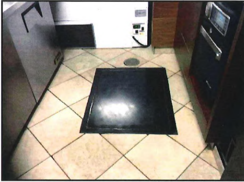
19 : Unused grease trap
