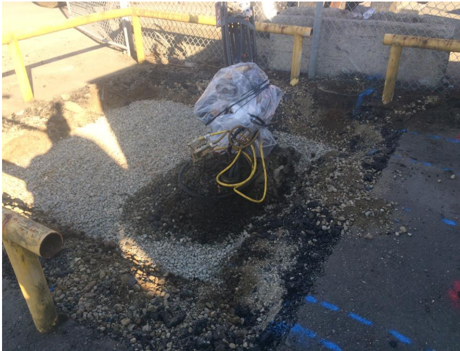
Figure 3: Impacted soils were constrained primarily to the area of the well pad.
