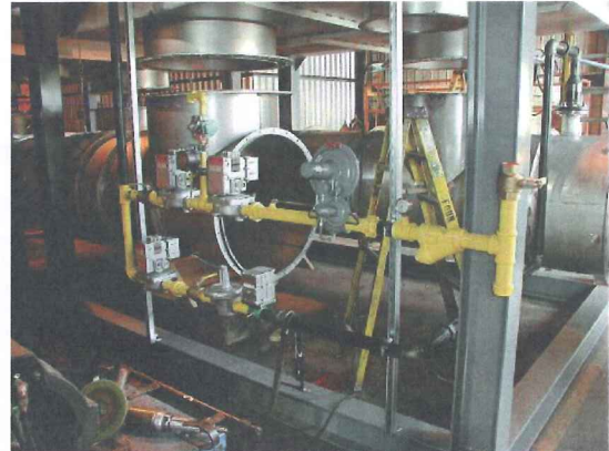
Supplemental Fuel Injection (SFI) Additional Fuel Train Piping
