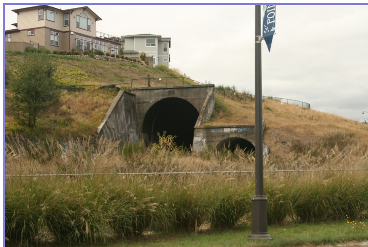
The tunnel on the right is the Ruston Tunnel, which the City of Ruston has filled with contaminated soil.
