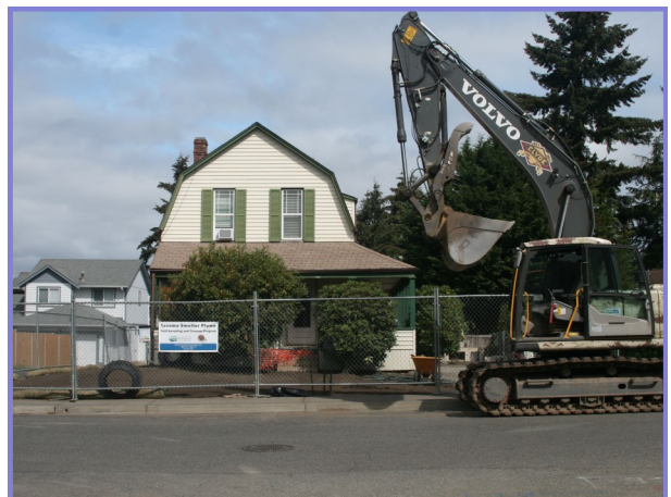
In most cases, we remove the top 12-18 inches of soil, then backfill and re-landscape the yard.
