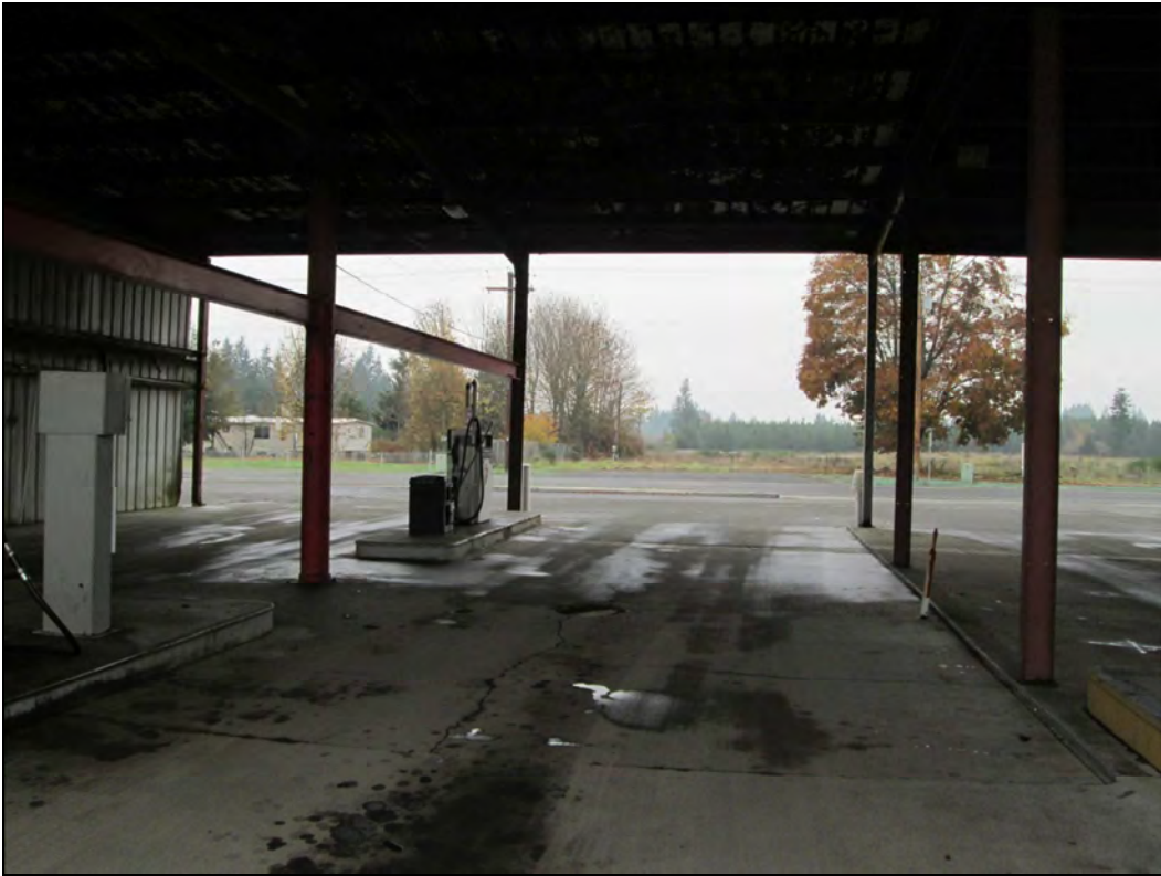
Fuel island and staining and disrepair
