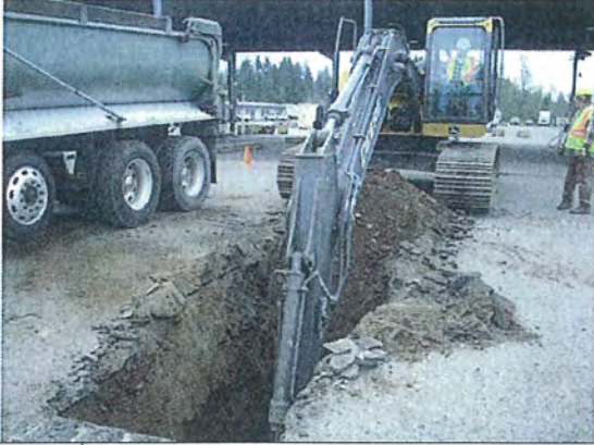
Photo #1: Excavating Soil at Location of Former Monitoring Well WDOE-6A (looking South)
