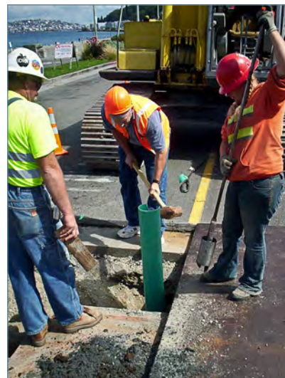
53rd Street Pump Station, Seattle, Washington
