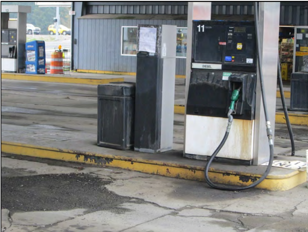
Staining on dispenser and concrete (note disrepair of concrete)
