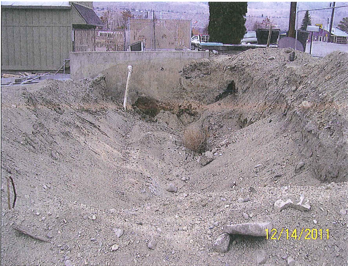
Lake Chelan Boat Company tank excavation December 14, 2011 Note areas of stained soil at far end
