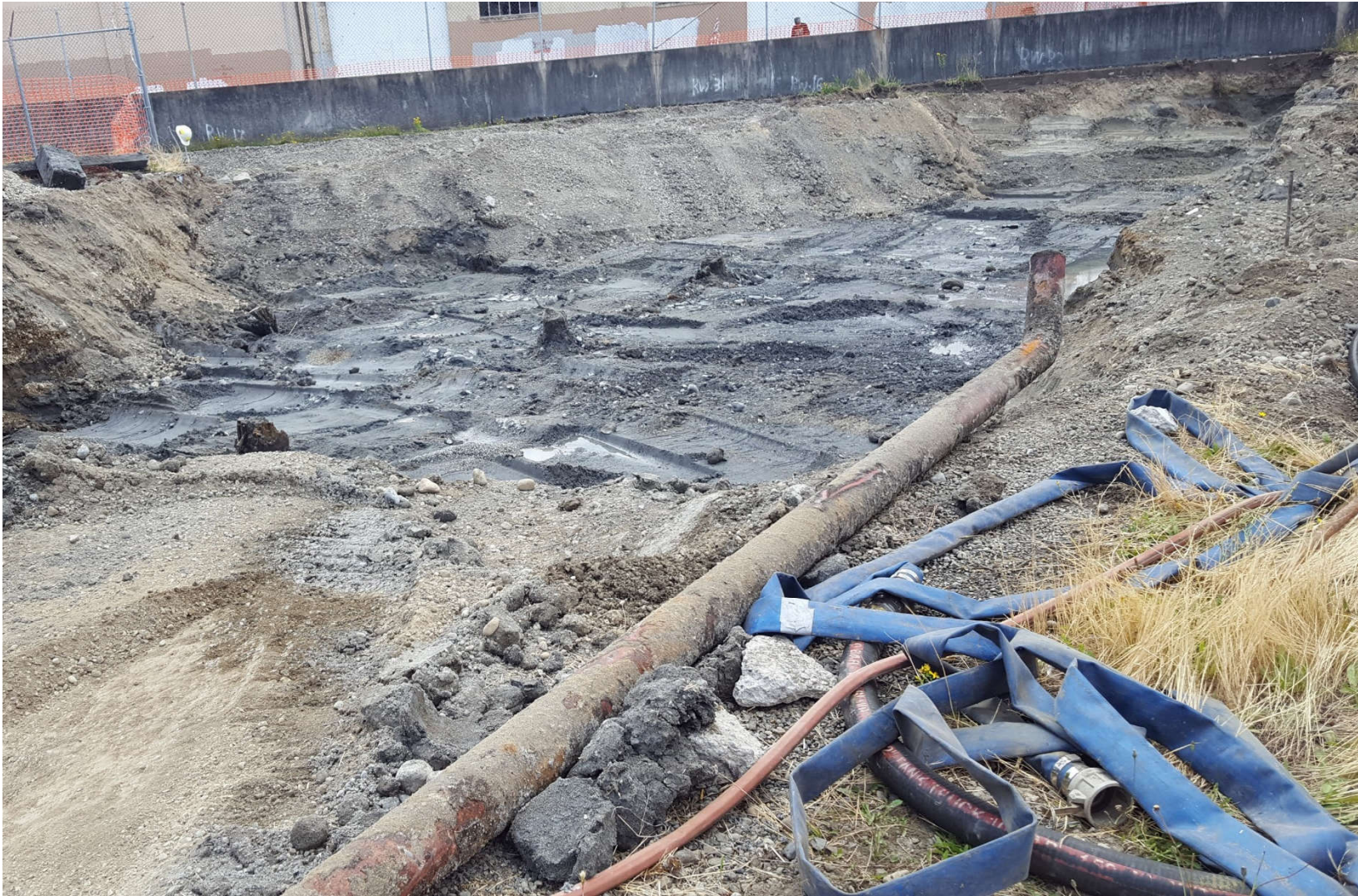
Photo #3: Day 2 of excavation. Progress made along the western edge of the Property. Approximate depth 3'.
