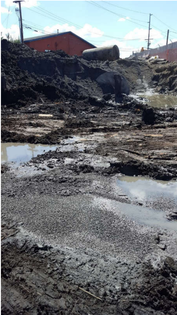
Photo # 11: Bottom of excavation pit Day 8. Total depth between 8-9 feet bgs. Extra one foot of soil was removed to expose clay layer.
