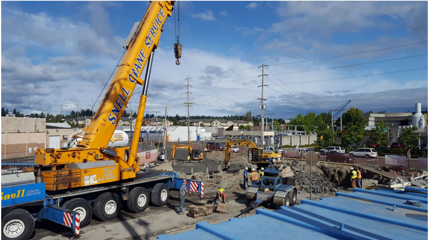
Photo # 16: Snell Crane Service brought in to remove the four, 8,000 gallon USTs.
