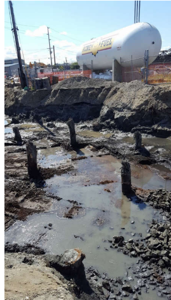
Photo #10: Beginning of backfill day 8 on the west side. Photo shows water sitting on top of clay layer.
