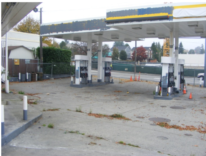
Photograph 1. The Alaska Street Texaco (SKS Shell) site prior to removal work, October 2013.
