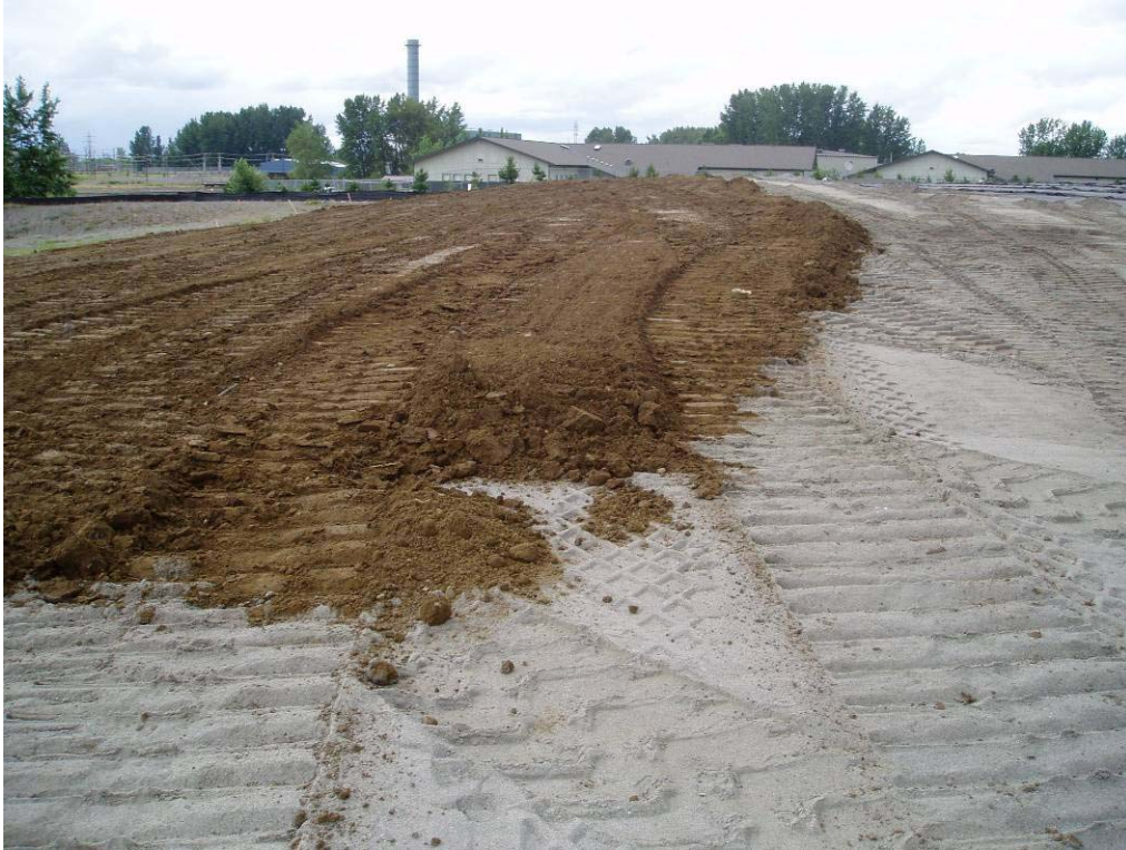
10127 June, 2004 – Spreading of 6-inch thick topsoil layer over 18-inch thick random fill layer. Both layers installed over geosynthetic layers. Looking north.
