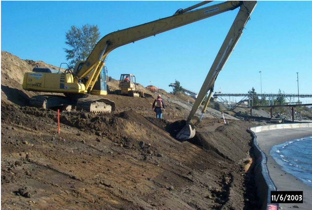
4169 November, 2003- Fill Placement activities along shoreline of Columbia River, in anticipation of 'Armorflex' installation. Note jersey barrier erosion fence along water's edge. Looking east.
