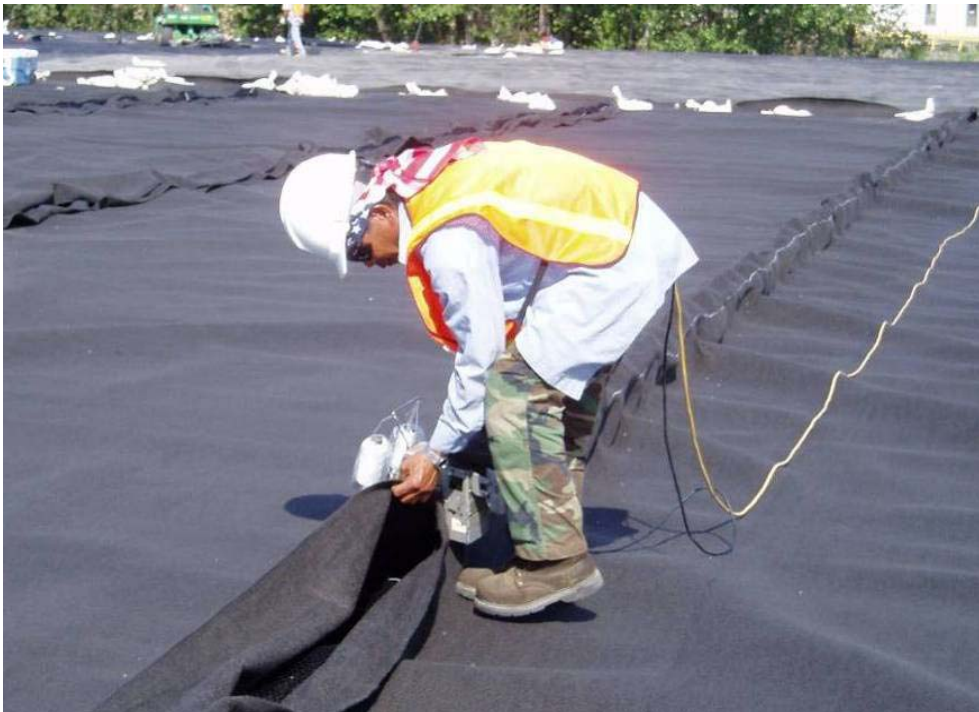
40185 June, 2004 – Field technician sewing adjacent panels of filter fabric seam bonded to synthetic drainage netting. White thread allows for quality control inspection.
