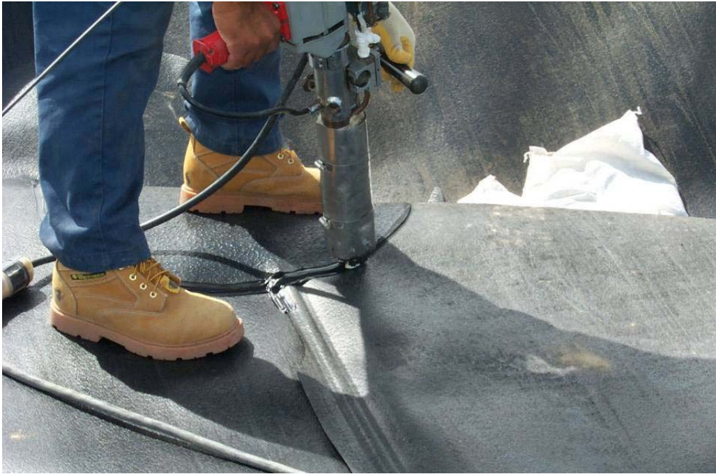
4506 May, 2004 – Extrusion fillet welding of a geomembrane patch adjacent to anchor trench. Left foot on patch. Extrusion fillet welding places ribbon of molten polymer over the edges of two geomembrane panels to be joined.
