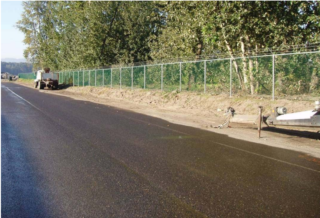
0218 October, 2004 Chainlink fence on east side of East Landfill property line, adjacent to Northwest Gateway Avenue. Looking south.
