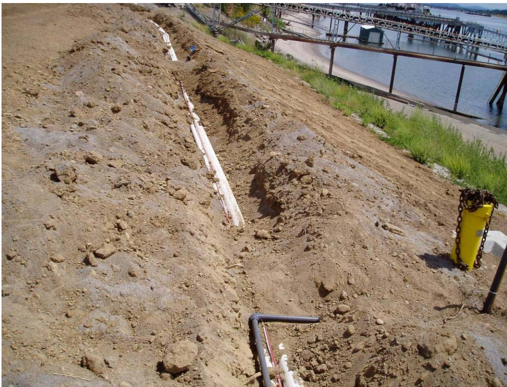
90007 July, 2004 – Installation of water pipeline and electrical conduit for sprinkler system along south embankment of East Landfill. Gray pipe is airline for use in monitoring well sampling. Looking east.
