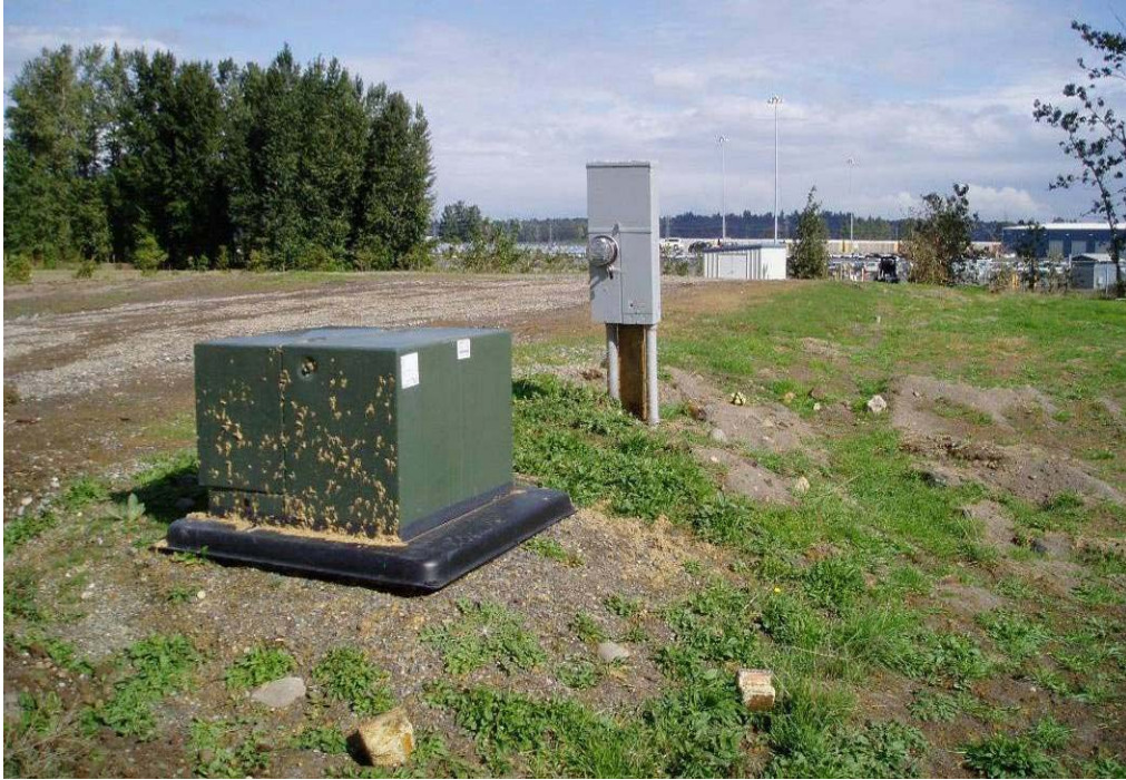
60066 August, 2004 – Electric transformer and power meter for sprinkler system. Storage-Operations building in background. Looking northeast.
