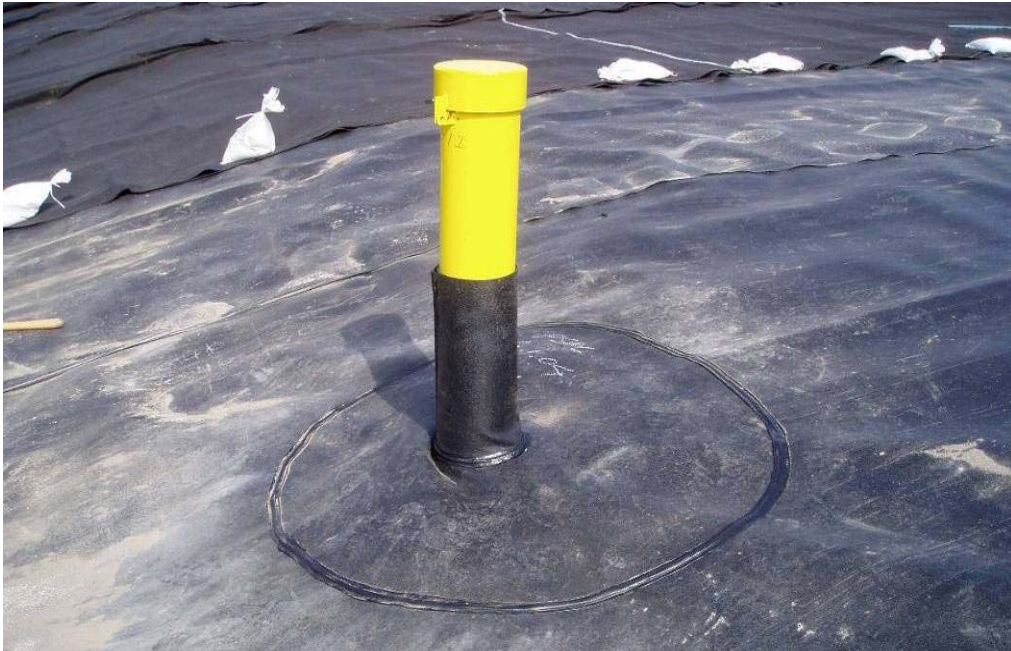
20140 June, 2004 – Completed installation of a 'boot' around a monitoring well. Boot is constructed using extrusion fillet welds, one at base of boot, one at patch over geomembrane and one vertical weld to create geomembrane column around well. Stainless steel straps secure boot to well casing.
