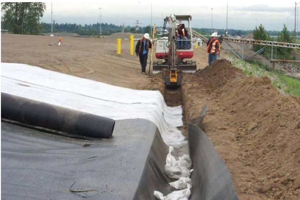
4521 May 2004 – Excavation of anchor trench on south side of East Landfill. HDPE geomembrane (black) and Geosynthetic Clay Liner (white) installed in conjunction with anchor trench excavation. Sandbags used to temporarily hold geosynthetics in place. Looking east.
