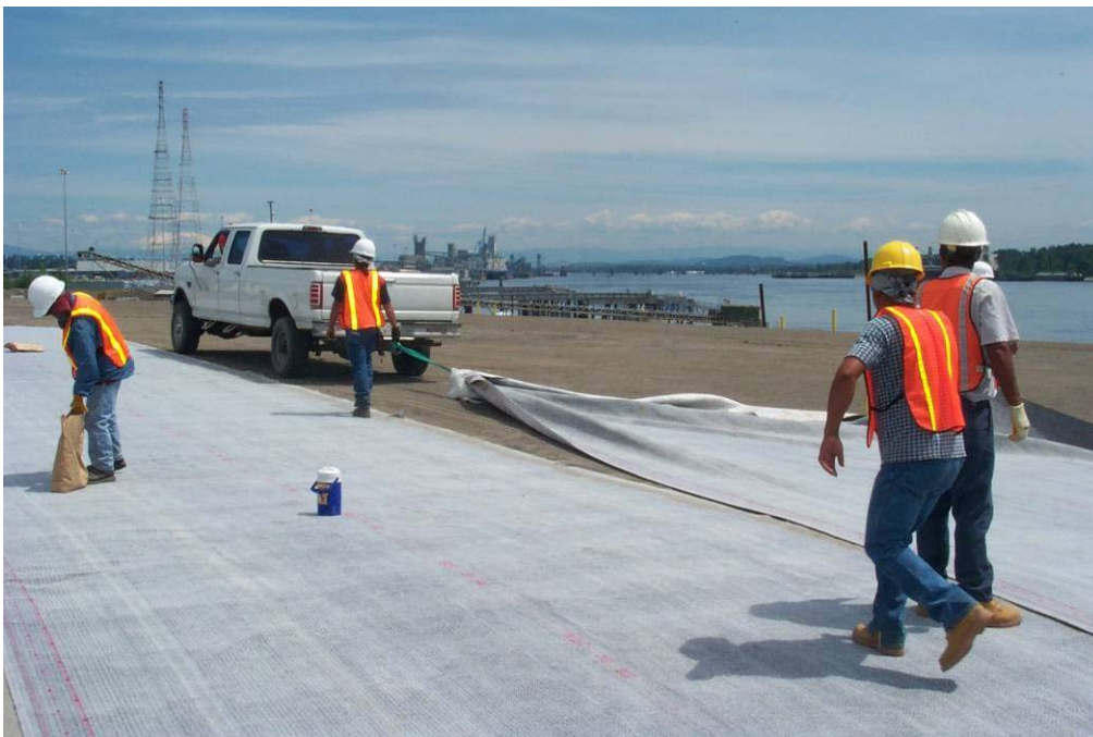
4486 May, 2004 – Placement of geosynthetic Clay Liner (GCL) over prepared soil surface of East Landfill. Looking southeast.
