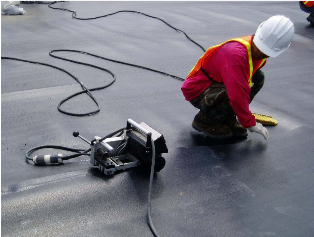
50079 May 2004 – Field Seaming of adjacent geomembrane panels. Operator removes fine debris from top and underside of geomembrane with brush to ensure quality seam.
