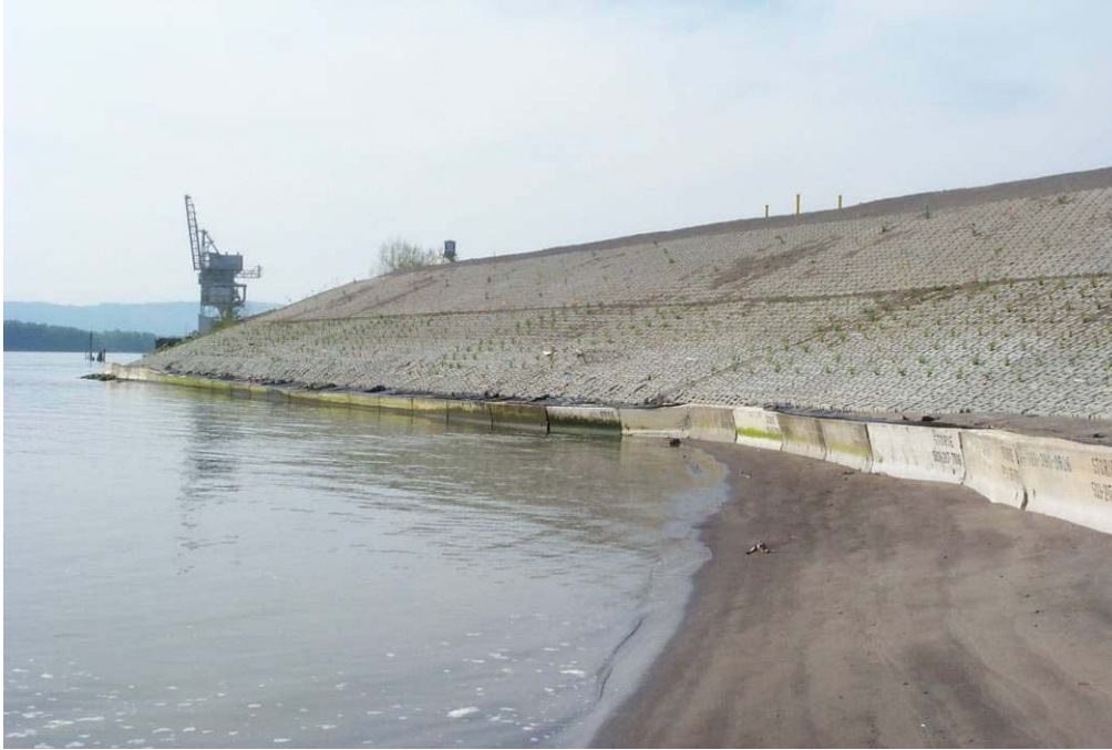
4348 April, 2004 – Completed 'Armorflex' installation. Note jersey barrier erosion fence along waters edge, used for erosion and sediment control. Looking northwest.
