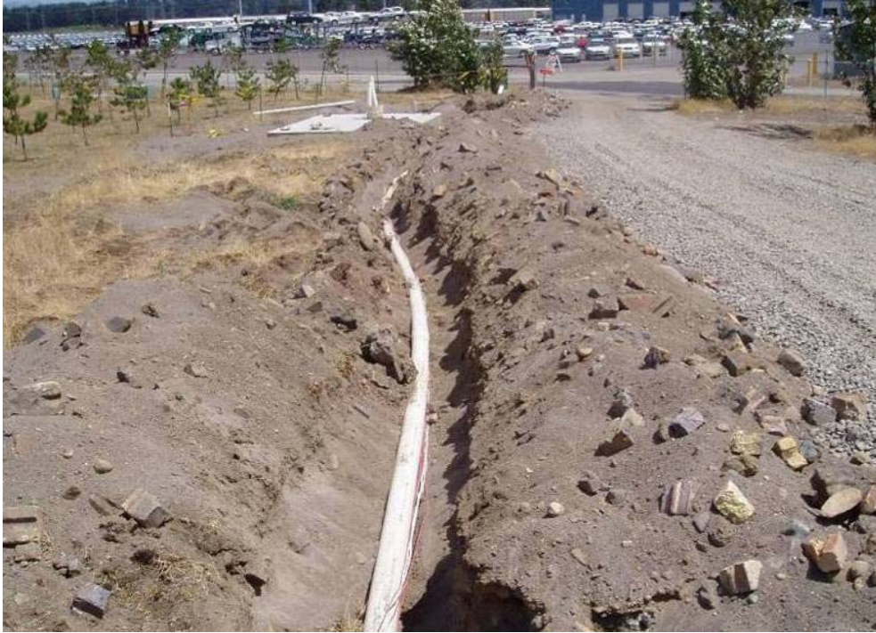
90002 July, 2004 - Installation of water pipeline and electrical conduit for sprinkler system. Lines extending from northeast corner of East Landfill (foreground) to storage-operations building foundation (background). Looking northeast.
