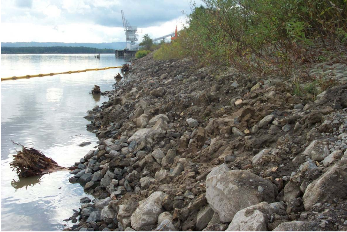
015 October 17, 2006 – Completed riprap toe repair. Note rootwad to left of picture and gravelly soils from bench area excavation infilling larger riprap. Looking east.
