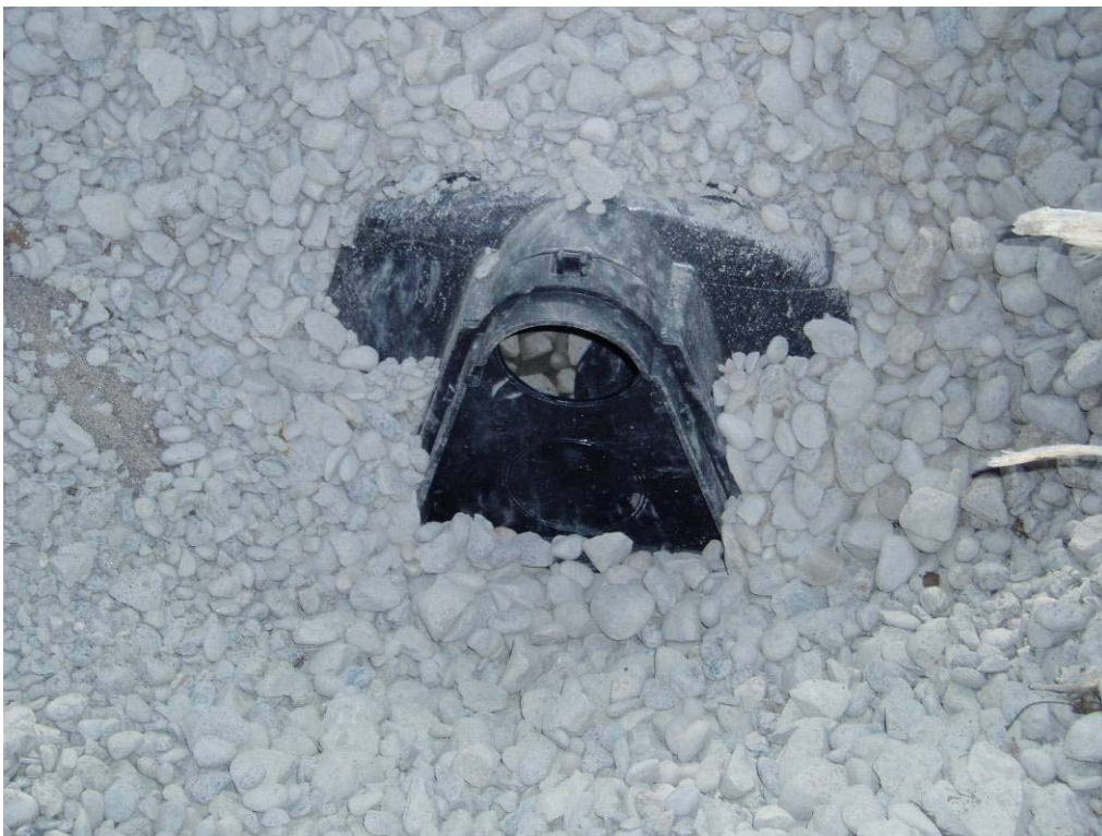
30148 June, 2004 – Biodiffuser unit with gravel backfill.
