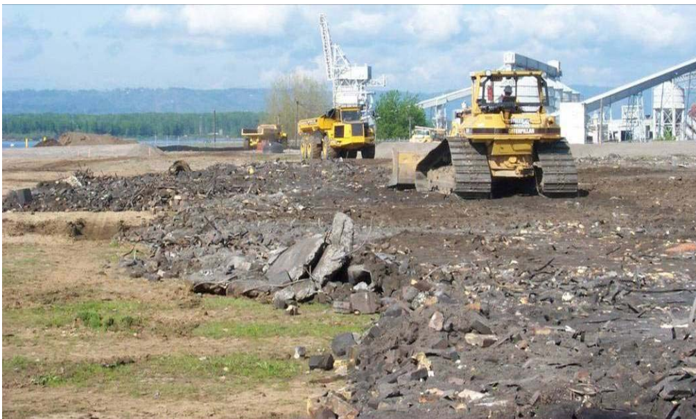
4320 April, 2004 – Spreading of 'Waste Soils' on surface of East Landfill, northeast corner. Waste Soils obtained from North2 Landfill. Looking west.
