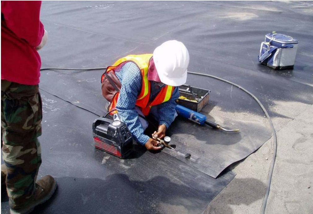
50082 May 2004- Field technician checking weld using pressurized dual seam process. The 1/4-inch wide air channel created by dual wedge weld is pressurized to approximately 30 psi and monitored for pressure loss for 5 minutes.
