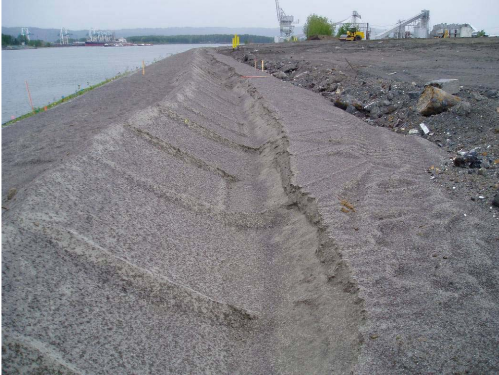
90054 April, 2004 – Construction of anchor trench embankment along south side of East Landfill. Note Waste Soils previously placed to right. Looking west.
