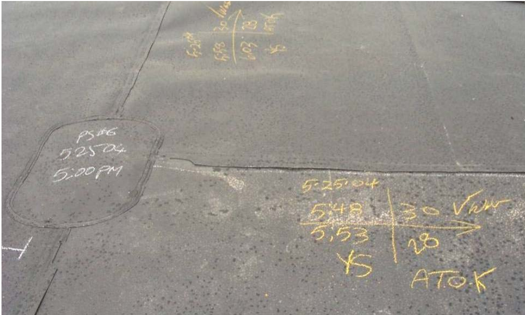
4512 May, 2004. Typical quality control inspection information. To right is inspection of welded seam. Information shown includes date, time and pressure to start test, time and pressure at end of 5 minute test, inspector initials and 'Air Test OK' To left is patch over destructive test sample location with extrusion fillet weld. Operator initials, date and time are provided.
