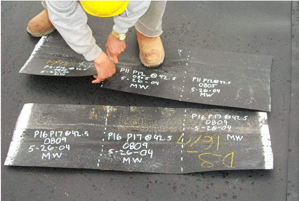
4518 May, 2004 – Destructive test samples cut and removed from HDPE geomembrane after welding process completed. Information on sample includes panel location, date, time and welding operator initials. One sample tested infield, one sample tested at approved off-site lab and one sample archived by Alcoa. Peel and shear tests conducted and compared to minimum requirements of manufacturer specifications.
