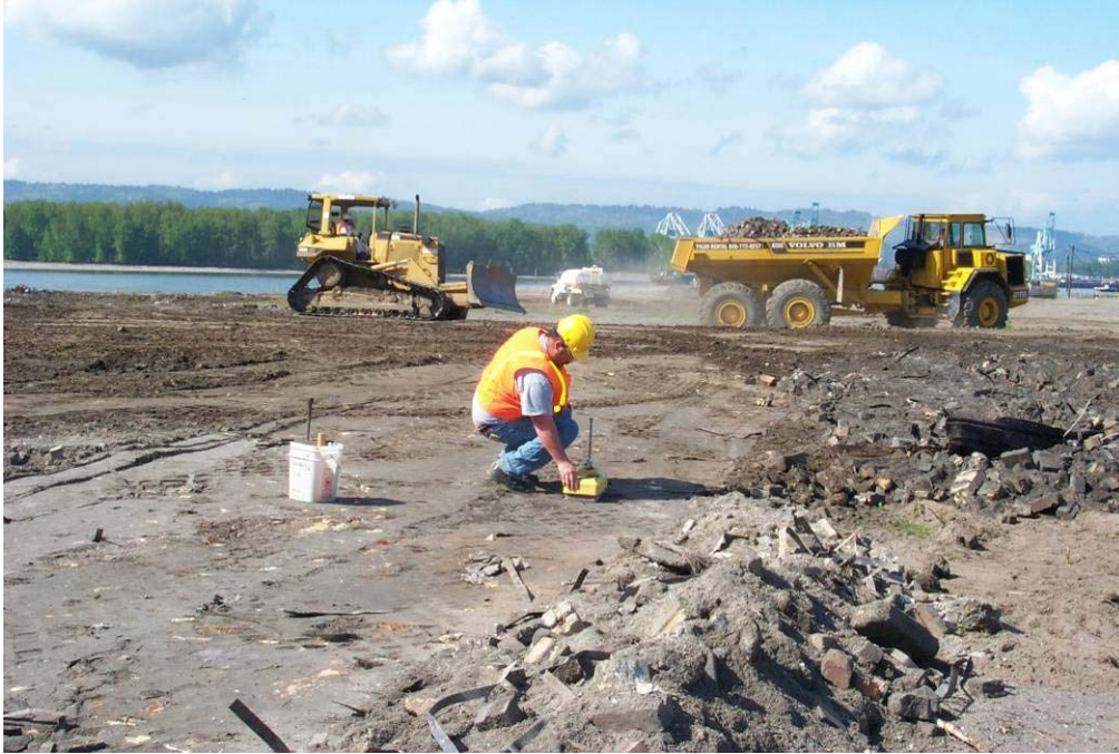
4326 April, 2004 – Density testing of 'Waste Soils' on East Landfill. Due to variability of soil makeup, a test fill was constructed to optimize compactive effort.
