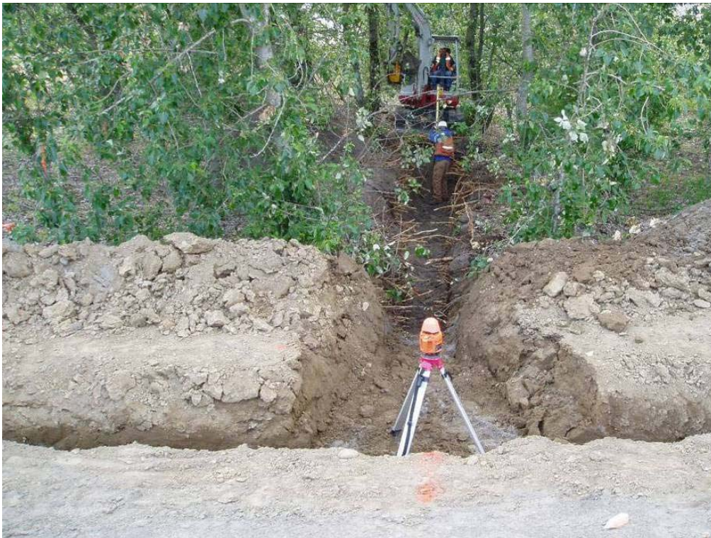
20120 June, 2004 – Excavation of Biodiffuser trench on east side of East Landfill. Perimeter anchor trench in foreground, perpendicular to biodiffuser. Looking east.
