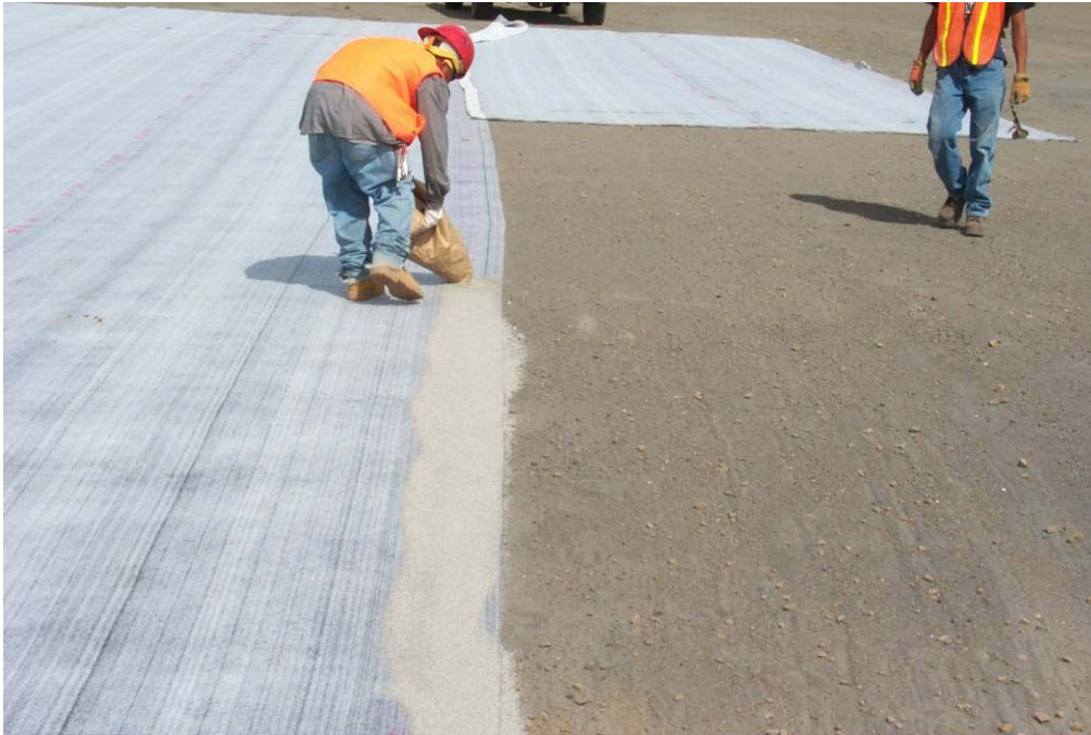
4501 May, 2004 – Application of a bead of bentonite prior to installation of adjacent Geosynthetic Clay Liner (GCL) panel. Bentonite bead required per specifications.
