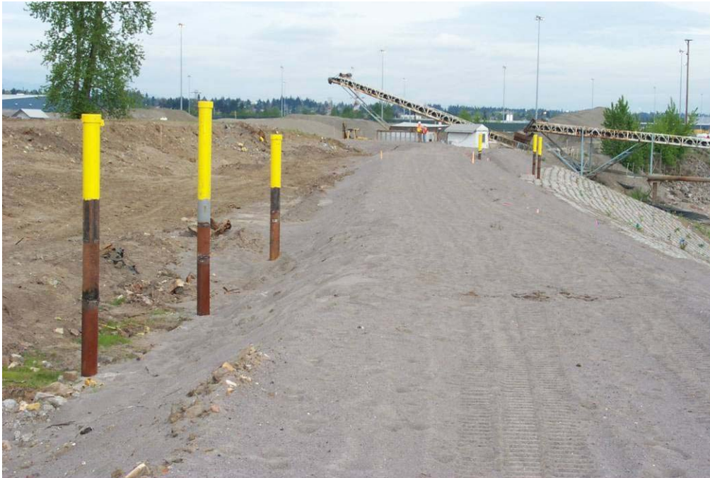
4473 May, 2004 – Anchor trench platform adjacent to ‘Armorflex’ revetment on south side of East Landfill. Monitoring well cluster 94-1 in foreground and monitoring well cluster 94-2 in background. Looking east.
