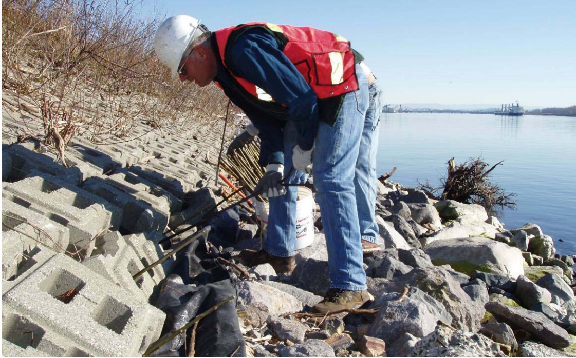
0867 January 30, 2007 – Driving of rods to create hole for planting of live stakes. Laborers standing on riprap toe. Note rootwad in background at water's edge. Looking east.
