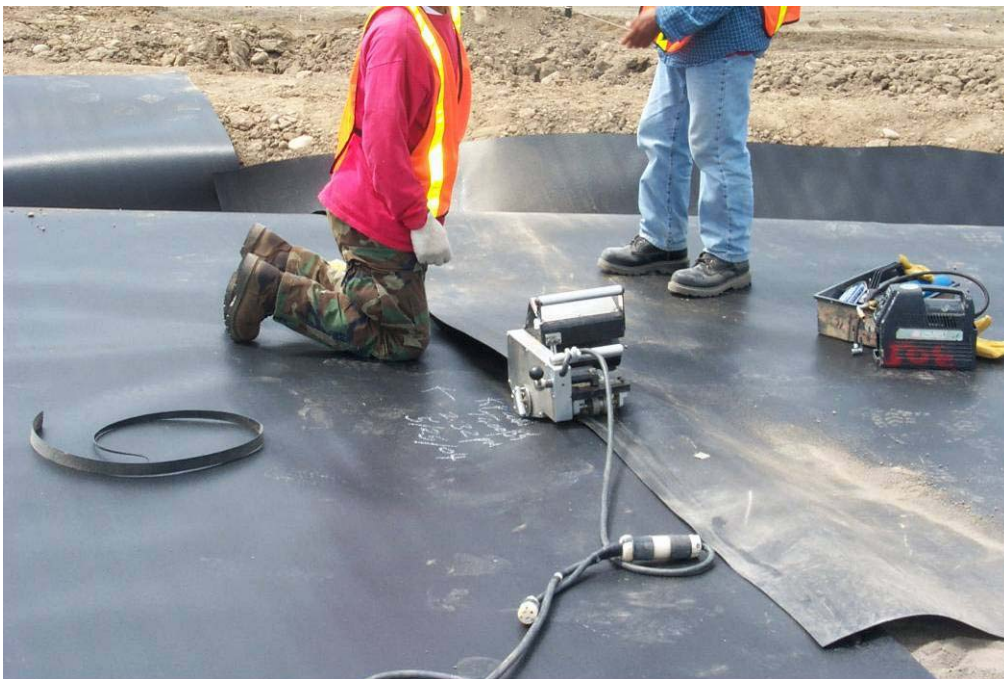
4490 May, 2004 – Field seaming of adjacent HDPE geomembrane sheets at northwest corner of East Landfill. Welding machine temperature and speed based upon thickness of geomembrane and results of peel and shear testing from test weld strip.
