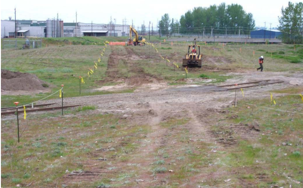
4312 April 2004 – Delineation of 'Contaminated Material Haul Road from North and North2 landfills to East Landfill using metal posts and rope/flagging. Posts capped to protect against impalement. Looking north.
