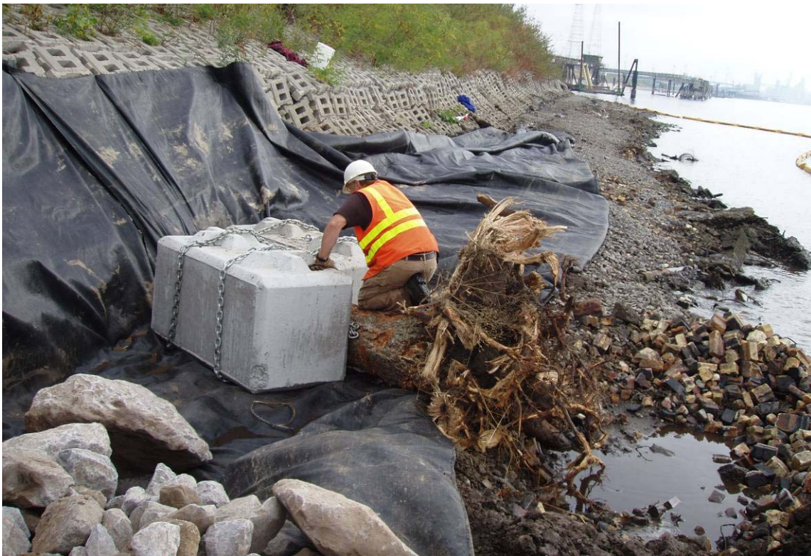
0612 October 6, 2006 – Connection of rootwad to ecology blocks using –chain. Note excavation of bench area and installation of filterfabric. Looking east.
