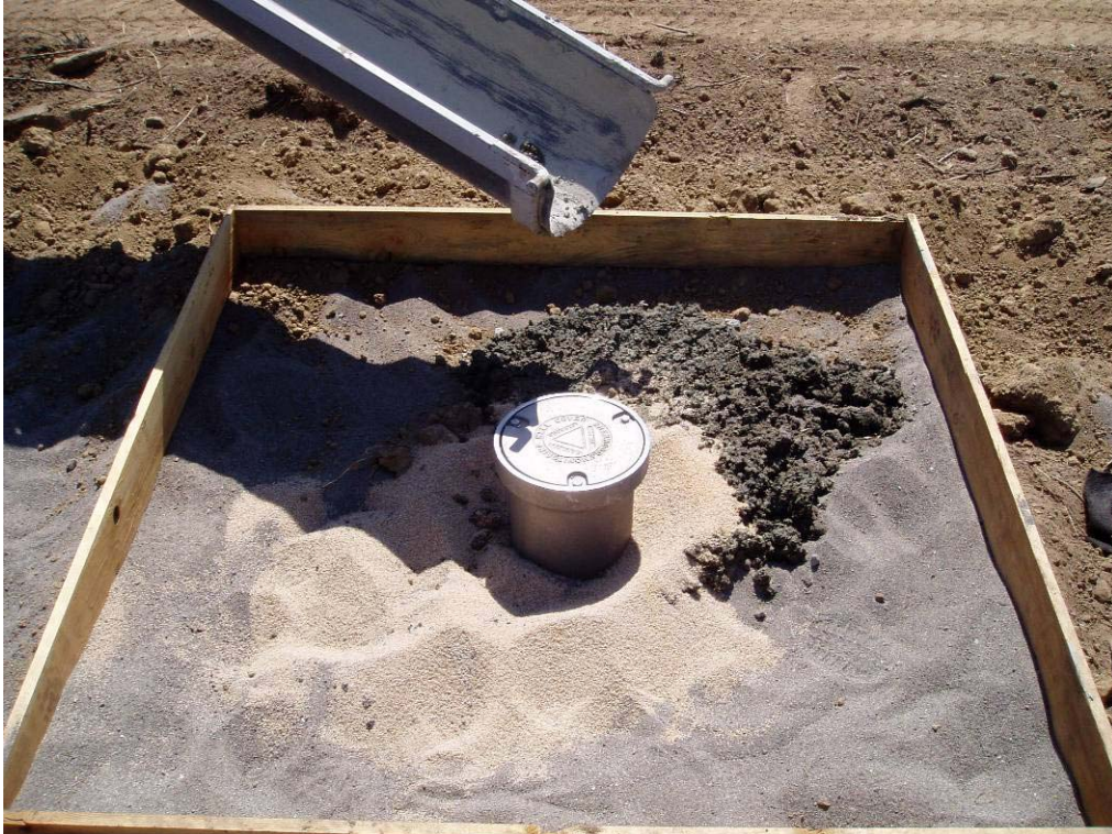
20061 August, 2004 – Placement of concrete for flush mount monitoring well pad. Concrete to be amended with 'Fibermesh' to increase tensile strength.
