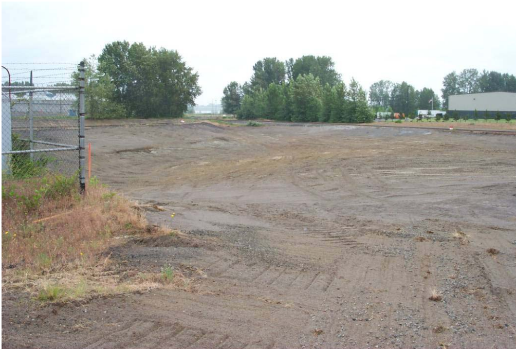
4545 May, 2004 – North 2 Landfill, after complete removal of Waste Soils and regrading of slopes. Vegetation applied in October of 2004. Looking east.
