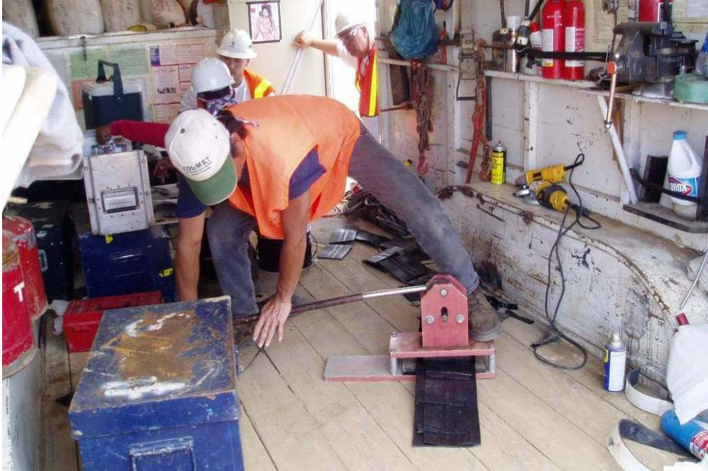
50073 May, 2004 – Geomembrane technician using a die to cut test specimen from a test weld strip. The dual wedge weld is located on the longitudinal centerline of the strip; the die cuts a 1-inch by 6-inch test specimen perpendicular to the weld. The weld of the specimen is field tested for peel and shear using a field tensiometer.
