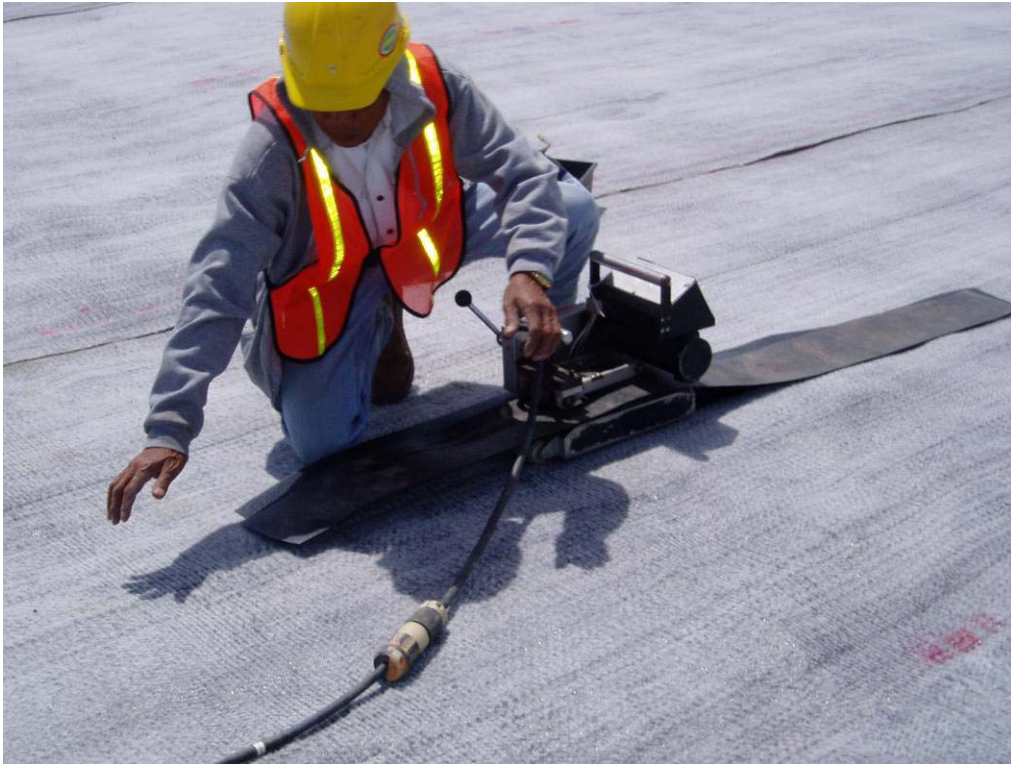
50068 May, 2004 – Field technician creating a test weld strip. The test must be performed on surface over which geomembrane is to be installed. Surface shown is Geosynthetic Clay Liner (GCL).
