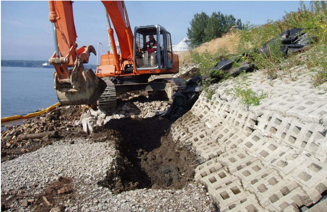
0610 October 4, 2006 – Excavation of shoreline bench area. Excavator tracking on access road constructed from riprap. Looking west.
