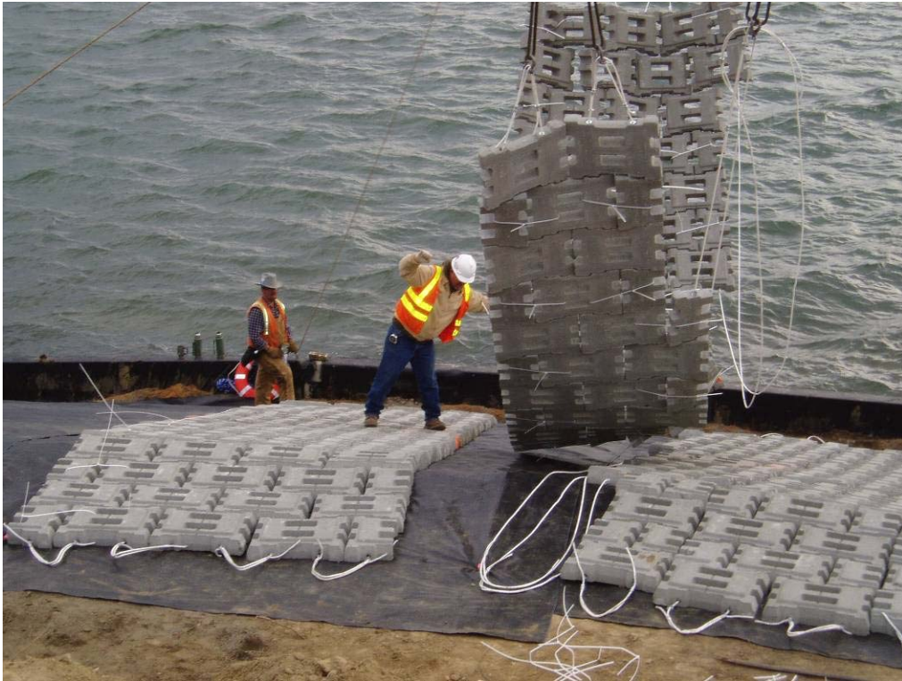
80016 November, 2003 – Installation of tapered 'Armorflex' panel along Columbia River. Note jersey barrier erosion fence in background. Looking south.
