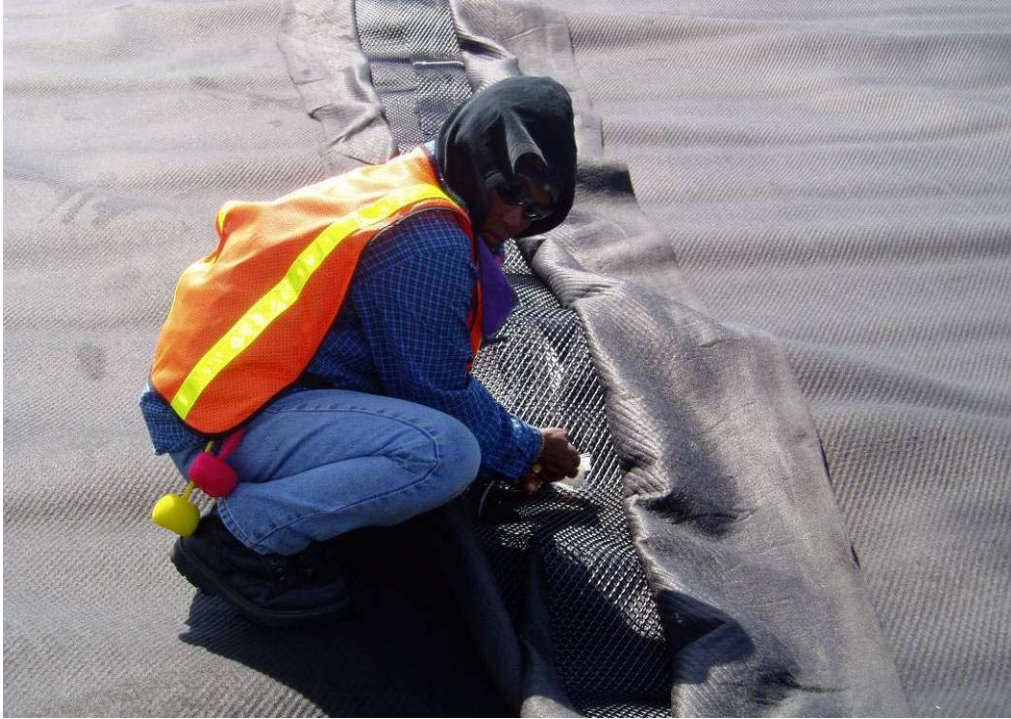
40186 June, 2004 – Field technician using white plastic zip fasteners to secure adjacent panels of drainage netting. The white color allow for quality control inspection of location (one fastener every 1.5 or 5 feet, depending on location). Filter fabric bonded to netting covers netting.
