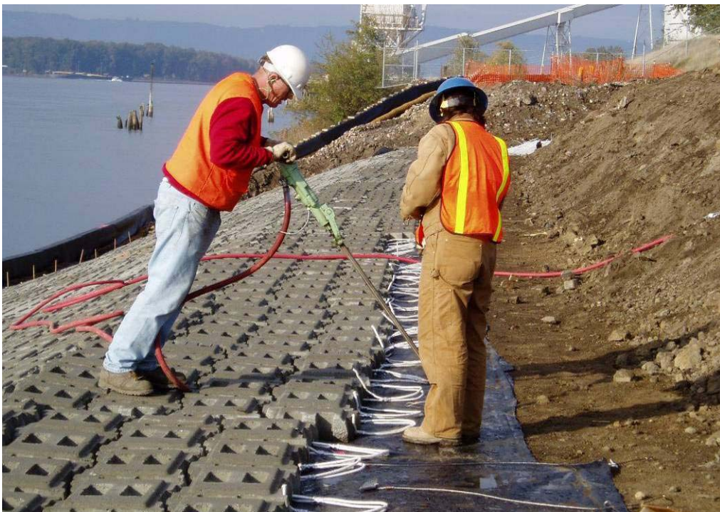
80021 December, 2003 - Installation of anchor screws at elevation 30 ft. AMSL for securing top of 'Armorflex' panels. Looking west.
