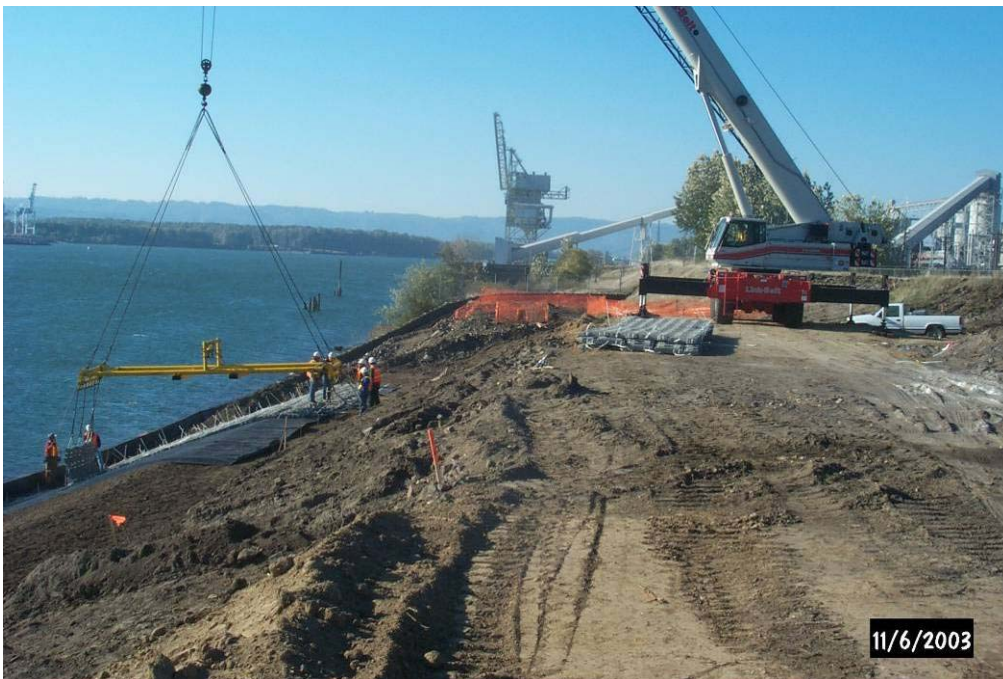
4176 November, 2003 – Crane and Spreader bar assembly used to lift and place 'Armorflex' panels. Panels delivered by truck and temporarily stored at top of embankment, if deliveries advance in front of placement. Looking west.
