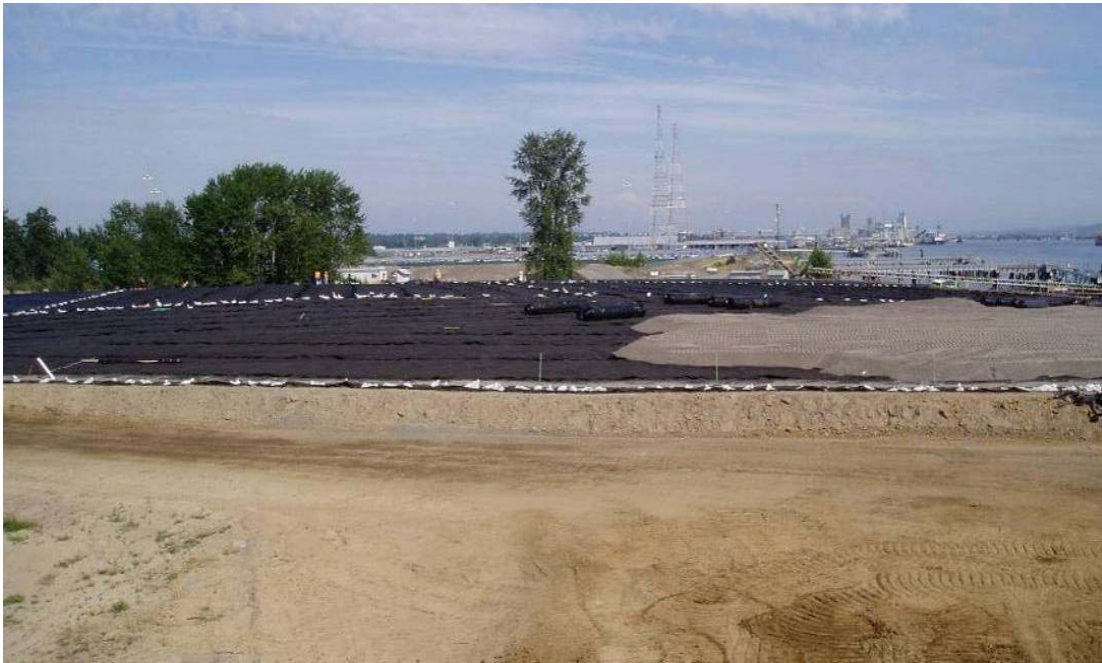
40183 June, 2004 – Panoramic view of East Landfill. Geosynthetic drainage netting (black surface) covered by random fill (gray soils). White sandbags delineate anchor trench location (sandbags used to prevent wind uplift). Note cleanout pipe in foreground at middle left. Looking east.
