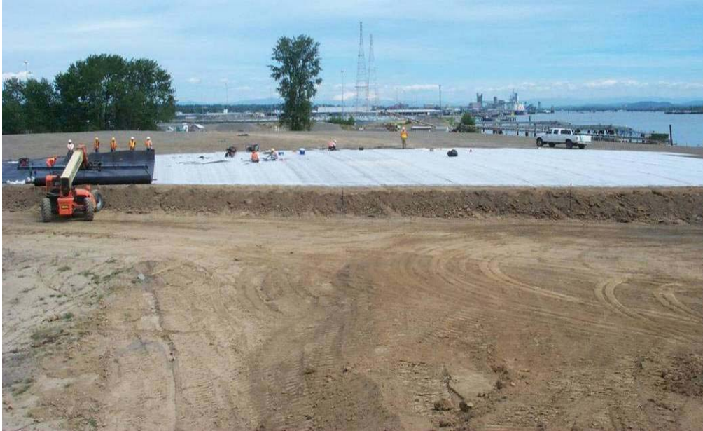
4492 May, 2004 – Installation in progress of the Geosynthetic Clay Liner (GCL) and the HDPE geomembrane at the East Landfill. Installation initiated at the west perimeter of the landfill. Geomembrane being installed at north end of landfill. Looking east.
