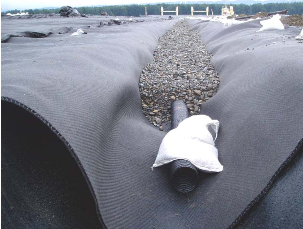
70087 May, 2004 – Placement of geosynthetic drainage netting, subsurface drainage pipe and gravel backfill in perimeter anchor trench. Filter fabric cover over gravel not present. Looking South.
