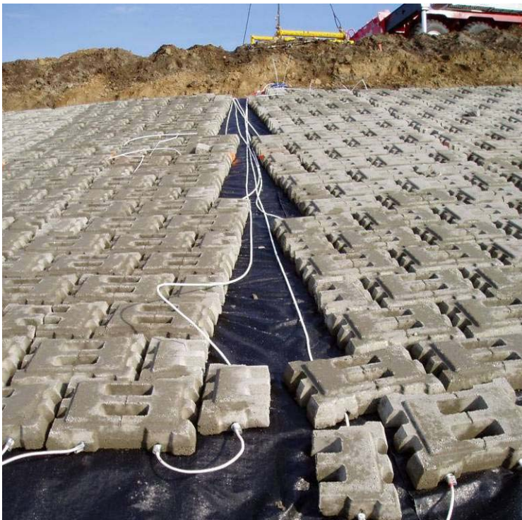
80022 November, 2003 – Placement of tapered "Armorflex" panels. Space between panels to be filled with grout. Looking north.
