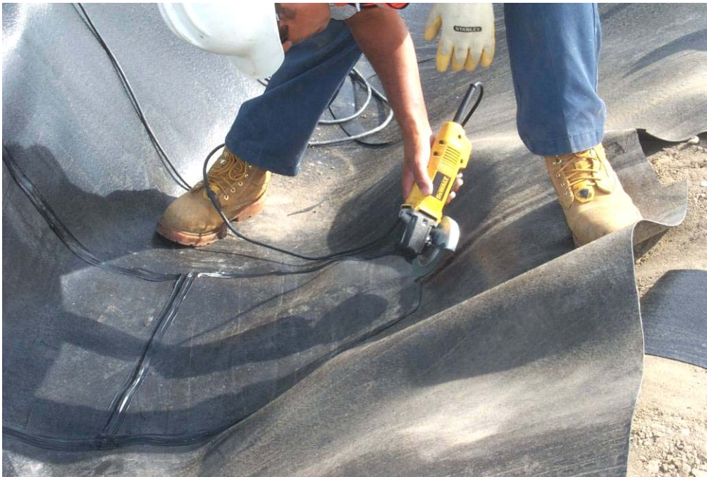
4507 May, 2004 – Grinding of geomembrane surface in preparation for extrusion welding process. Extrusion welding used at locations inaccessible to dual wedge welding machine. Grinding required to roughen surface for extrusion weld.
