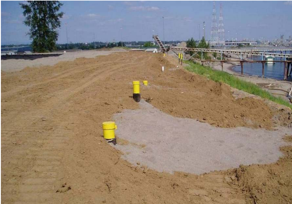
50006 June, 2004 - Spreading of 6-inch thick topsoil layer over 18-inch thick random fill layer at south anchor trench location. Monitoring well cluster 94-1 in foreground. Looking east.
