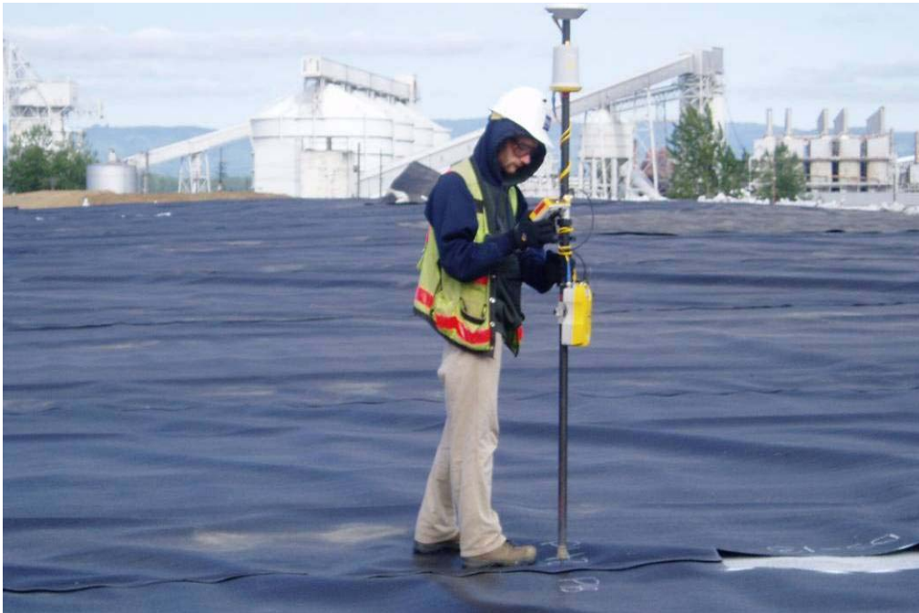
20129 June, 2004 – W&H Pacific technician locating edge of seam with global positioning system (GPS). Information to be used in development of as-built drawings.
