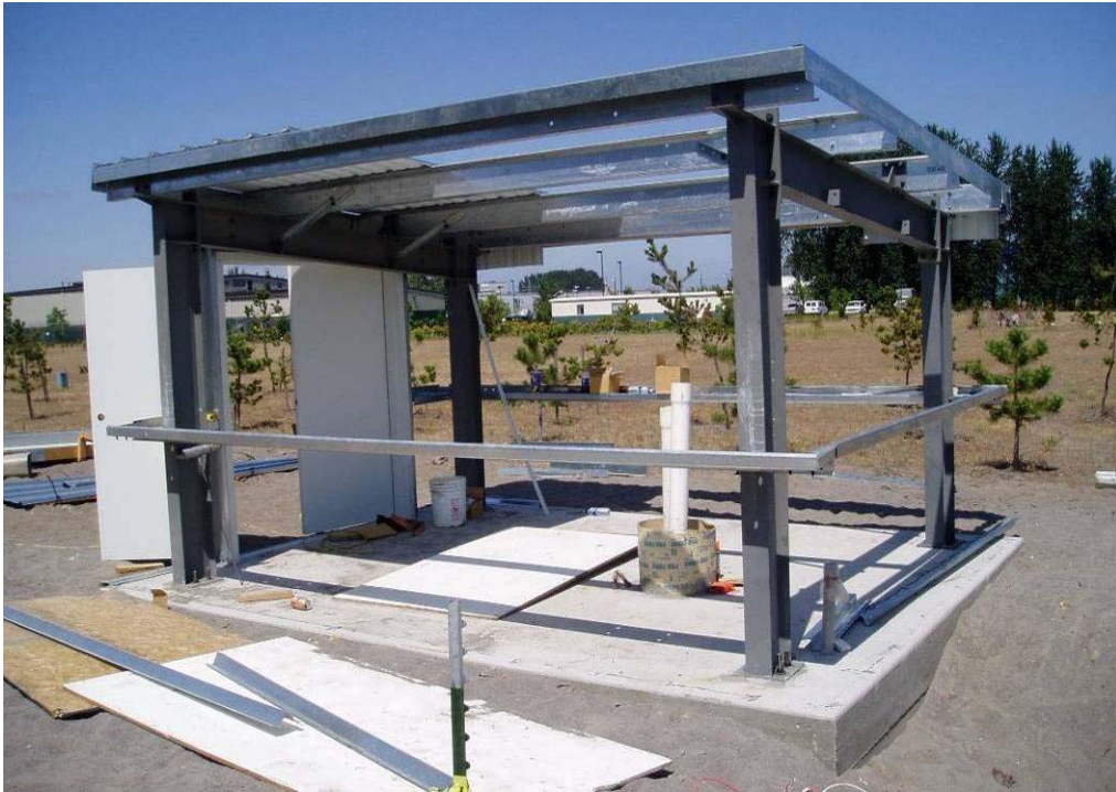
20055 August, 2004 – Structural assemblage of Storage-Operations building. Pipes extending up from center of floor are water supply line (originating from east (right side) of picture) and water feed line for sprinkler system (extending to west (left side) of picture).
