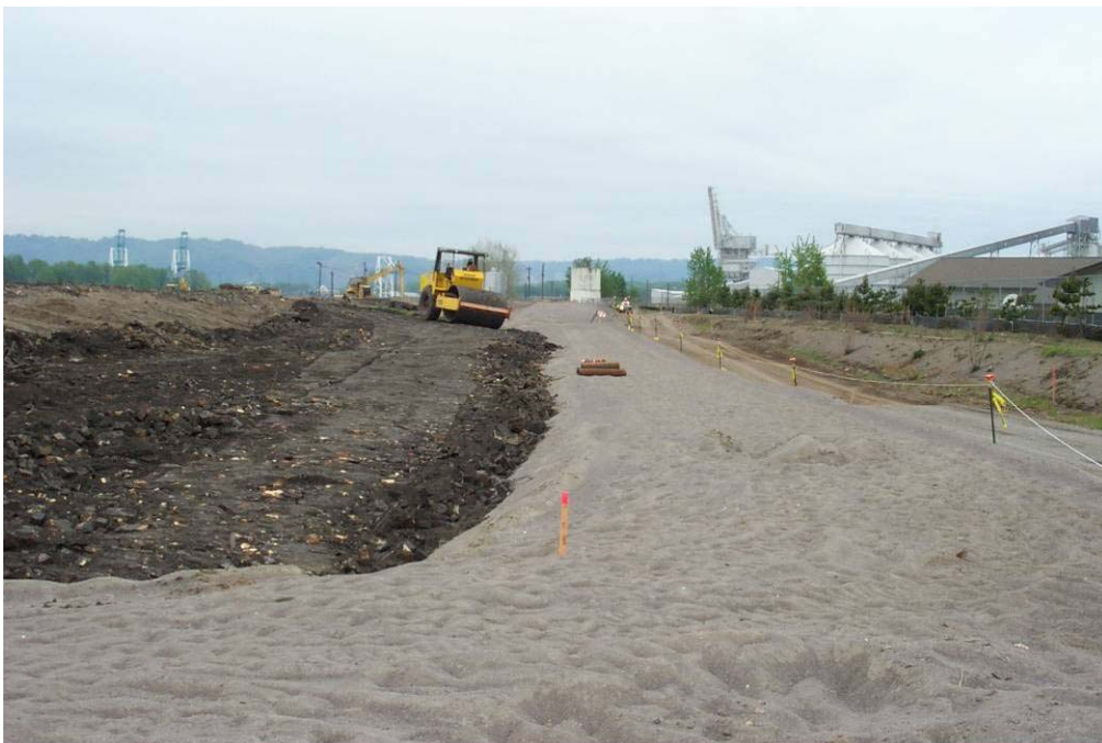
4452 May, 2004- Placement of 'Waste Soils' against anchor trench platform on north side of East Landfill. Looking west.
