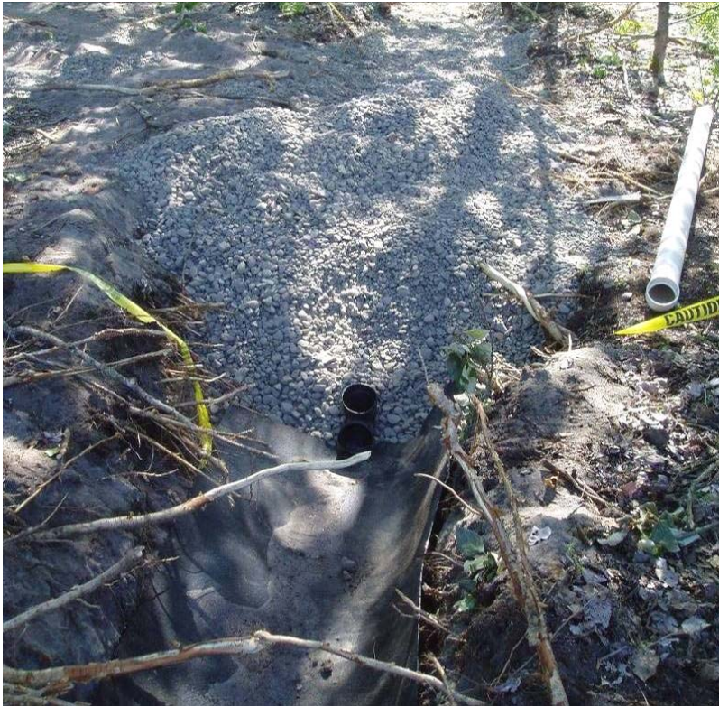
40177 June, 2004 – Completed Biodiffuser trench with gravel backfill. Exposed pipe to be connected to tee from perimeter anchor trench drain.
