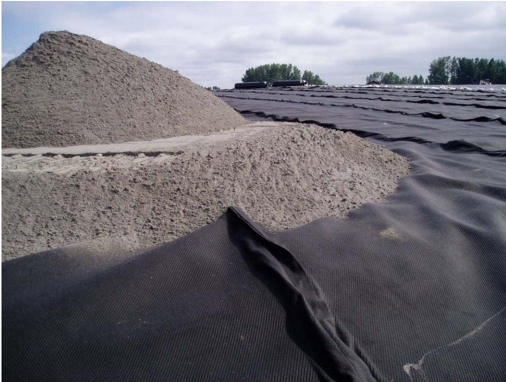
20138 June, 2004 – Stockpile of sand for construction of 18-inch thick random fill layer.
