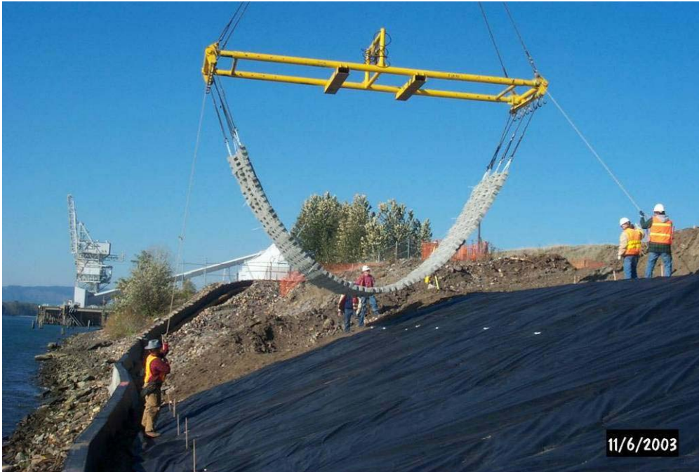
4170 November, 2003 – Installation of the first full panel of 'Armorflex' at west end of regraded shoreline along Columbia River. Looking west.
