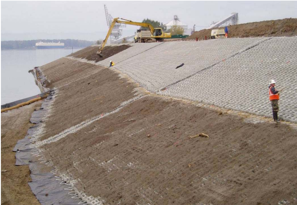
40100 December, 2003 - Placement of topsoil within open spaces of 'Armorflex' panels at west end of shoreline, above elevation 18 ft. AMSL. Black line gaps in panels (from top of slope to bottom) are tapered panel locations (to be filled with grout). Looking west.
