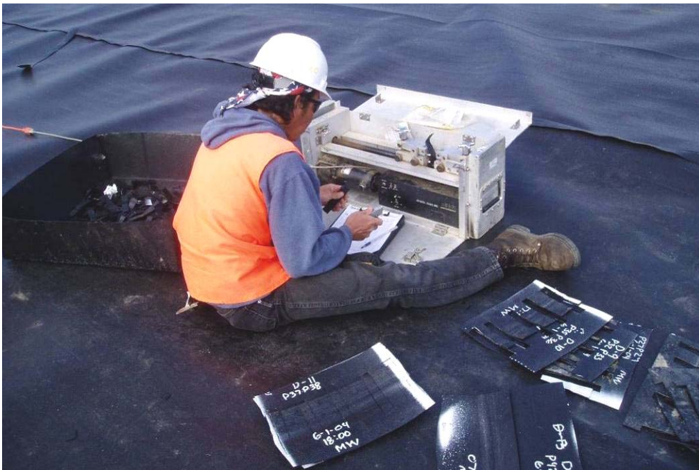
20127 June, 2004 – Field technician using field tensiometer to check shear and peel strengths of destructive test samples removed from completed geomembrane panel welds.
