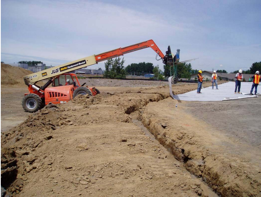
50071 May, 2004 Installation of Geosynthetic Clay Liner (GCL) within anchor trench on east side of East Landfill. Looking North.
