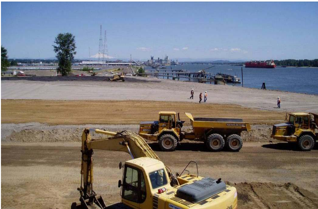
50004 June, 2004 - Spreading of 6-inch thick topsoil layer over 18-inch thick random fill layer. Both layers installed over geosynthetic layers. Looking east.
