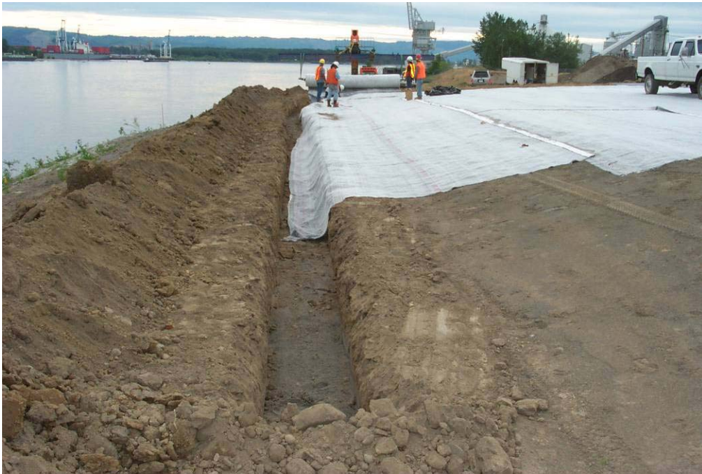
4510 May, 2004 – Geosynthetic Clay Liner (GCL) installed in southern anchor trench, along Columbia River. Looking west.
