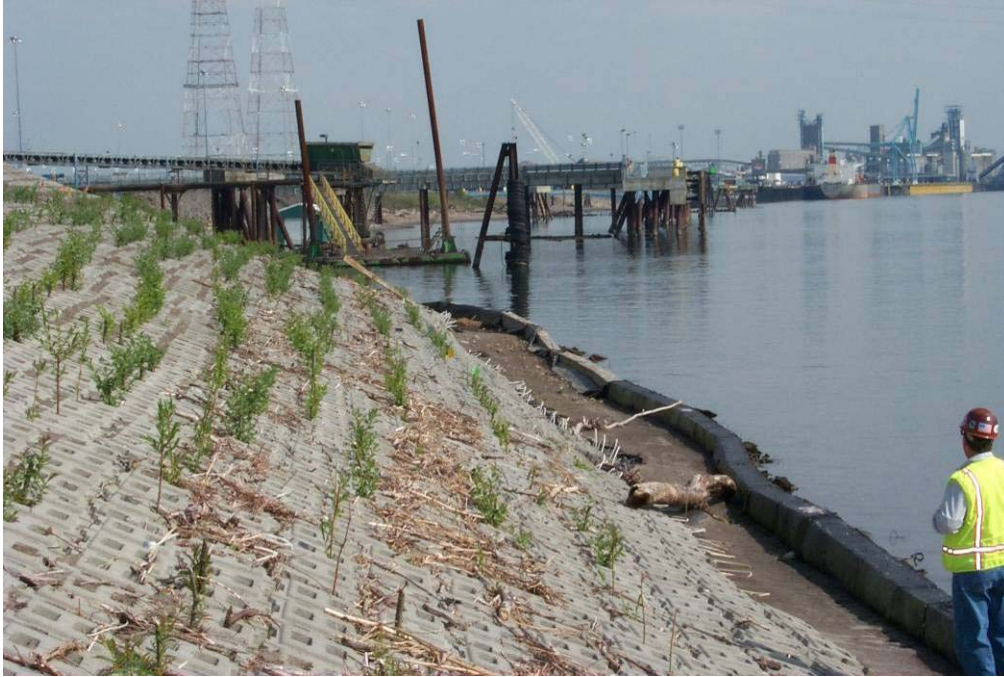
4337 April, 2004 – Completed construction of 'Armorflex' concrete revetment along reconstructed embankment of Columbia River. Vegetation in picture is 3 months old. Looking east.
