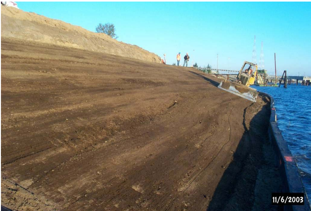
4182 November, 2003 – Fine grading of 2.5H:1V slope prior to 'Armorflex' installation. Looking east.
