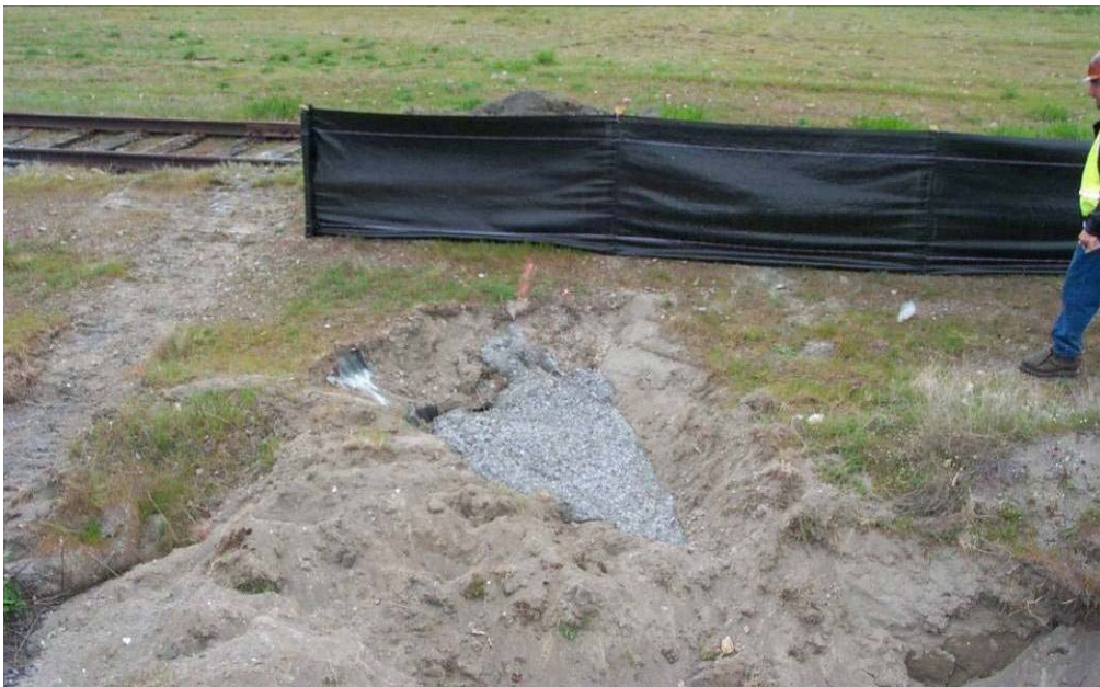
4314 April, 2004 – Low-density concrete backfill of an abandoned culvert formerly used to divert flow from adjacent area to North 2 Landfill. Looking north.
