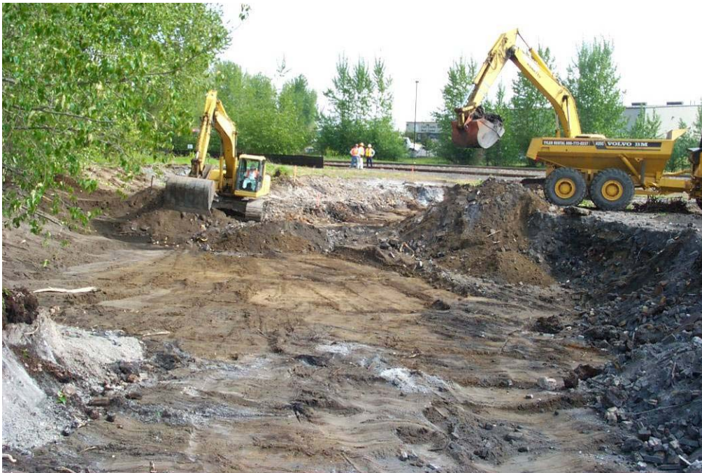
4331 April, 2004 – Excavation of 'Waste Soils' at east end of North 2 Landfill. Looking east.
