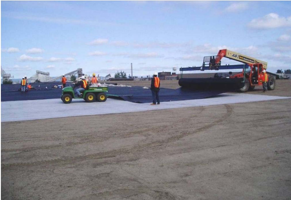
20125 June, 2004- Unrolling of geomembrane over geosynthetic clay liner (GCL). Geomembrane pulled across East Landfill with ATV. Spreader bar used to suspend geomembrane roll in air for ease of deployment.
