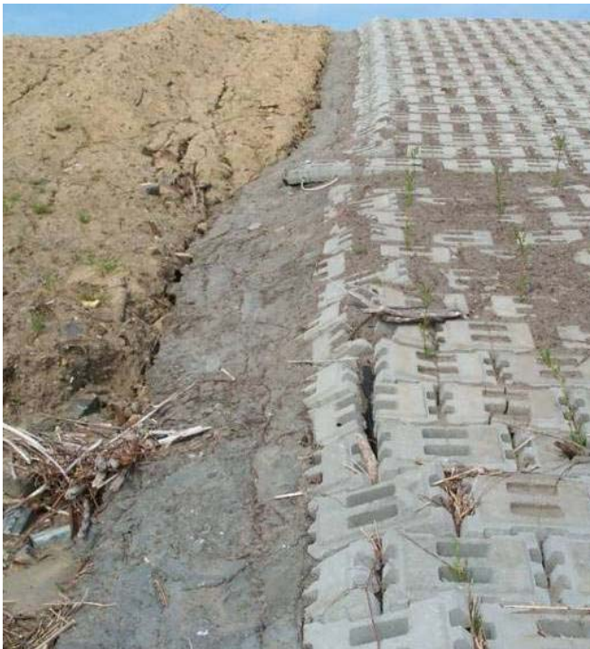
4340 April, 2004 – The grout filled anchor trench at the downstream end of the 'Armorflex' revetment, required by the manufacturer's installation manual. Trench is 3 feet deep. Looking north.
