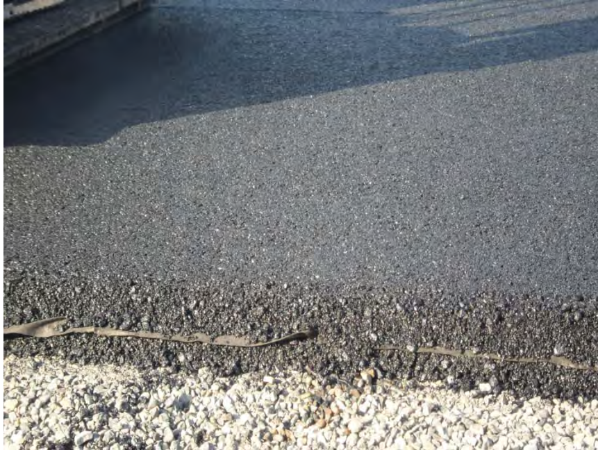
Photo 15 SPL Test Pad Geotextile Interlayer between HMA Base Layer and Top Layer 3/05/2010
