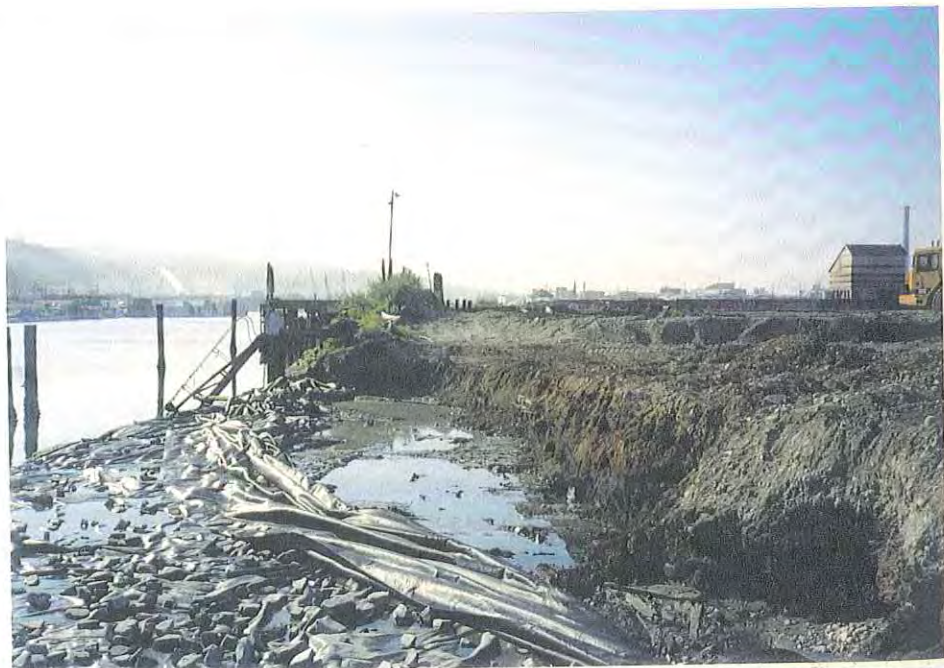
Looking up the Waterway at the Shoreline Excavation, Dark Material in Cut is Sawdust
