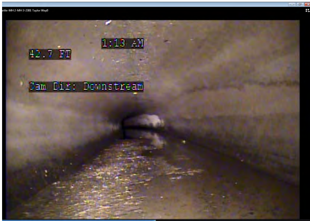
Photo #7 - Accumulation of Sediment at 43 Feet Downstream of MH2
