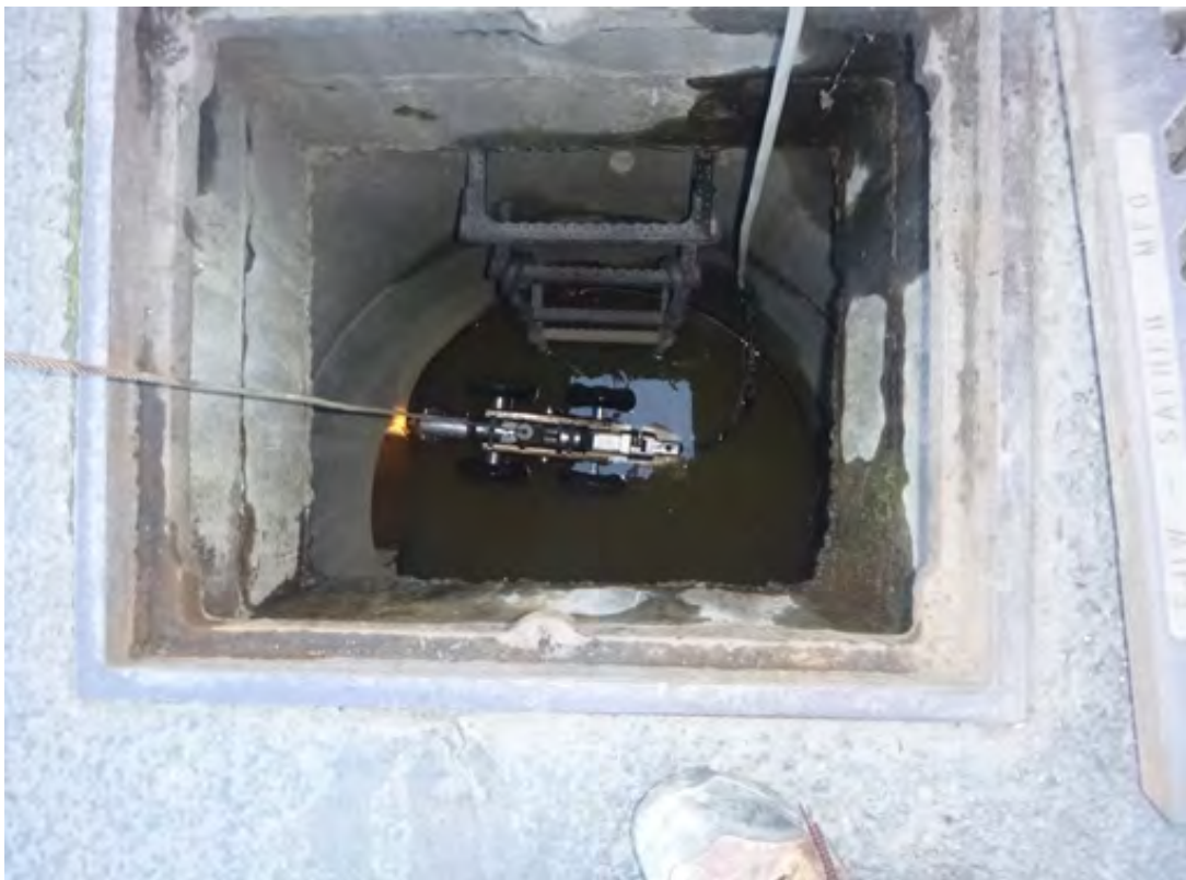
Photo #1: MH1 Showing Seepage
