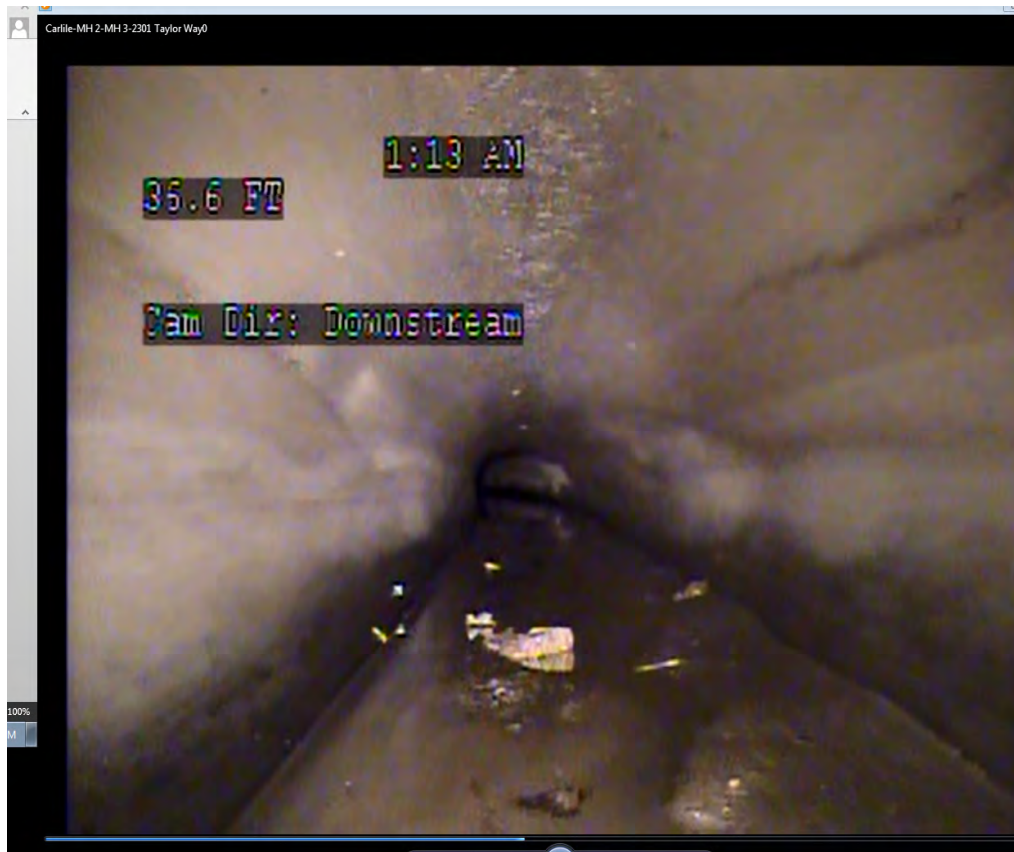
Photo #6 – Accumulation of Sediment at 37 Feet Downstream of MH2
