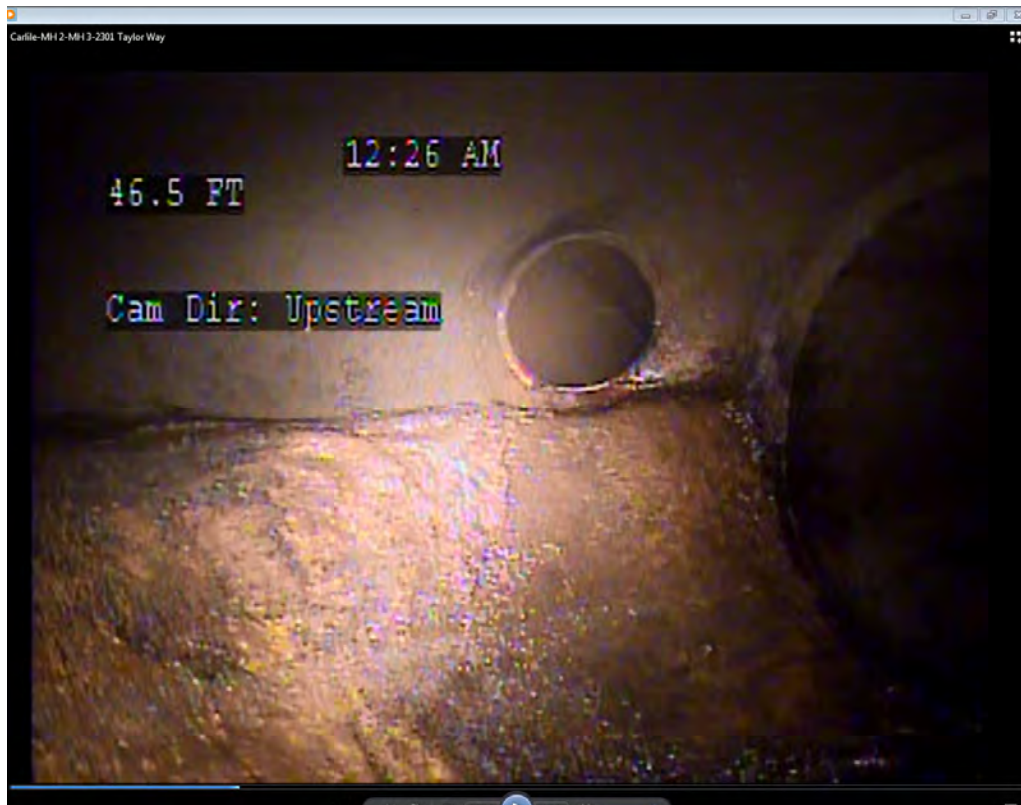
Photo #8 – MH5 Showing the Outfall of an Unknown Section of Storm Drain Line
