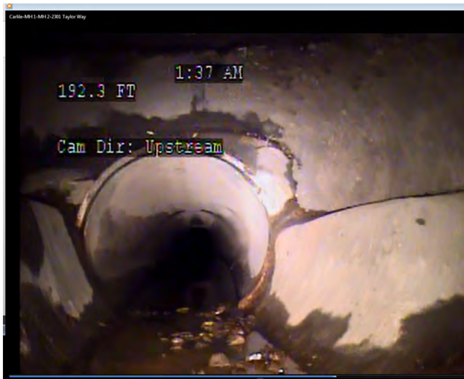
Photo #5 - MH6 with Seepage around the Mortared Pipe Connection
