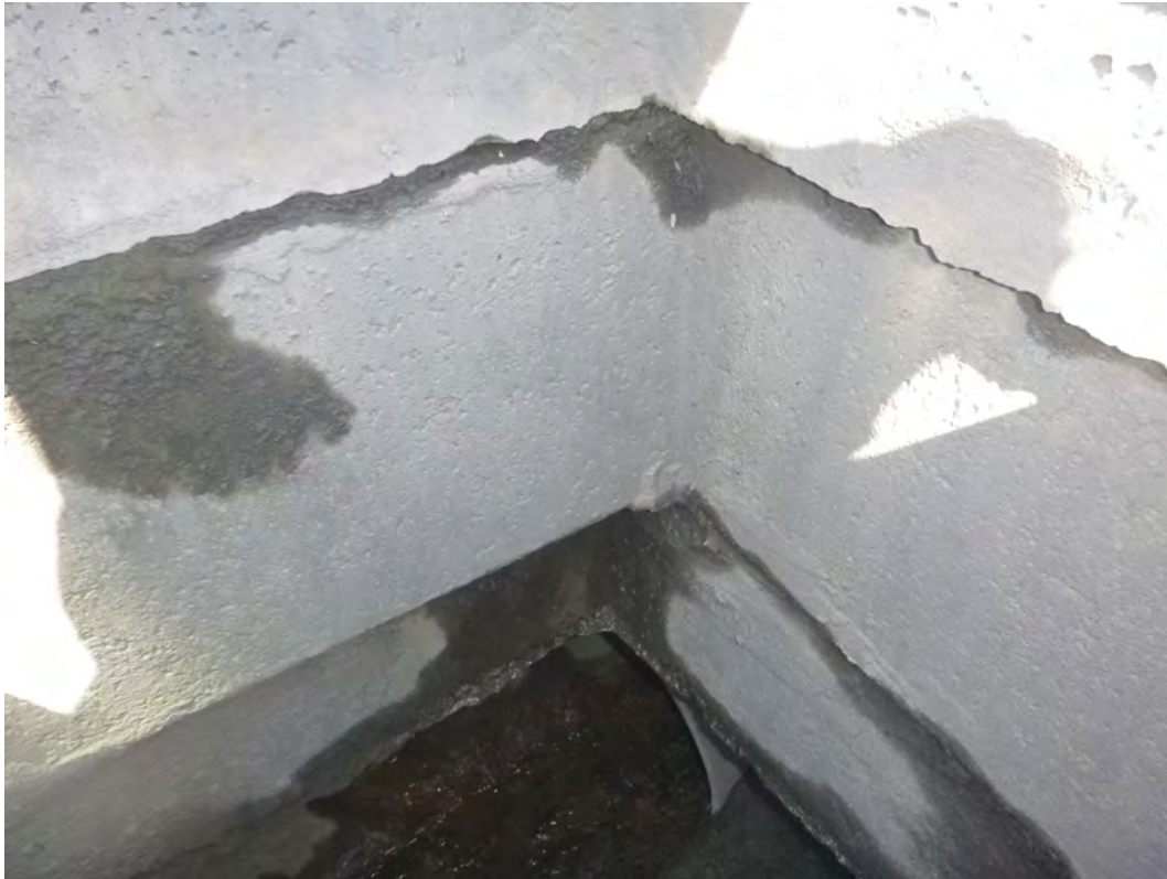
Photo #2: MH6 Showing Seepage
