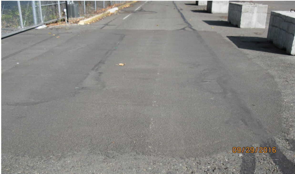
Photo 5: Cap Repair and Sealing at the Western Property Boundary of the Site– from the North
