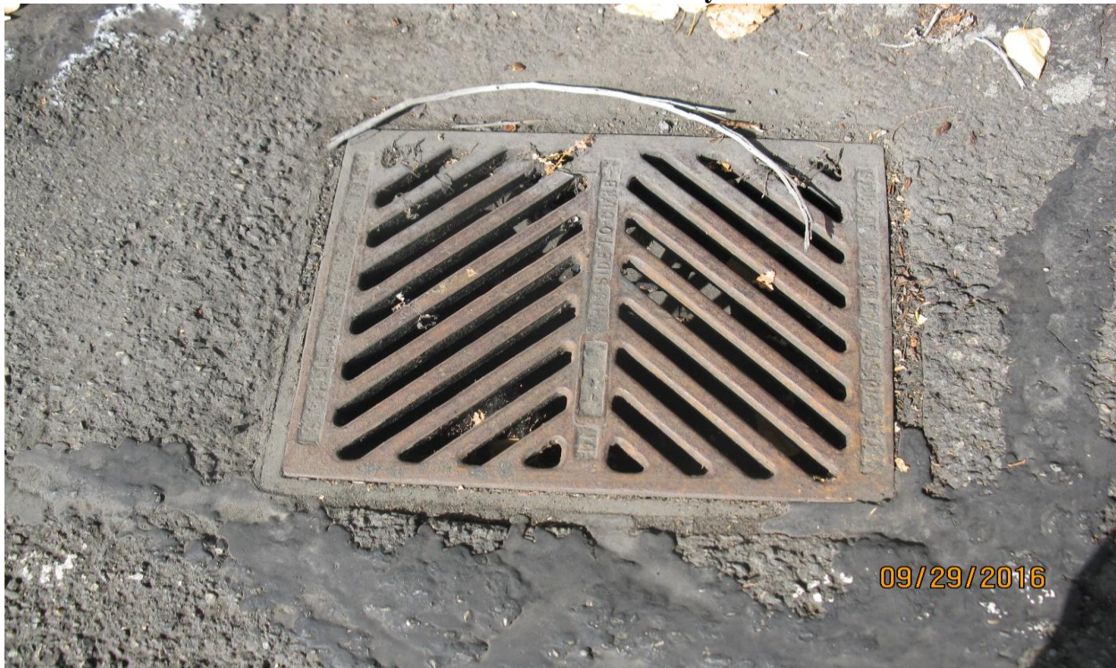
Photo 6: One of the Catch Basin at the Western Boundary of the Site
