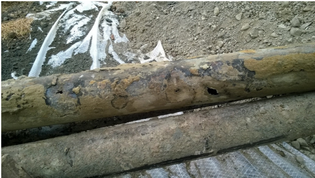
Photograph. Close up of corrosion and holes in Pipeline 8.
