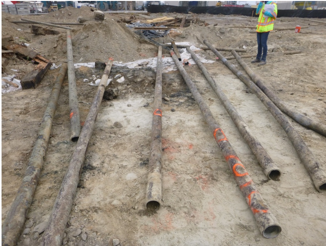
Photograph 3. Holes and corrosion in Pipeline 8 outlined by orange paint.
