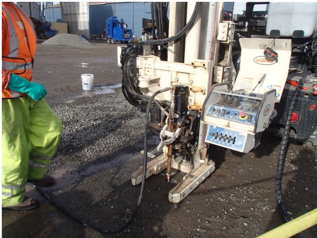
Photograph 18. Bio-injection point in S. Cedar Street.
