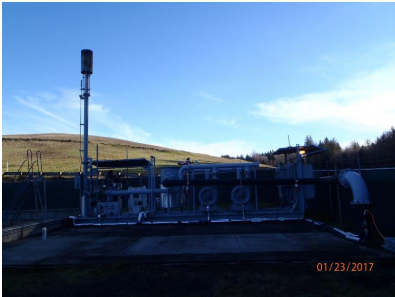
Photo 4: Landfill gas blowers and flare
