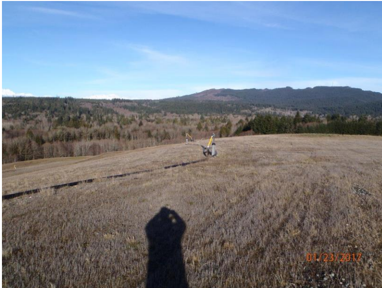
Photo 3: Landfill gas extraction wells on top of Phase II cover
