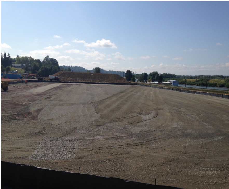
Looking southwest at crushed surfacing placed on ballast in the sediment handling area. Minor grading still required.
