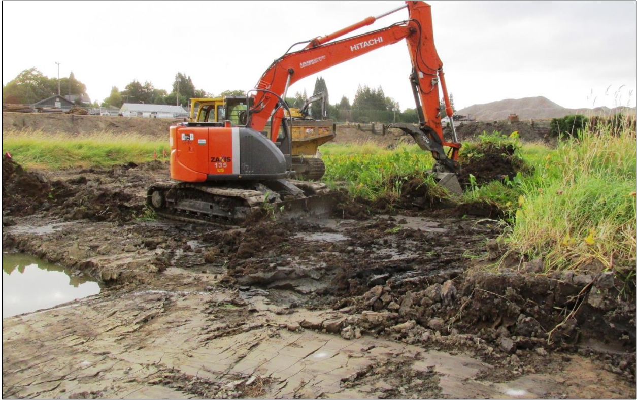
Figure 4. View of sediment removal excavation in the central portion of the remedy area on September 8, 2014, facing southeast.
