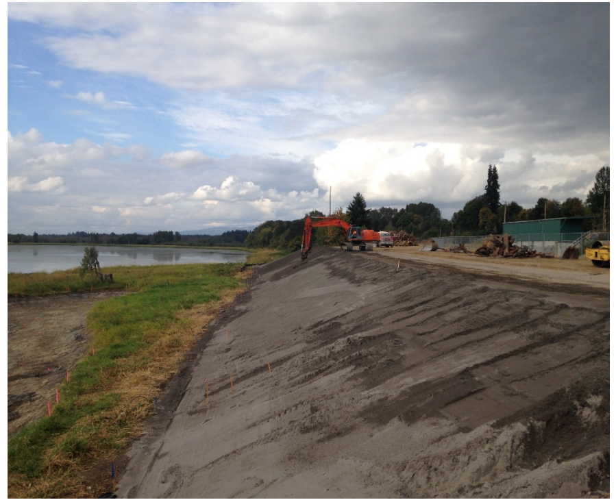
Looking north at the excavator dressing the slope of the east embankment. Note the tracks from the roller passes on the top lift.
