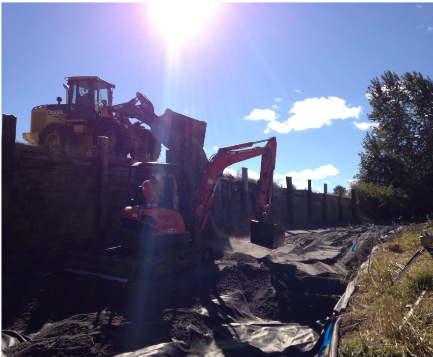
Looking west at the placement of sand on fabric at the westernmost extent of the stabilization embankment.
