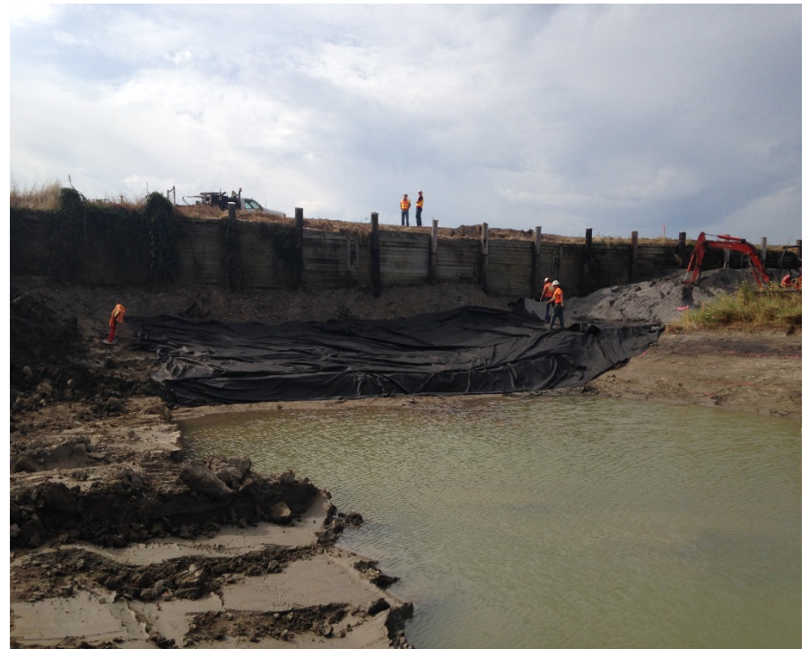
Looking south at the placement of filter fabric on the embankment and keyway subgrade on the south embankment.
