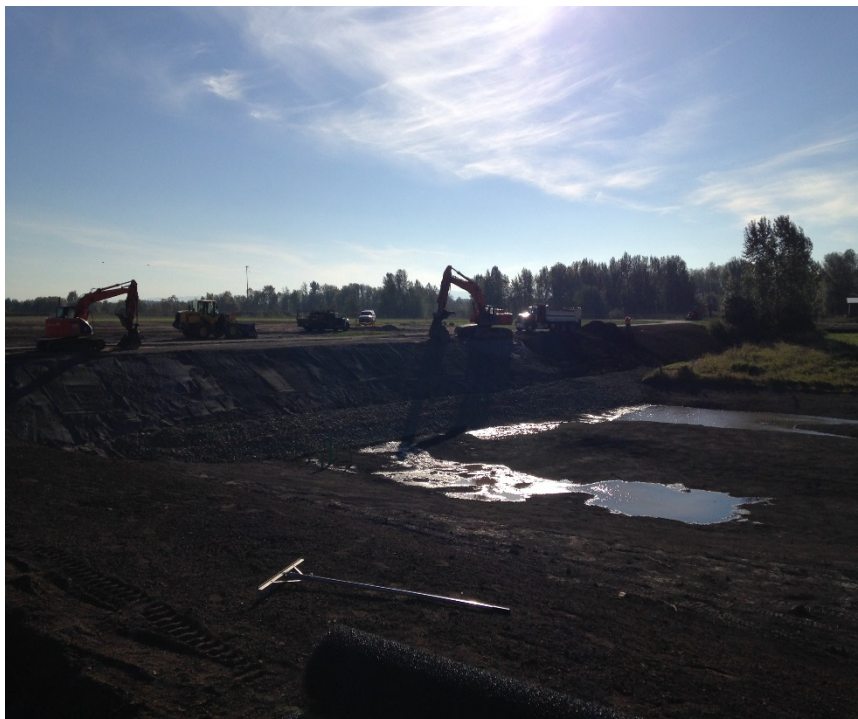
Looking southwest at the extent of structural fill and topsoil placed on the south embankment today.
