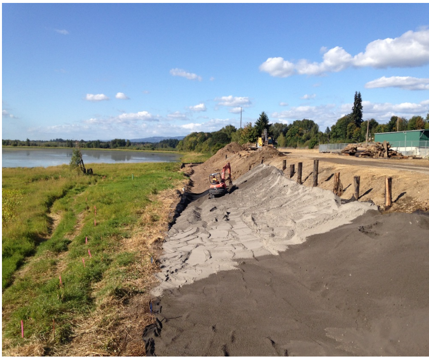
Looking west at the placement of sand on fabric on the east stabilization embankment.
