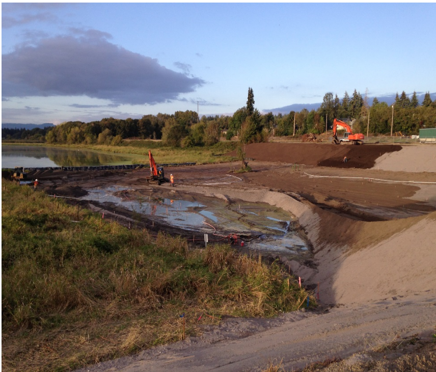
Looking northeast at the remedy area progress. Note the extent of topsoil placed on the east embankment and amended sand placed in the lake.
