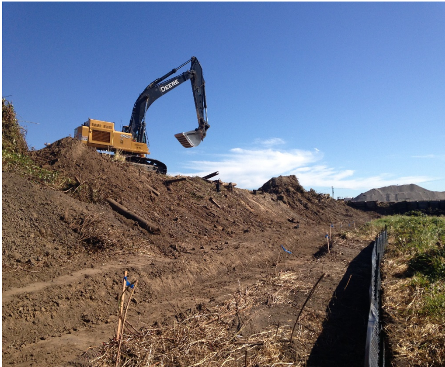
Looking south at the east embankment being cleaned up to prepare for fill placement.
