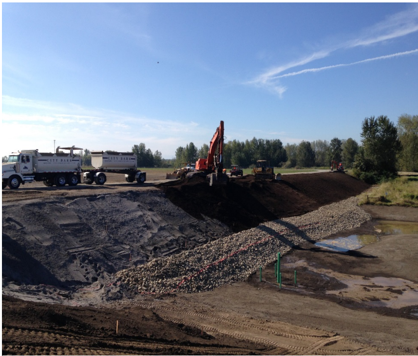
Looking southwest at the extent of topsoil placed on the south embankment by mid-day. Note the two grade breaks on the embankment.
