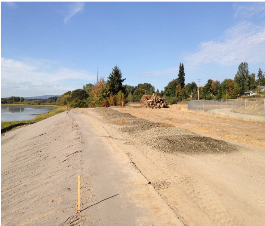
Looking south at crushed surfacing base course placed on the hard trail subgrade for placement and compaction.
