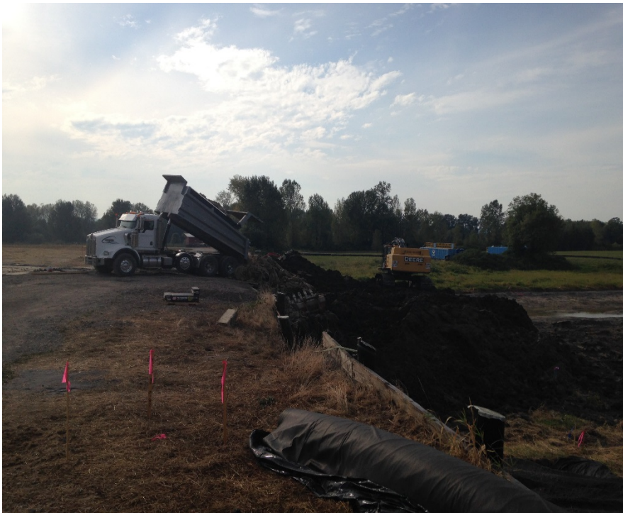
Looking west at Strider dumping the fabric from the upland staging and sediment handling area on the sediment stockpile for disposal.
