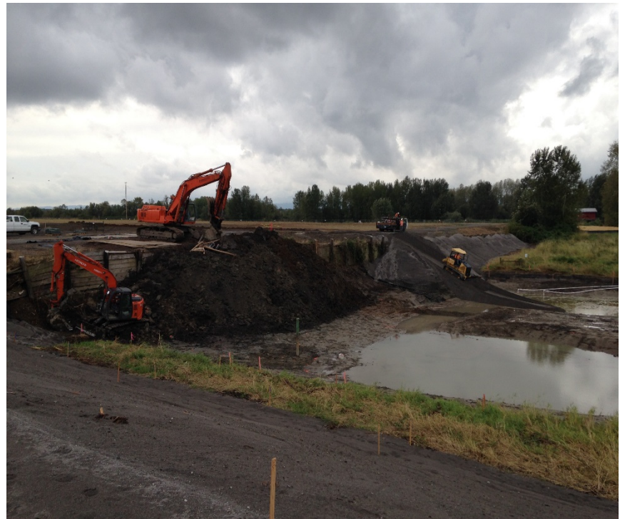
Looking southwest at the progress on the stockpile and the sand "road" to the remedy area.
