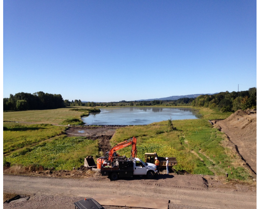
Looking north at extent of completed sediment excavation. Note equipment fueling up from bulkhead.
