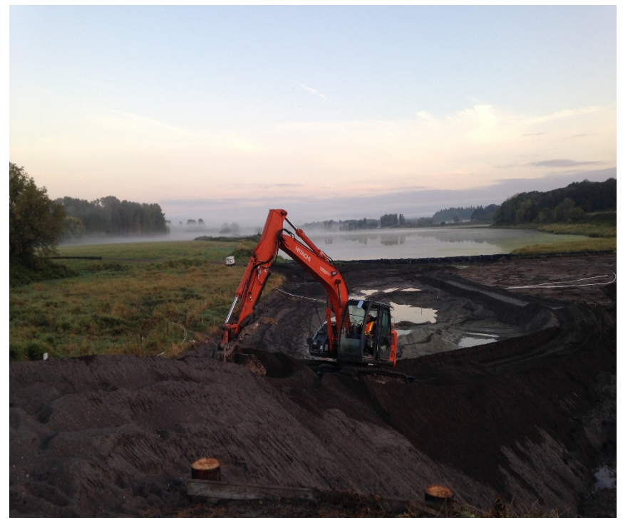
Looking north at the Hitachi cleaning up amended sand from the "access ramp." Note the dewatered remedy area.
