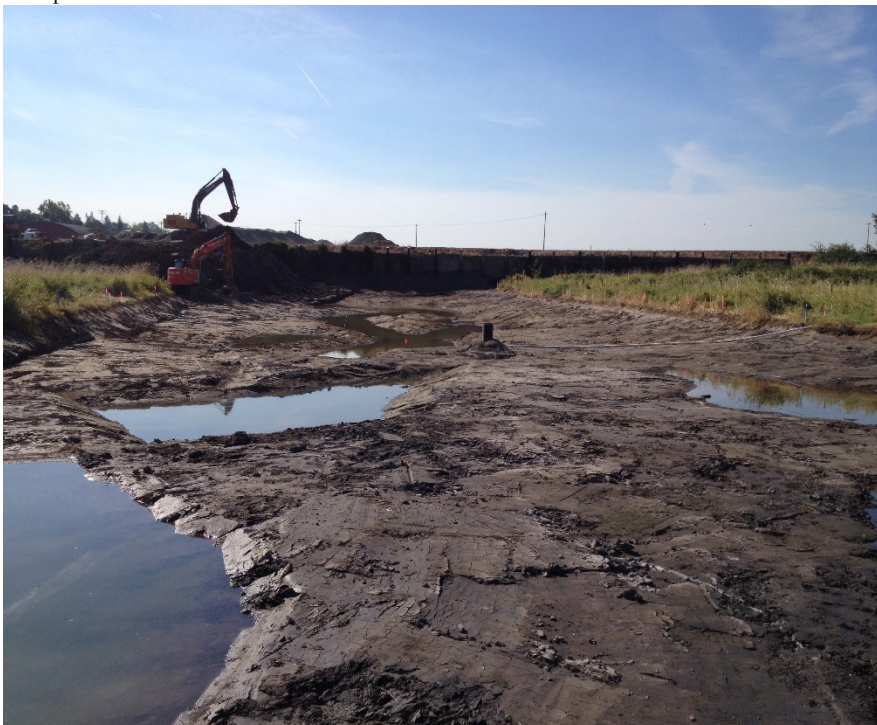
Looking south at the western portion of the remedy area with the sediment stockpile and bulkhead in the background.
