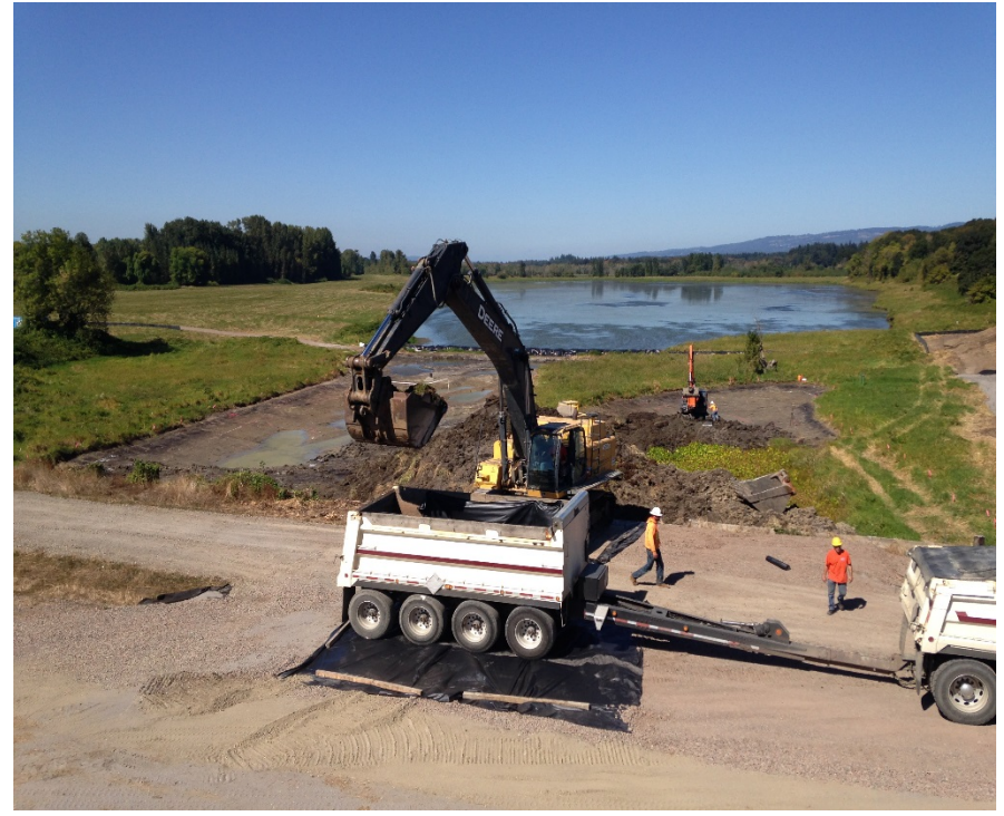
Looking north at the first truck getting loaded with sediment for disposal.
