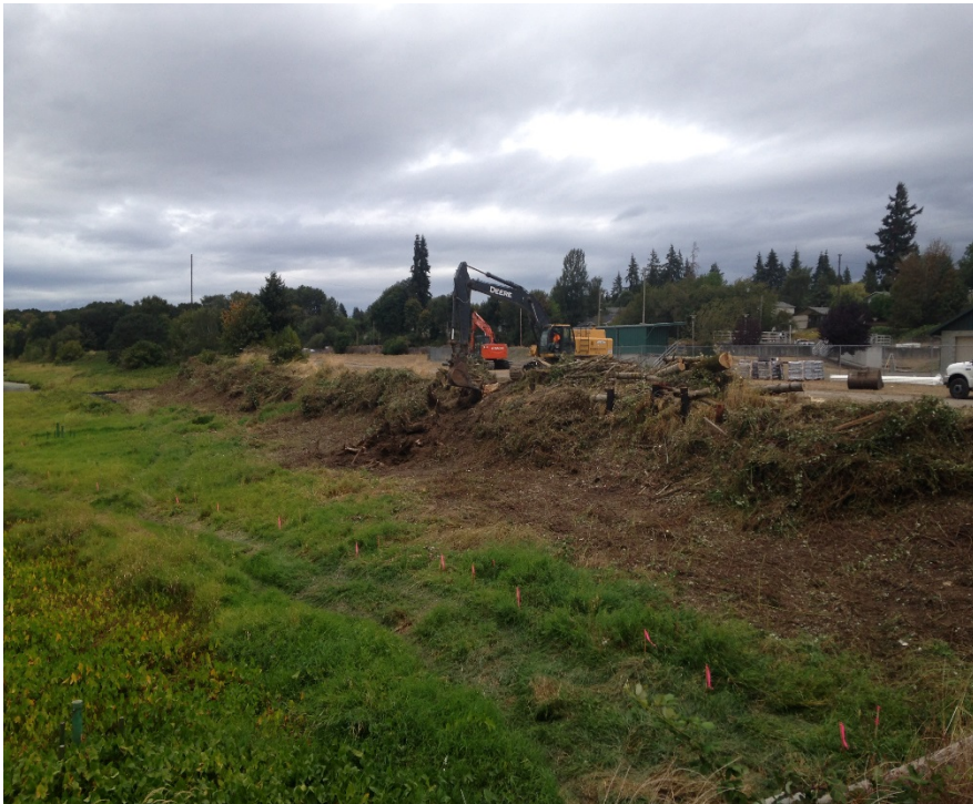
Looking northeast at the 450 excavator removing a stump on the east embankment.
