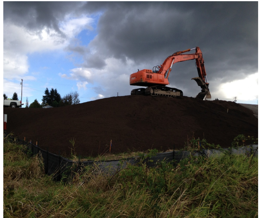
Looking southeast at the north corner of the east embankment, at the placement of the topsoil overlay.
