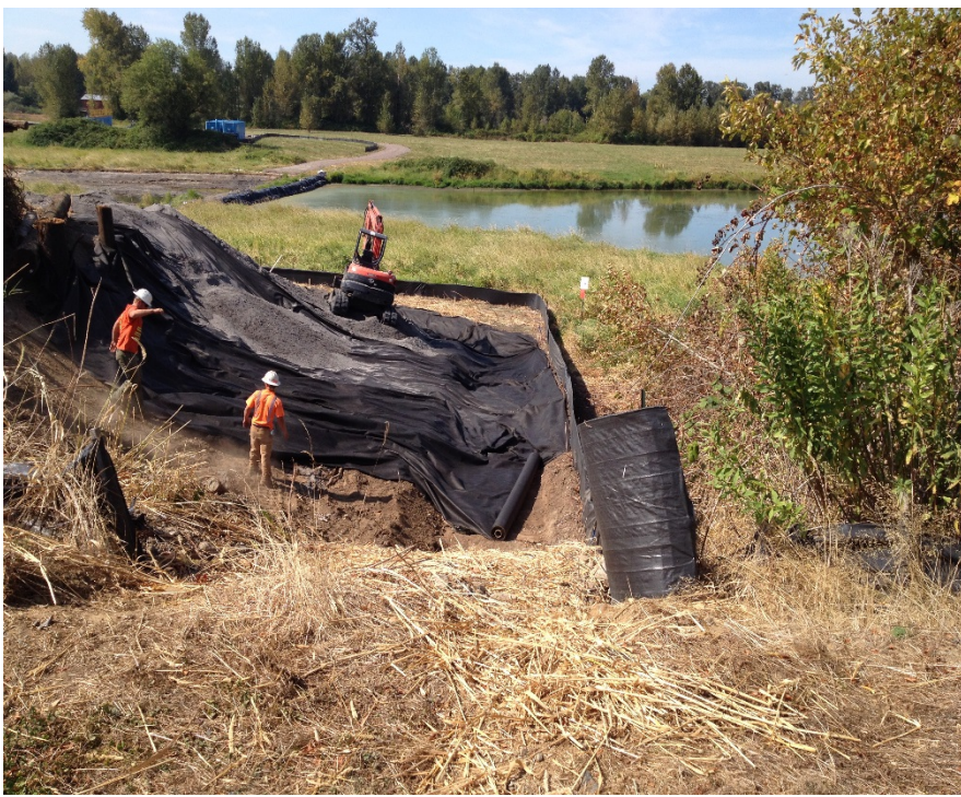
Looking west at filter fabric installation within the footprint of the northern terminus of the east embankment.
