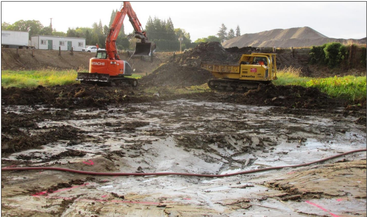
Figure 5. View facing south of an excavator stockpiling sediment for removal from the site on September 12, 2014.
