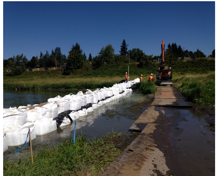
Looking east at the temporary isolation barrier, before the final wrap with visqueen.
