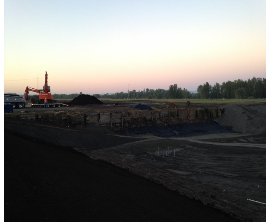
Looking southwest at the ramp and structural fill placed on fabric on the south embankment. The last area is awaiting survey.
