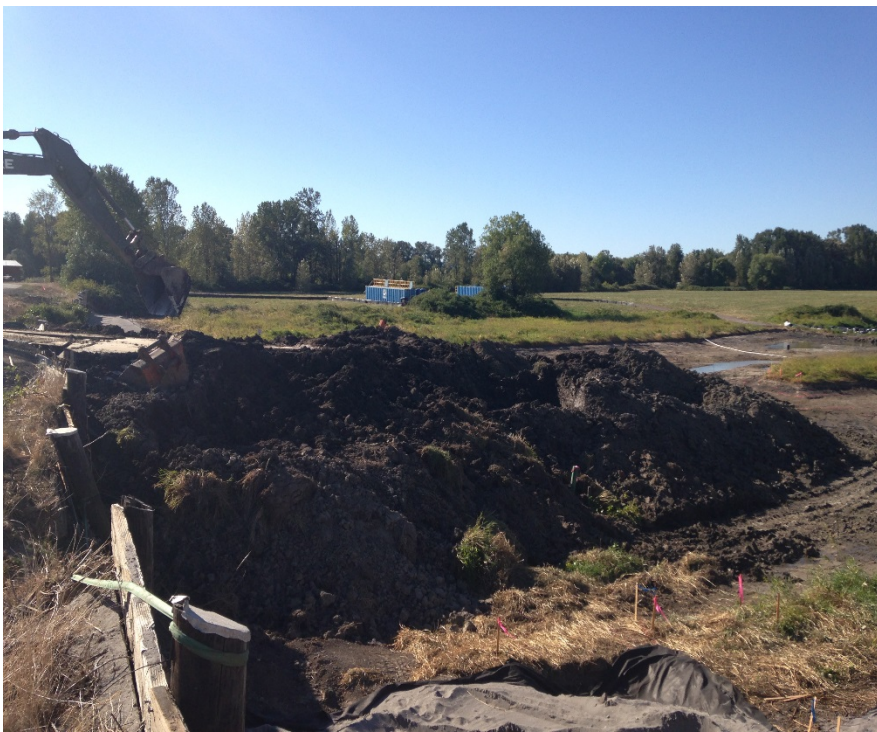
Looking west at the stockpile of contaminated sediment awaiting transport and disposal.
