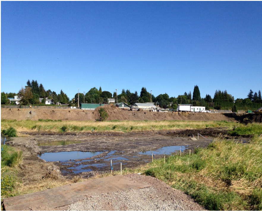
Looking north at extent of completed sediment excavation. Note equipment fueling up from bulkhead.
