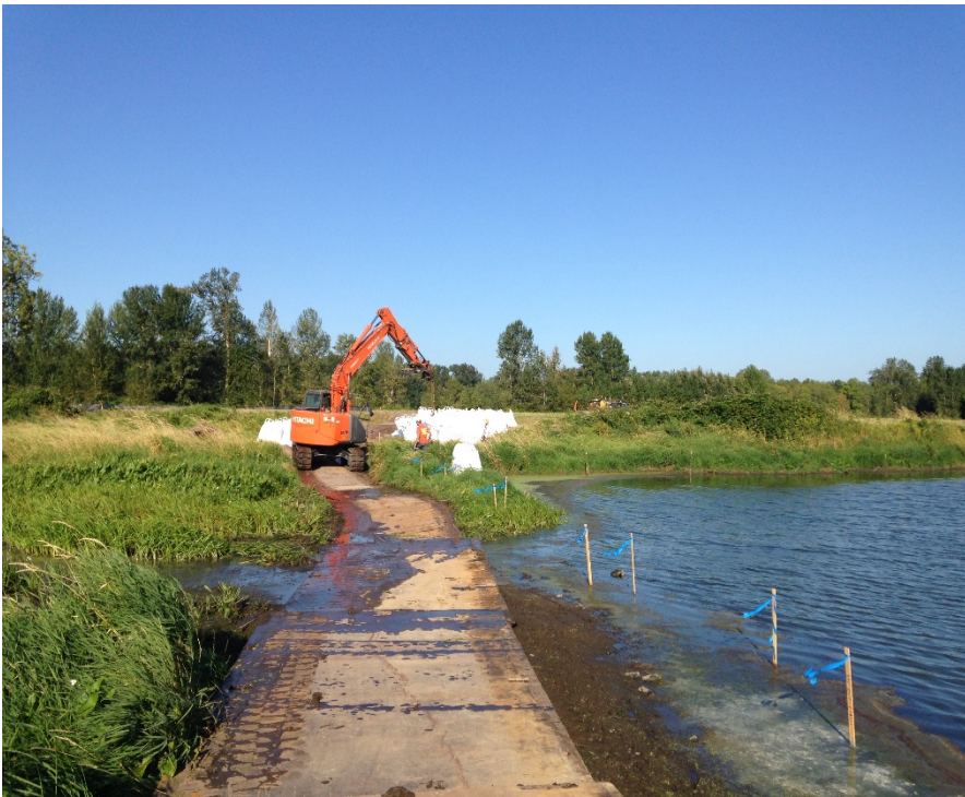
Looking west at the first bulk bag being placed in Carty Lake.
