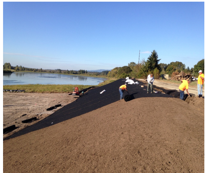
Looking north at the placement of TRM by Paul Bros. on the east embankment.
