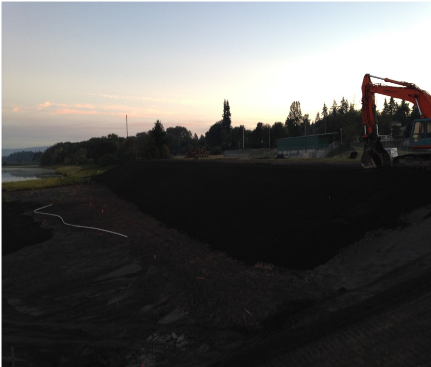
Looking northeast at the east embankment progress. Note the topsoil placement completed to date.
