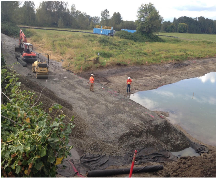
Looking northeast from the bulkhead at the crushed surfacing placed on the south embankment to date. Note Strider staking grade for the embankment cross section with the GPS rover.
