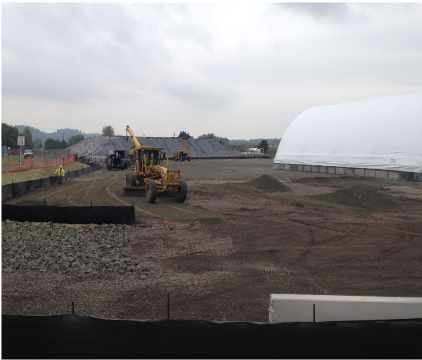
Looking south at the completion of the upland staging and sediment handling area.
