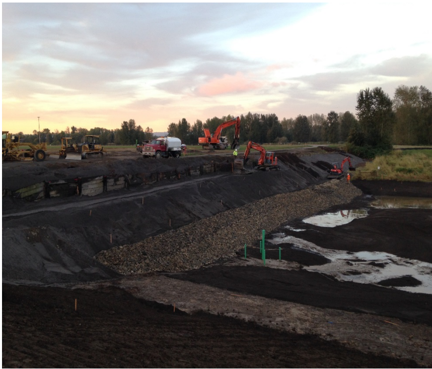
Looking southwest at the extent of structural fill and fish mix rock placed on the south embankment today.
