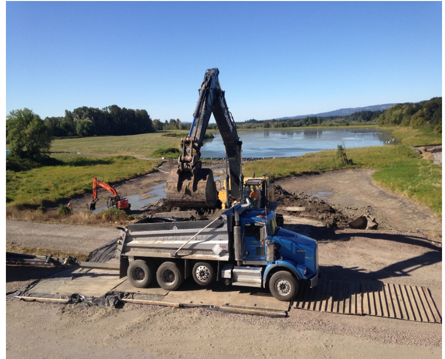
Looking north at a truck getting loaded with sediment for disposal. Note the steel plates, visqueen, and rumble strip.
