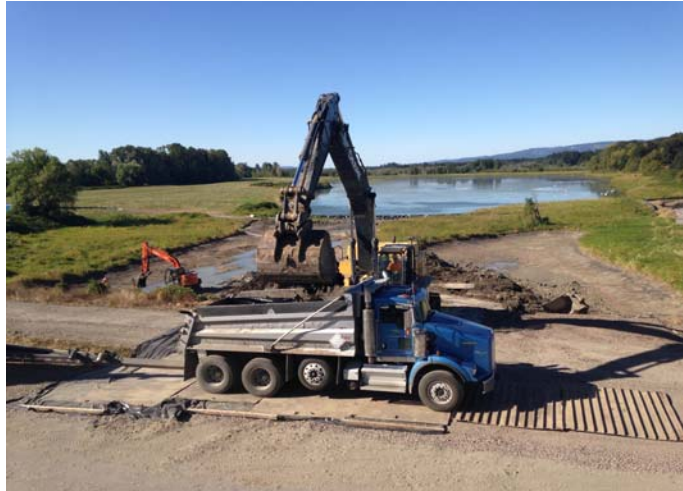
Photo 1: Looking north at a truck getting loaded with sediment for disposal. Note the steel plates, visqueen, and rumble strip.
