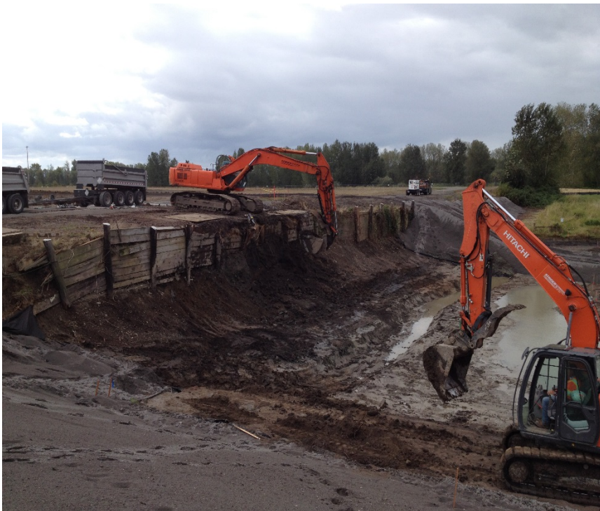
Looking west at the last bit of sediment being loaded into trucks.
