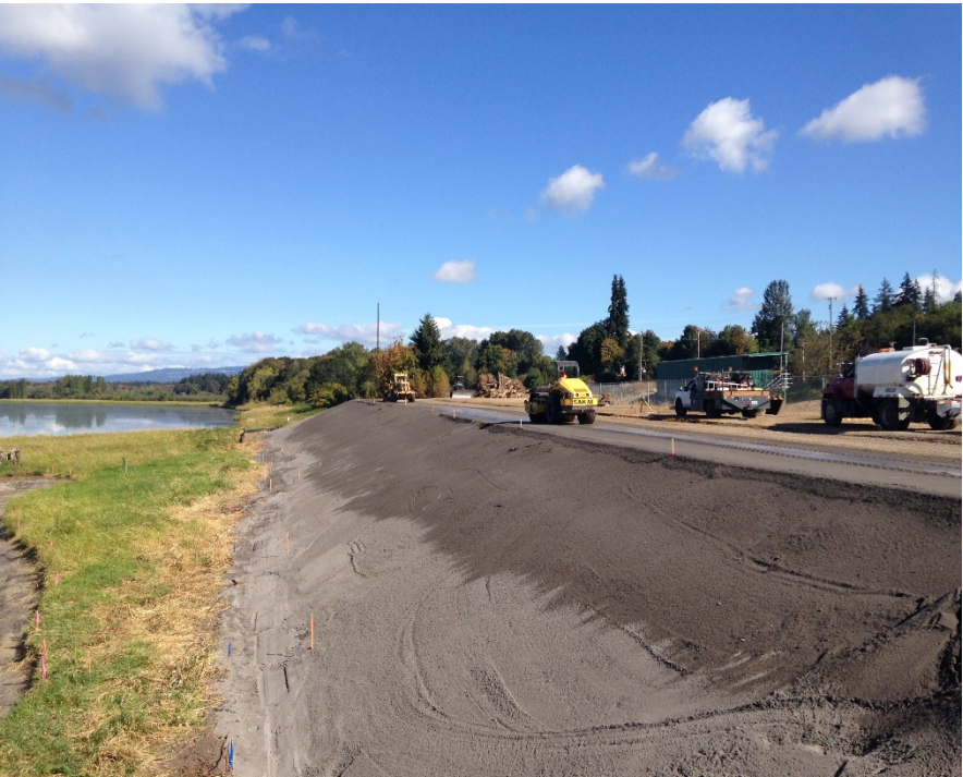
Looking northeast from the bulkhead at the compaction of hard trail subgrade.
