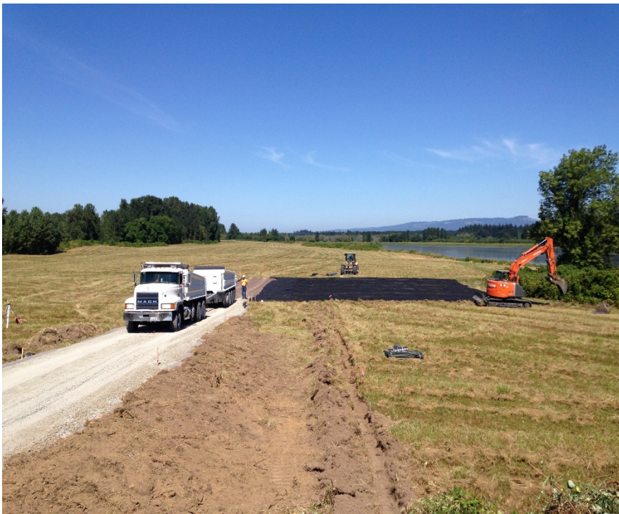
Looking north at the placement of ballast for the temporary equipment staging area.
