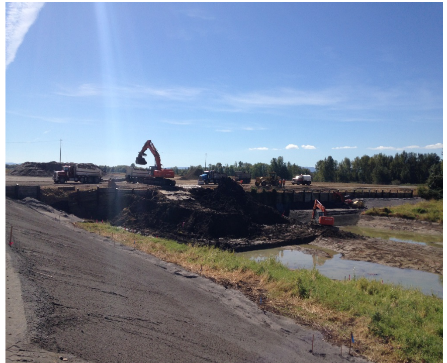
Looking southwest at sediment load-out operations and fill placement for the south embankment. Note the transition from crushed rock to sand at Elev. 12'.
