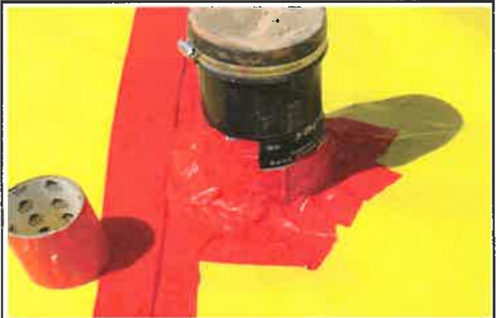
Photo 6. Pipe penetrations taped.
