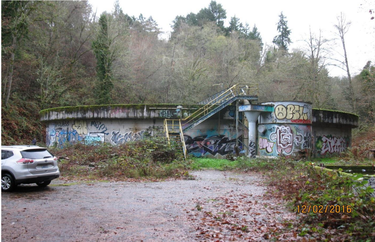
Photo 8: Wastewater/Processed Water Treatment Clarifier – From the East
