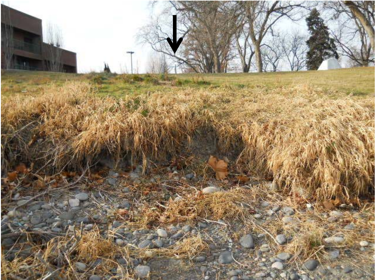
Figure 15. Photo of Cutaway Bank Along Columbia River Downgradient of the Jackpot Food Mart (Looking West. Arrow is pointing to fencepost of fence shown on many of the site maps).
