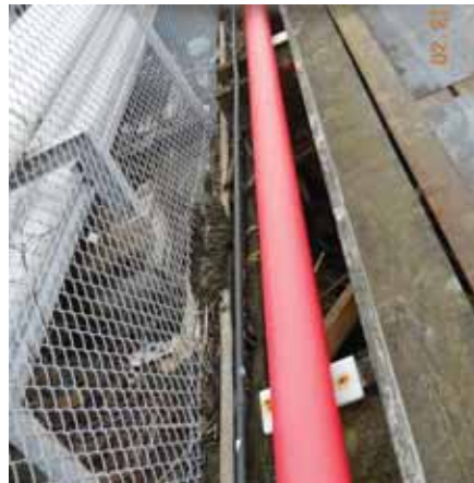
P4 PHOTO - FIRE LINE, ELECTRICAL CONDUIT Ⓧ ABANDONED PIPES
