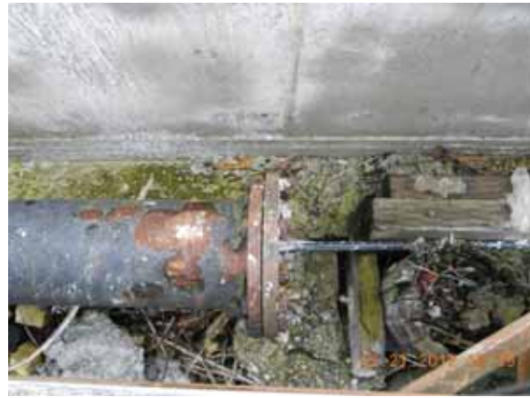
P3 PHOTO - ABANDONED PIPE (ONE SHOWN)
