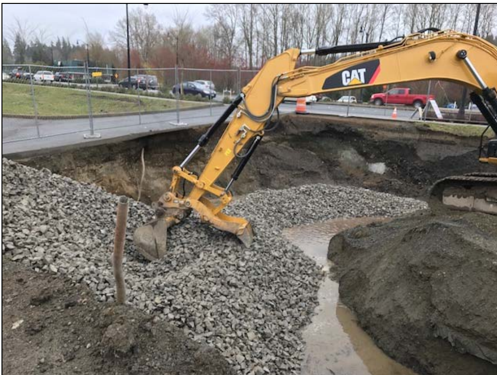
Photograph 4: View facing Southeast toward the March/April 2017 Bothell Riverside remedial excavation during backfilling activities. Quarry spalls were placed in the bottom 1 to 2 feet of the excavation.
