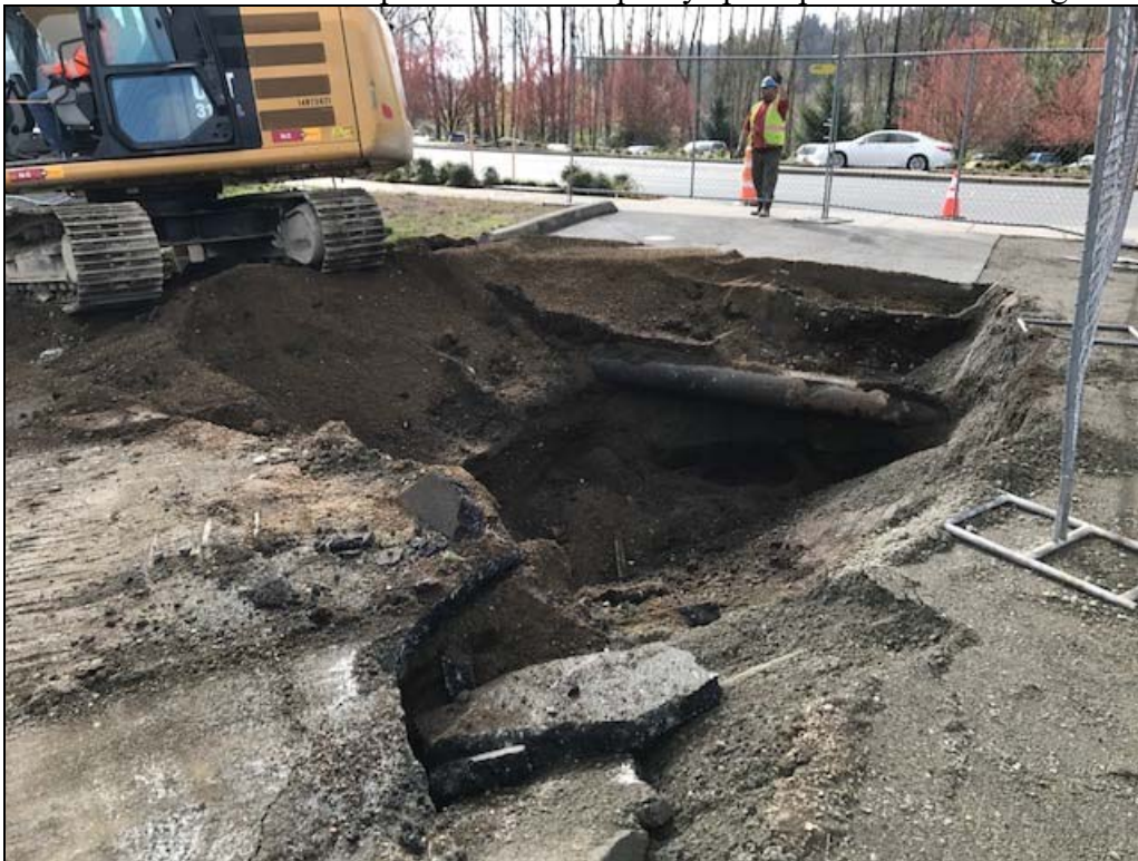
Photograph 6: View facing Southeast toward the March/April 2017 Bothell Riverside remedial excavation. Cleanup efforts continued to the East side of the driveway located just off of State Route 522 leading into the Baskin Robbins and Gallo De Oro Mexican restaurant parking lot.
