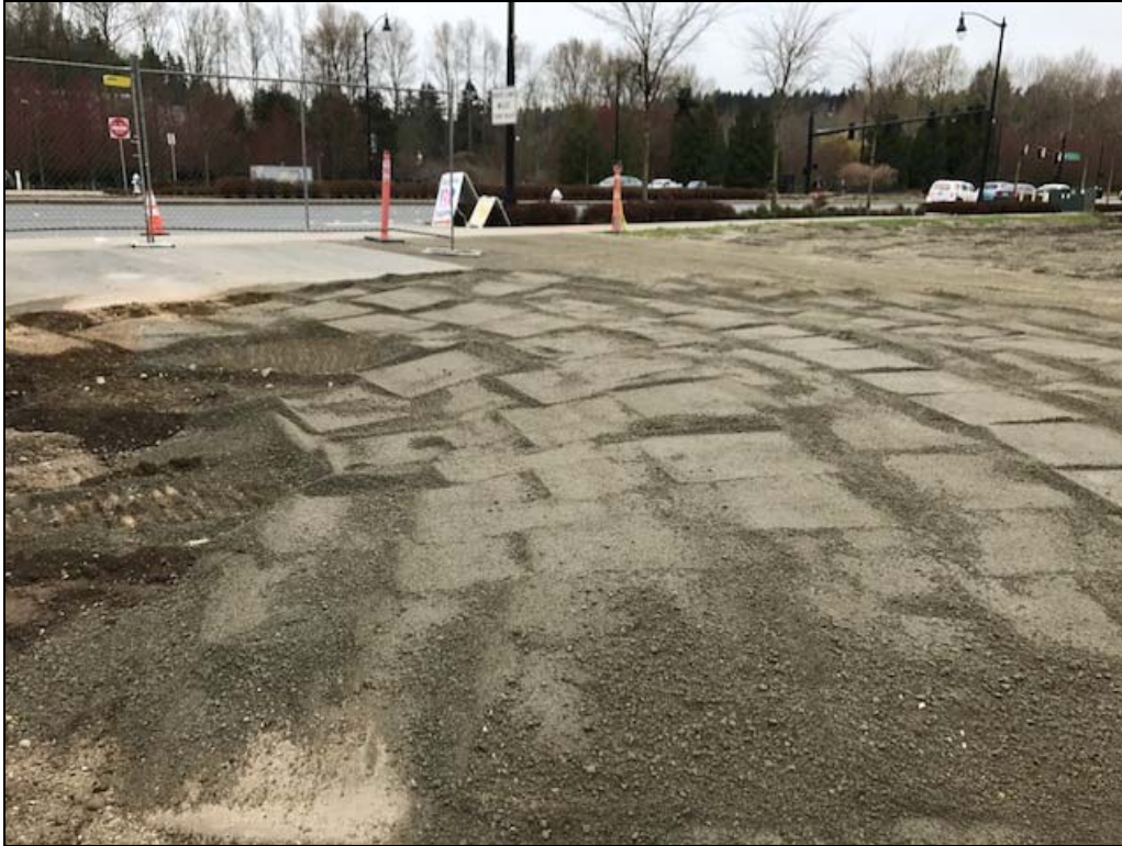
Photograph 7: View facing Southwest toward the March/April 2017 Bothell Riverside remedial excavation during the end backfilling activities. Gravel borrow materials were placed in 10" lifts and compacted from approximately 9' bgs to grade. A layer of 5/8-inch minus crushed rock was placed and compacted in the top six inches of fill where the original paved driveway was located.
