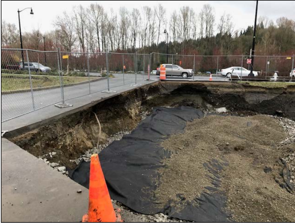
Photograph 5: View facing Southeast toward the March/April 2017 Bothell Riverside remedial excavation during backfilling activities. A filter fabric was placed over the quarry spalls prior to backfilling with gravel borrow.
