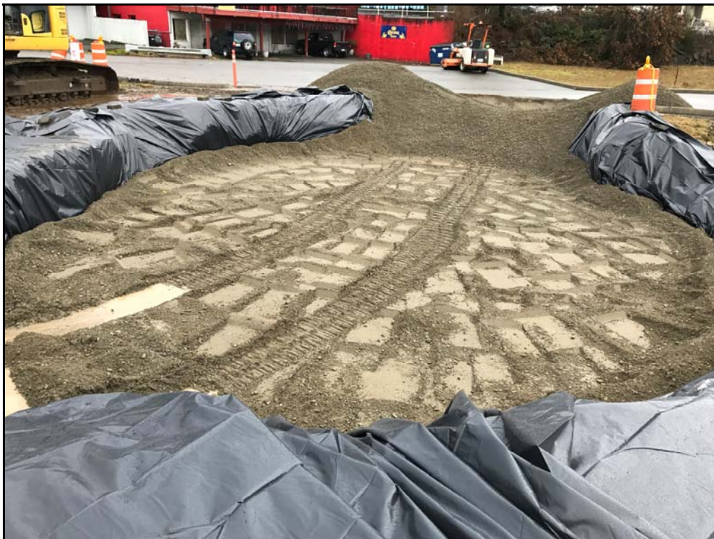
Photograph 2: View facing Northeast toward the January 2017 Bothell Riverside remedial excavation during backfilling activities. Polyethylene sheeting placed in the excavation as an indicator of the boundary between contaminated soils and clean backfill.
