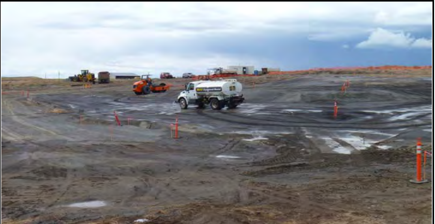
Photo 5: View of the southern edge of G-layer near end of the day with watering truck and roller. Note that former holes in Photo 4 have been backfilled and compacted. View looking west/northwest from AE-5.
