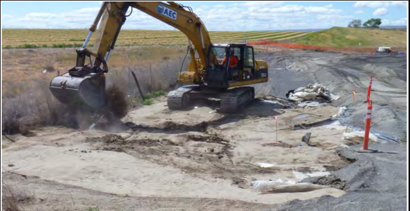
Photo 3: View of AEC trackhoe cleaning up sand area along the eastern edge of the site. View looking south from NE corner.
