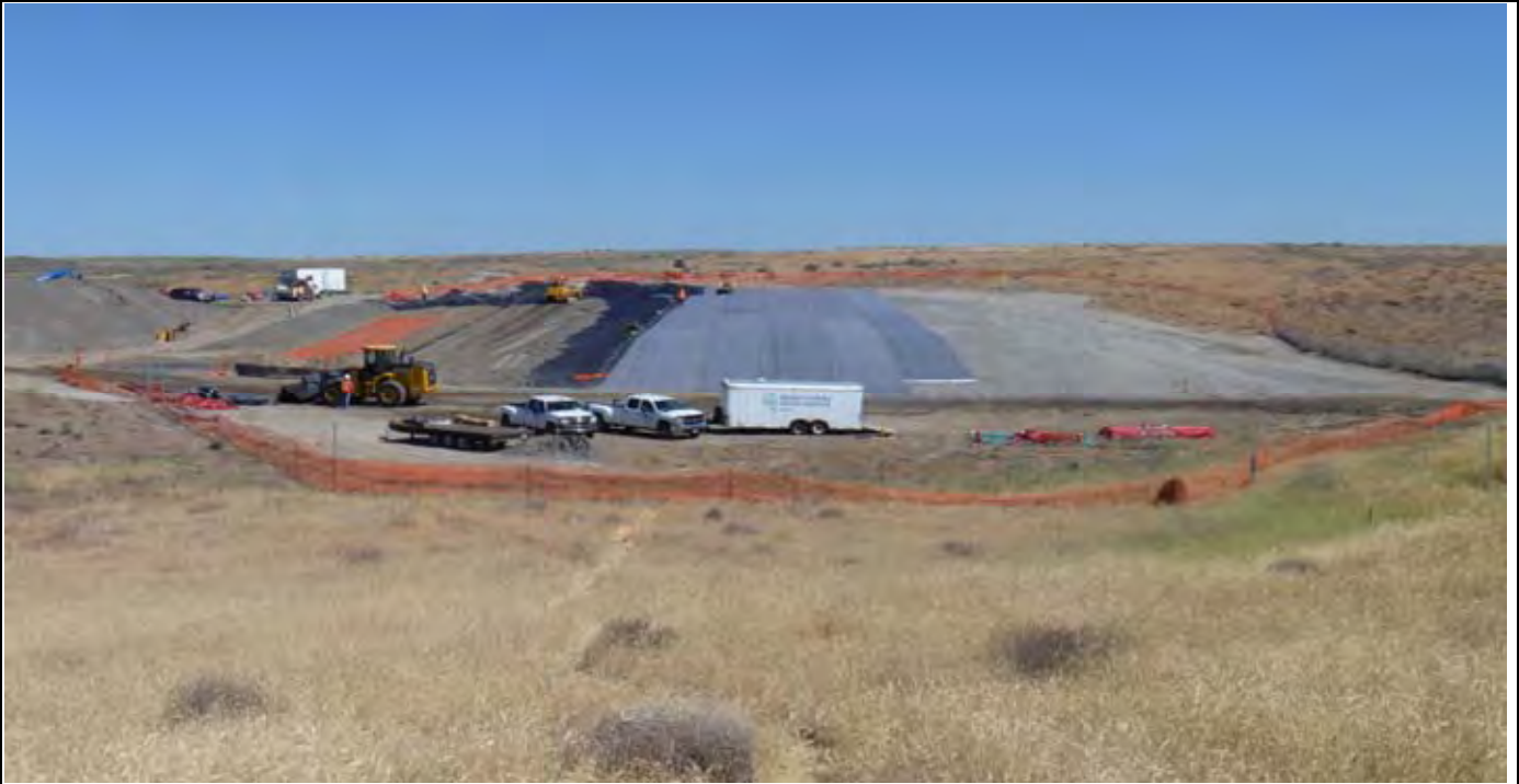
Photo 7: View of the CAP after NWL has exhausted all but three rolls of GCL (left for tomorrow AM work) and is preparing to install geomembrane panels. View looking north from area south of the site.
