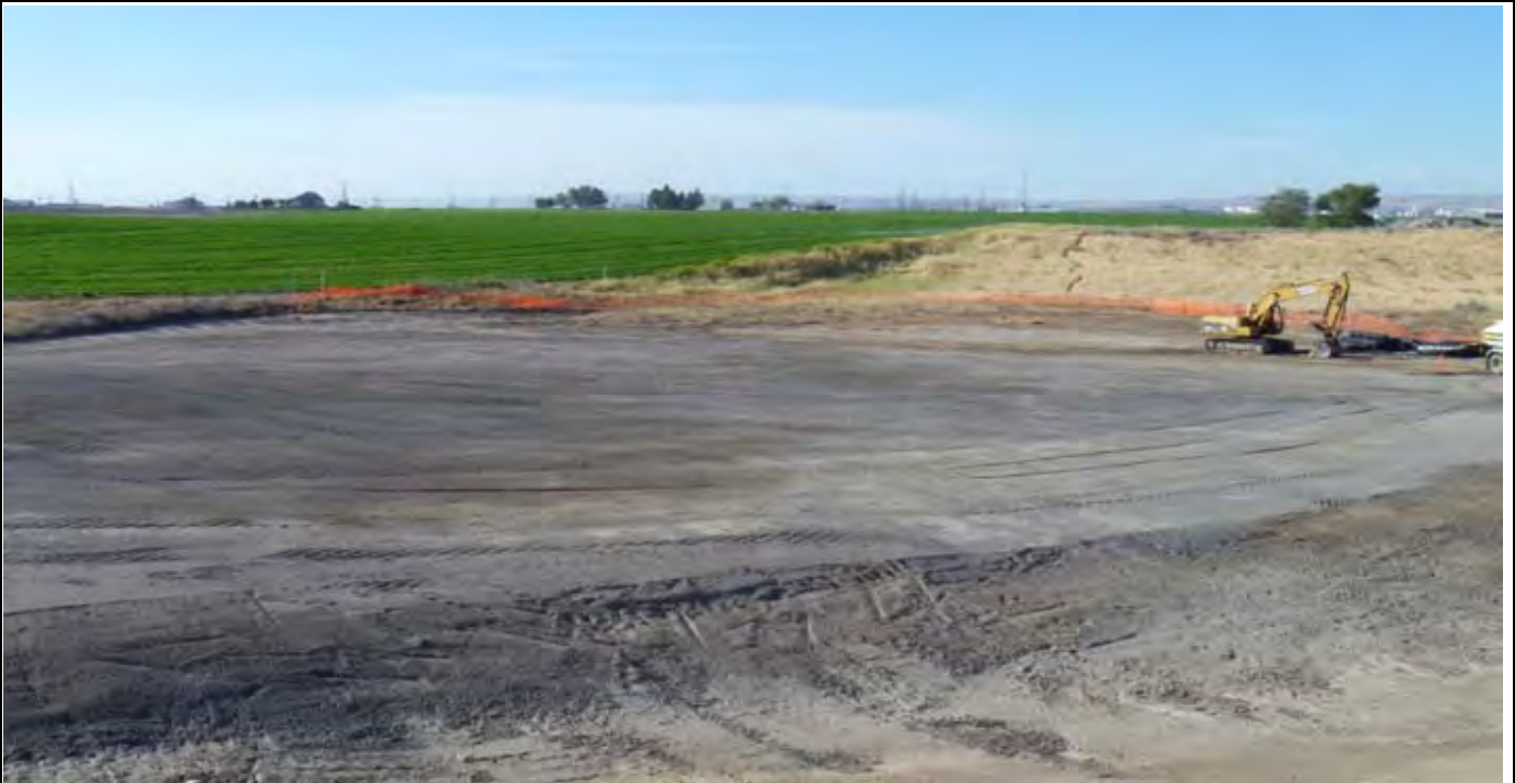
Photo 1: View of the site at the beginning of work for the day. View looking to the South / SE towards the trackhoe.
