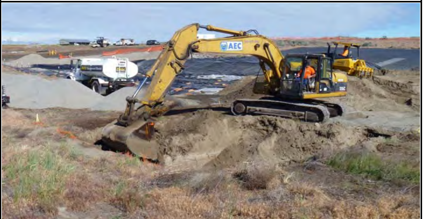
Photo 4: AEC begins the excavation of AE-5 down to 4-ft bgs. View of AE-5 looking to the north/northwest.
