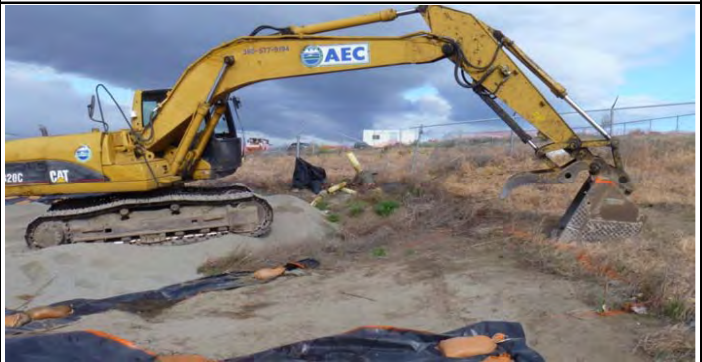
Photo 2: AEC preparing to excavate AE-3 (see triangular area with orange paint outline and cut out liner). View looking to the west from the eastern edge of the site.
