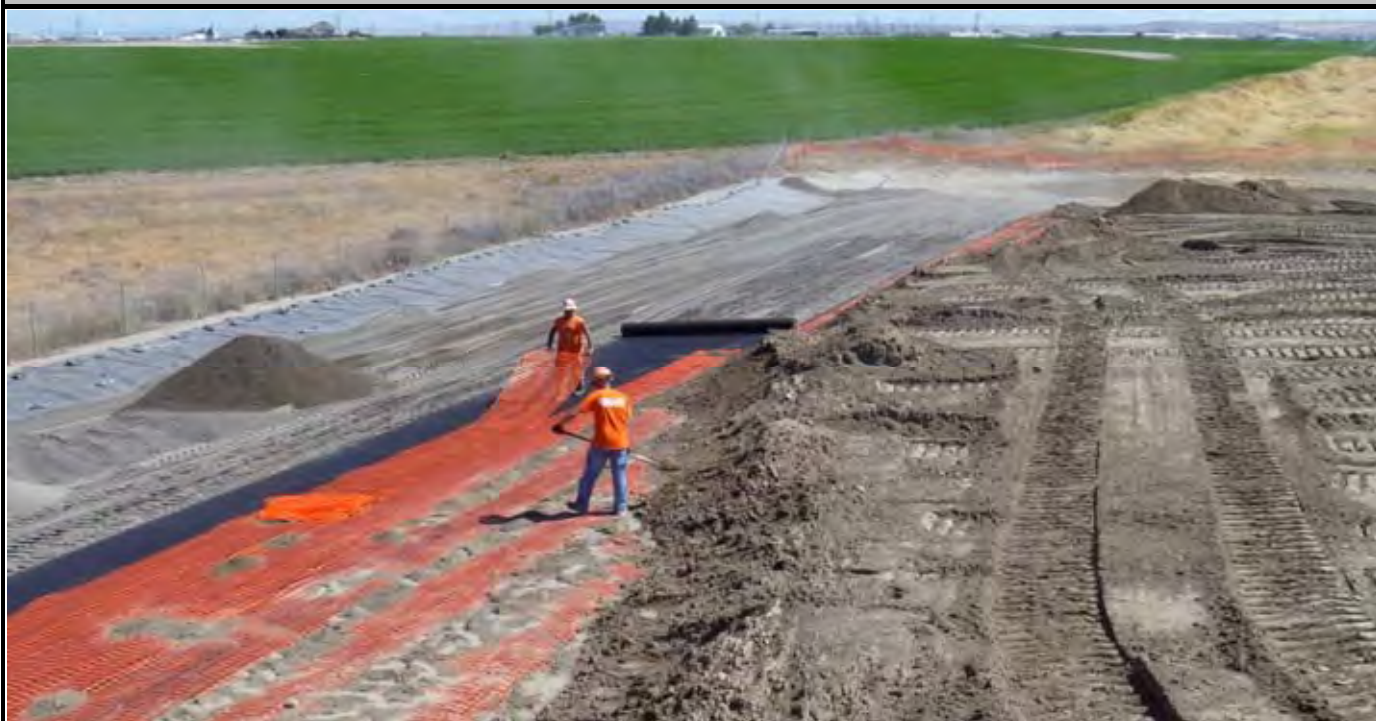
Photo 7: View of AEC personnel laying out Geo-Fabric and OCF over recently graded sand layer. View looking south/southeast from area east of the center of the CAP.
