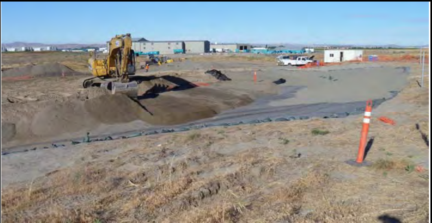
Photo 7: View of the northern swale area as AEC grades the EOC into the swale with topsoil and sand layers. Note the Geo-Fabric and perimeter rock layer installed on NW corner of the swale. View looking west/southwest from area along the northern end of the site.
