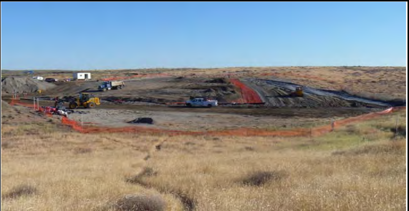
Photo 1: View of the site at the beginning of work for the day. View looking to the north from area south of the site. Note extent of topsoil layer (west edge of OCF shows it) and sand layer (see bulldozer grading it).
