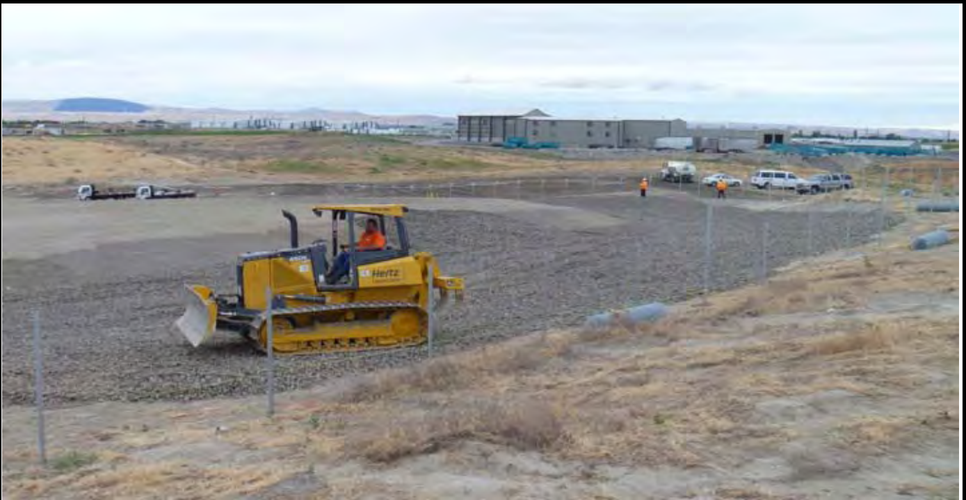
Photo 5: View of AEC using the bulldozer to complete finish grading and smoothing of the perimeter erosion rock and Rick's custom fencing installing the top bar and bar wire mounts to posts along the western perimeter of the CAP. View looking southwest from area north of the site.
