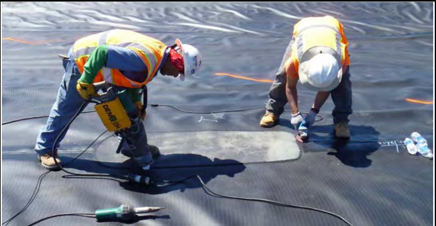
Photo 13: View of NWL installing patch around an area of seam S-2 that was removed for testing. Note tool on left that extrudes bead of molten HDPE along the edge of the patch. Patch was vacuum tested and passed the test and seam S-2 approved. View looking west from geomembrane pass P-3.
