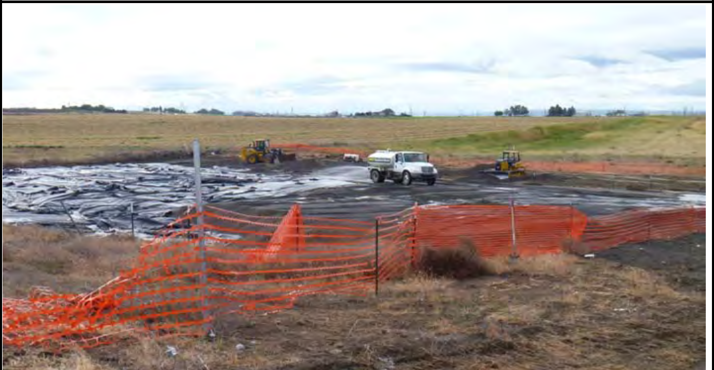
Photo 4: View of AEC water truck wetting down G-layer materials on cap. View looking to the southeast.
