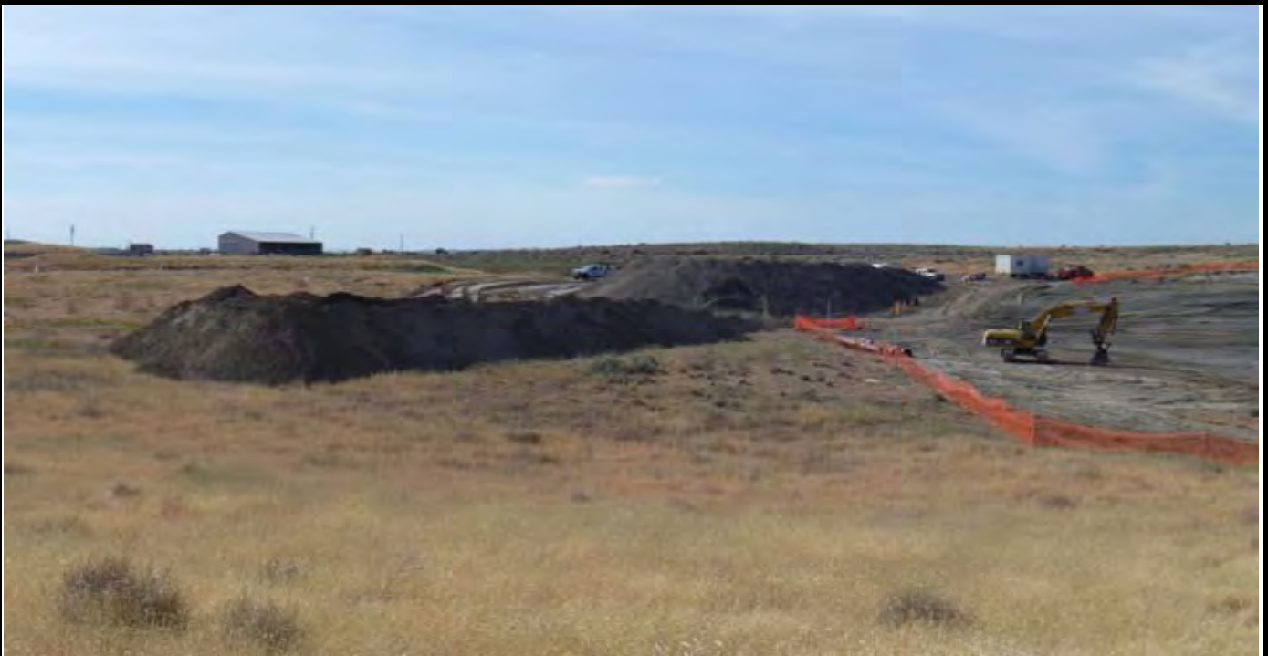
Photo 9: View of the topsoil (front) and sand (back) stockpiles at the end of the work day and three new rolls of geomembrane (left of trackhoe). Note that the other two geomembrane rolls are stockpiled up on the road and will be brought down to the others tomorrow. View looking NW from area south of the site.
