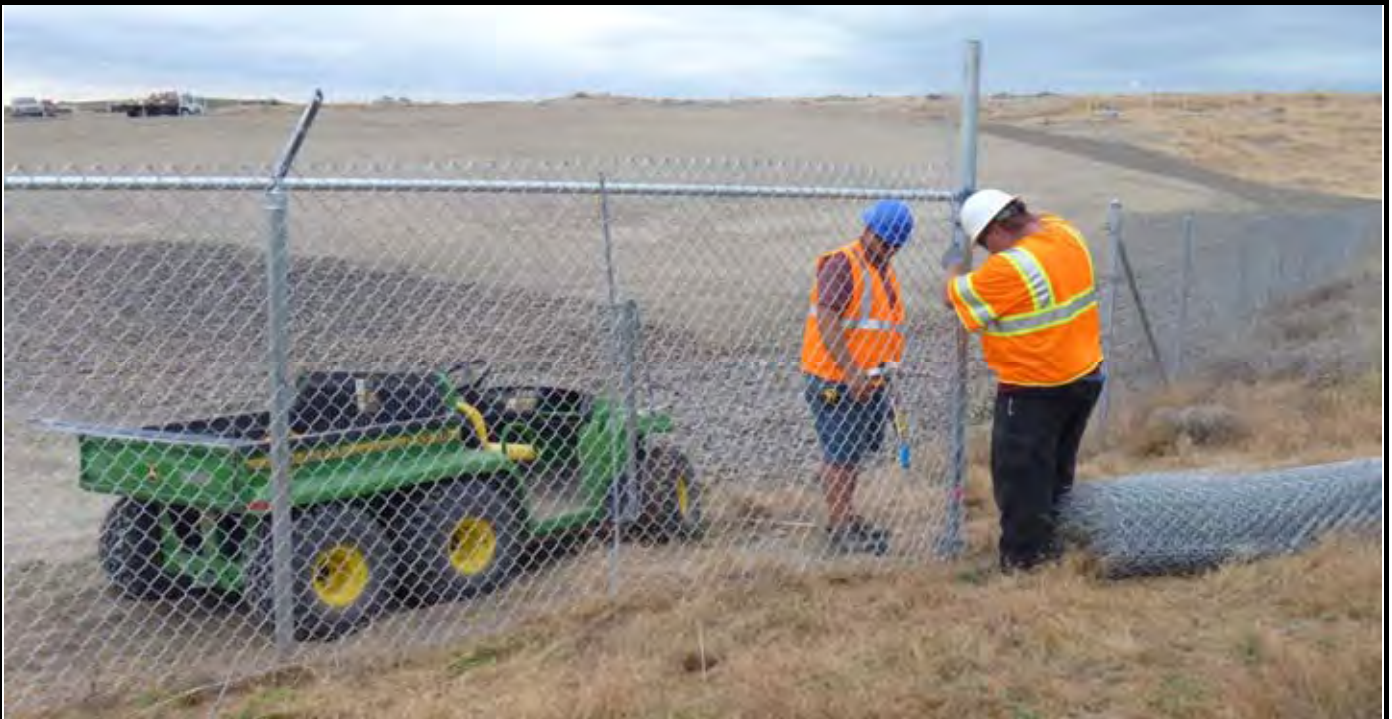
Photo 7: View of Rick's Custom Fencing beginning the installation of the first couple rolls of cyclone fencing material. Note the winch and spreader bar pulling the fencing to the post. View of area along SE corner of the CAP looking to the North/Northwest.
