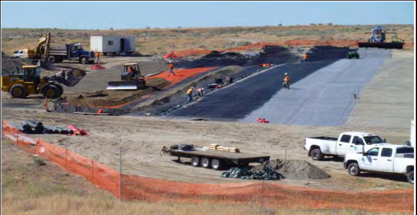
Photo 17: View of western side of the CAP showing NWL installing fifth pass (P-5) of geomembrane and AEC installing topsoil over orange construction fencing (OCF) visual barrier over the Geo-fabric and sand layer along the western edge of the CAP. View looking north by northwest from area south of the southern edge of the infiltration basin (area just inside the installed OCF in foreground).
