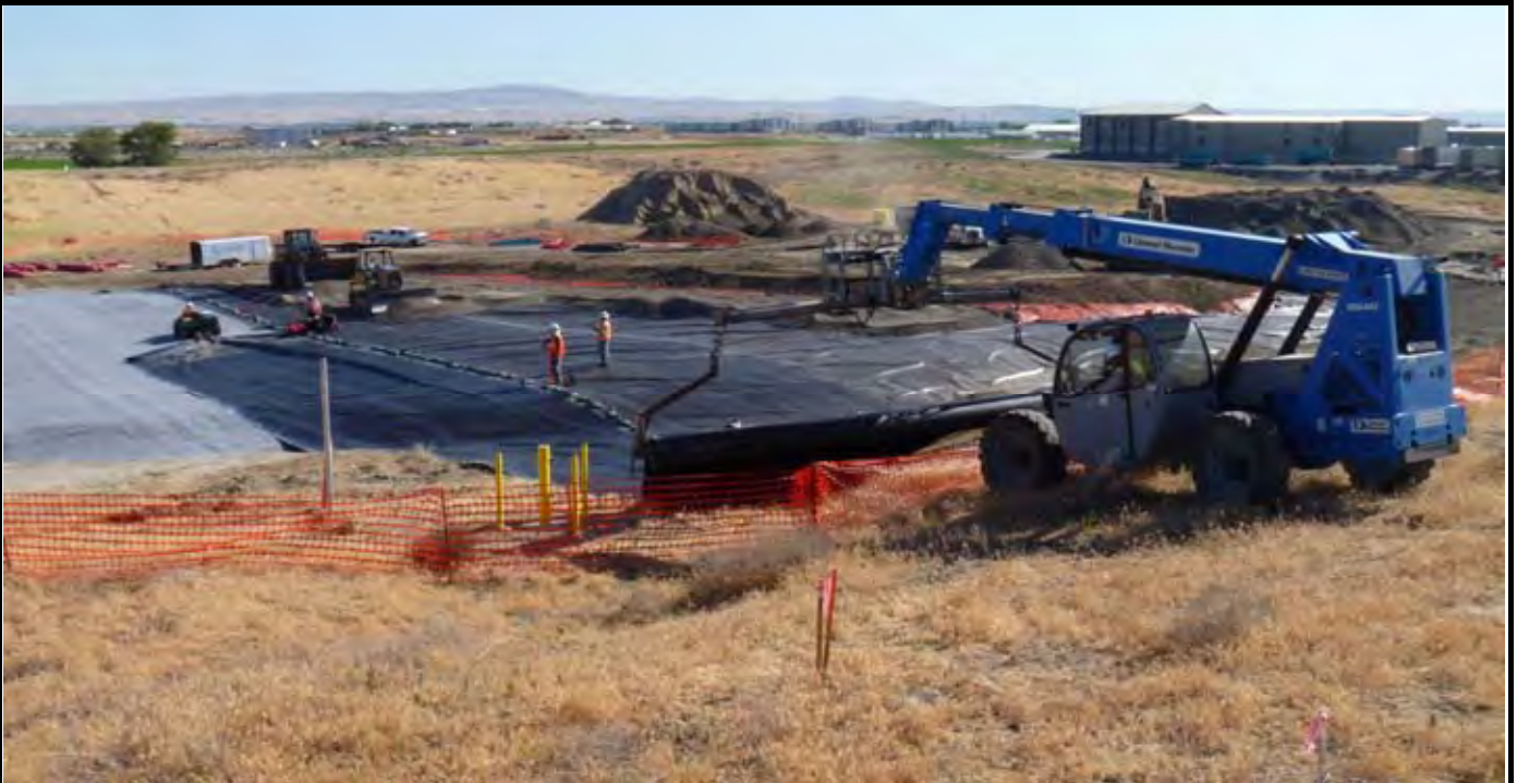
Photo 9: View of NWL laying out geomembrane panel from northern edge of the site with telehandler and JD Gator. Note AEC in background grading and spreading sand layer near the existing eastern edge of the geomembrane. View looking south/southwest from area north of the site.
