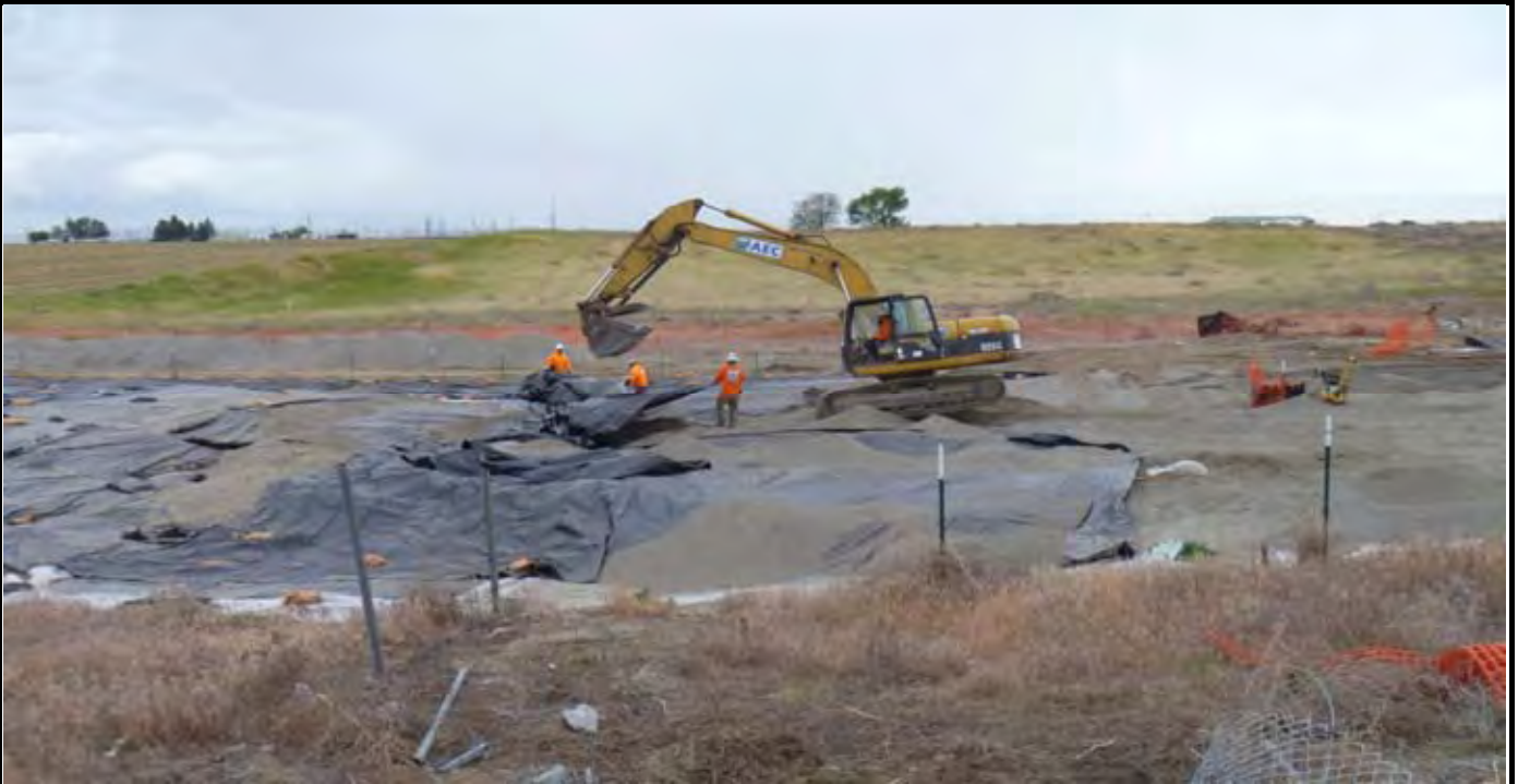
Photo 9: AEC laying out 12-mil liner over the AE-1 and AE-2 excavated soils. AEC uses clean gravel to hold down the edges and middle of the liner. View looking south from north side of the site.
