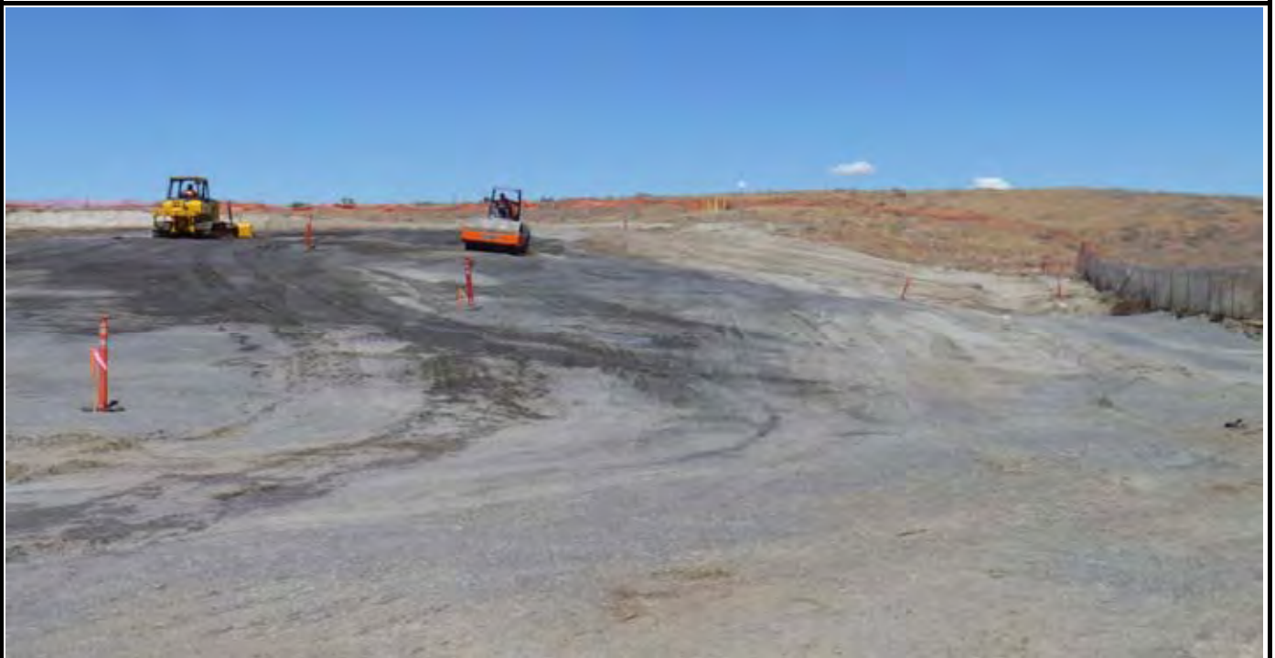
Photo 4: View of the eastern side nearing completion and the NE corner / swale area after grubbing completed. View looking north from the SE corner of the site.
