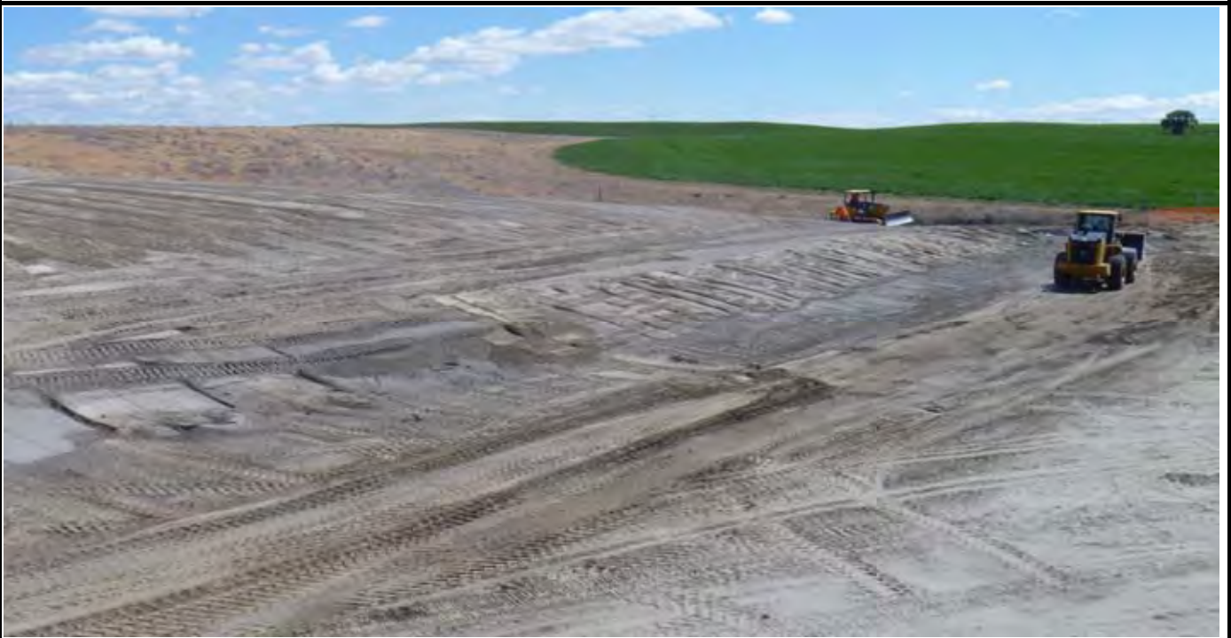
Photo 6: View of the rough grading along the southern EOC to EOL and almost ready to accept perimeter rock. Note AEC equipment nearly completing eastern swale rock work. View looking east/NE from rock pile SW of the SW corner of the CAP.
