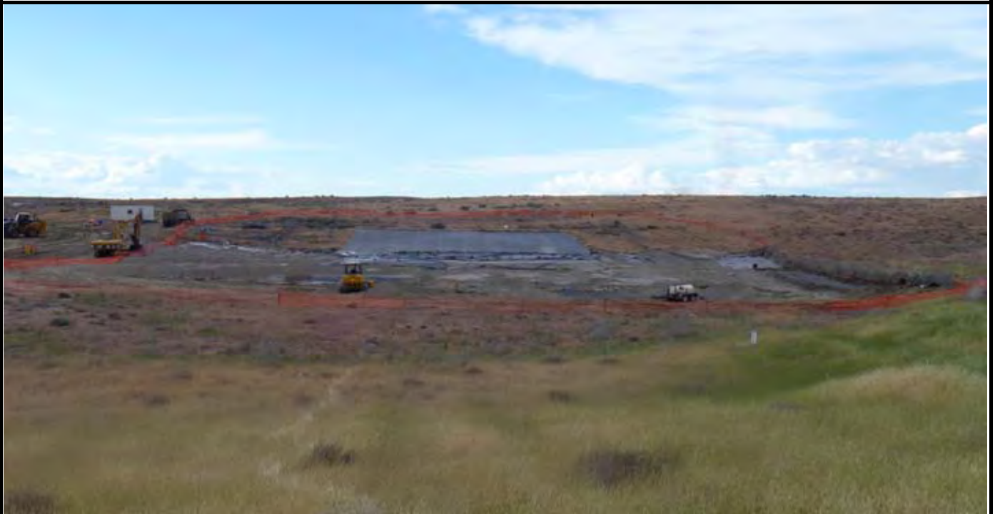
Photo 10: View of the site at the conclusion of work for the day. Orange construction fence is up around the site and the 12-mil tarps covering the excavated soils is covered mostly with gravel. View of the site looking north.
