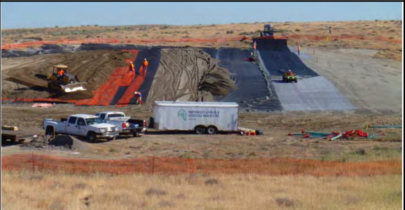
Photo 4: NWL laying out first panel from geomembrane roll #4. Note NWL using JD Gator to pull roll downhill (south) over GCL later. Note AEC laying out OCF over Geo-Fabric (center) and sand layer. View looking north from area south of the south end of site.
