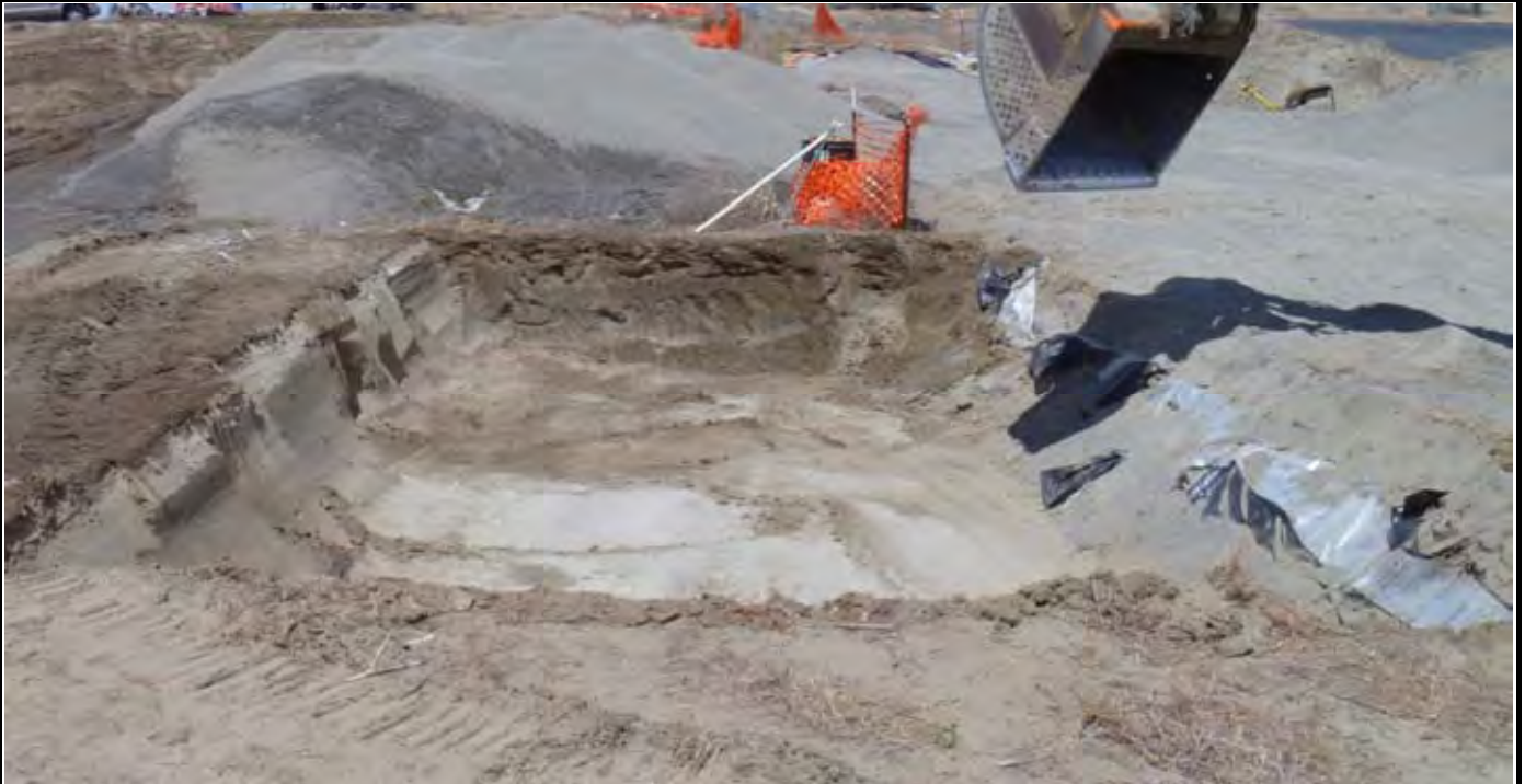
Photo 7: View of AE-1 after final 5-ft bgs excavation work. Note gravel stockpiles that will be used for backfilling AE-1 and AE-2. View looking north from south side of AE-1.
