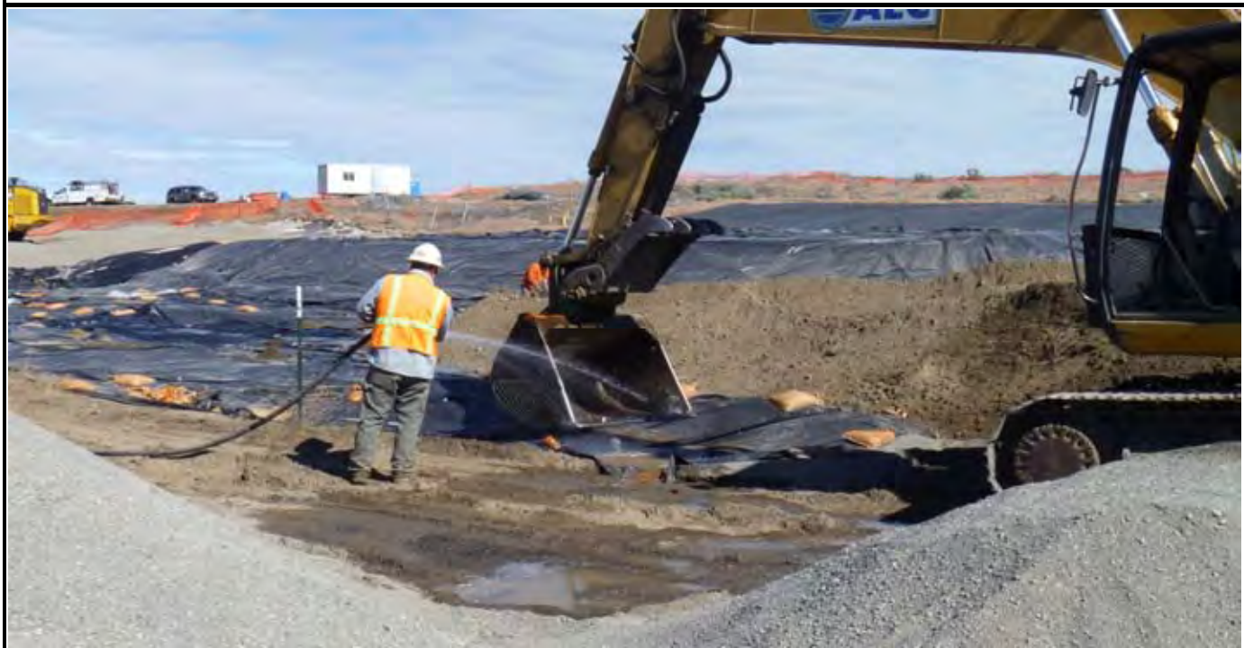
Photo 6: View of AEC decontaminating the trackhoe bucket over the containment sump. View looking to the northwest towards the job trailer.
