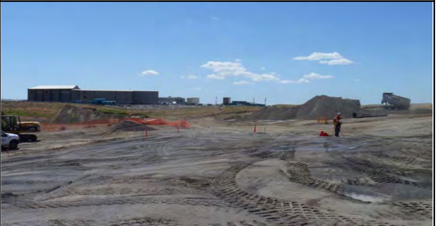
Photo 4: View of AEC's surveyor (Tim Scott) installing grade control points with topsoil (left) and sand (right) layer stockpiles behind him. View looking west from eastern side of the cap.
