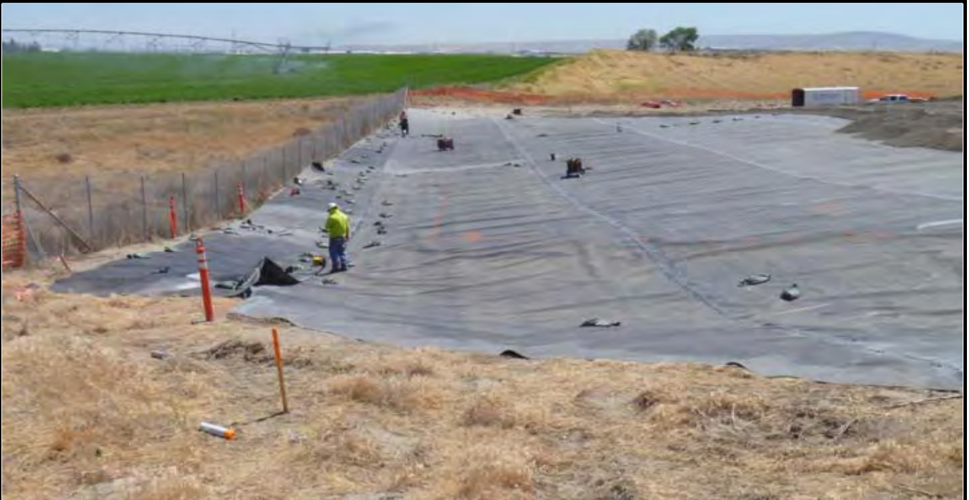
Photo 7: View of the installation and welding (see yellow worker in center of picture) of seam between geomembrane panels P-13 and P-14 (both panels required butt joint welding). Note that geomembrane panel P-14 is installed all the way to the fence line. View looking south from area just north of the NE corner of the EOL.
