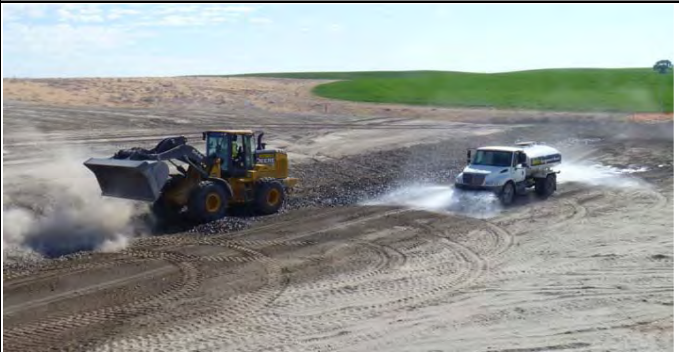
Photo 2: View of AEC placing erosion protection rock and watering along the southern EOL / Cap. View looking NE from area SW of the CAP.
