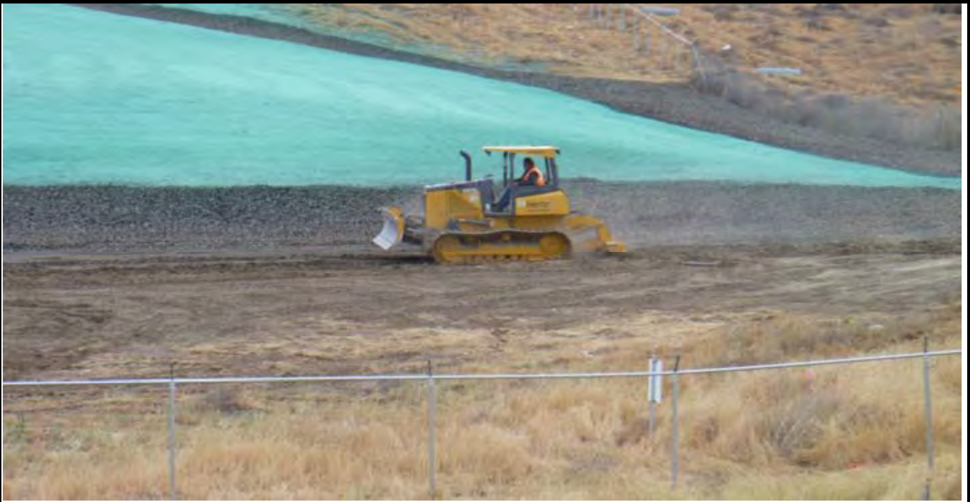
Photo 7: View of AEC using bulldozer to plow the infiltration basin area to break up the surface soils to allow for easier infiltration of precipitation. View of the southern side of the CAP from area south of the site.
