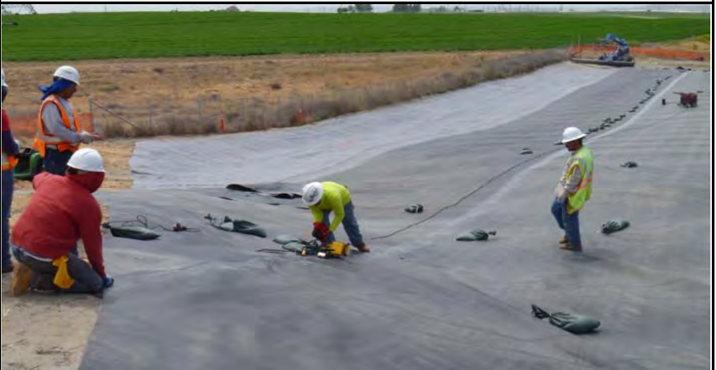
Photo 6: View of NWL starting seam weld between geomembrane panels P-11 and P-12. View looking SE from northern edge of EOL. Note small yellow seam welding machine in center of picture.
