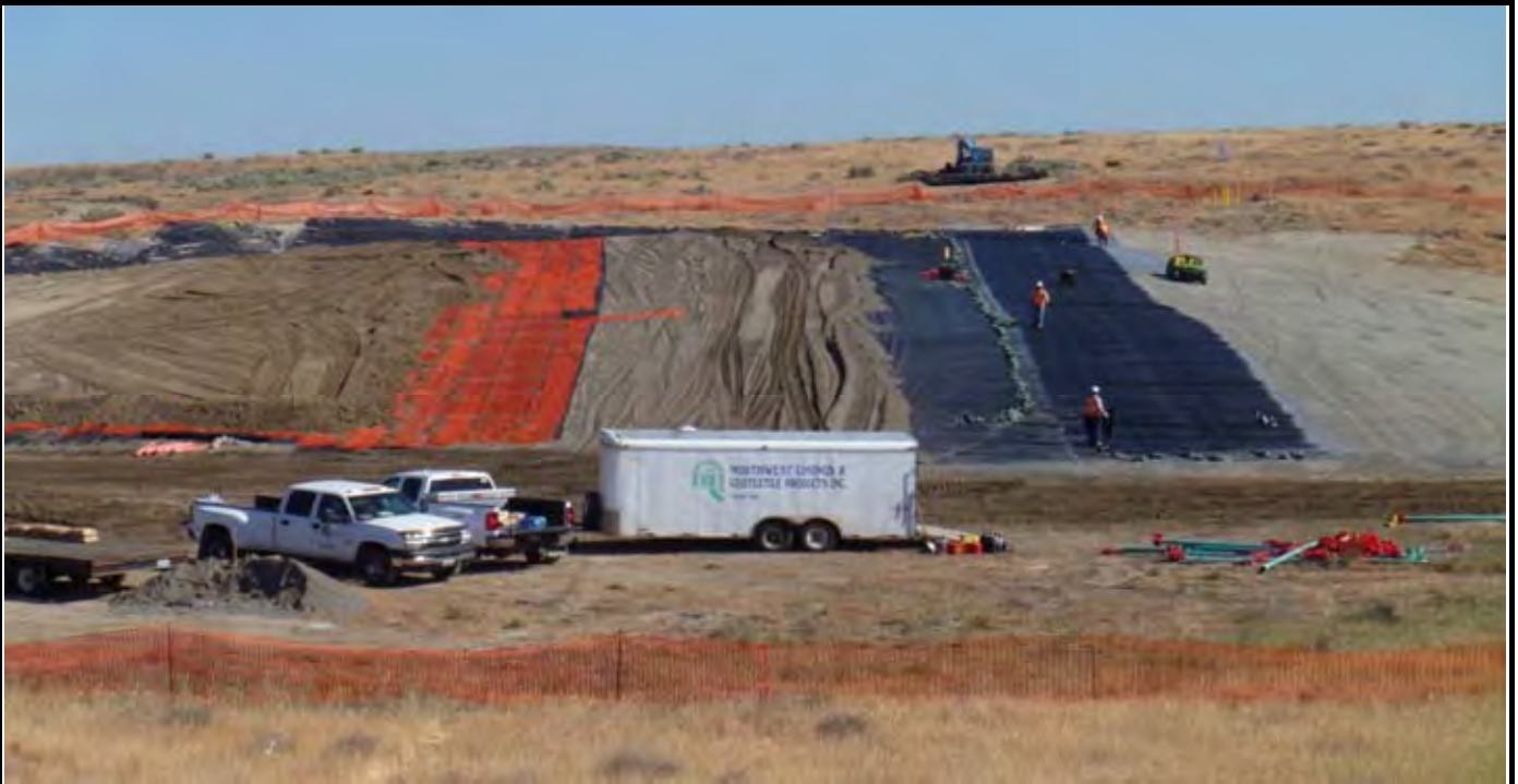
Photo 5: View of geomembrane panel fully laid out and ready for seam welding. NWL is moving sandbags to eastern edge of geomembrane panel. AEC ready for topsoil placement over OCF layer. View looking north from area south of the site.
