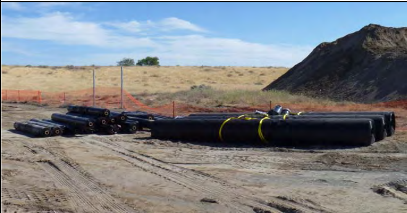
Photo 8: View of 3 geomembrane rolls (new ones) and 20 geosynthetic rolls stockpiles in area just SW of the SW corner of the CAP. Note the double fence posts in background for fence gate. View looking south from the SW corner of the CAP.
