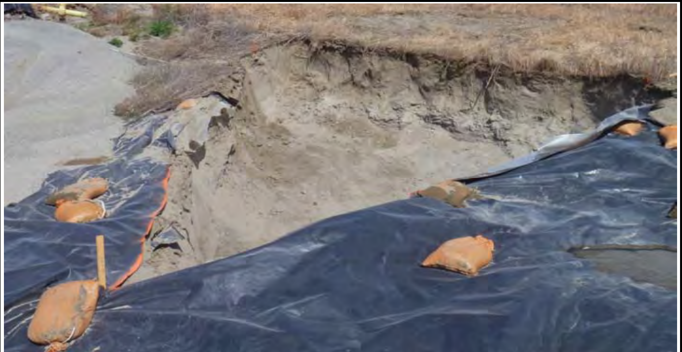
Photo 4: AE-3 after final 5-ft bgs excavation work. View looking NW from SE corner of AE-3.
