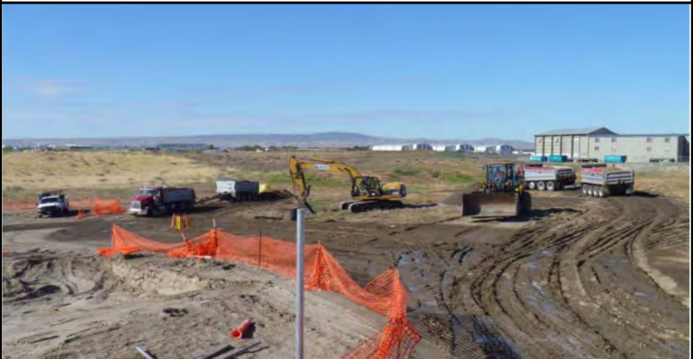
Photo 2: View of the first sand (interior of "loop" - trackhoe is in "loop") and topsoil (down below sand - see red truck) stockpiles on the site. View looking to the SW from the NW corner of the site.
