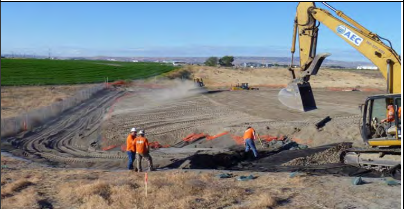
Photo 2: AEC grading perimeter swale sand and laying out Geo-Fabric and perimeter rock on Northeastern swale. View looking south from NE corner of the site.
