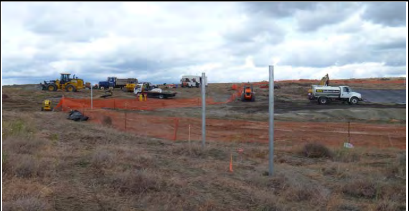
Photo 5: View of new fence corner posts (two in foreground are for new double gate on SW site of perimeter). View looking north from SW corner of site.
