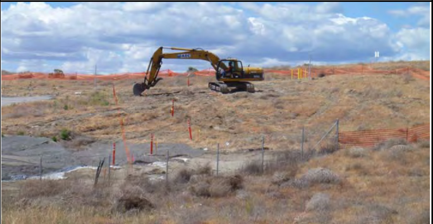
Photo 4: AEC begins grubbing for NE swale area. Note orange lines that locate the EOL and EOC for the NE swale. View looking North to Northwest from east side of site.
