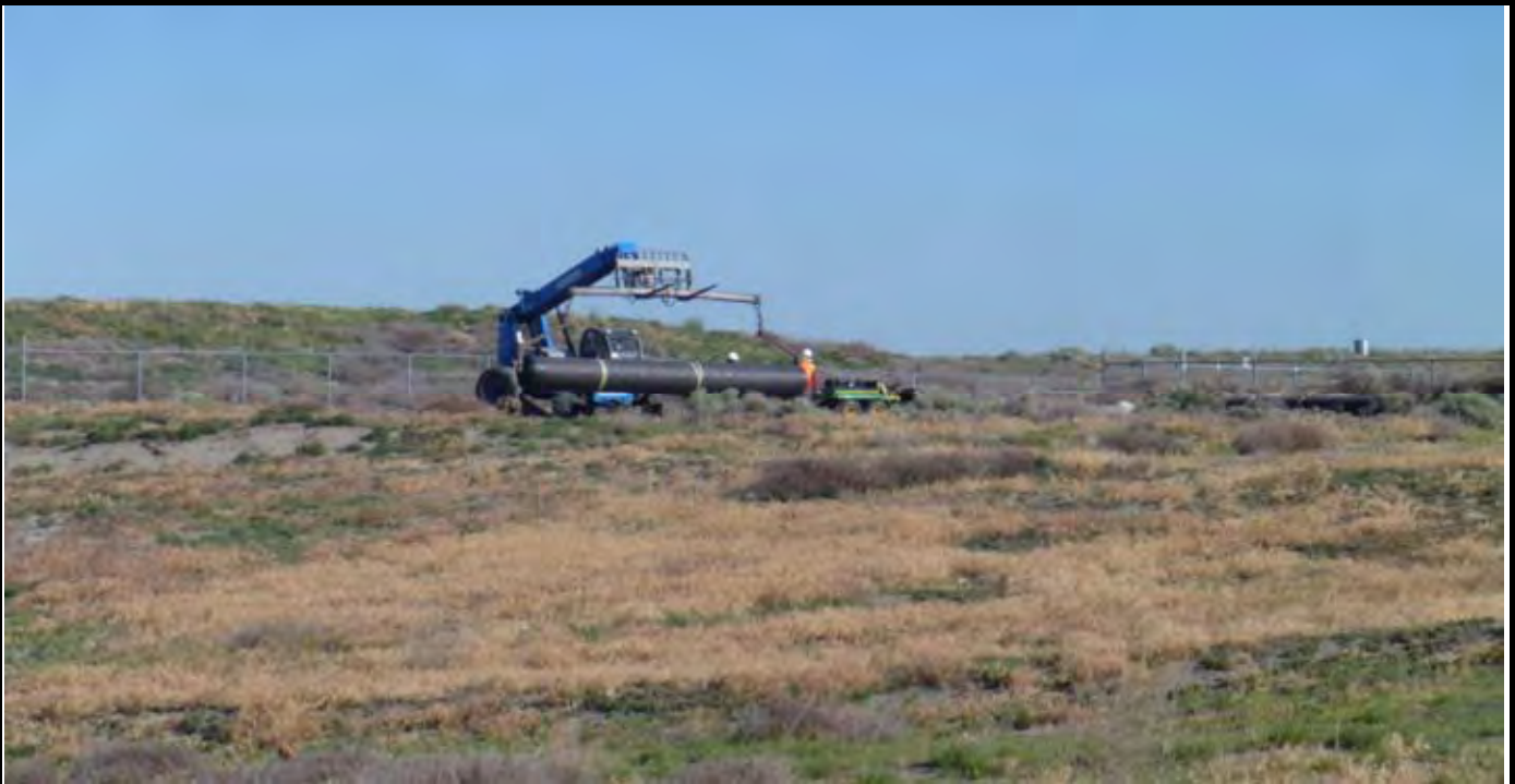
Photo 3: View of NWL recovering geomembrane roll #4 (one of two original rolls) from stockpile area along entry roadway. View looking north to northwest from area adjacent to job trailer (west of NW corner of CAP).
