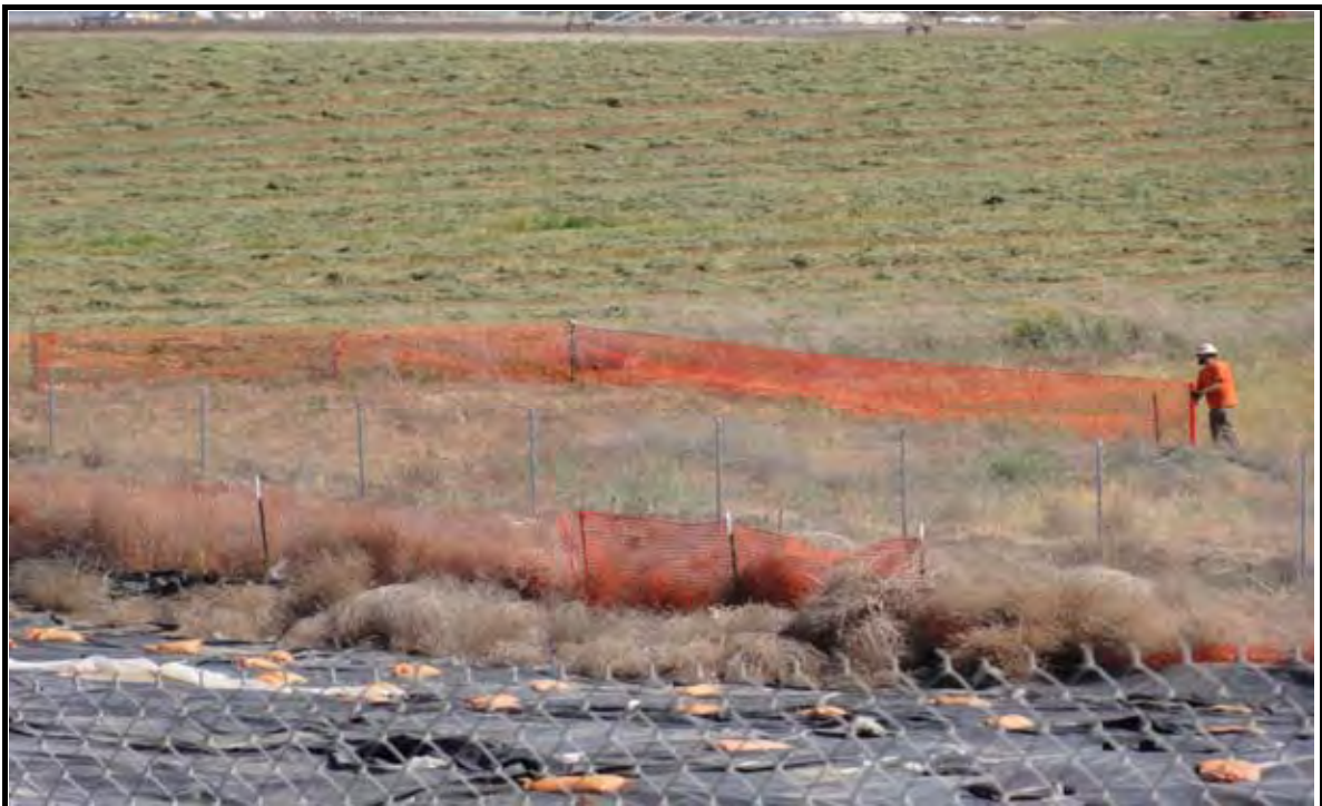
Photo 4: Installation of orange construction fence around perimeter of construction zone near the southeast corner of the site. Fence mounted to new T-bars. View looking southeast.
