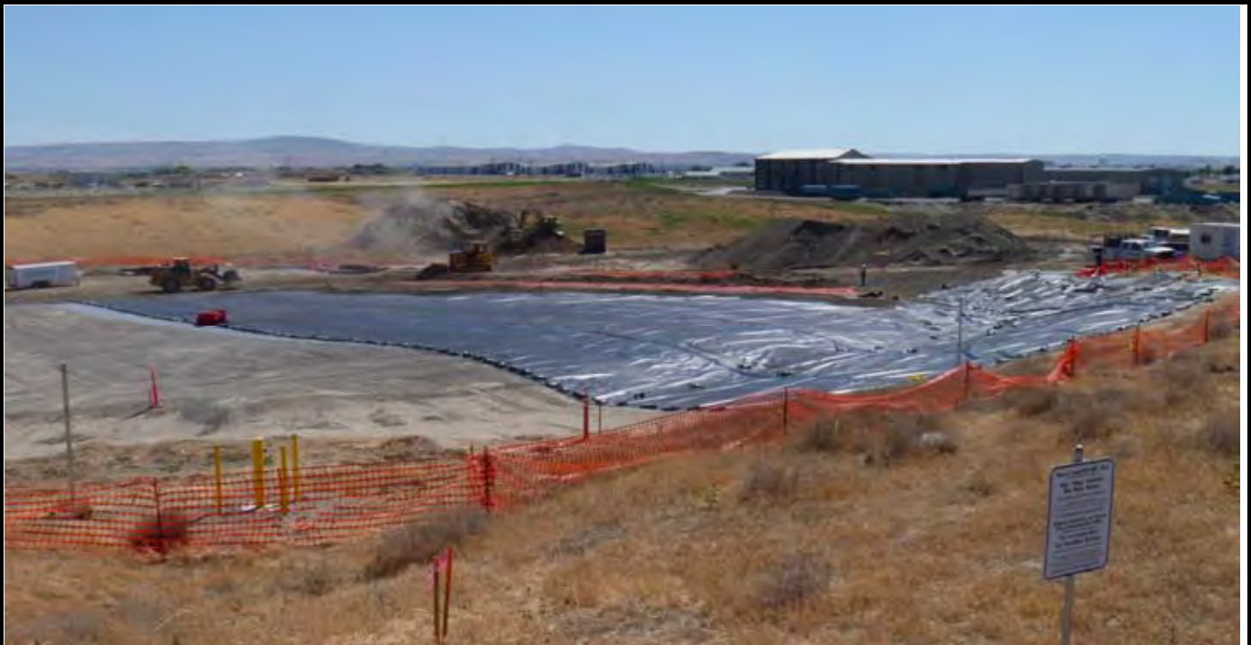
Photo 9: View of the CAP after NWL completes their work for the day. Note sand bags along the outer perimeter of the geomembrane. Note AEC grading topsoil over OCF/geo-fabric layer in background. AEC trackhoe loading AEC dump truck with topsoil and AEC loader moving sand. View looking SW from area NE of the site.
