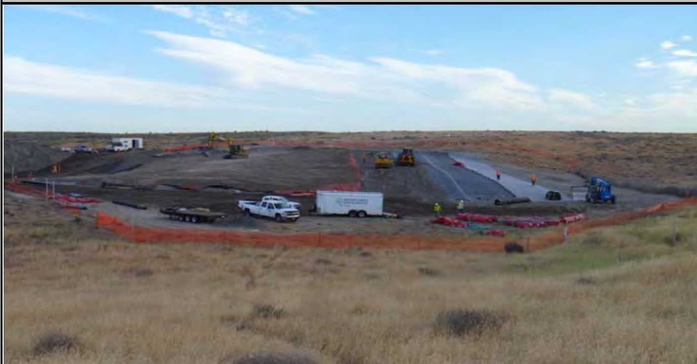
Photo 1: View of the site at the beginning of work for the day. Note NWL setting up to begin rolling out GCL layer on the eastern side of the CAP. View looking north from area south of the south side of the site. Note AEC spreading and grading sand layer just to the west of NWL's workers.
