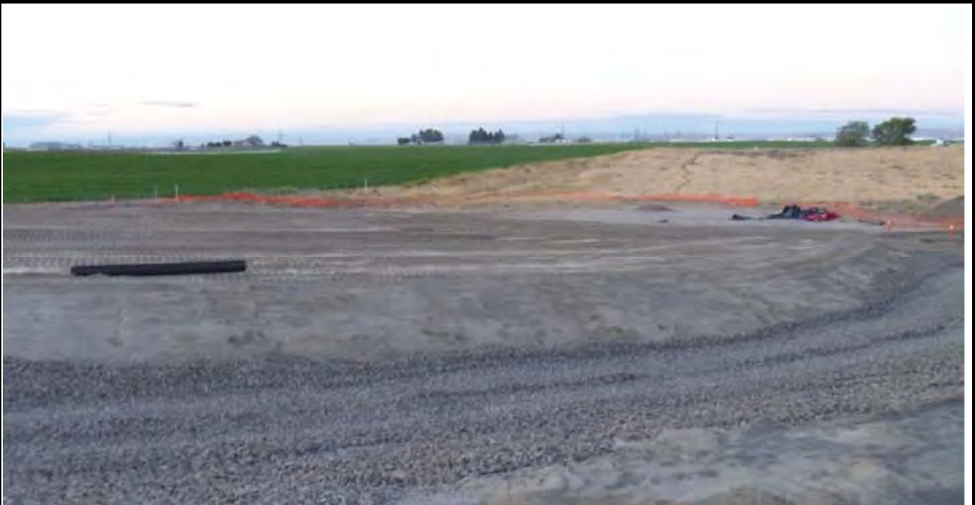
Photo 1: View of the site at the beginning of work for the day. View looking to the south. Note the perimeter rock in the NW and western swale adjacent to the NW side of the CAP.
