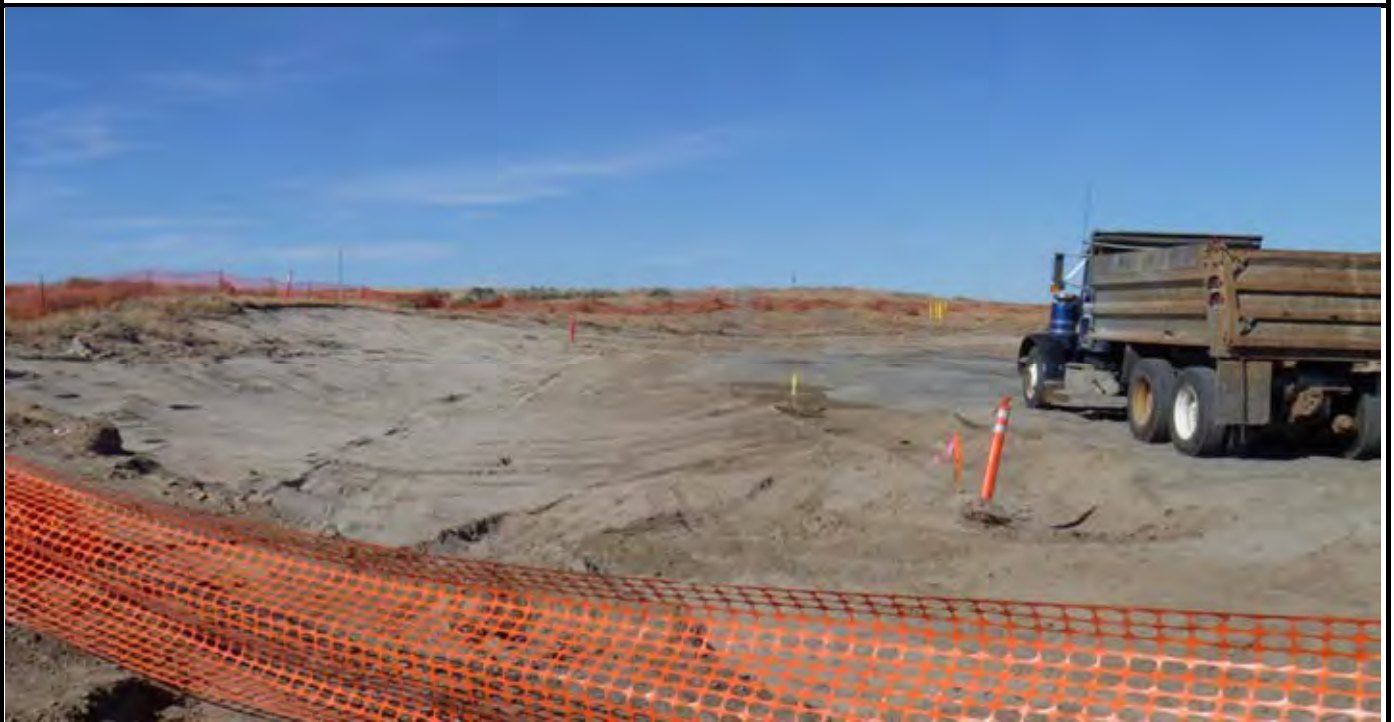
Photo 6: View of the NW corner of the liner extension/swale area after grubbing work. View looking NE from the western side of the site.
