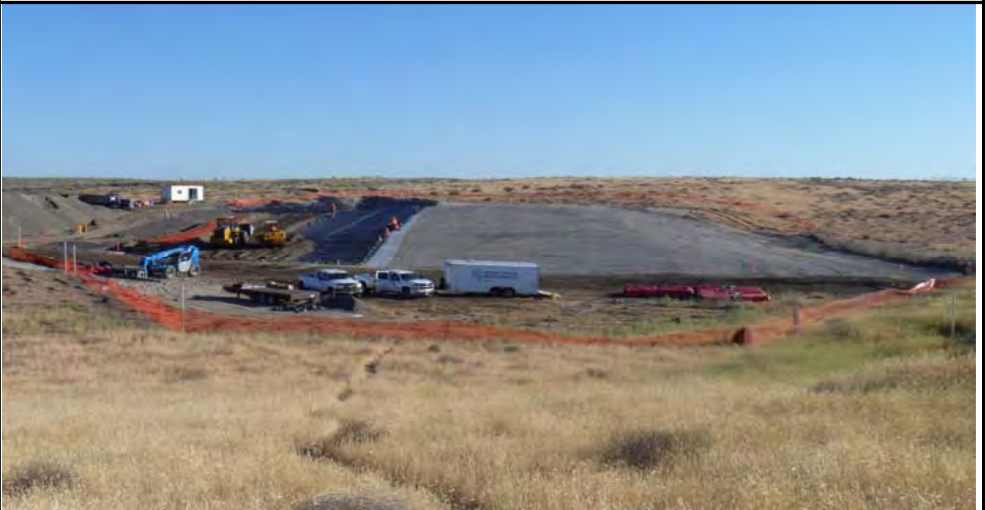
Photo 2: Status of the liner cover at 7AM when NWL crew arrives and begins to install more GCL rolls (see red rolls along southern edge of CAP). View looking North from area south of site.
