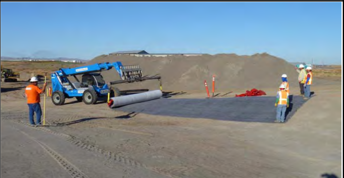
Photo 2: NWL rolling out the first GCL roll with telehandler along the western Edge of Liner (EOL). GCL roll starts at the NW corner of EOL (where NWL crew is standing on it). View looking west from western edge of cap (EOC).
