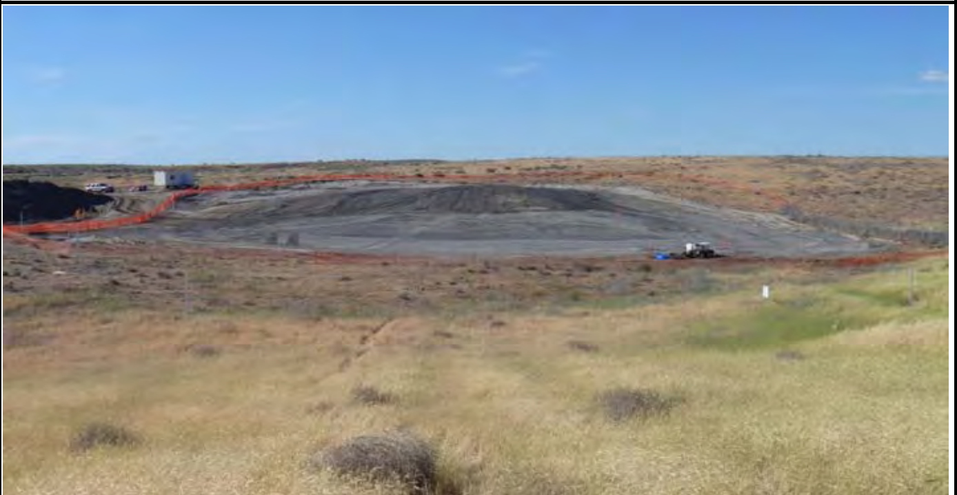
Photo 6: View of the site and G-layer near completion. Small area in SW corner is unfinished. View looking north from area beyond south end of site.
