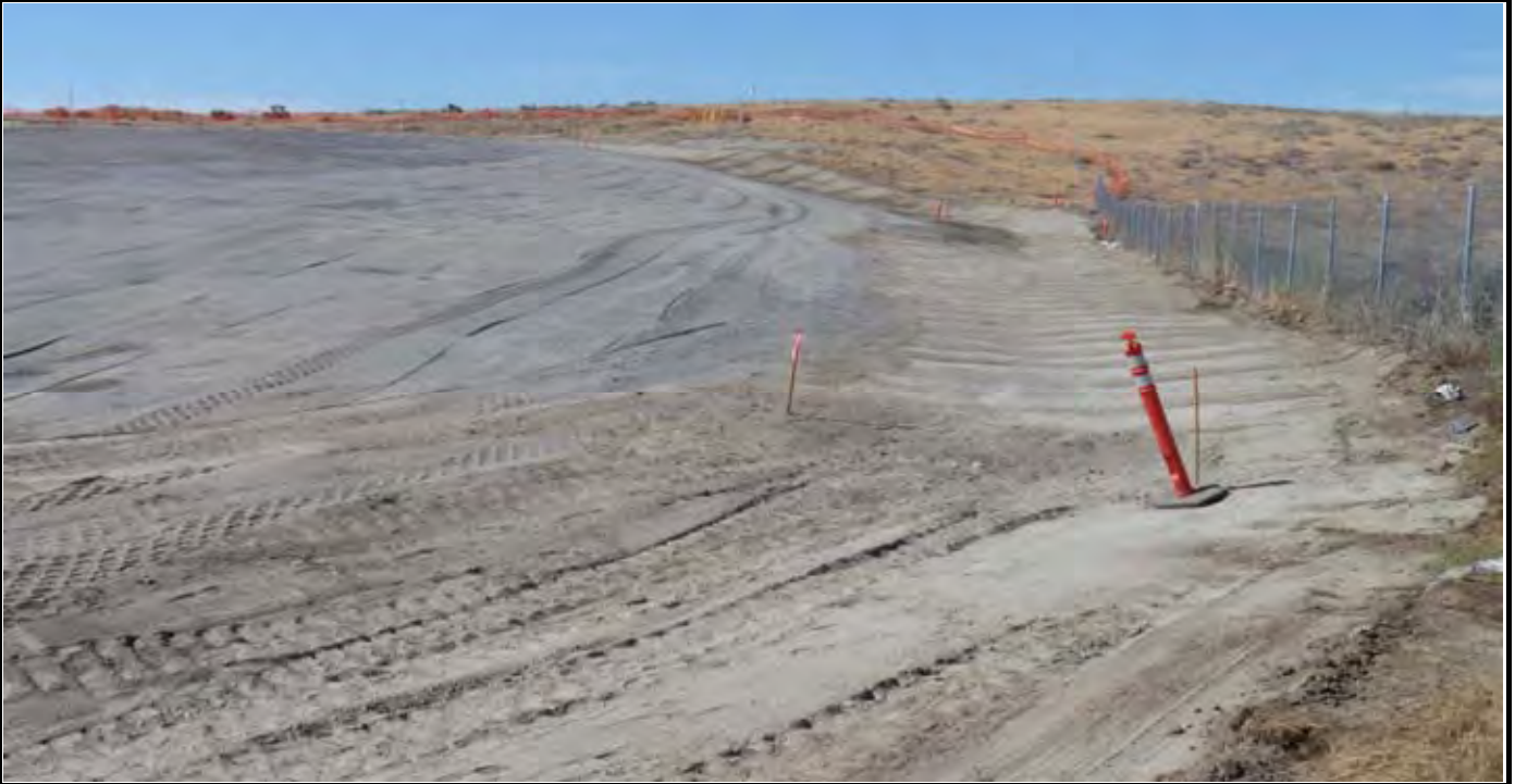
Photo 9: View of the completed and compacted area along the eastern side of the cap and area along the eastern fence line and NE swale area. View looking north from the SE corner of the CAP. Note the stakes in the foreground for EOC and EOL in SE corner.
