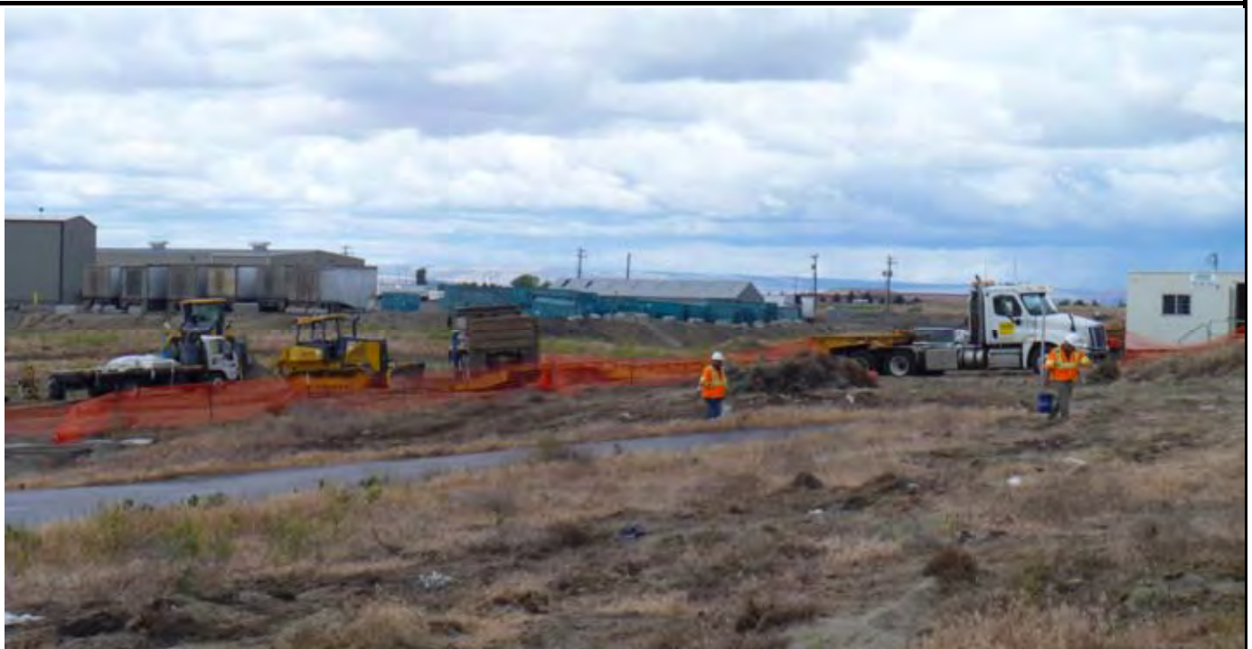
Photo 6: View of northern cyclone fencing area completely removed. View looking west from northern end of site.
