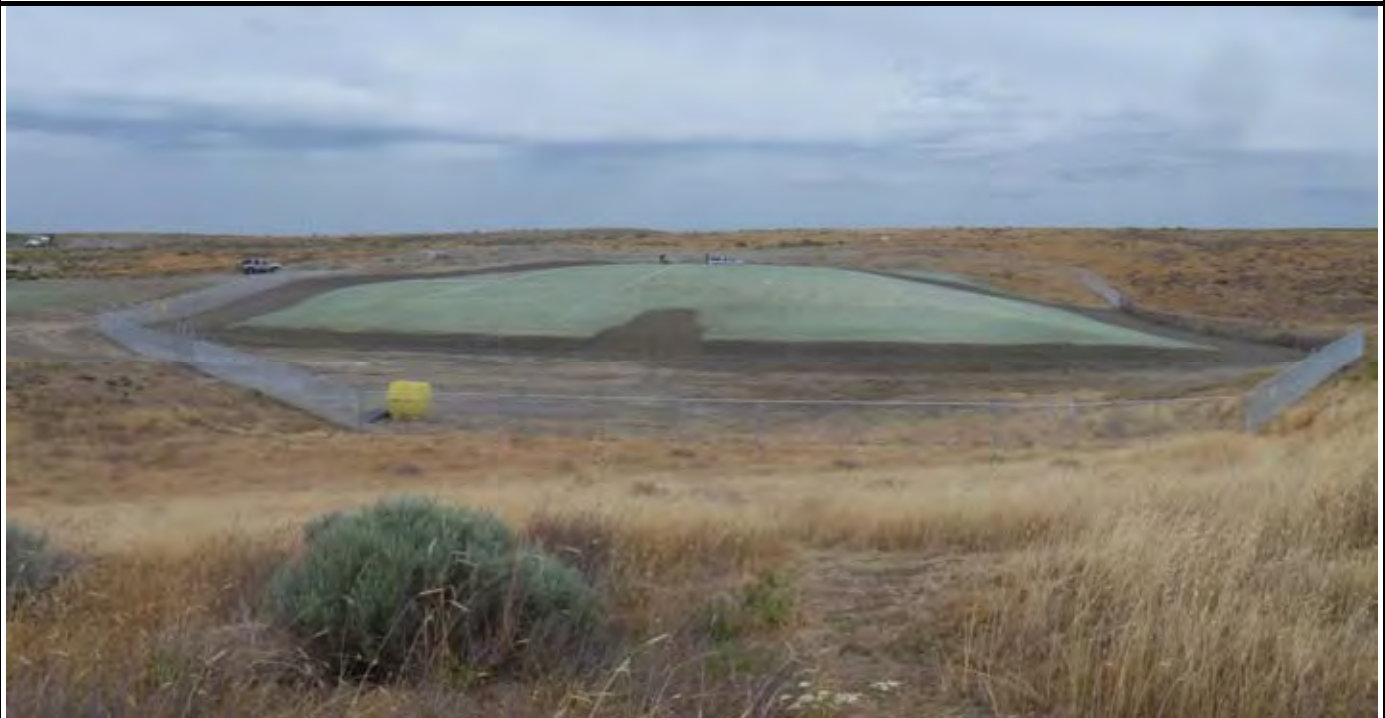
Photo 6: View of the completed CAP, perimeter fencing, hydroseeding, and irrigation system (currently installed in the picture). View of the CAP from area south of the CAP. Note that the yellow container has been moved back inside the CAP perimeter fencing.
