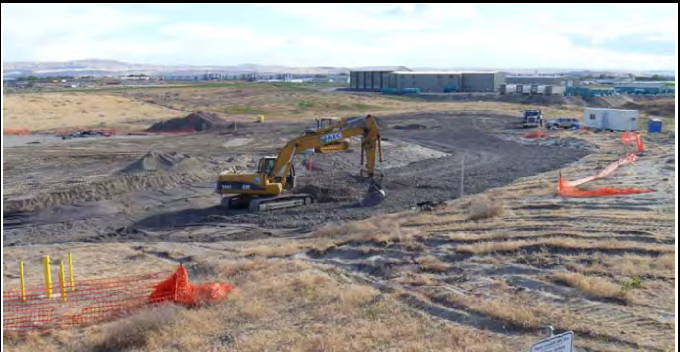
Photo 8: View of the northern swale area at the end of the day. Note that EOC grading is complete and perimeter rock has been installed beyond the swale ridge on the northern end. View looking SW from north end of the site.
