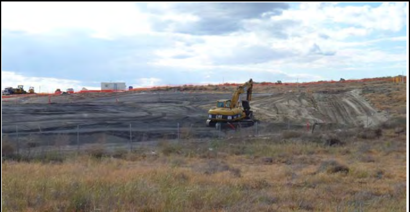
Photo 7: View of the NE swale after grubbing work at the end of the day. View looking NW from eastern side of the site.
