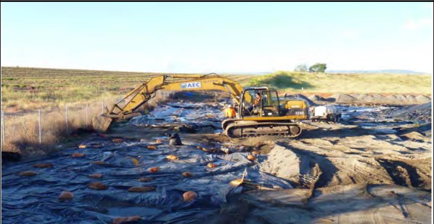
Photo 2: AEC beginning to excavate the northern edge of AE-4. View looking to the south.
