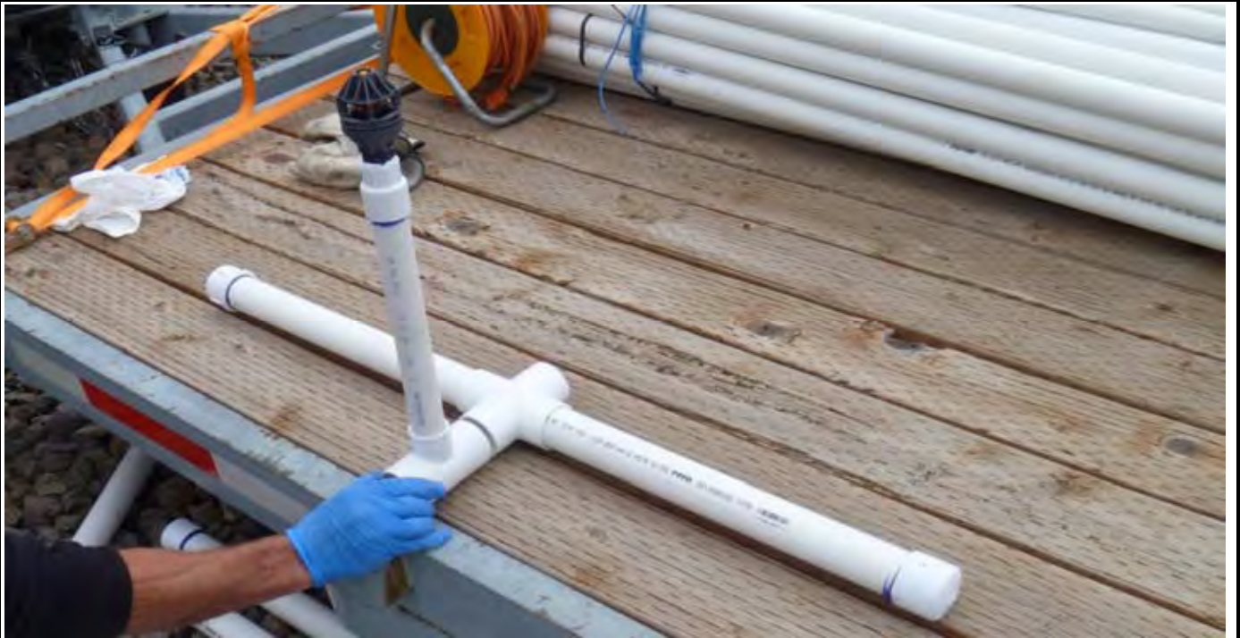
Photo 3: View of typical irrigation sprinkler head and stabilizing bars. Many of these heads were installed across the CAP surface to help establish the vegetation layer.
