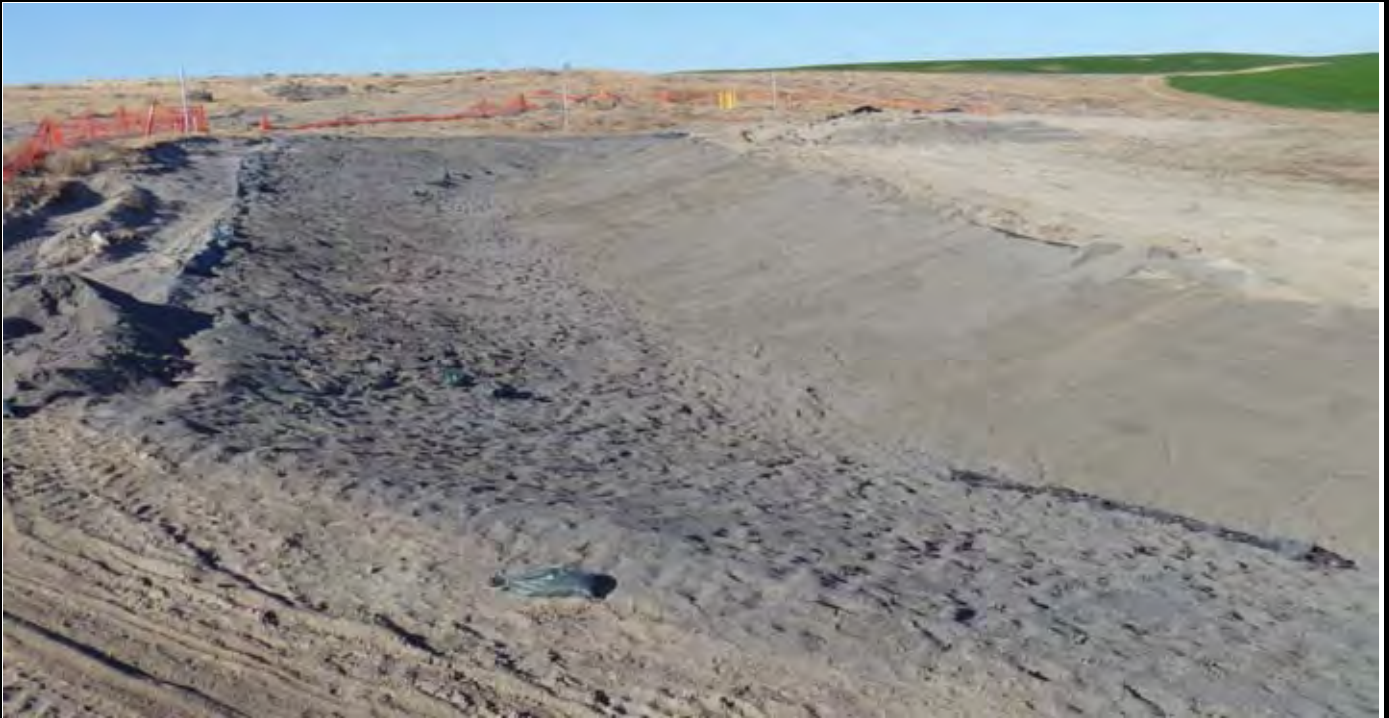
Photo 9: View of the NW and W swale area at the end of the day with sand and topsoil grading completed and ready for perimeter rock and Geo-Fabric placement. View looking NE from western EOL.
