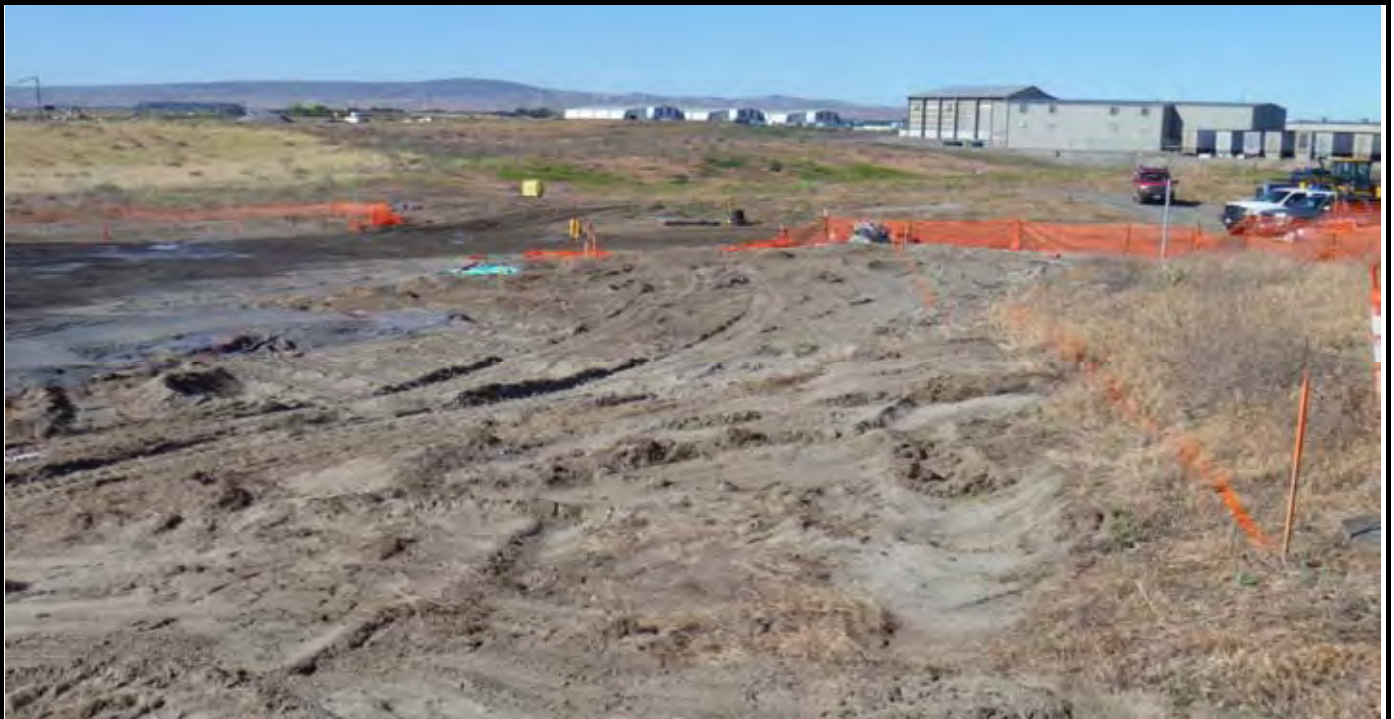
Photo 3: View of the Liner extension area / NW swale area prior to grubbing work by trackhoe. Note orange line denoting edge of liner extension. View looking to the southwest from the northwest corner of the site.
