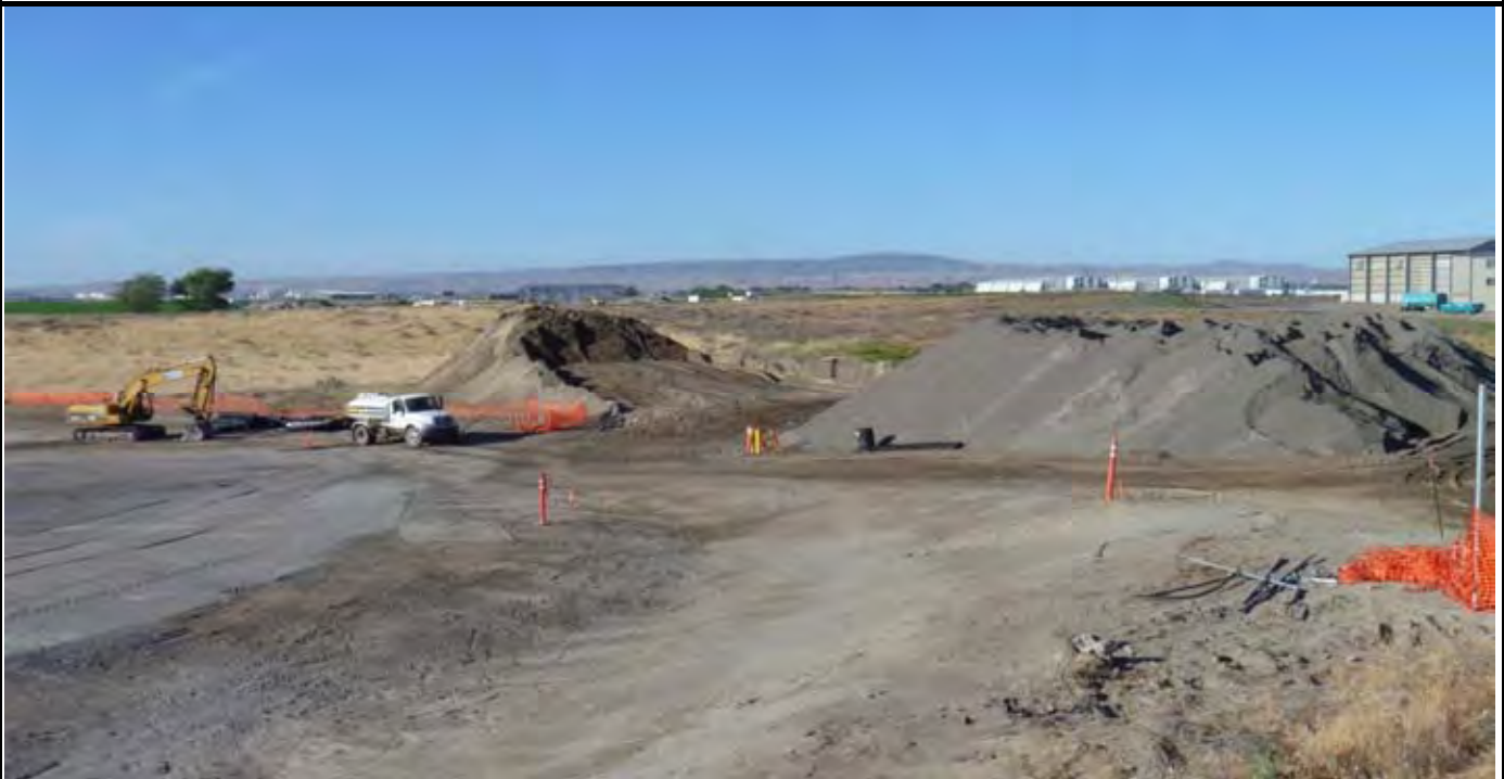
Photo 2: View of the sand (right side) and topsoil (left) stockpiles located to the west and southwest of the CAP. View looking south from NW corner of the site.
