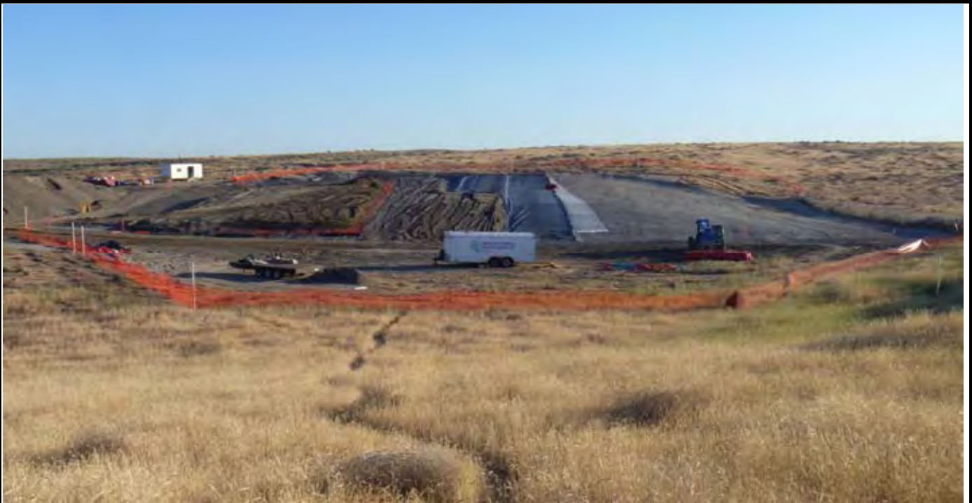
Photo 1: View of the site at the beginning of work for the day. View looking north from area south of the site. Note that geomembrane and GCL layer (small sliver of GCL on eastern edge of geomembrane) are about 55% installed.
