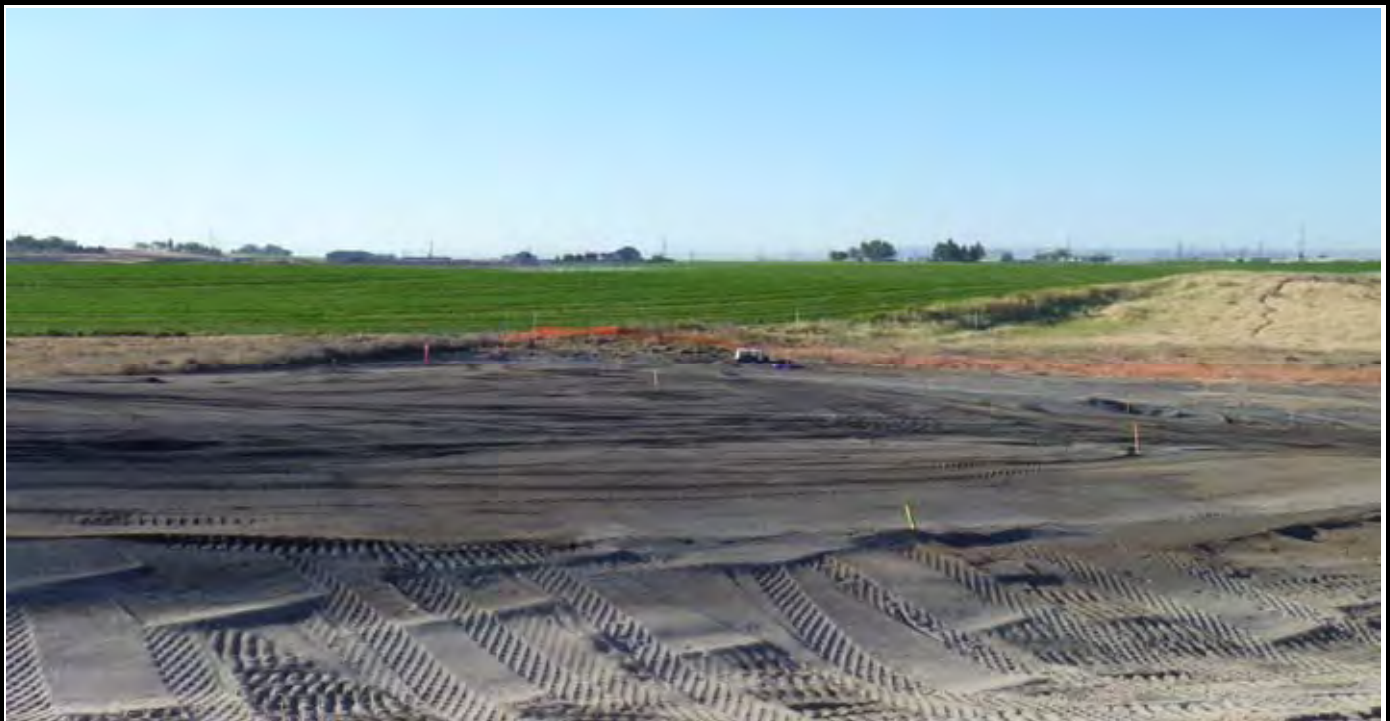
Photo 1: View of the site at the beginning of work for the day. View looking to the South / SE towards the water trailer.
