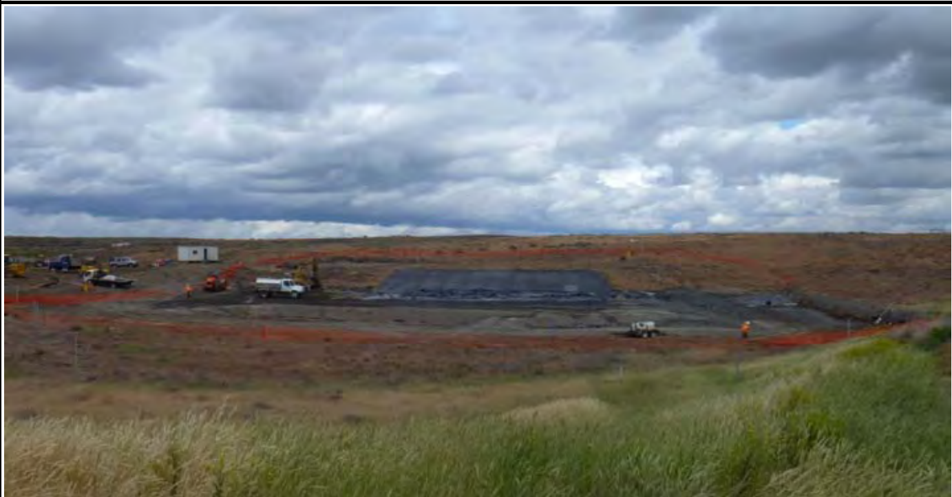
Photo 8: View of the site near the end of the work day. View looking north from hill past southern end of site.
