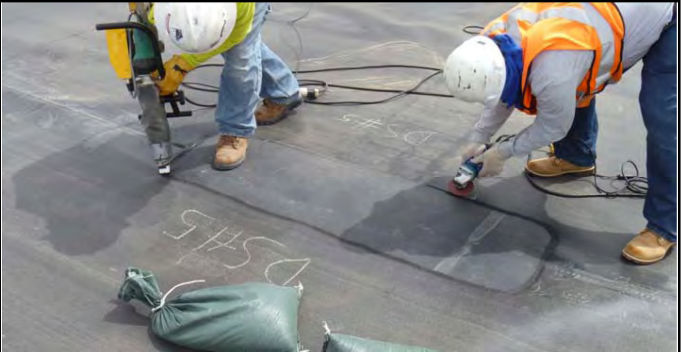
Photo 5: View of NWL patching the seam sample DS-5. Note worker with grinder (right) roughing up new patch seam and worker welding seam (left). View looking east from geomembrane panel P-10.
