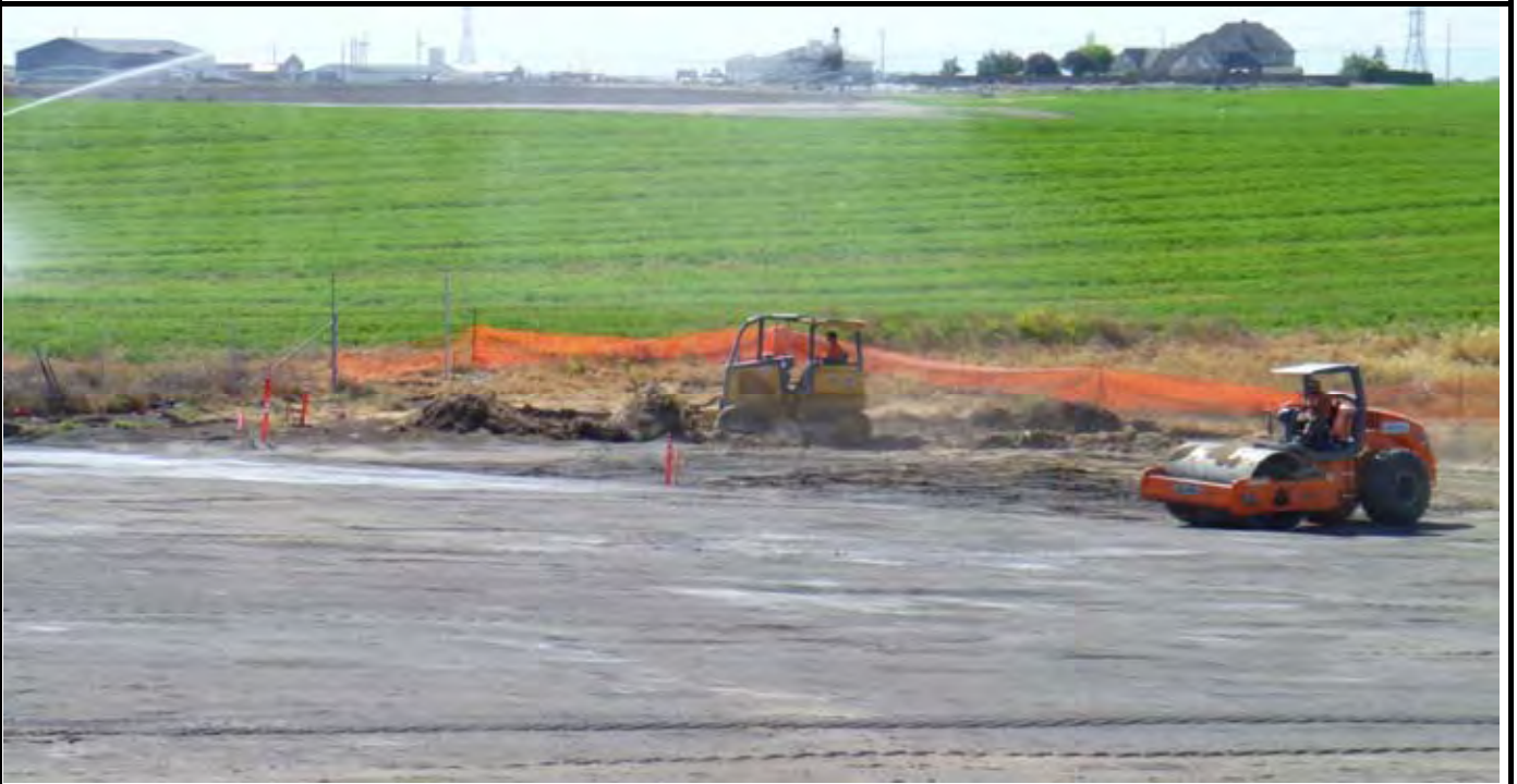
Photo 4: AEC begins grading area beyond the SE corner of the cap in accordance with design. Note AEC roller compacting area along SE corner of g-layer cap. View looking SE from center of cap
