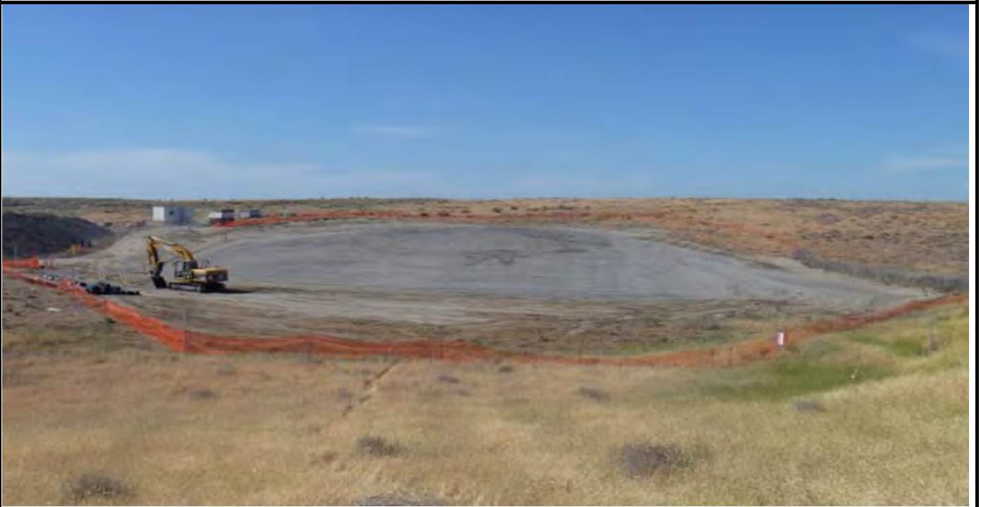
Photo 10: View of the site at the conclusion of work for the day. Orange construction fence is up around the site. Note geomembrane and geosynthetic stockpiled on left side of picture next to trackhoe. G-layer is complete and prepared for GCL and geomembrane installation.
