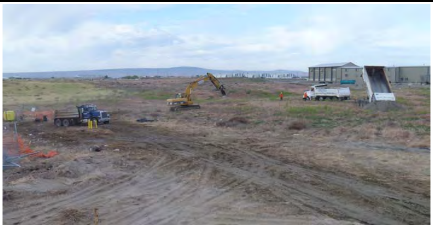
Photo 4: View of first G-layer material drop by dump trucks. Material is being dropped inside loop area west of the new CAP. View looking south/southwest from northern edge of the CAP.
