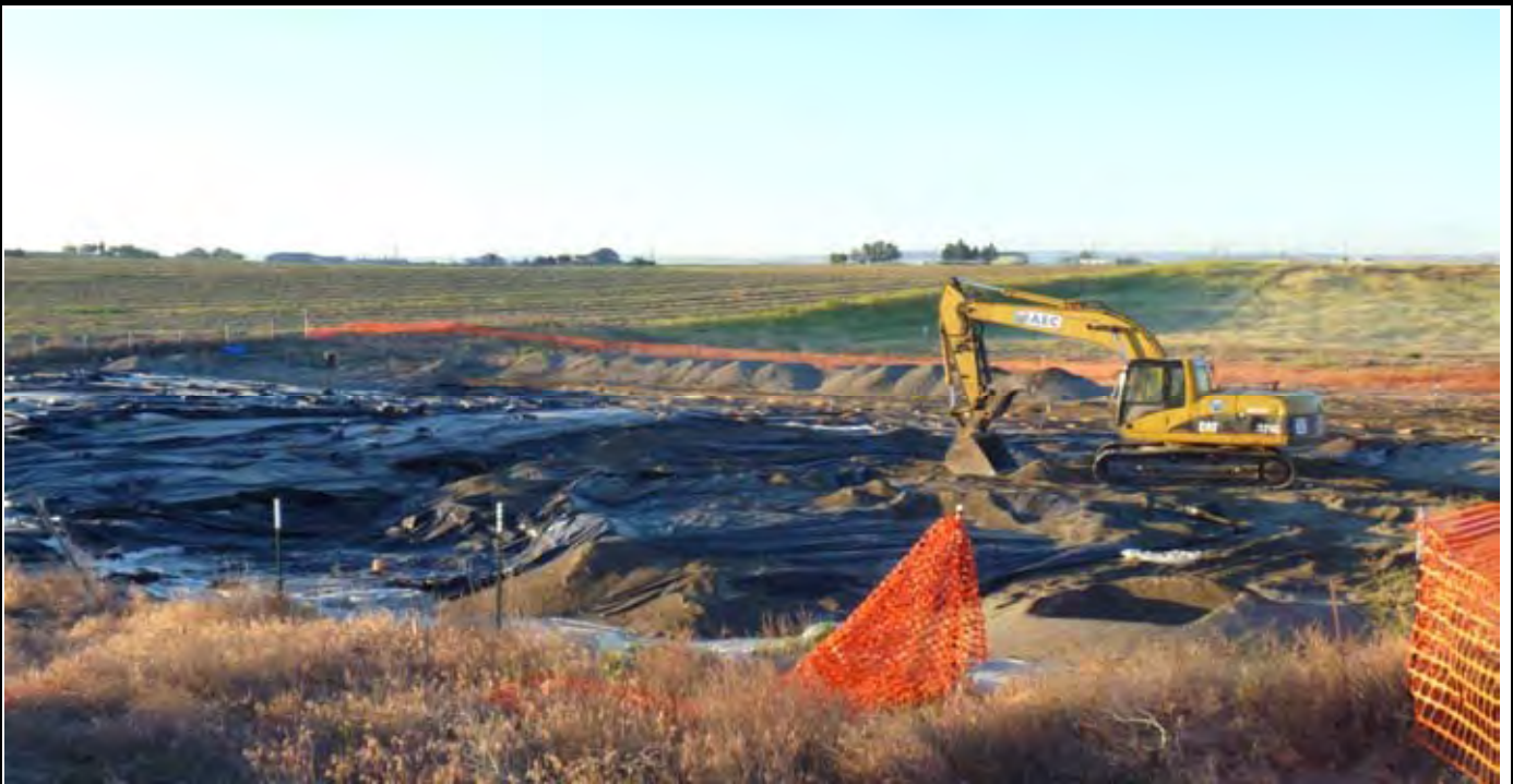
Photo 1: View of the site at the beginning of work for the day. View looking to the South / SE towards the trackhoe. Note that all of the soils from AE-1 and AE-2 were covered with 12-mil and then covered with gravel.
