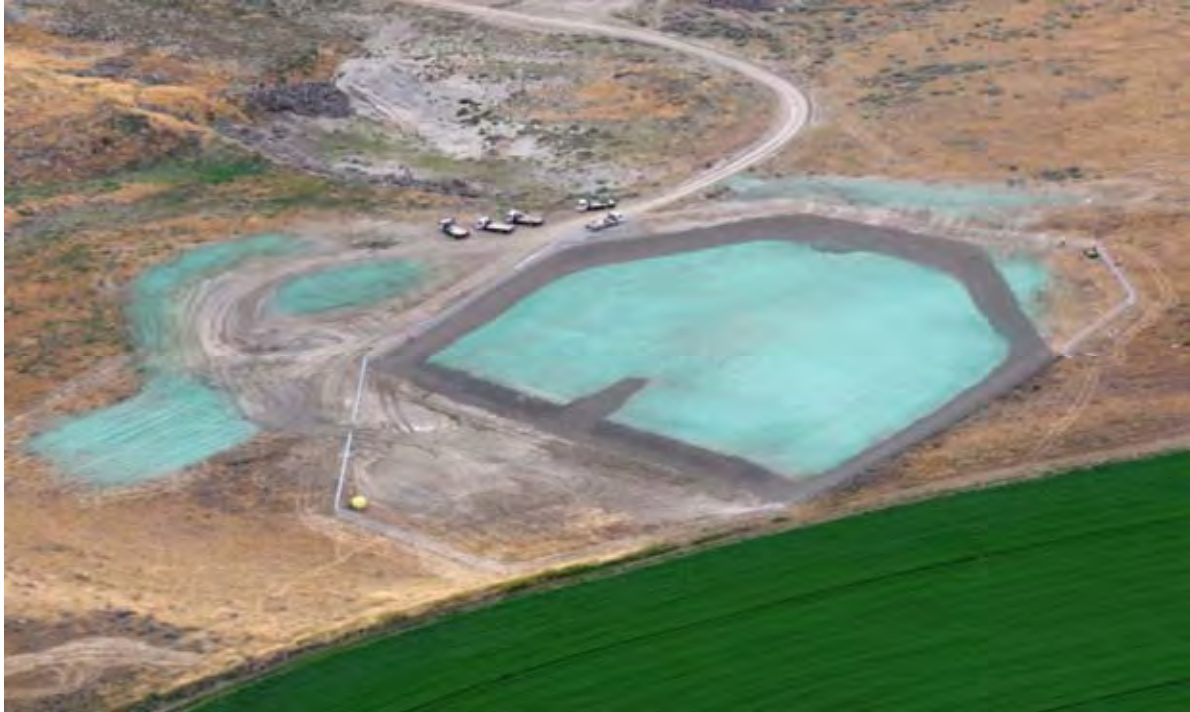
Photo 7: View of the completed CAP and perimeter fencing and hydroseeding on the CAP and surrounding areas that were disturbed during the CAP construction. This is an aerial photograph taken in the sky southeast of the landfill.
