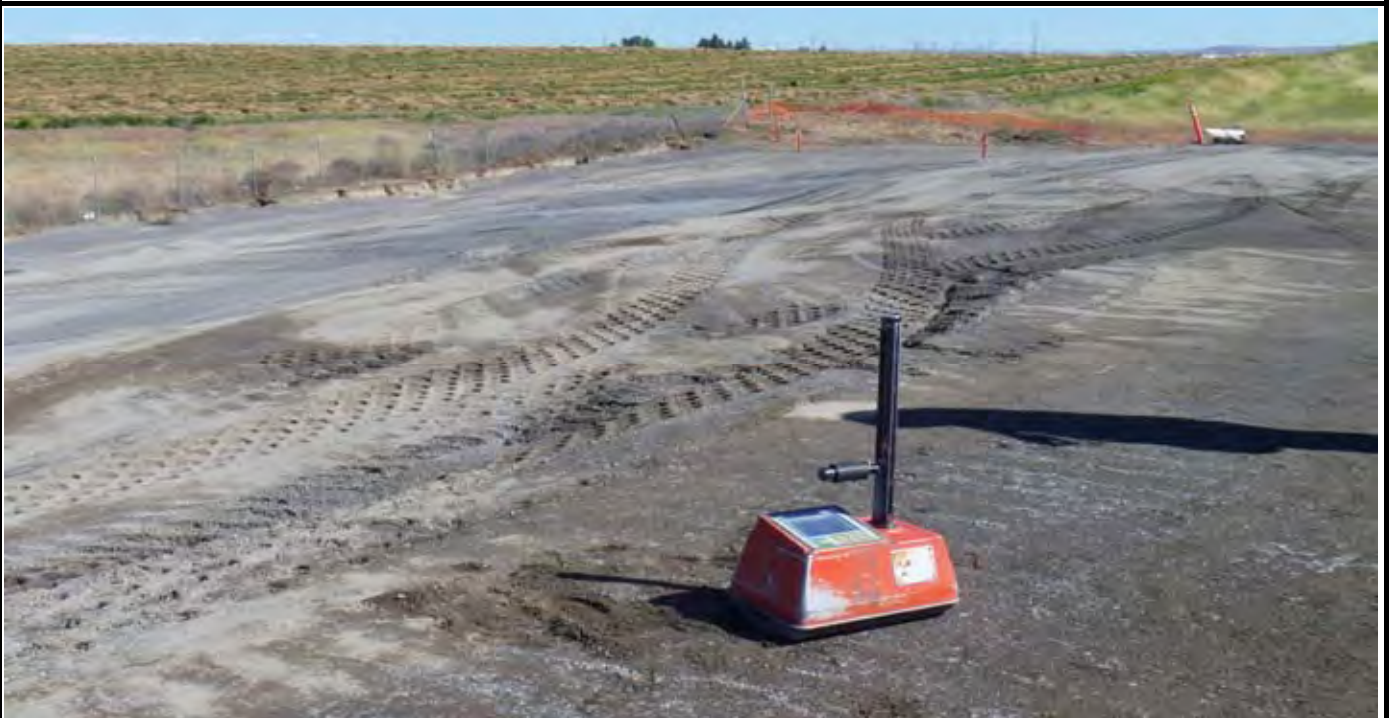
Photo 8: View of compaction density testing along the eastern side of the G-layer. View looking to the SE from the northern end of the CAP area.
