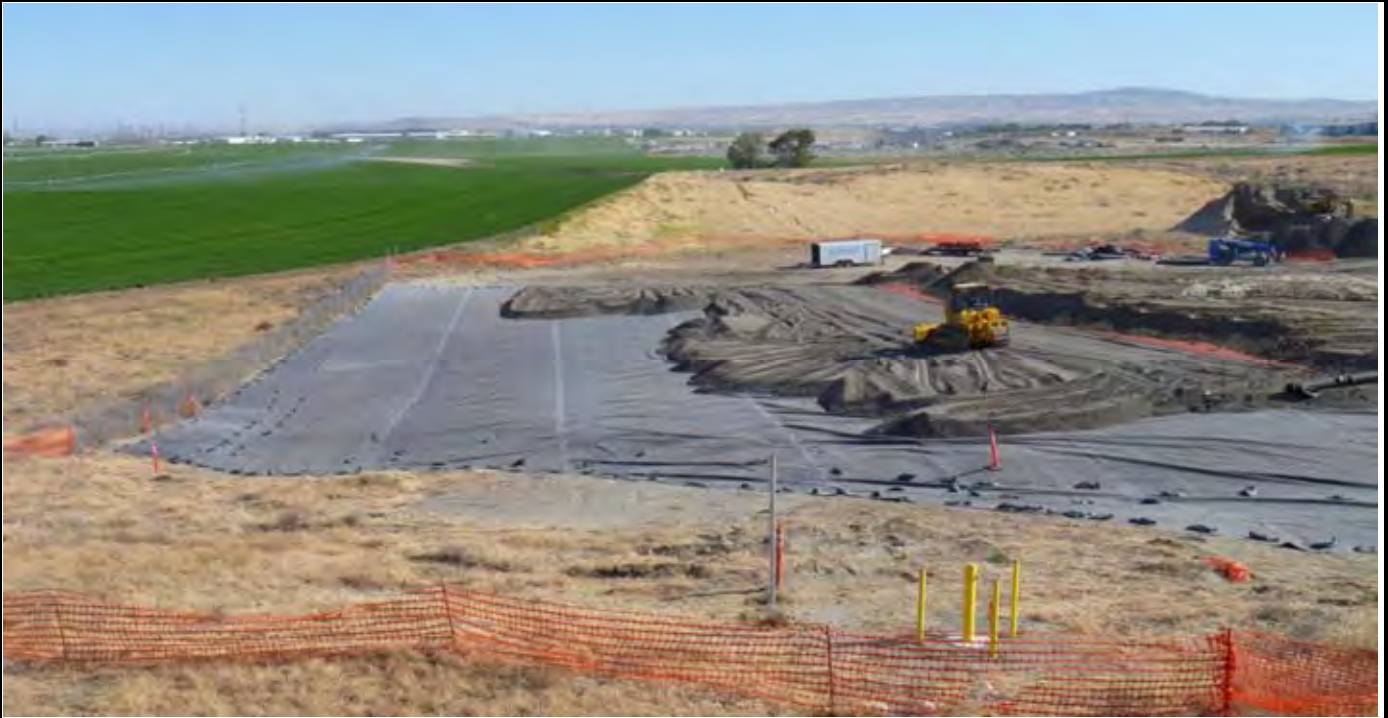
Photo 9: View of the completed geomembrane area (eastern side of CAP) and AEC spreading and grading sand layer. View looking south from area north of the northern OCF edge.
