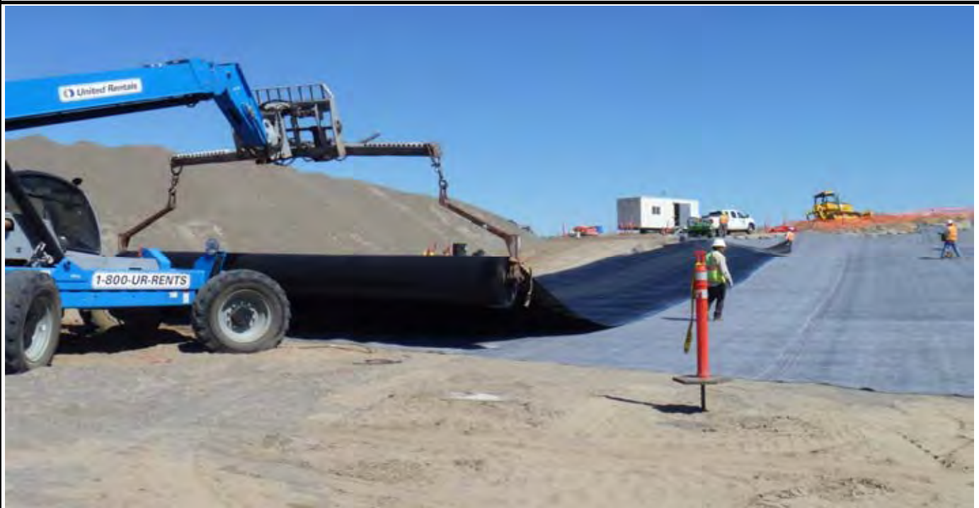
Photo 8: View of NWL rolling out the first pass of geomembrane over the GCL along the western edge of the EOL. Note the different roller assembly held up by the telehandler. View looking north from area near the SW corner of the EOL.
