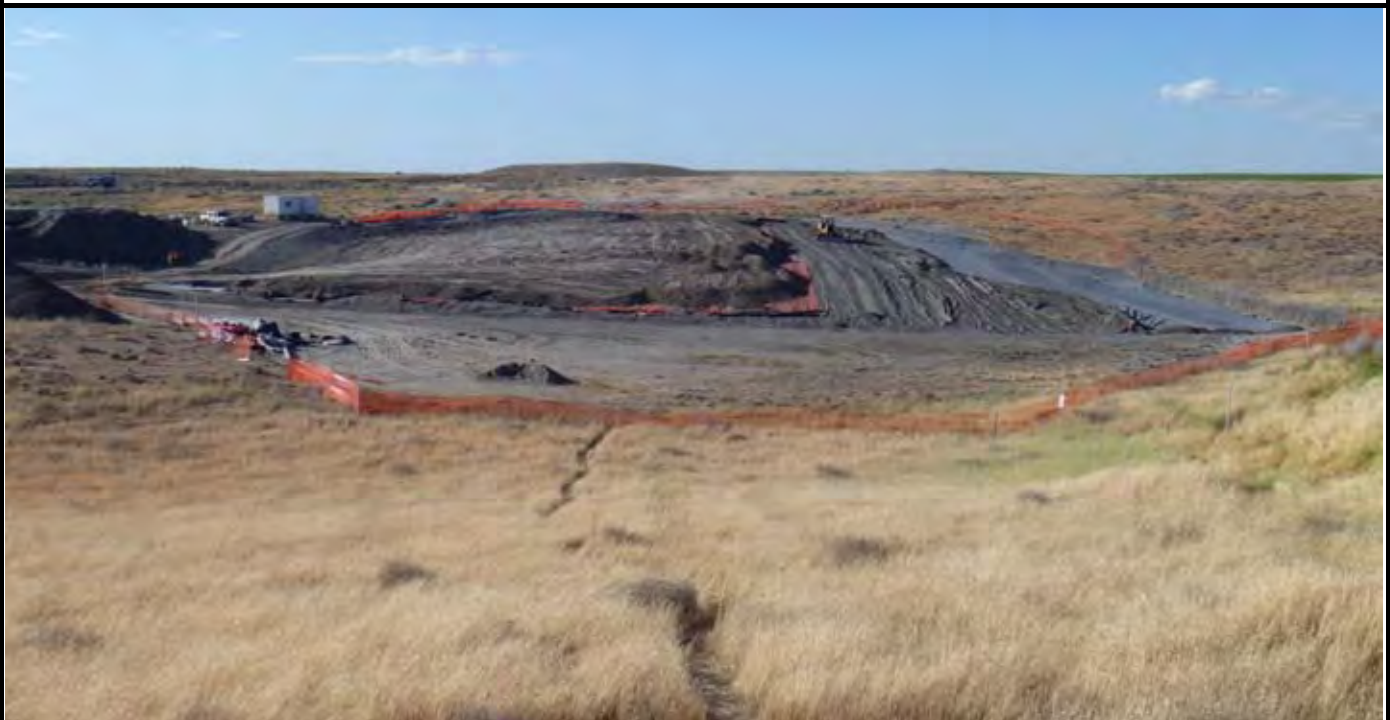
Photo 12: View of the site at the conclusion of work for the day. Note completed geomembrane installation and sand (approximately 75% complete) and topsoil (approximately 60% complete) layers. View looking north from area south of the southern edge of the site.
