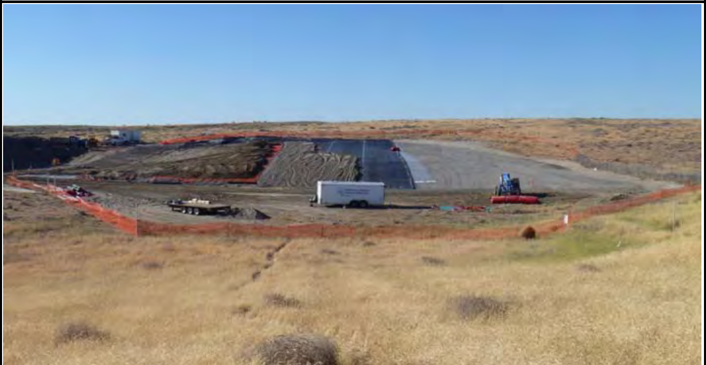
Photo 10: View of the site at the conclusion of work for the day. Note large sand layer over all but one exposed geomembrane panel and topsoil covering nearly all of the exposed OCF/geo-fabric (so it won't blow away). View looking north from area south of the site.
