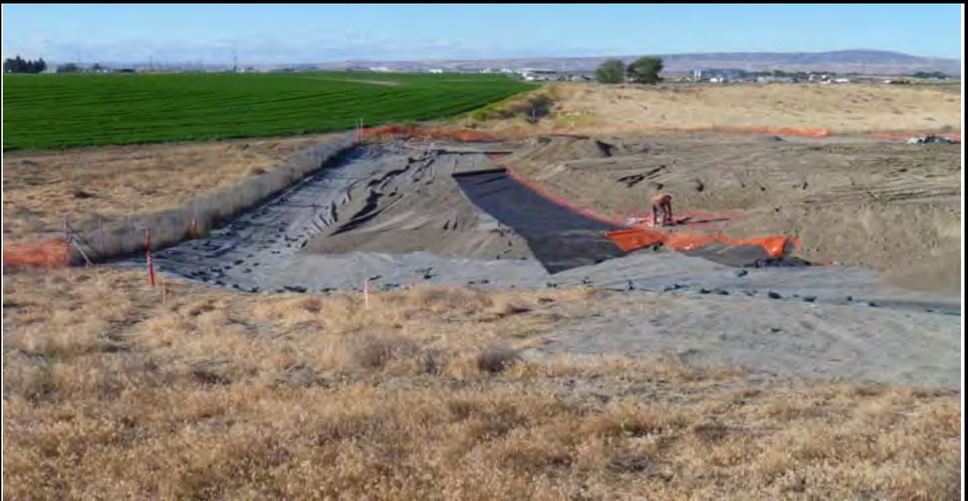
Photo 5: View of the eastern edge of the CAP (EOC) and northeastern and eastern swale areas (showing only the geomembrane liner with sandbags on it). View looking south from NE corner of the site. Note AEC laying out Geo-Fabric and OCF over the sand layer which extends to the EOC and adjacent topsoil layer.
