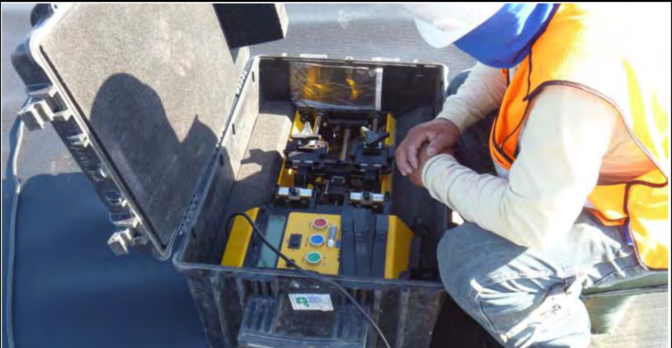
Photo 6: View of field testing equipment used to test the DS samples of the seams. Note two parallel tracks testing two seam samples at the same time.
