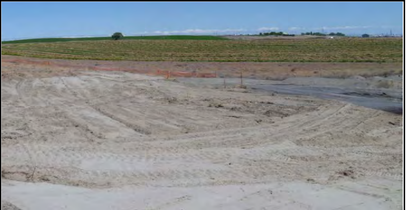
Photo 5: View of the northern end of the liner extension area after majority of grubbing completed. View looking to the east from the NW corner of the site.
