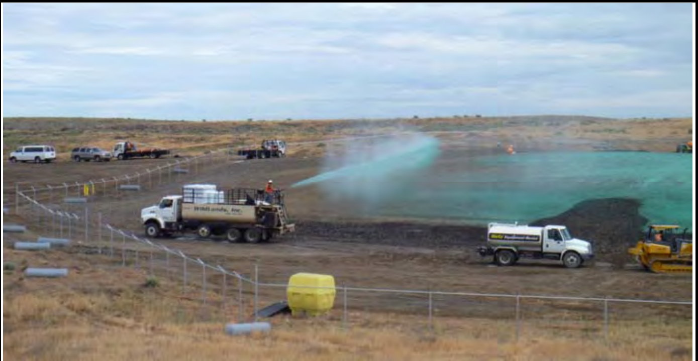
Photo 5: View of Wildlands hydroseeding the SW corner of the CAP. Note water truck and bulldozer on right side. View of the western half of the CAP from area south of the site. Note fencing is staged for installation.
