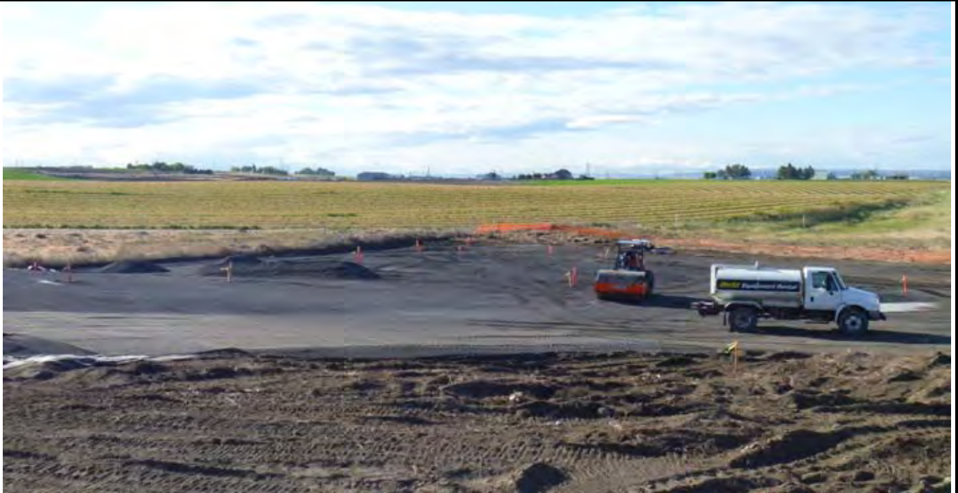
Photo 1: View of the site at the beginning of work for the day. View looking to the South / SE towards the roller.
