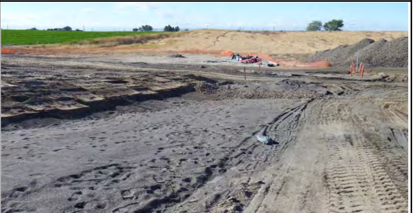
Photo 2: View of the southern end of the western swale as AEC begins to install the perimeter rock. Note perimeter rock stockpile in upper right. View looking south from western EOL.
