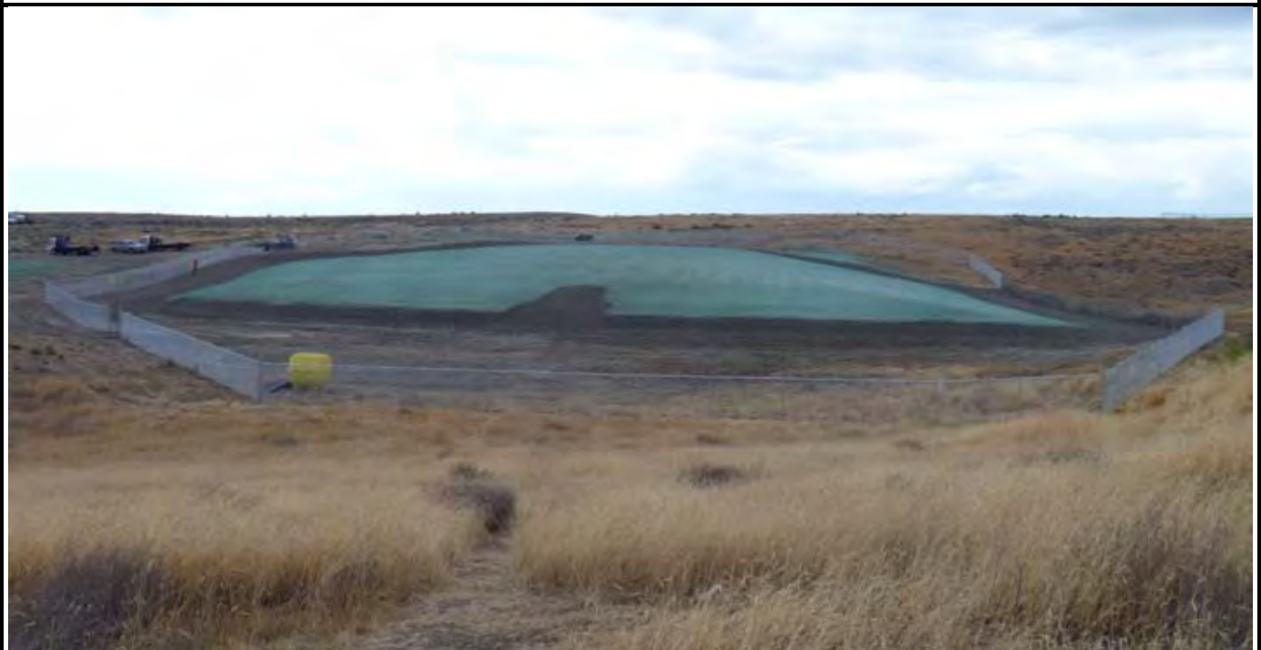
Photo 10: View of the site at the conclusion of work for the day. Note the perimeter fencing is up (no gates or barb wire yet) and hydroseeding work has been completed by Wildlands. View looking north from area south of the site.
