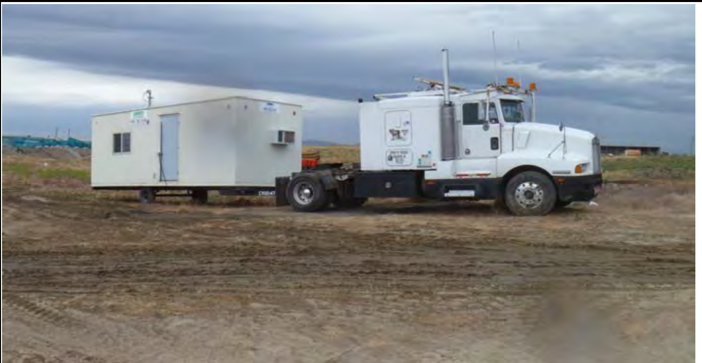
Photo 8: Jobsite trailer being delivered to the site. Trailer placed along west side of the access road west of the western side of the CAP. View looking NW from the western side of the CAP.
