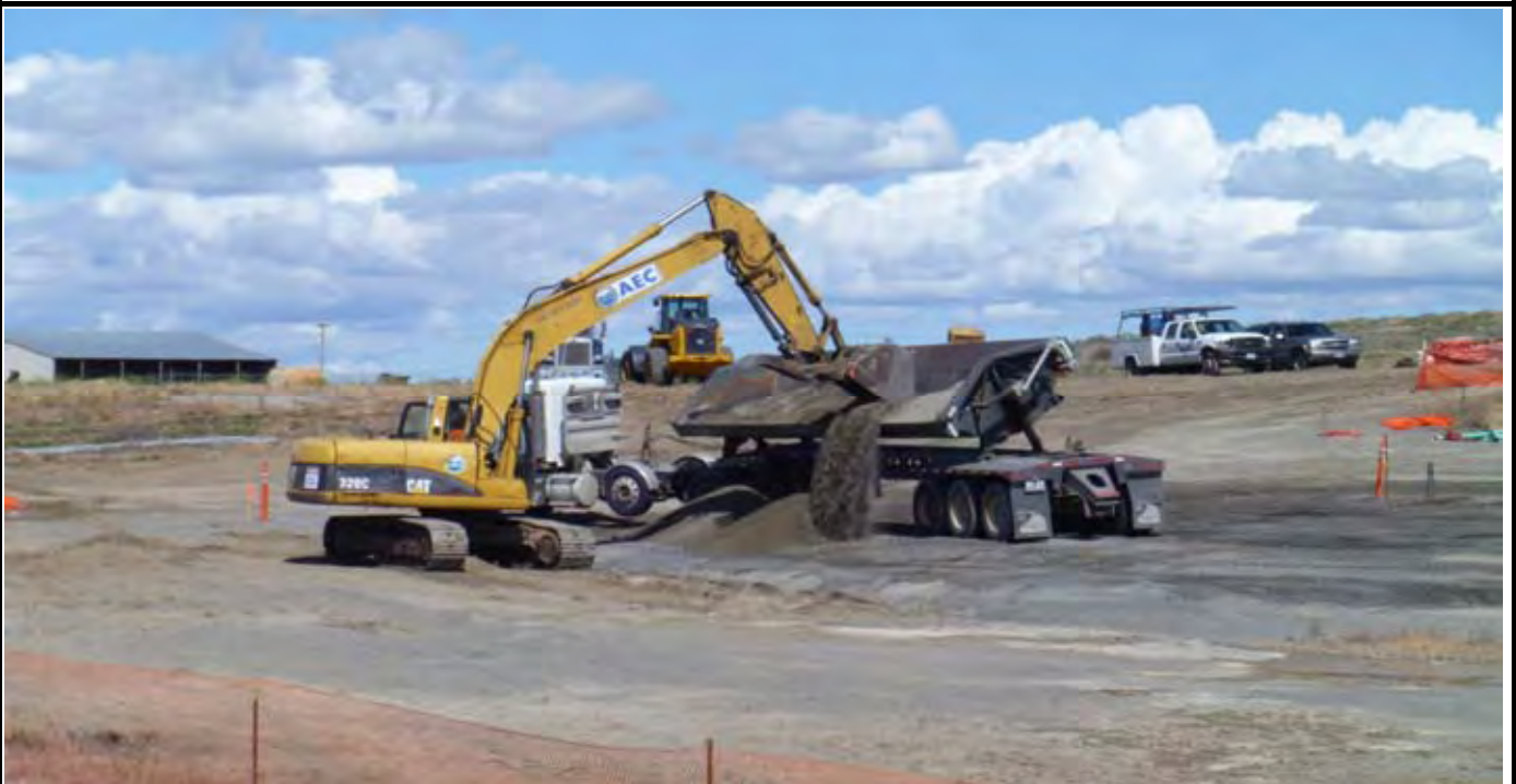
Photo 2: AEC using the trackhoe to empty the gravel from the trailer that is having mechanical issues. View looking west from SE corner.
