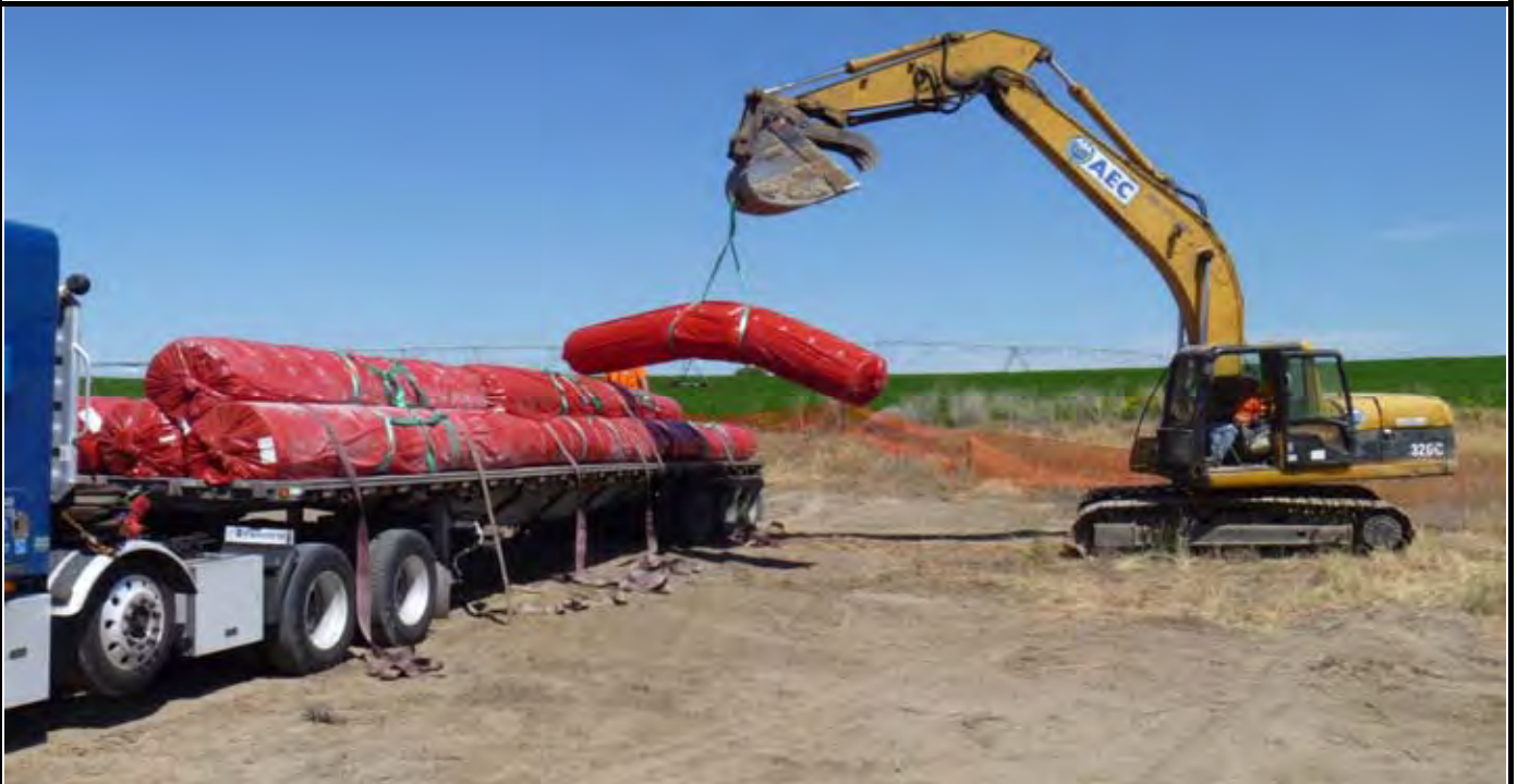
Photo 8: View of AEC off loading last (3rd) shipment of GCL rolls (14 rolls on truck for total of 41 rolls of GCL delivered). View looking east from area south of the southern edge of the EOL.
