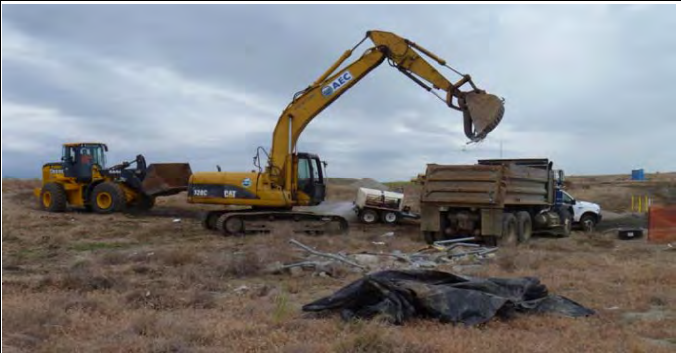
Photo 7: View of AEC loading metal fencing material into dump truck for recycling. View looking west from the SW corner of the CAP area.
