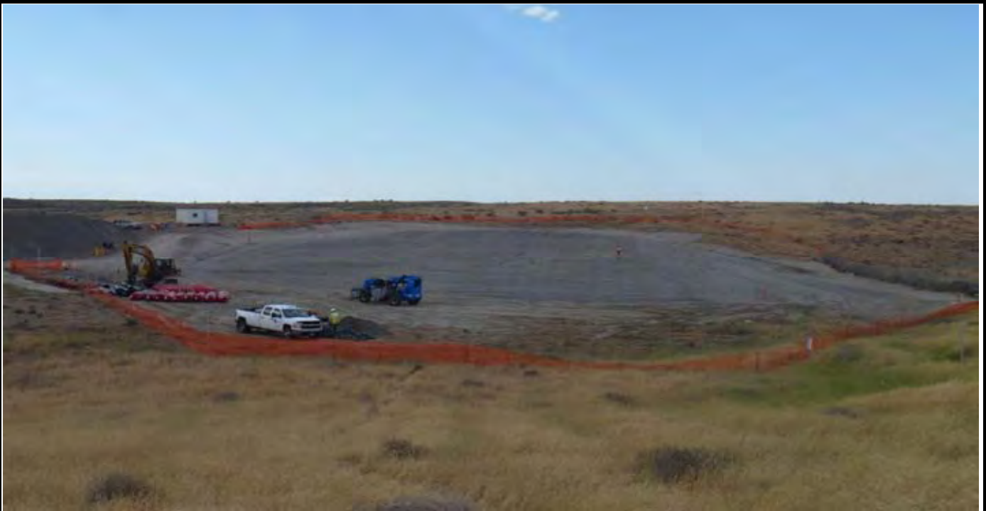
Photo 7: View of the site at the end of the day. Note NWL telehandler, rolls of GCL (red), geomembrane and fabric rolls (black by trackhoe), NWL white truck and sand pile for sand bags. View looking north beyond southern infiltration basin.
