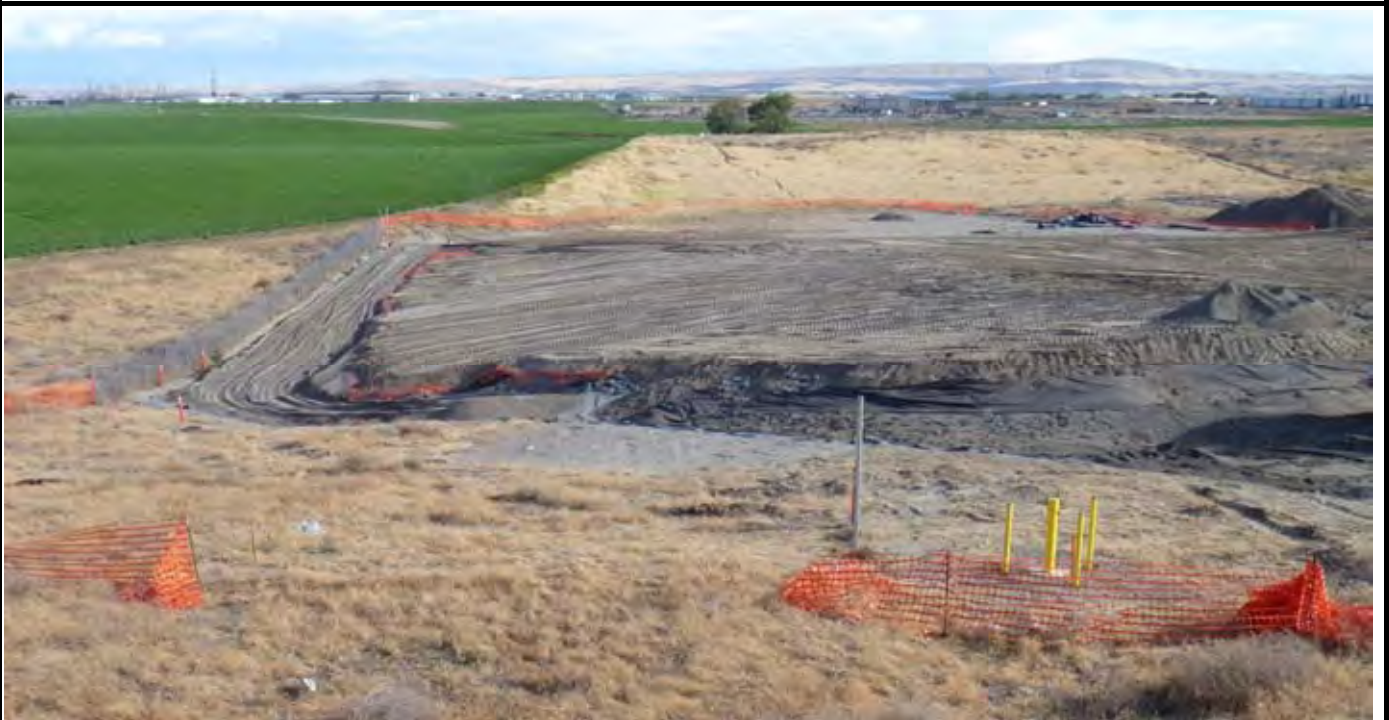
Photo 6: View of the eastern half of the CAP and eastern and northeastern swales with installed sand layer over the geomembrane at the end of the day. View looking south from area just north of the site.
