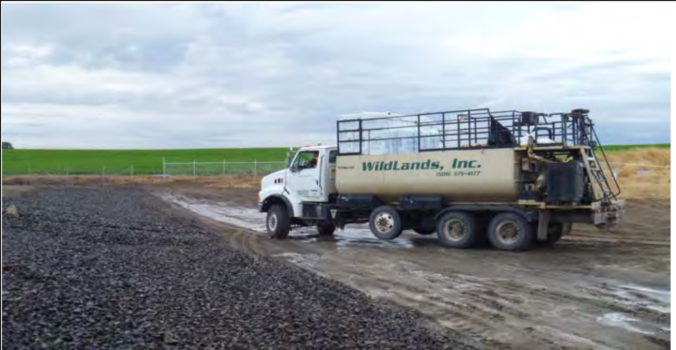
Photo 1: View of the hydroseeding truck (Wildlands, Inc.) along the southern side of the CAP just prior to them commencing with hydroseeding work. View of the southern edge of the CAP (EOL) from SW corner of the CAP.
