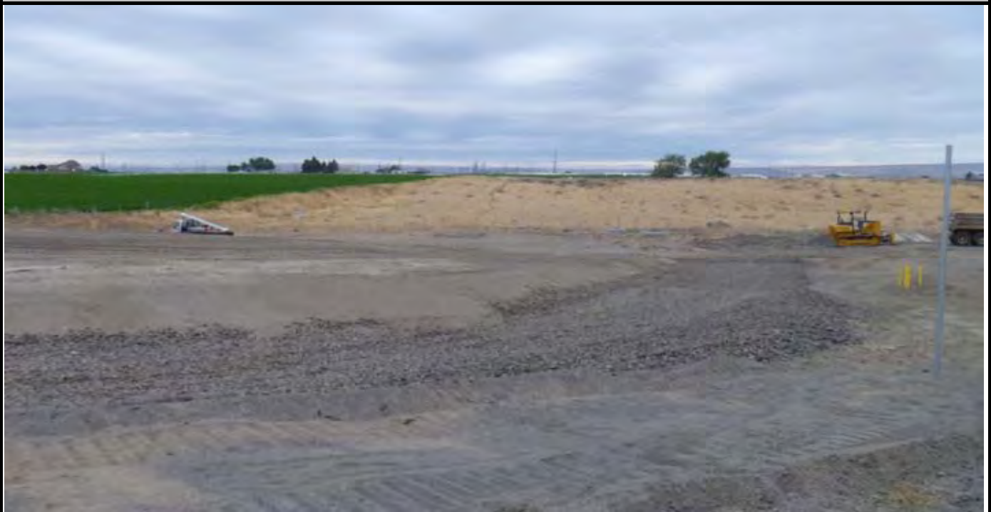
Photo 1: View of the site at the beginning of the work day. Note that many of the fence posts have not yet been installed on the western side of the CAP perimeter. View looking south from NW corner of the CAP.
