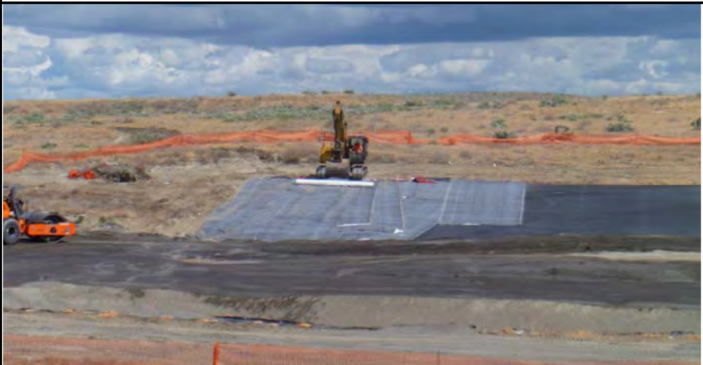
Photo 2: AEC rolling out the "Old GCL" rolls along the NW corner of the existing liner. AEC did not drive their trackhoe over the existing original cap liner. View looking north from south side of site.
