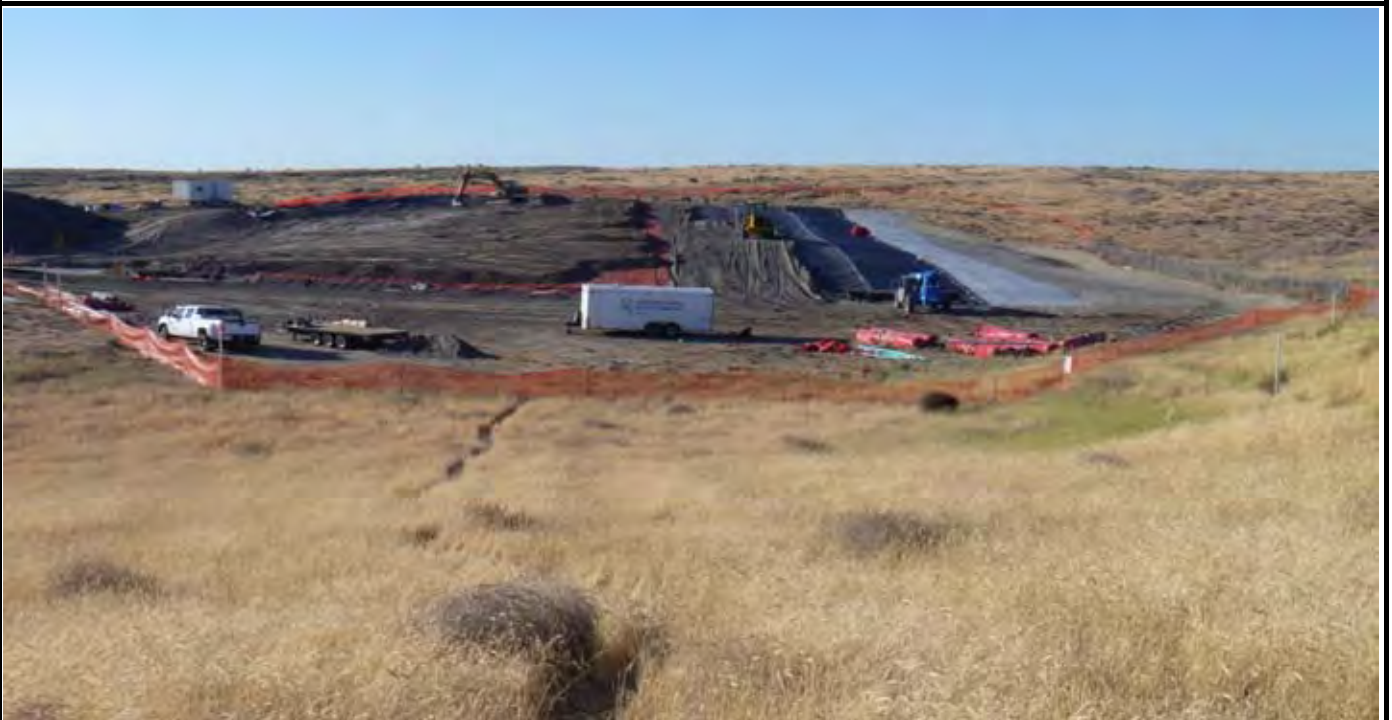
Photo 10: View of the site at the conclusion of work for the day. Note that GCL layer is about 80% done and geomembrane layer is about 75% installed. View looking north from area south of the site.
