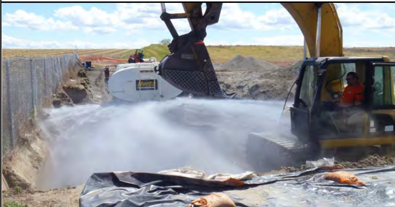
Photo 8: View of AEC watering truck watering the backfill materials in AE-4. View looking to the south over the top of the water truck.
