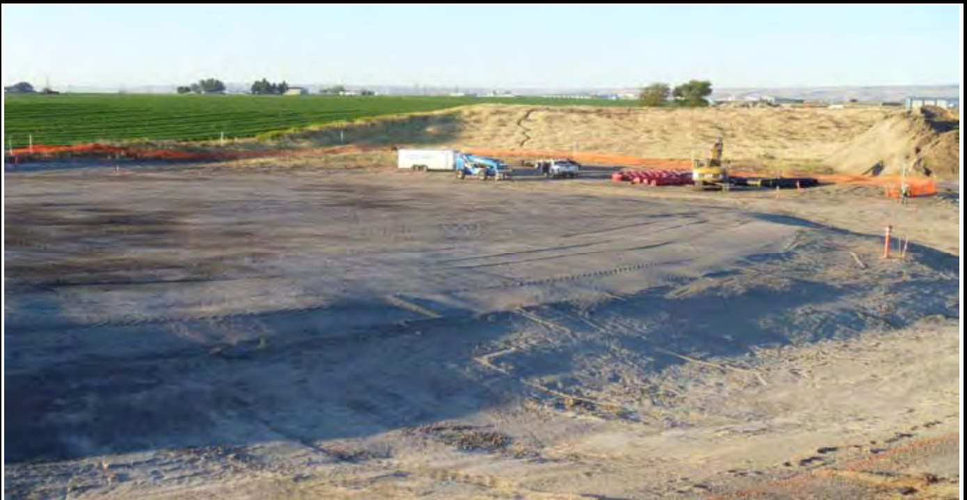
Photo 1: View of the site at the beginning of work for the day. View looking to the South / SE towards the staged materials and NW Linings (NWL) trailer and telehandler.
