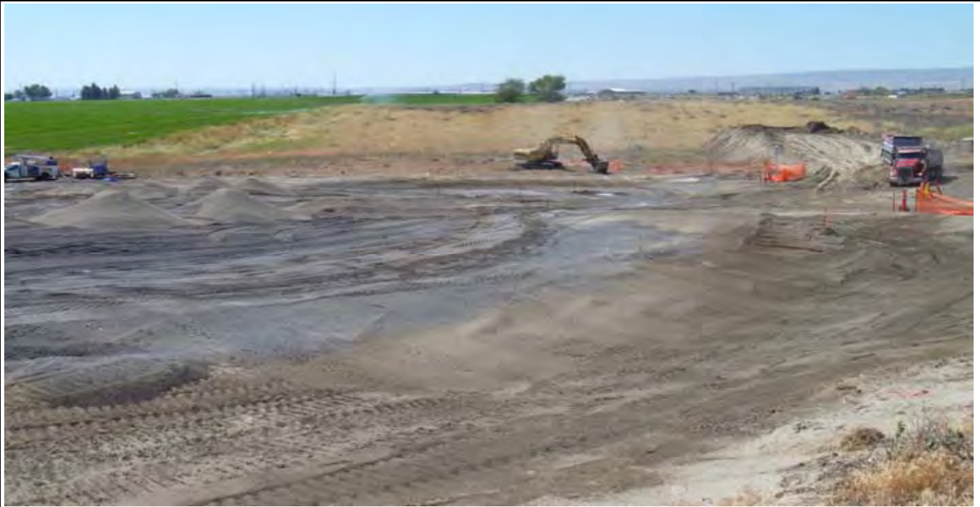
Photo 3: View of SW corner of cap nearing completion and AEC trackhoe beginning grubbing/grading work in the infiltration basin area during bulldozer repair. Note OCF installed along new outer fence posts. View looking south from NW corner of site.
