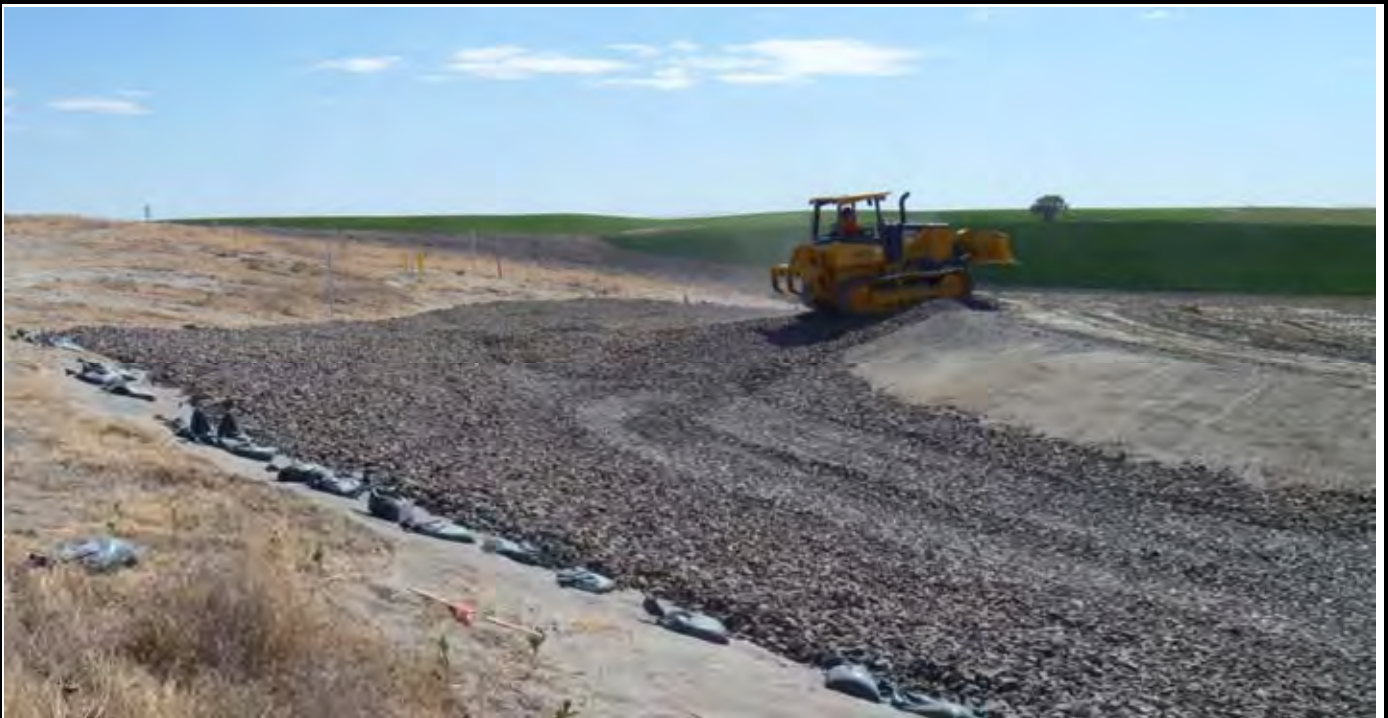
Photo 4: View of AEC finish grading the erosion protection rock roadway access point on the northern end of the EOC to EOL area. View looking east from NW corner of the CAP.
