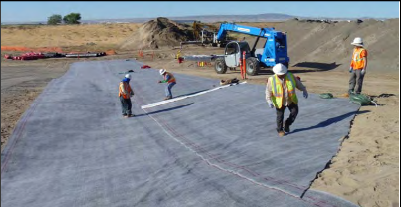
Photo 5: View of NWL installing small piece of GCL just north of the first GCL roll to finish off the western EOL. Note that NWL has cut the northern edge to match the angle of the EOL perimeter. View looking south from the northwestern EOL.
