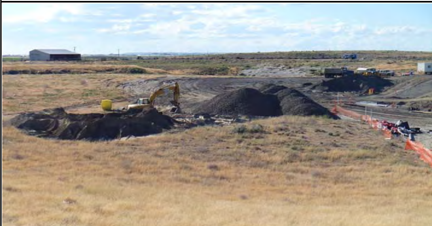
Photo 8: View of the topsoil and perimeter rock stockpiles at the end of the day. View looking northwest from area south of the site.
