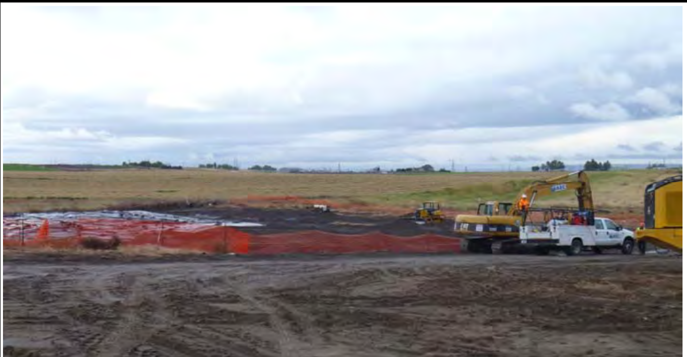
Photo 1: View of the site at the beginning of work for the day. View looking to the South / SE towards the trackhoe.
