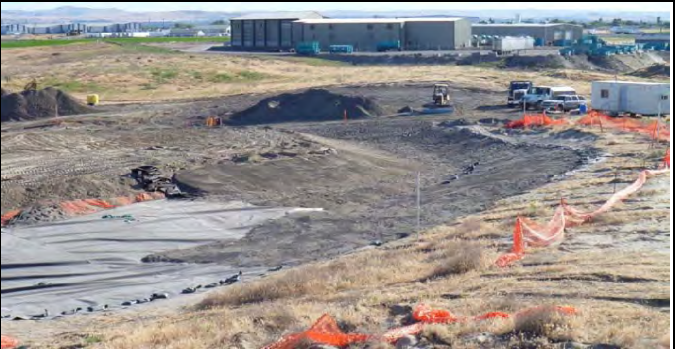
Photo 11: View of the NW corner of the CAP and NW / N perimeter swale areas after completion of sand and topsoil grading work at the end of the day. Note OCF fencing has been opened for trackhoe access to place sand into swale areas. View looking SW from area north of the site.
