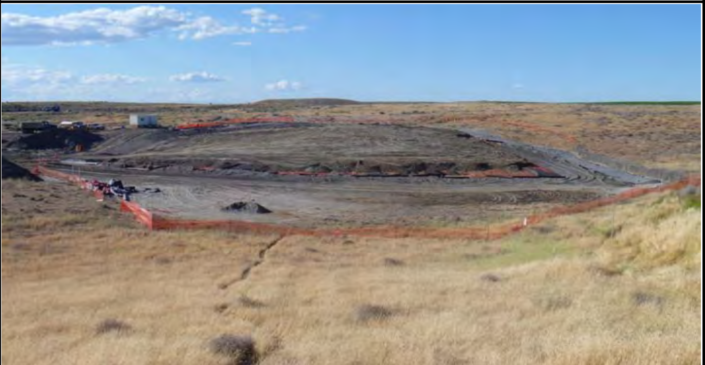
Photo 12: View of the site at the conclusion of work for the day. Note completion of sand layer over entire EOC zone and nearly complete topsoil layer. View looking north from area south of the site.
