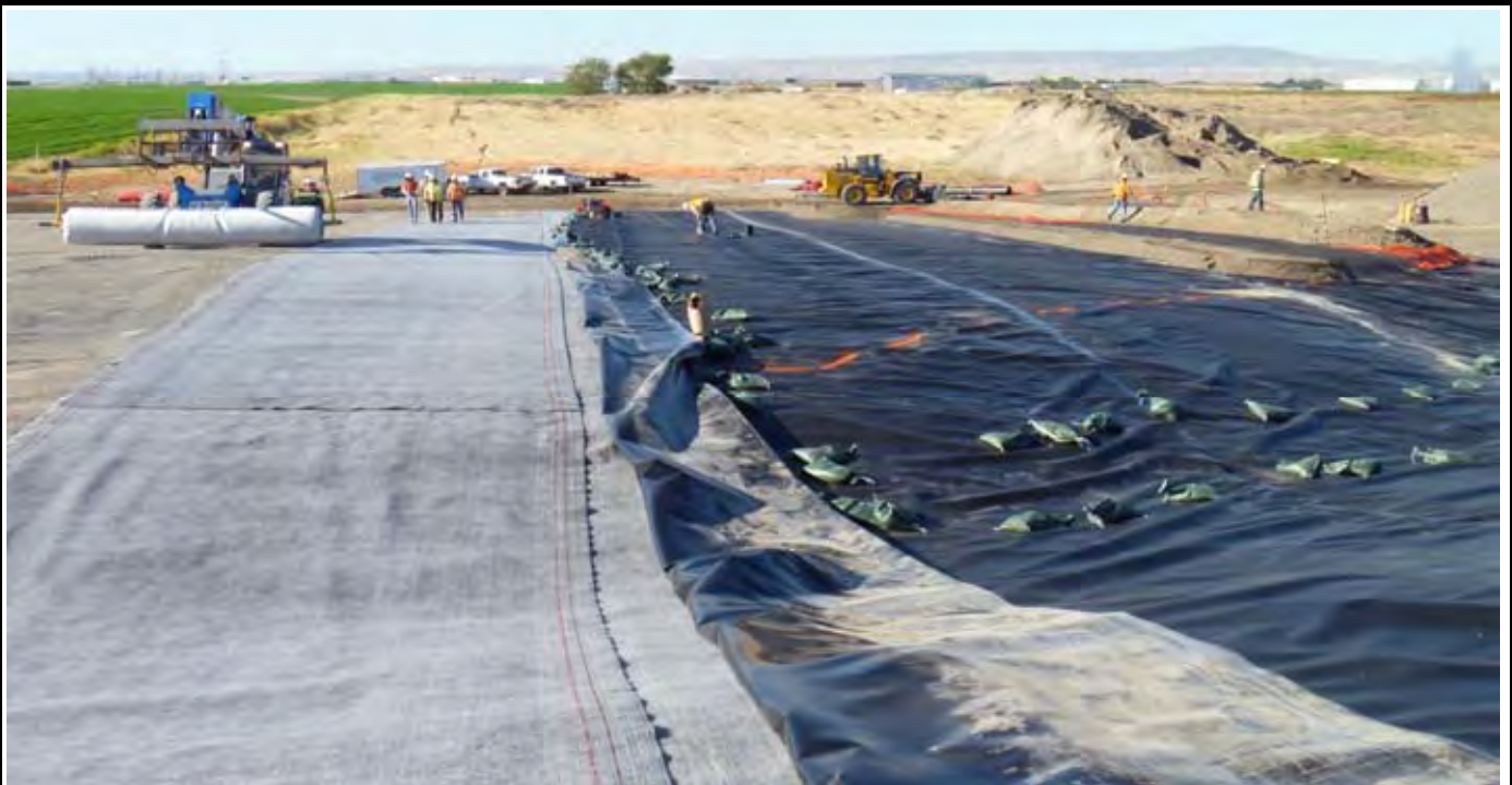
Photo 5: View of NWL starting to lay out rolls of GCL prior to geomembrane installation. Note geomembrane being pulled back (foreground) for GCL installation and orange dash lines (denotes EOC along NW corner of CAP). View looking south from northern EOL. Note GCL roll on telehandler on left side of picture.
