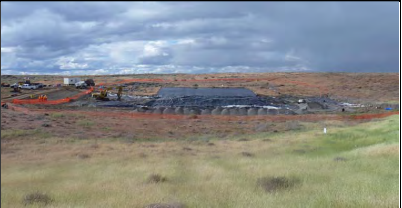
Photo 10: View of the site at the conclusion of work for the day. Orange construction fence is up around the site and gravel is stockpiled for next day's excavation and backfilling work at AE-4 and AE-5. View looking north from hill south of the southern end of the site.
