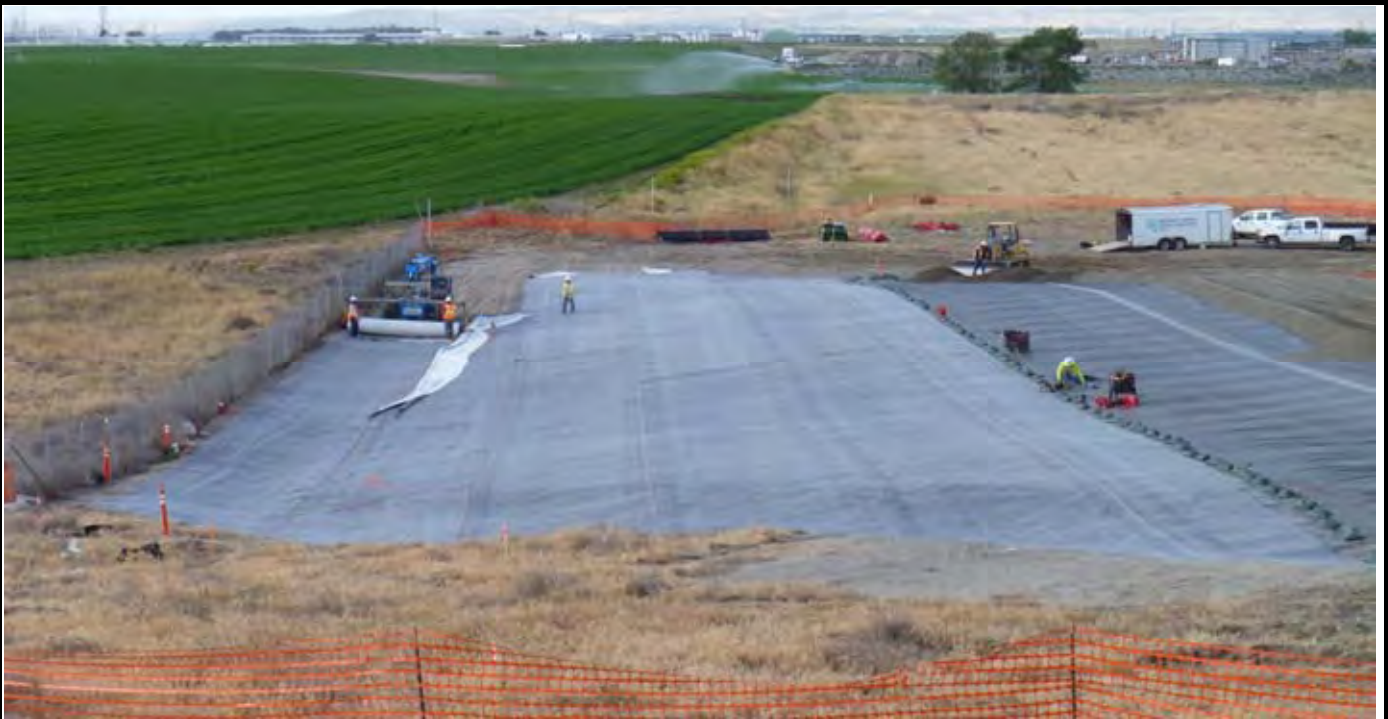
Photo 3: View of NWL rolling out last roll of GCL along the eastern edge of the CAP (EOL zone along fence). View looking south from area north of the northern OCF (see foreground).
