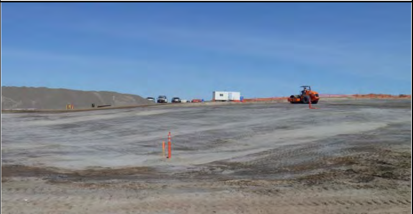
Photo 6: View of AEC compaction roller nearing completion of compacting and smoothing the top of the G-layer cap. View looking NW from SE corner of the site.
