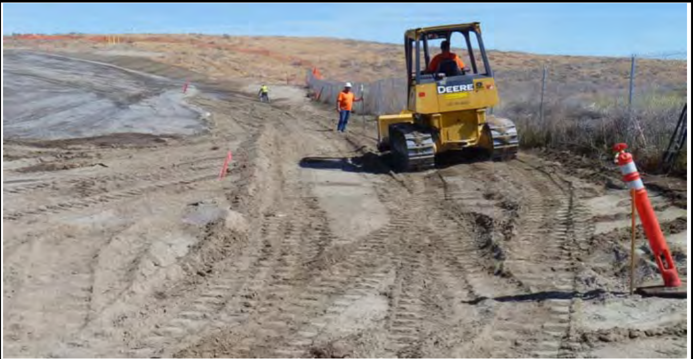
Photo 5: View of AEC grading eastern edge of the site between the EOC (edge of cap) and fence line in accordance with the design. View looking north from SE corner of the site. Note AEC laborer in background smoothing out compaction edges with rake.
