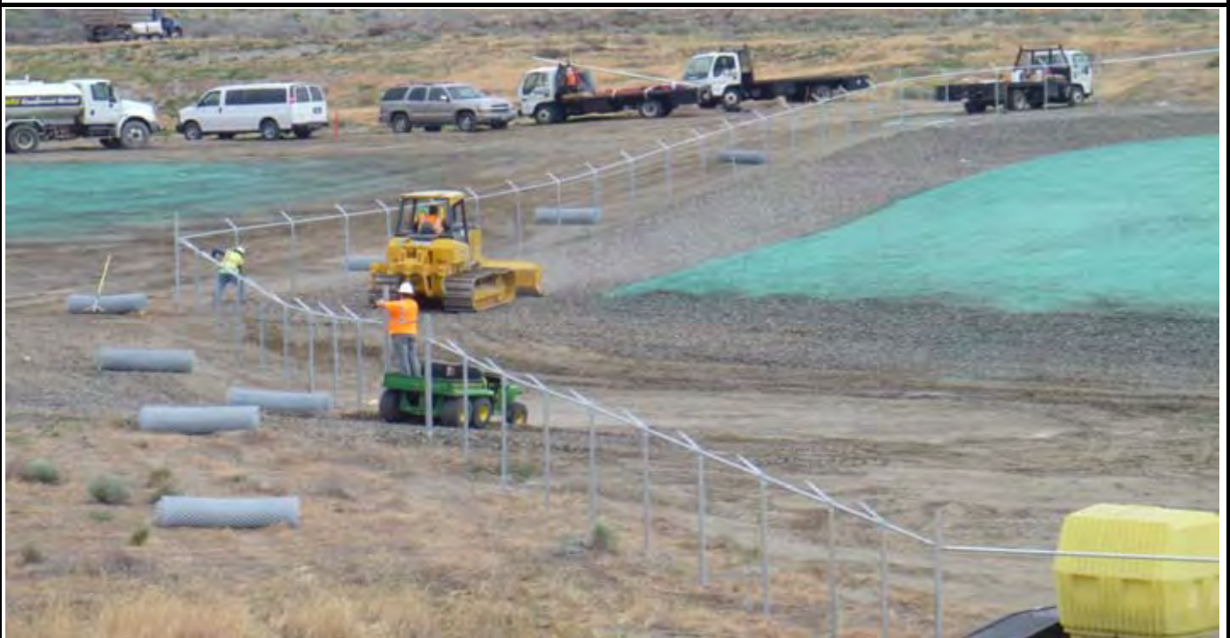
Photo 8: View of Rick's Custom Fencing (RCF) crew installing perimeter fencing components. Note the rolls of fencing materials staged along the perimeter. View of the western side of the CAP from area south of the site.
