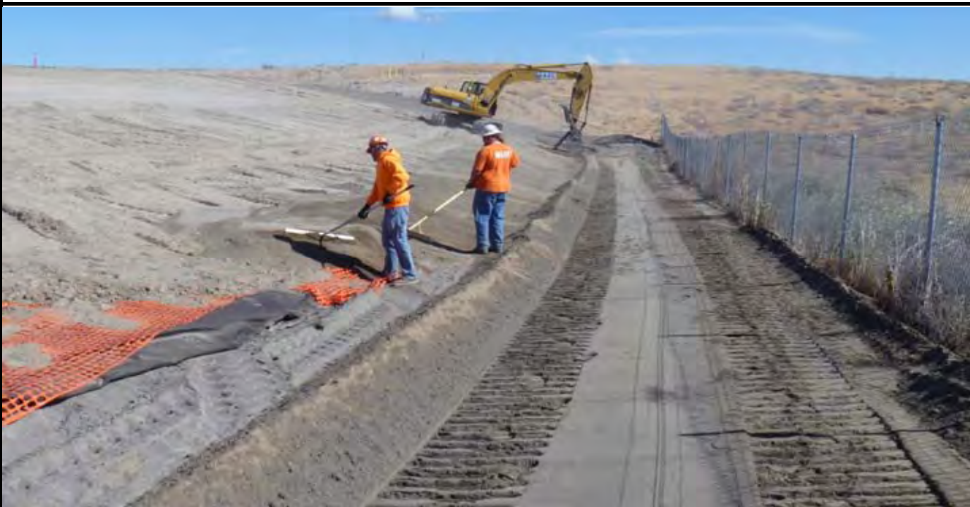
Photo 4: AEC fine grading the EOC along the eastern perimeter of the CAP. Note the bulldozer has graded the perimeter sand layer and prepared it for the Geo-Fabric. View looking north from SE corner of CAP.
