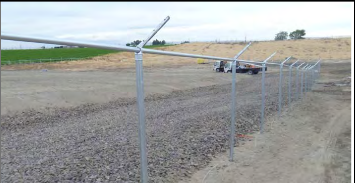
Photo 6: View of the western perimeter fencing with the posts, top bar, and barb wire mounts installed. View looking south from NW corner of the CAP.
