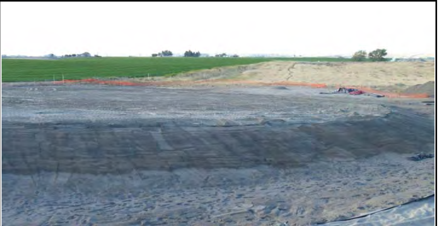
Photo 1: View of the site at the beginning of work for the day. View looking to the South / SE. Note that the NW and western EOC has been graded down into the western and northwestern swales.
