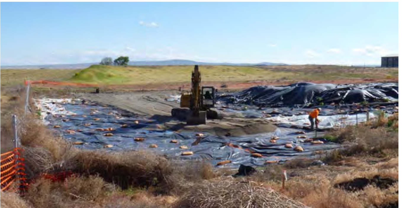
Photo 10: View of AEC installing G-layer access road into the construction zone for trucks and equipment. Photo taken at the end of the work day. View looking south from NE corner of the CAP.
