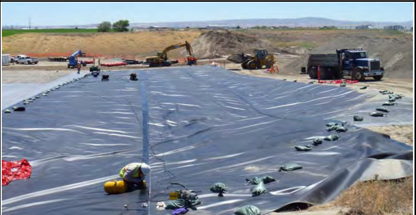
Photo 12: View of NWL worker conducting air test on small section of the weld (S-2) between passes 2 and 3 (P-2/P-3). Seam S-2 failed and NWL conducted several air tests to find the leak. Leak was found on the northern end of the weld and patched by NWL. View looking south from northern end of EOL.
