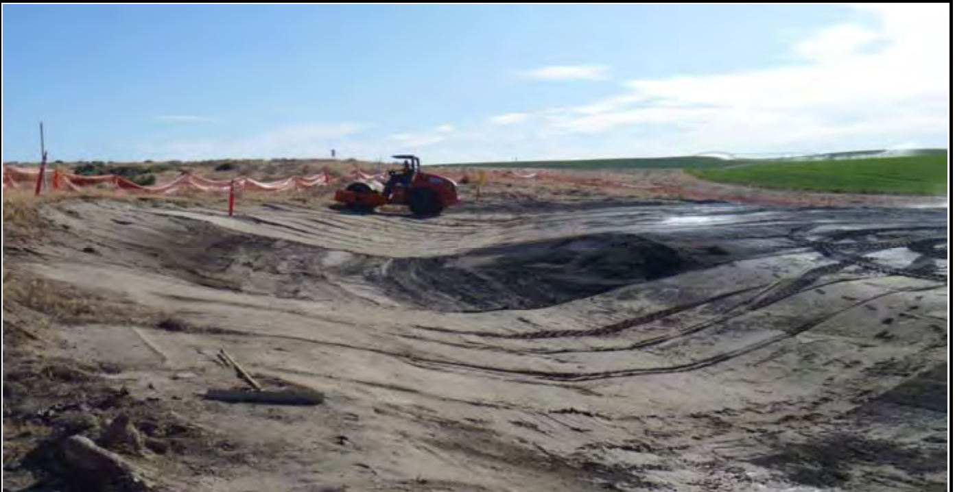
Photo 2: AEC compacting NW swale area and northern edge of cap for preparation for GLC/geomembrane View looking east from NW corner of the site. Un-compacted area needs slight grading work.
