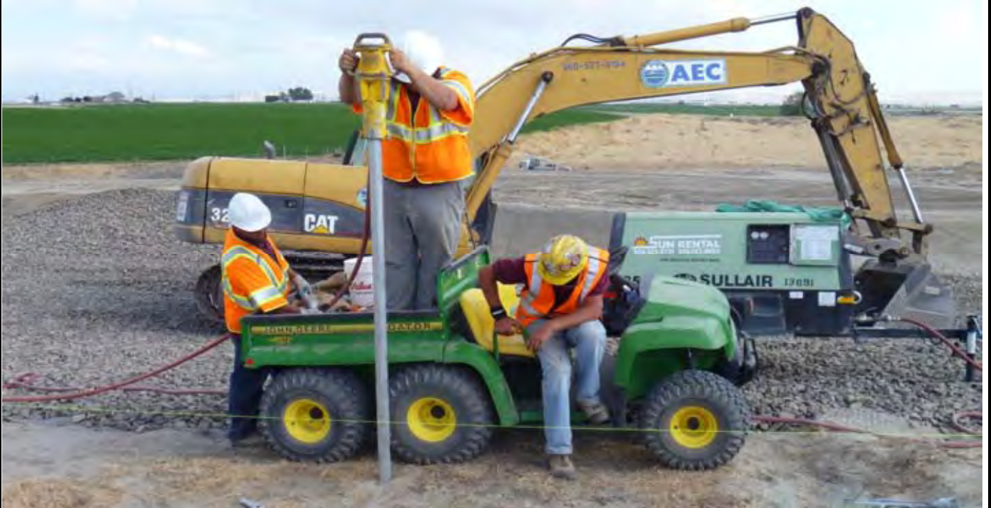
Photo 9: View of Rick's Custom Fencing using a pneumatic hammer (see green compressor in background) to install the majority of the fence posts. Corner posts were installed with concrete early in the project with larger posts. View looking south from NW corner of the CAP.
