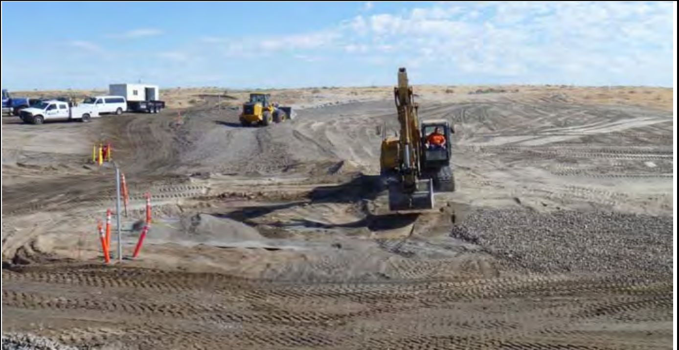
Photo 3: View of AEC grading EOC to EOL area on the SW corner of the CAP and placing rock with loader in the background. View looking north on western half of the CAP from area SW of the CAP.
