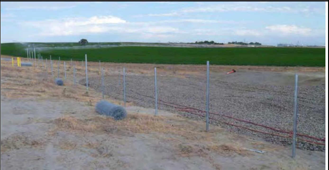
Photo 8: View of the fence posts installed along the northern edge of the CAP perimeter. View looking east to SE from area NW of the CAP perimeter. Note the fencing rolls are not staged for installation.
