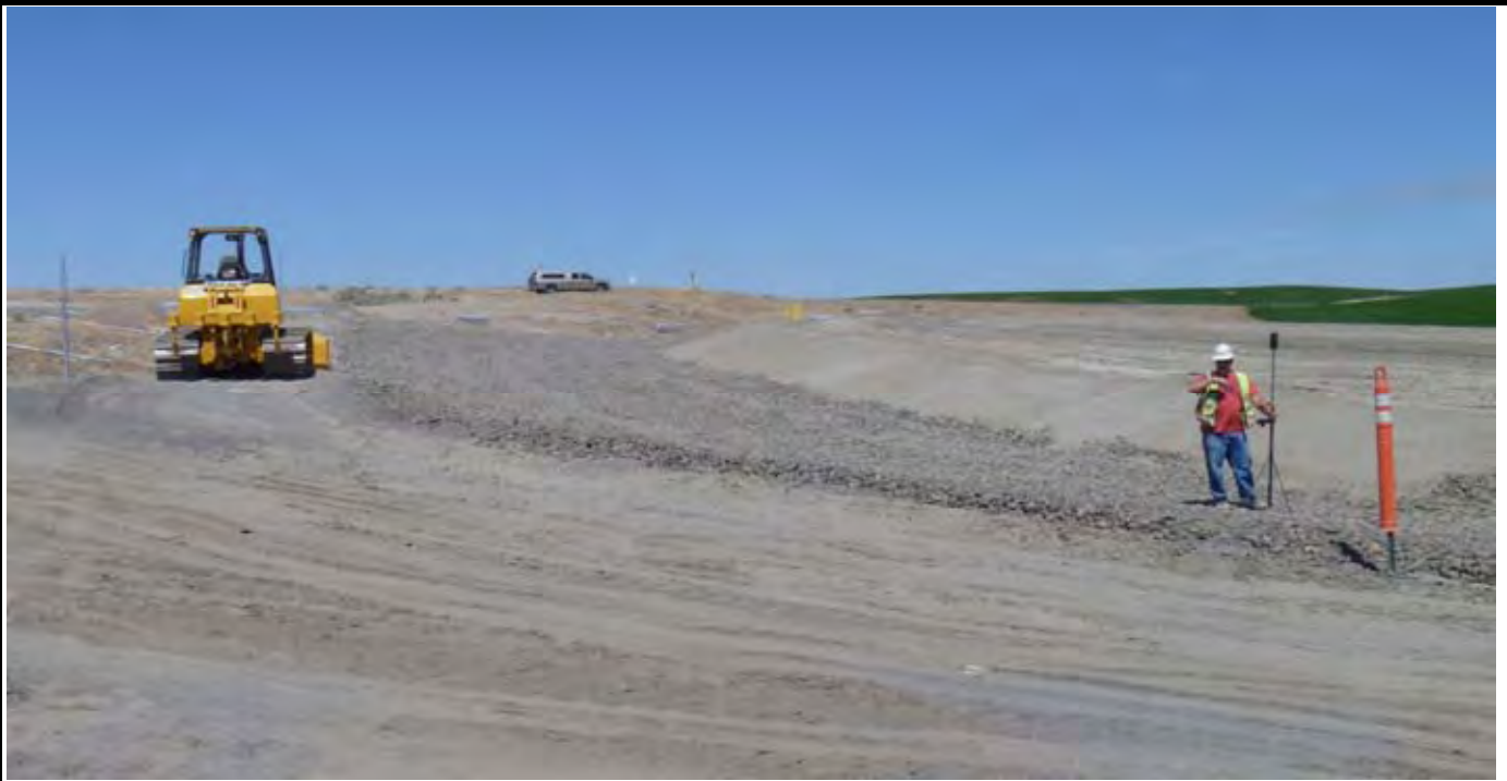
Photo 5: View of DSE conducting the quality control survey of the final CAP grading. View looking NE from western side of the CAP area.
