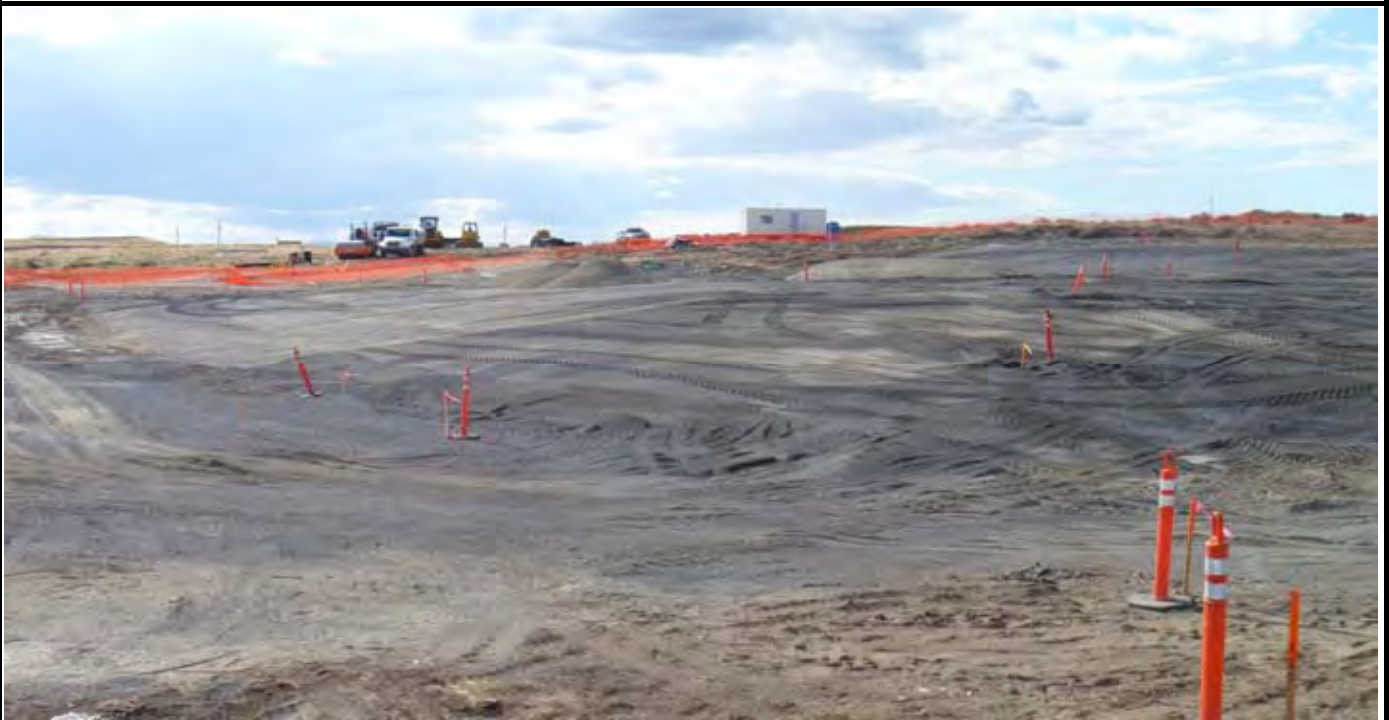
Photo 6: View of the south side of the cap at the end of the day. The G-layer is near final G-layer grade. View looking NW towards the job trailer.
