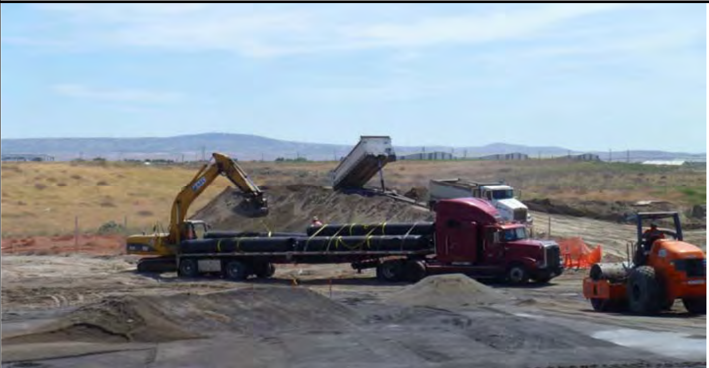
Photo 4: View of AEC off loading three rolls of geomembrane from NW Linings truck. Note trailer in background dumping load of topsoil on stockpile. View looking SW toward SW corner of cap from northern end of site.
