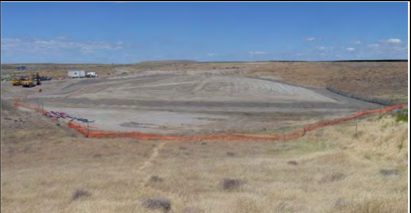
Photo 10: View of the site at the conclusion of work for the day. Note the perimeter rock is installed along the southern EOC to EOL and the CAP is rough graded and ready for final finish grading on Monday and for QC survey on Monday. View looking north from area south of the site.
