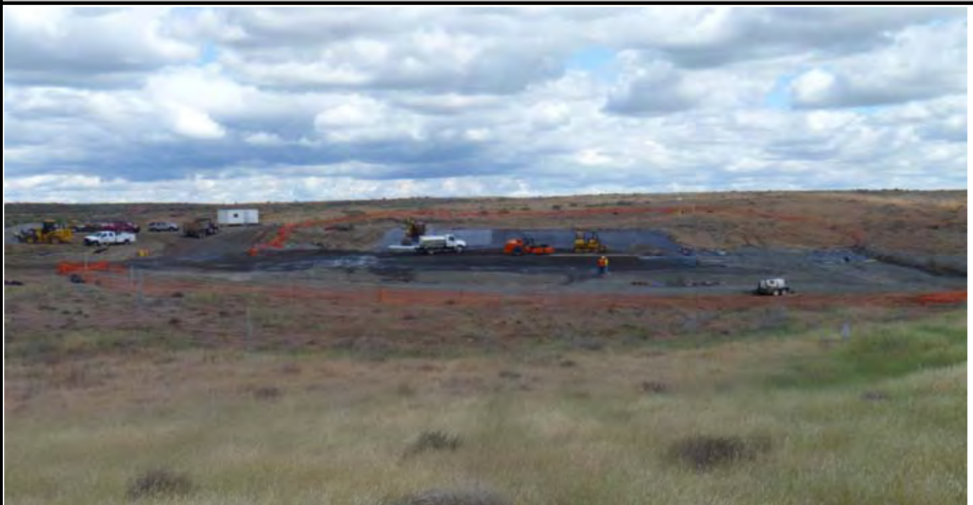
Photo 1: View of the site at the beginning of work for the day. View looking to the north from the south (off of site).
