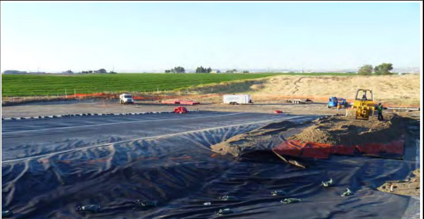
Photo 1: View of the site at the beginning of work for the day. View looking to the South / SE towards the water truck. Note AEC crew prepping for work prior to NWL crew arriving (at 7AM) at about 6:15AM.
