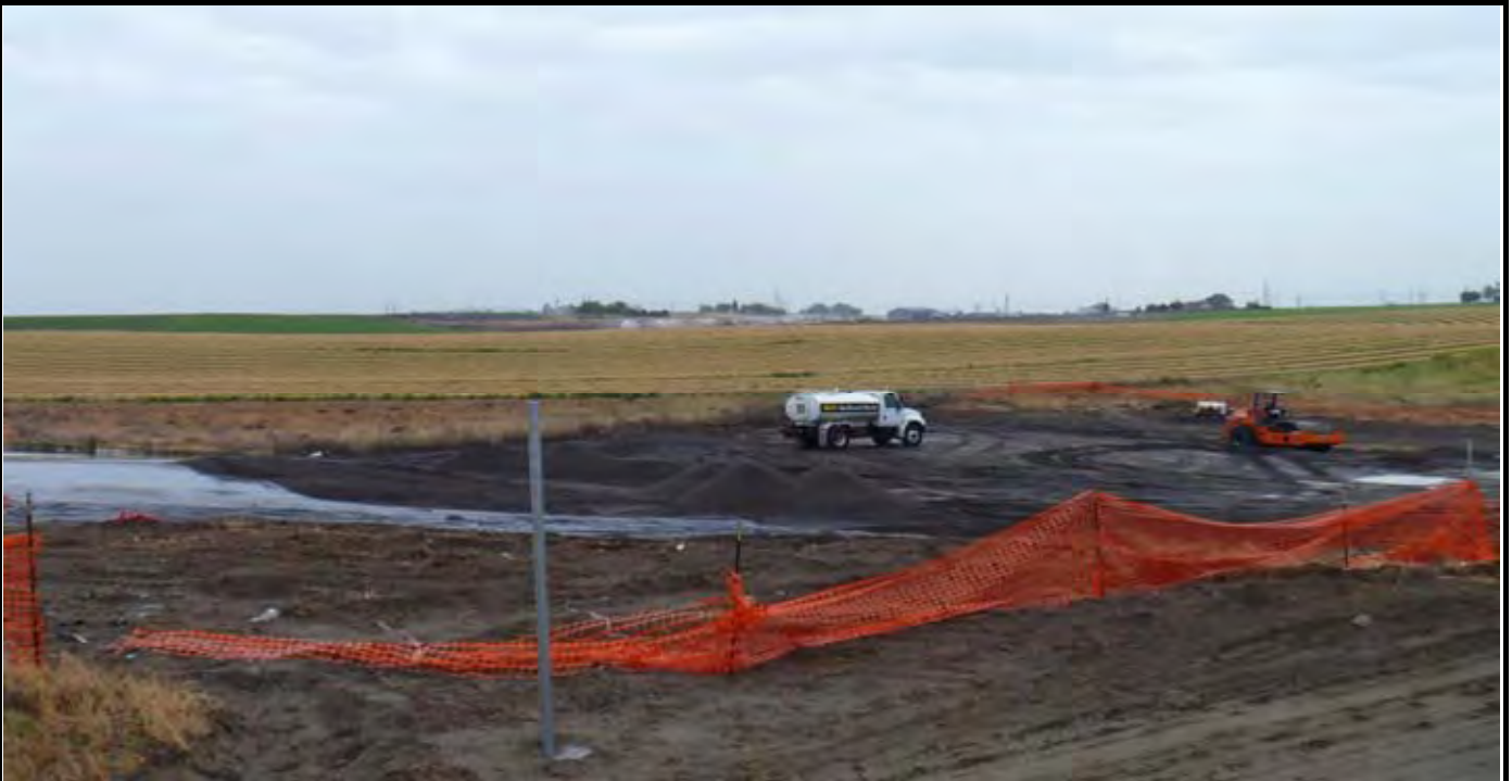
Photo 1: View of the site at the beginning of work for the day. View looking to the SE towards the Roller. Note that all of the surface is wet due to early morning rain.
