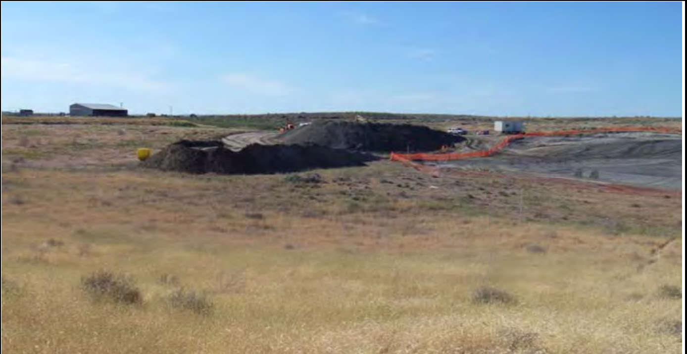
Photo 5: View of the topsoil (front) and sand (back) stockpiles at the end of the day. View looking NW from area beyond south side of site.
