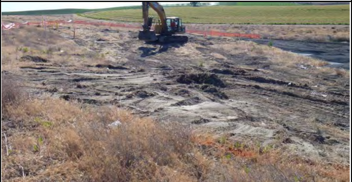
Photo 2: AEC beginning grubbing work on northern end of the site between Edge of Cap and Edge of Liner extension. View looking to the east from the NW corner of the site.
