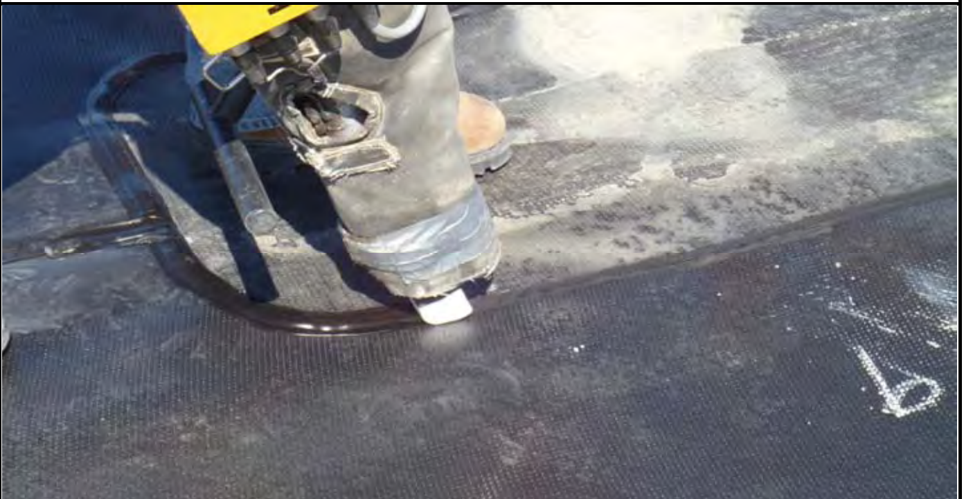
Photo 6: Close-up view of the patch welding machine welding an HDPE seam along patch for seam sample DS-4.
