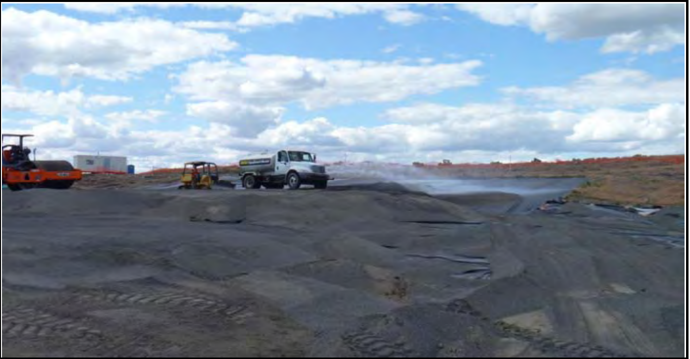
Photo 4: View of AEC water truck watering down G layer gravel that is spread over original cap liner. View looking to the North/Northwest from the SE corner of the site. Note the water truck is on top of the covered "Hump".
