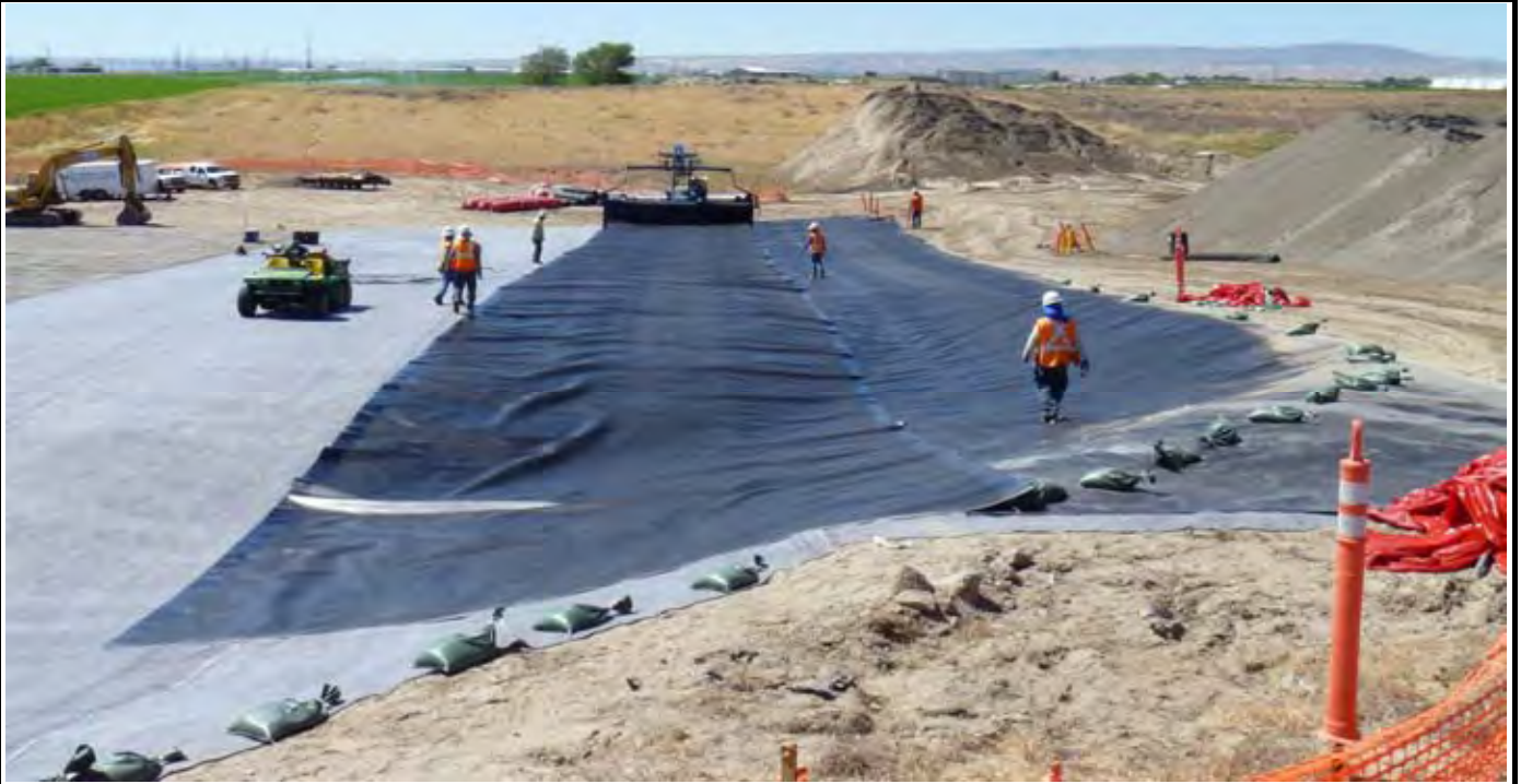
Photo 9: View of the first two passes of the geomembrane (40-mil HDPE liner with microspike texture on one side). Note second liner overlaps the first. View looking south from area north of the NW corner of the EOL.
