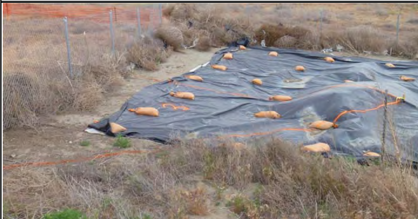
Photo 5: View of AE-3 area marked out in orange spray paint prior to fence removal. View looking east from western side of AE-3.
