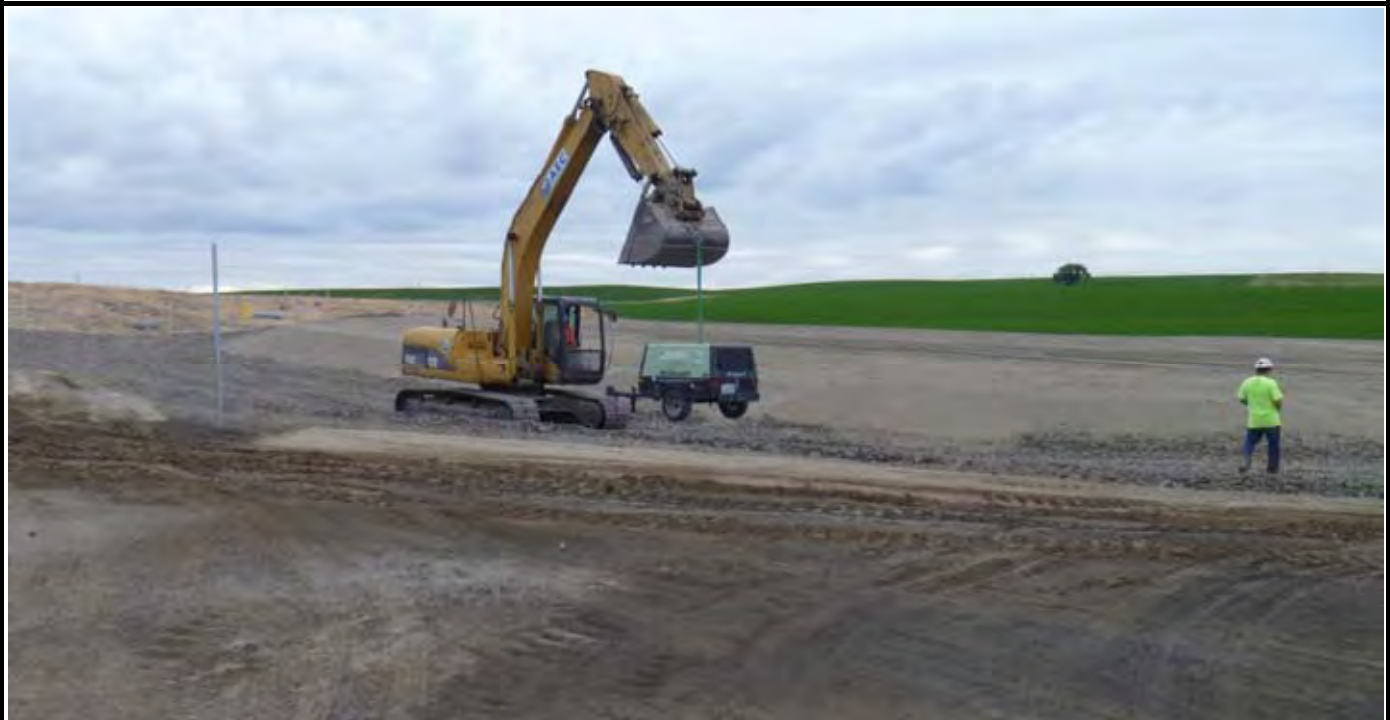
Photo 2: View of AEC moving the towable compressor for Rick's Custom Fencing to the western perimeter of the CAP so they can use it to install the fence posts. View looking east from the western side of the CAP.
