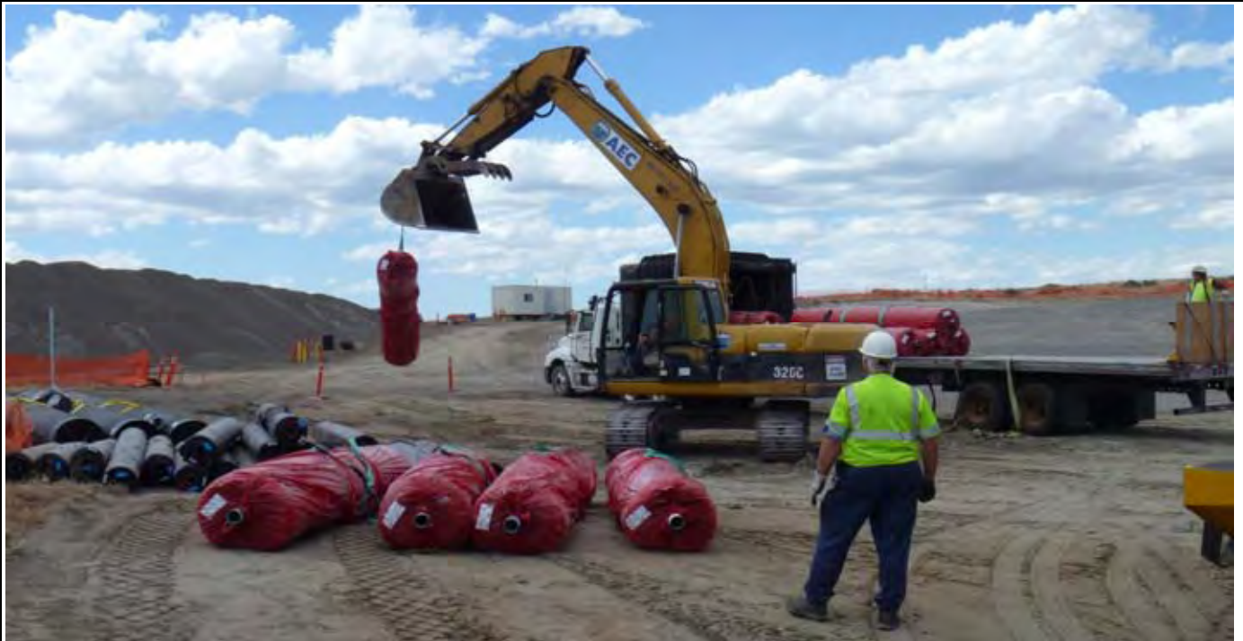
Photo 5: View of AEC trackhoe off loading the rolls of GCL (red rolls) from the flat bed truck. View looking NW from southern end (infiltration basin area) of site.
