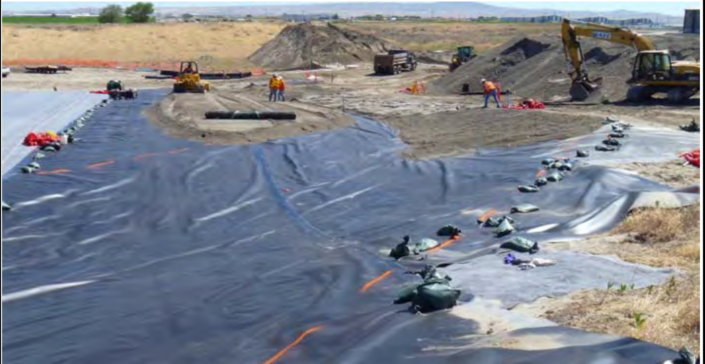
Photo 15: View of EOC installing sand layer over the geomembrane along the western side of the geomembrane (only three passes of geomembrane). Note orange dashed lines (foreground = EOL and center is EOC lines) and geosynthetic fabric (geo-fabric) rolls on sand that AEC is about to roll out over top of sand. View looking south from northern edge of EOL.
