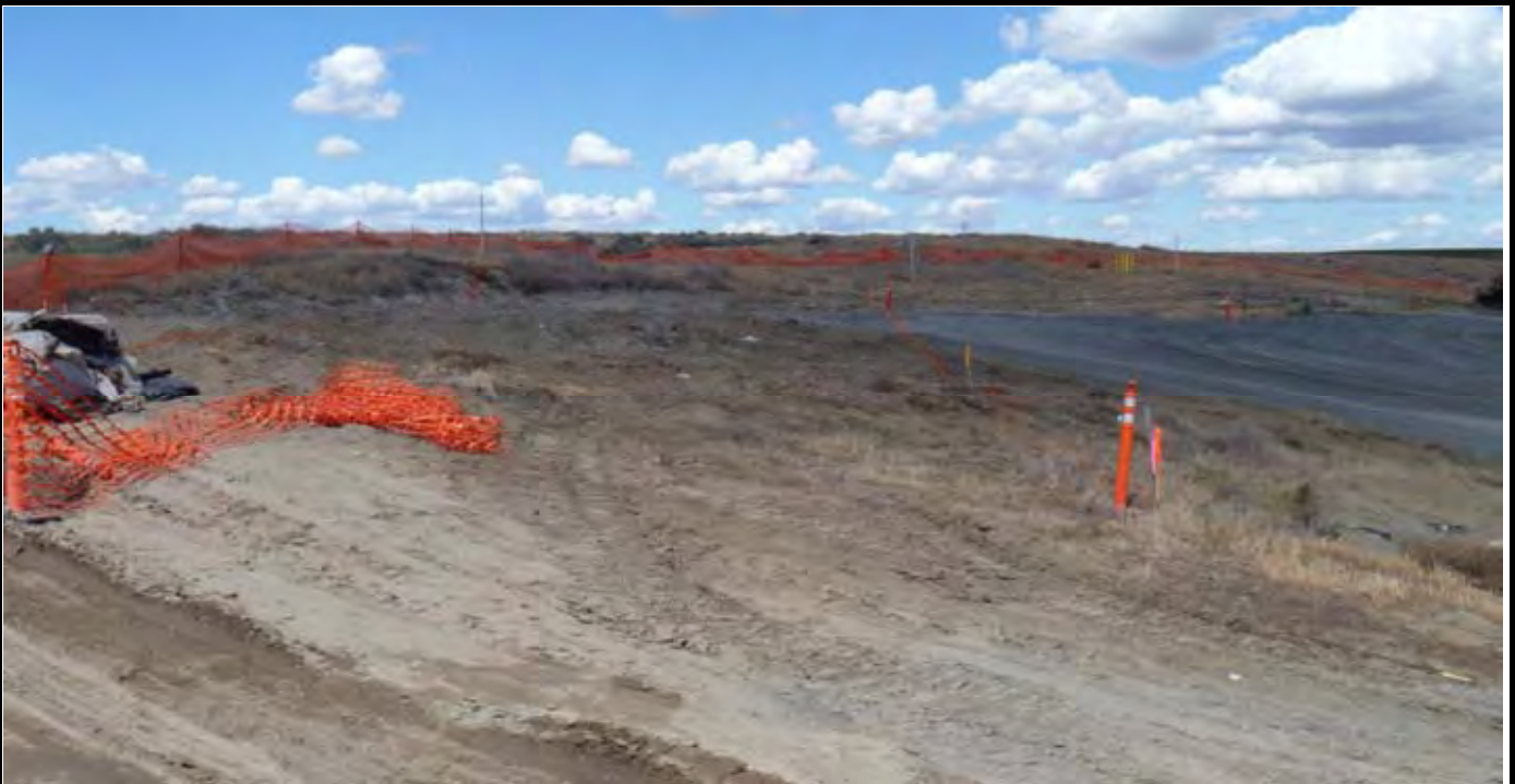
Photo 5: View of the layout lines (orange) for NW swale between the EOC and EOL. View looking NE from the western edge of the site.
