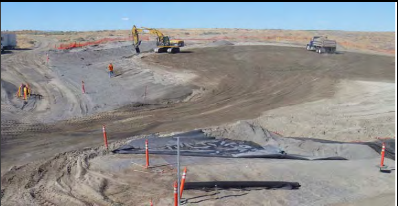
Photo 4: AEC trackhoe grading out the EOC with western and NW swales with sand and topsoils. Note that the water truck has watered the roadway and top of cap to keep dust down. View looking N from SW corner of the site.
