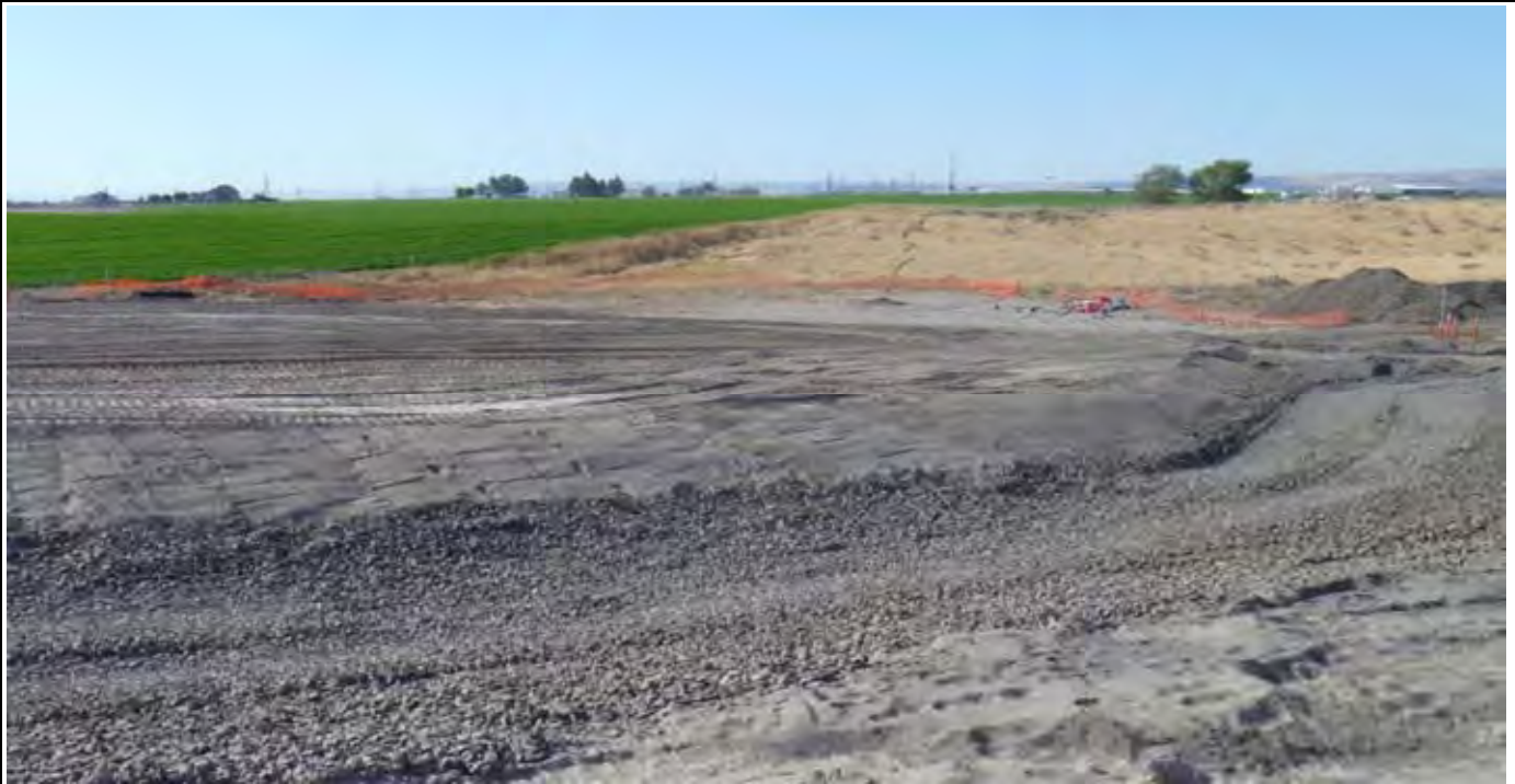
Photo 1: View of the site at the beginning of the day. Note the erosion protection rock stockpile (right edge of photo) and lack of fence posts. View looking south from NW corner of the CAP.
