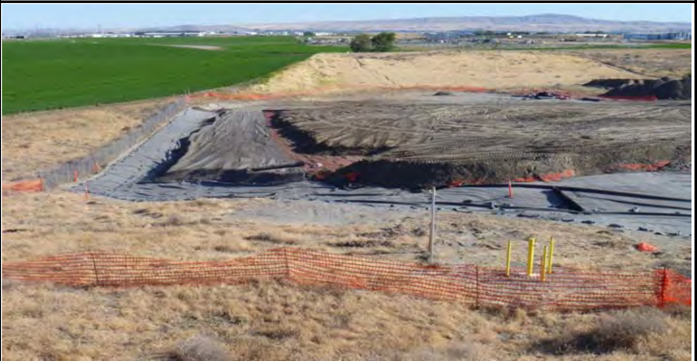
Photo 10: View of the eastern half of the CAP and showing that the sand layer has been completed to the boundaries of the EOC (edge of CAP). Remaining work for CAP include Geo-Fabric/OCF placement and topsoil placement and grading. View looking south from area north of the site (near survey pin).
