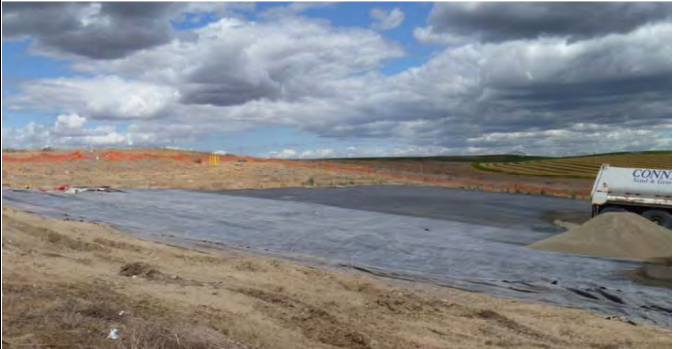
Photo 5: View of the Old GCL rolls completely rolled out onto area along western edge of the original cap. Note the gravel on the right side. AEC is beginning to cover the old GCL with G layer gravel. View looking to the east from the western side of the site.
