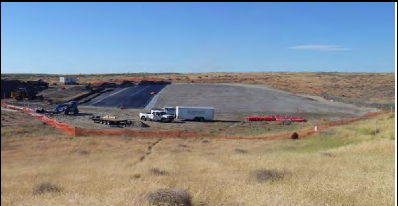
Photo 18: View of the site at the end of the day. NWL has installed approximately 35% of the GCL and geomembrane. AEC has just begun covering the geomembrane with sand and topsoil layers along the western edge of the CAP. View looking north from the area south of the southern end of the site.
