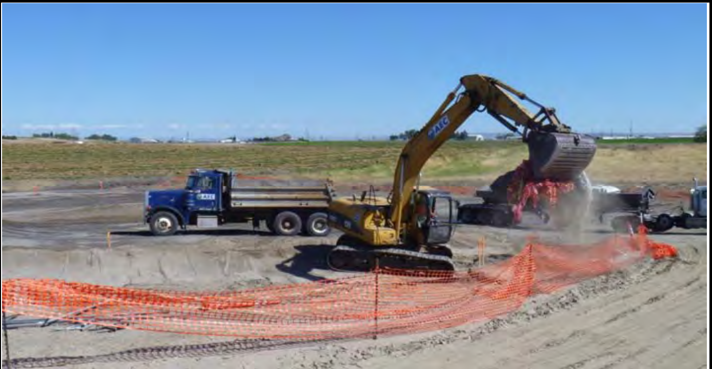
Photo 7: View of the AEC trackhoe loading remaining debris and garbage into the AEC dump truck along the western side of the site. View looking to the SE from the NW corner of the site.
