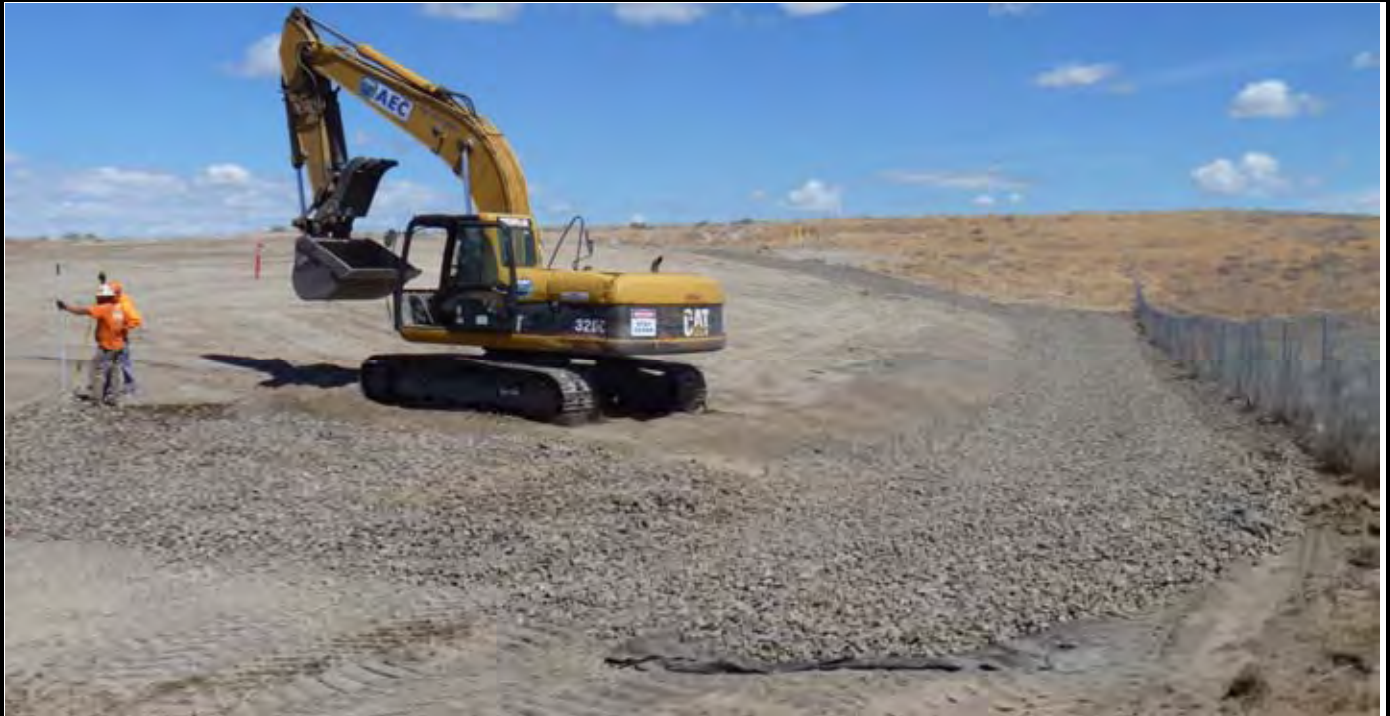
Photo 7: View of AEC completing the perimeter rock installation on the eastern swale and starting the perimeter rock work on the southern EOC to EOL zone. View looking north from the SE corner of the site.
