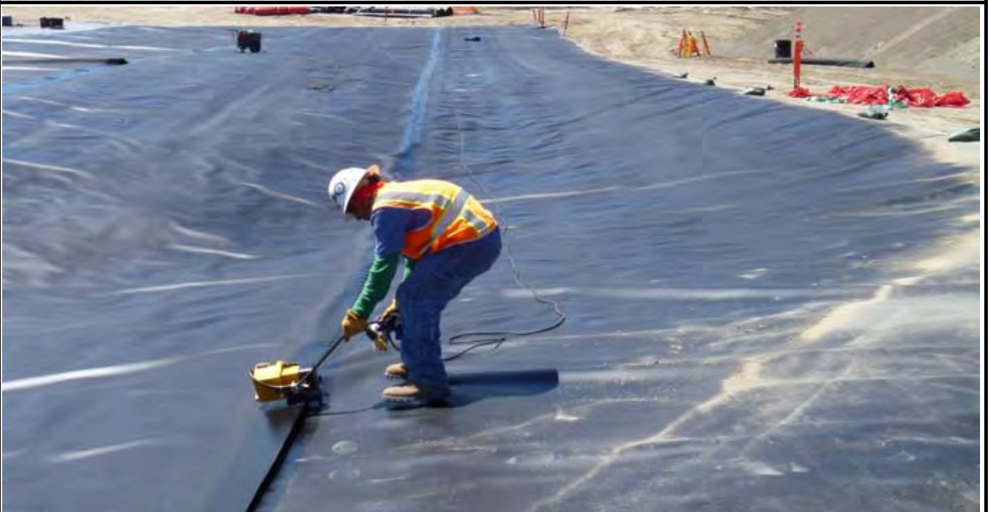
Photo 10: View of NWL worker welding the first and second pass of geomembrane together with welding machine. Note that there are three passes of geomembrane over the GCL now. View looking south from NW corner of EOL.
