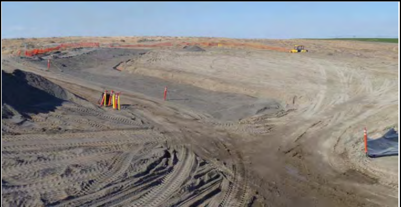
Photo 11: View of the NW and western swale (between EOC and EOL) with sand installed and ready for Geo-Fabric and overlying perimeter rock layer. View looking NE from area just west of the SW corner of the CAP.
