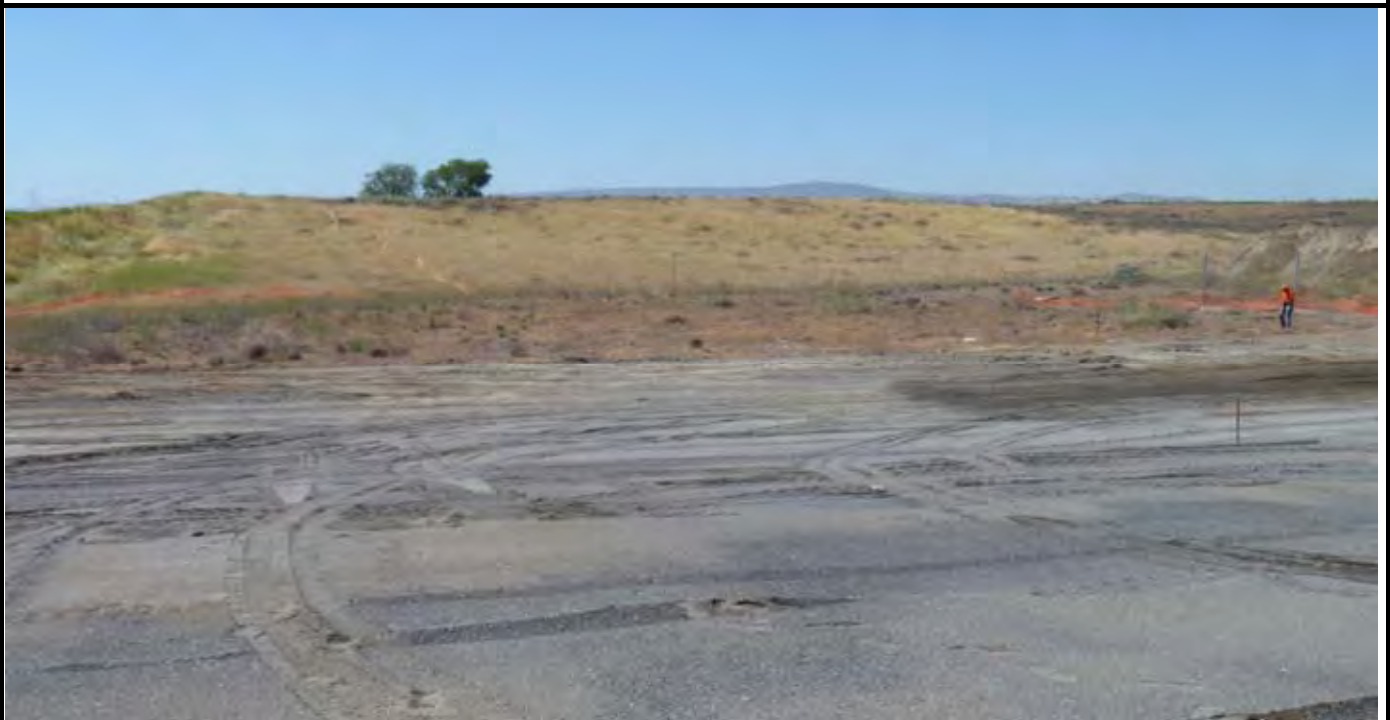
Photo 2: View of infiltration basin area prior to grubbing/grading work. Note AEC is moving OCF back to posts for the new perimeter fencing. View looking south from south end of cap.
