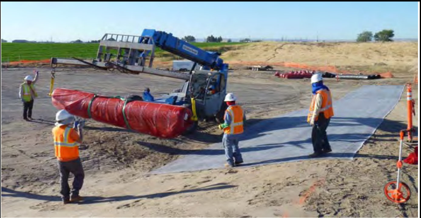
Photo 3: View of NWL positioning to roll out the second GCL roll along the eastern edge of the first GCL roll (which is installed along the western EOL down to the SW corner - see background). View looking south from NW corner of EOL. Note roller assembly held up by telehandler.
