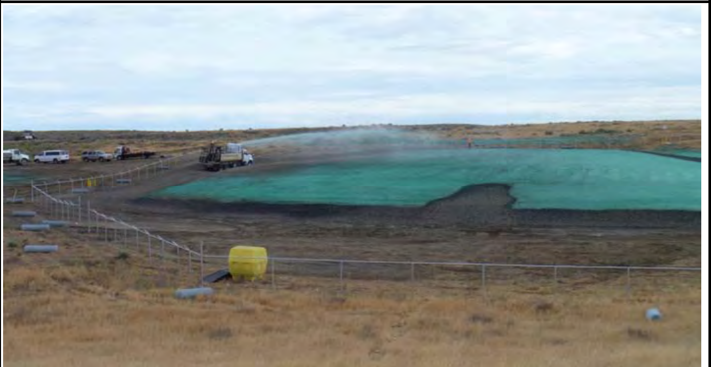
Photo 6: View of Wildlands completing the hydroseeding of the western half of the CAP from the western perimeter access road. View of the site from area south of the site.
