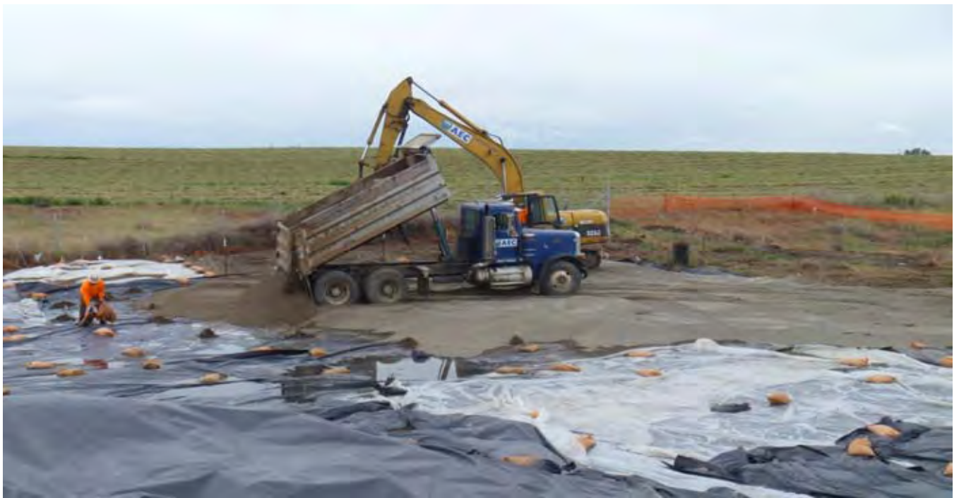
Photo 9: View of AEC installing base layer of G-layer material to provide access to the construction area for trucks and equipment for further G-layer installation. View of SE corner of the CAP from center of CAP.
