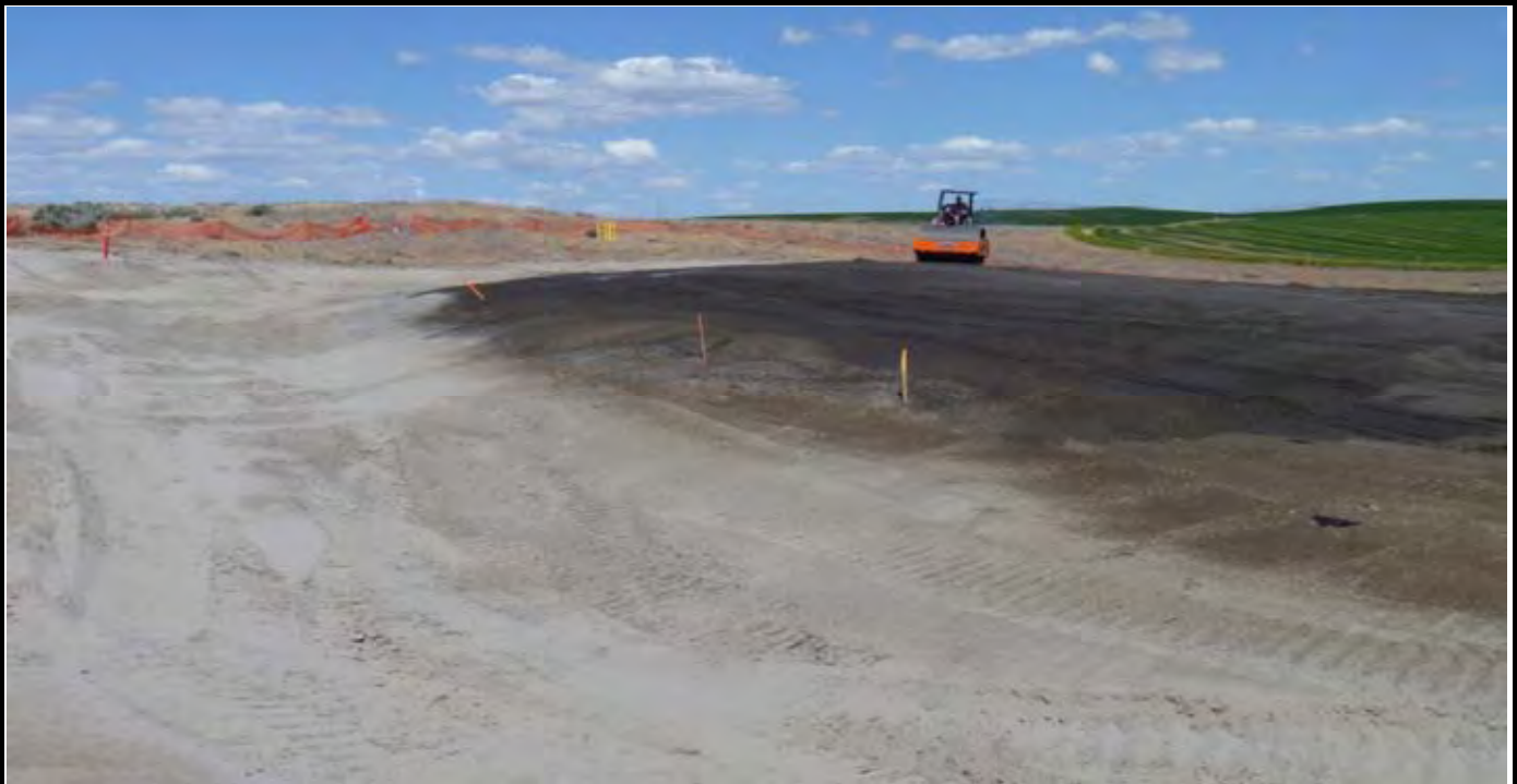
Photo 3: View of the northern end of the G-layer. Note the peak along the northern edge of the cap area. View looking northeast by east from western side of site.
