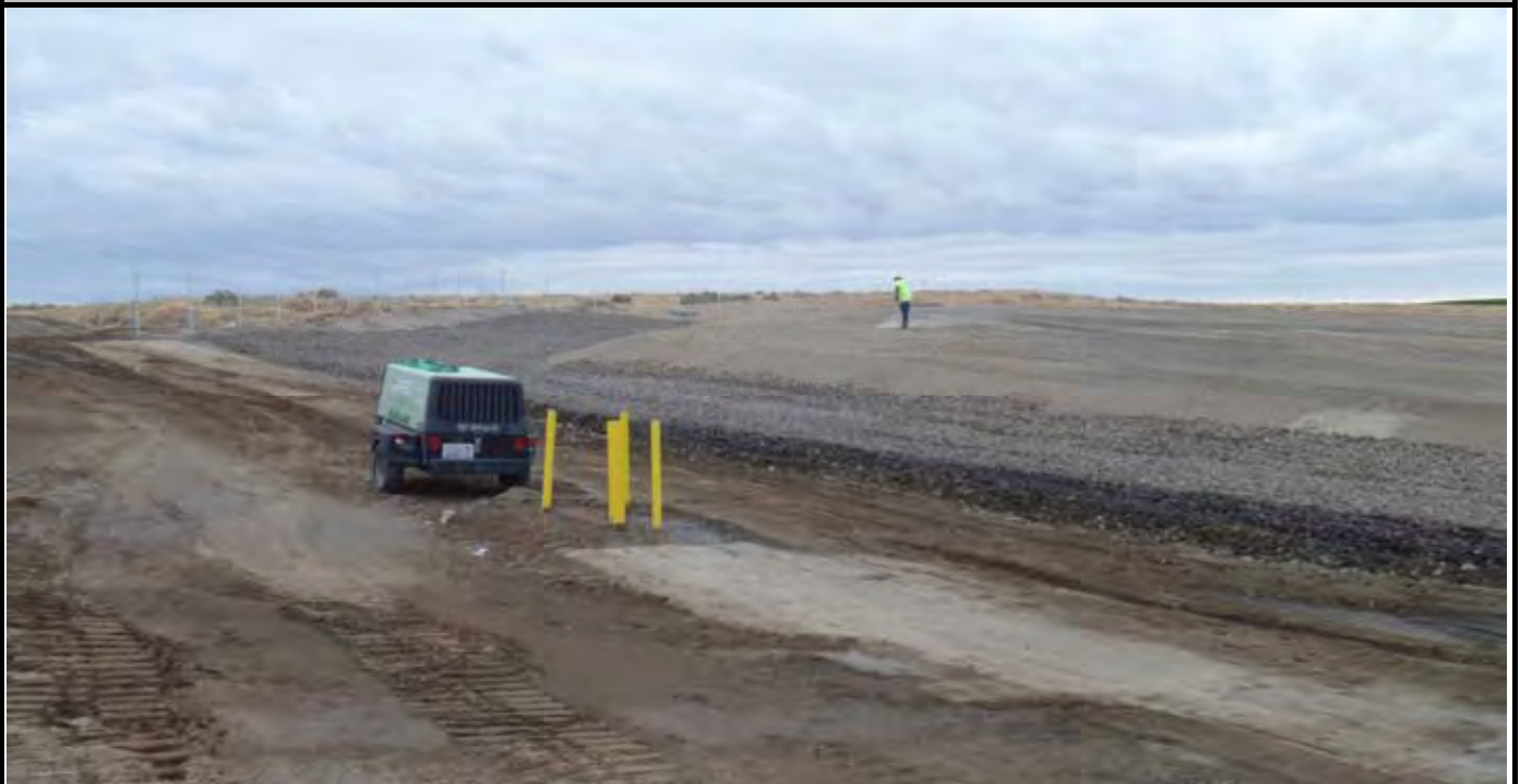
Photo 3: View of the western side of the CAP prior to installation of the fencing posts. Note the towable compressor near the monitoring well. View looking north/northeast from SW corner of the CAP.
