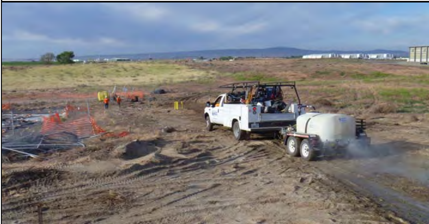
Photo 2: AEC watering the site roadways at the beginning of the day with trailer mounted watering equipment. View looking south along western side of CAP.
