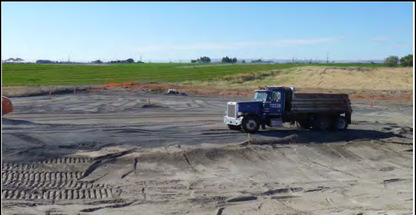
Photo 1: View of the site at the beginning of work for the day. View looking to the South / SE beyond the dump truck. Note the NW swale in the foreground and grading control points.
