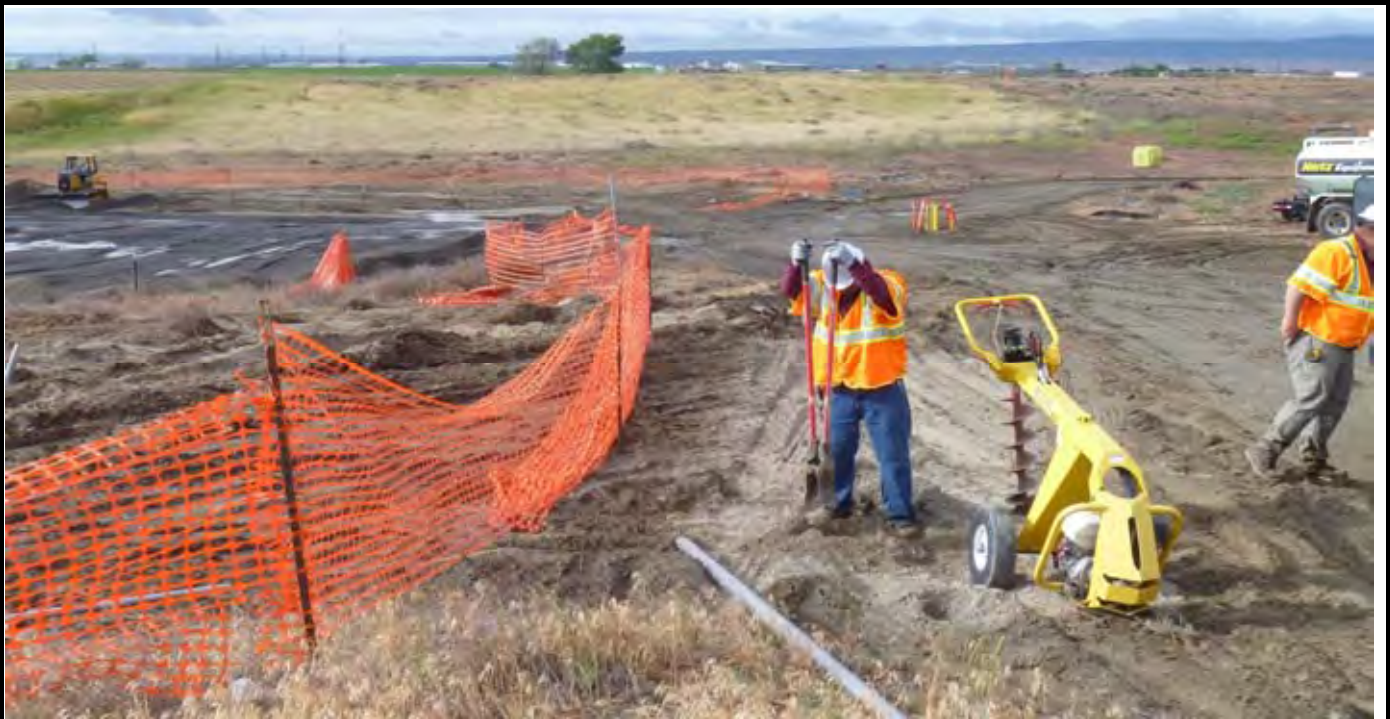
Photo 3: View of Rick's Custom Fencing beginning the installation of the corner fence posts for the perimeter fencing outside the construction zone. View looking to the south.
