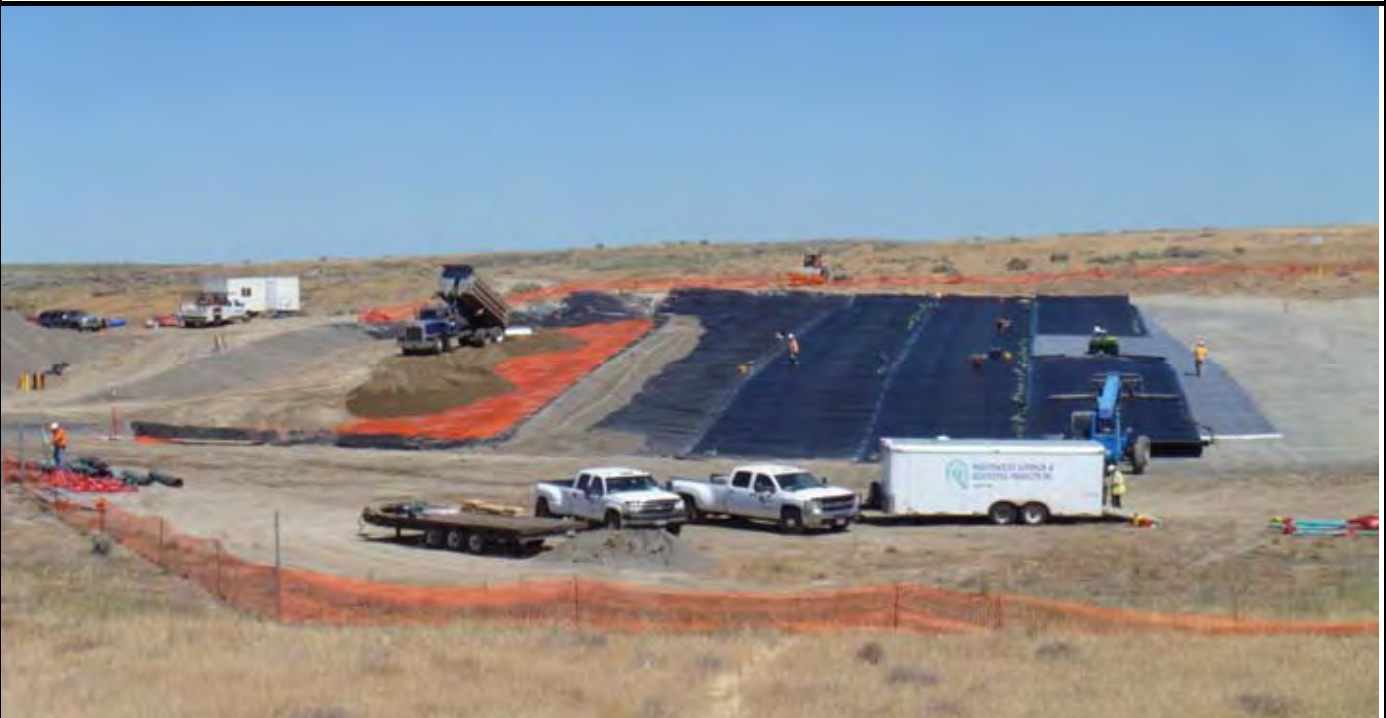
Photo 8: View of NWL pulling last geomembrane panel of the day up to butt joint over final GCL panel. View of AEC dropping and grading topsoil (see dump truck) over OCF overlying black geo-fabric which overlies the 1-ft sand layer. View looking north from area south of the site.
