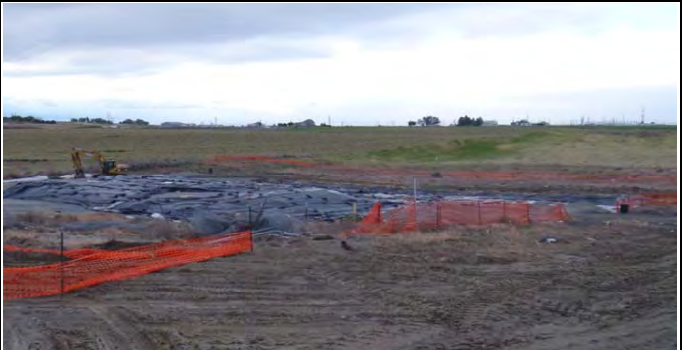
Photo 1: View of the site at the beginning of work for the day. View looking to the SE corner (adjacent to trackhoe).
