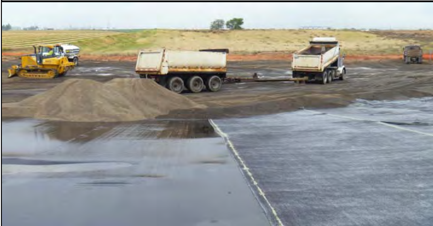
Photo 3: View of gravel trucks dropping gravel on G-layer on top of old GCL rolls and original cap liner. View looking south from northern edge of original cap liner.
