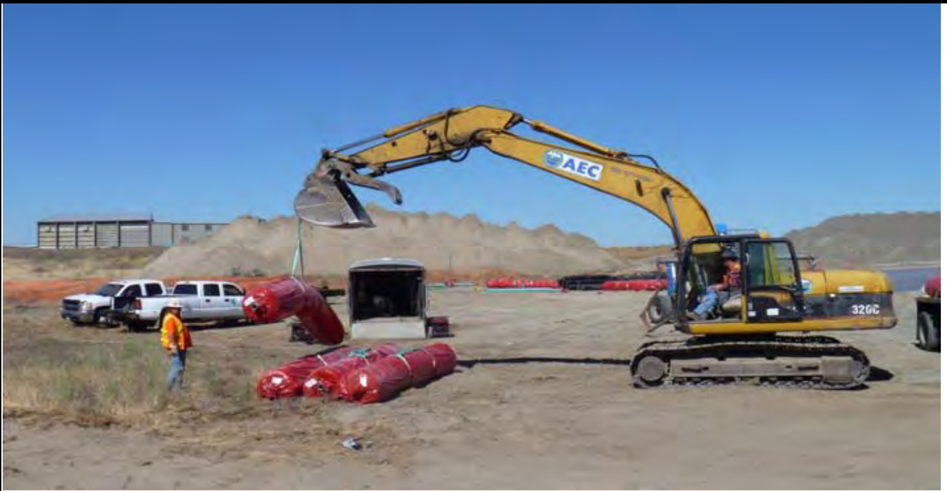
Photo 7: View of AEC trackhoe and crew off loading 14 new GCL rolls from the flatbed truck and staging them in area south/southeast of the CAP (note GCL rolls in the background that were off loaded yesterday). View looking west from area south of the SE corner of the EOL.
