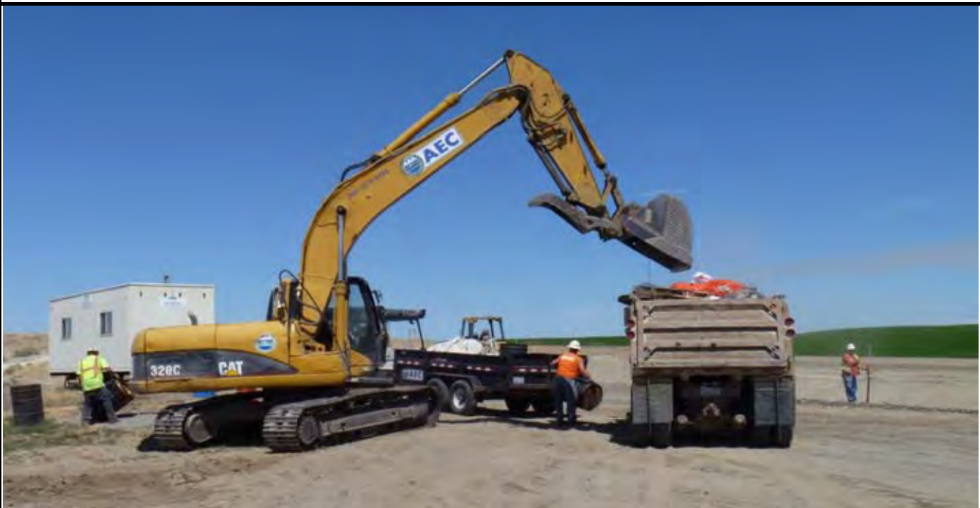
Photo 6: View of AEC loading out the remaining debris from the site during the DSE quality control survey work. View of area west of the CAP from area SW of the CAP.
