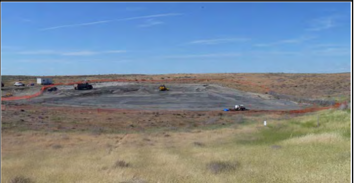
Photo 10: View of the site at the conclusion of work for the day. Orange construction fence is up around the site and all crews gone. View of the site looking north from beyond the southern edge of the site.
