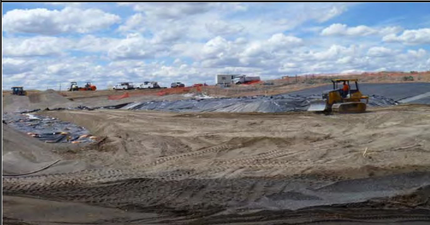
Photo 7: View of the excavated soils from AE-4 and AE-5 being spread around the base of the "hump" by the bulldozer. View looking to the Northwest.
