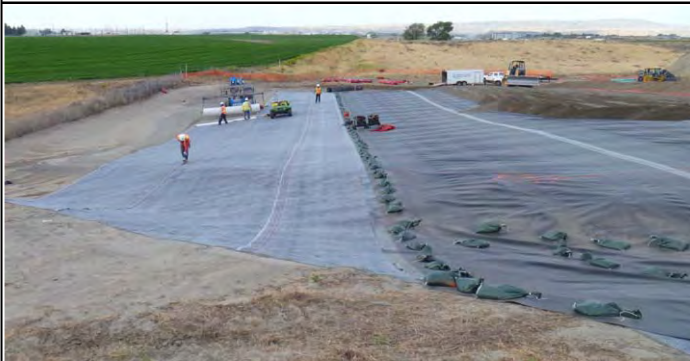
Photo 2: View of NWL rolling out GCL layer on east side of CAP. Note AEC working on sand layer on the right side of the picture. View looking south from north side of the EOL.
