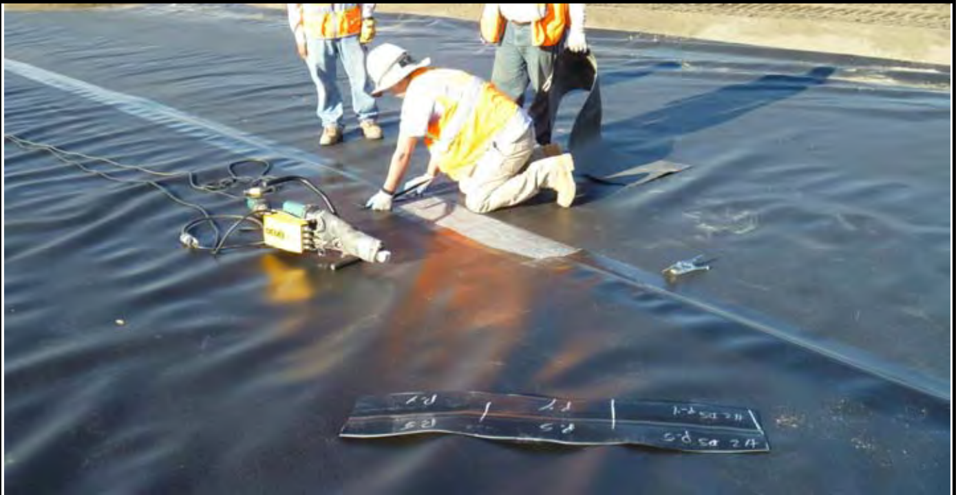
Photo 3: View of NWL crew cutting out destructive test sample DS-2 along seam S-4 for field testing. View looking southwest towards SW corner of CAP.
