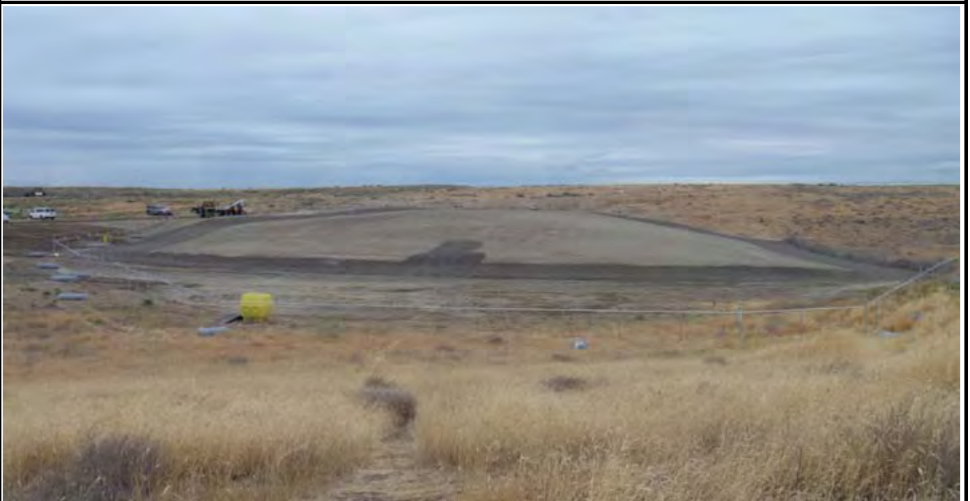
Photo 8: View of the entire site near the end of the working day from area south of the site. Note that fencing work is underway with rolls staged around fence perimeter.
