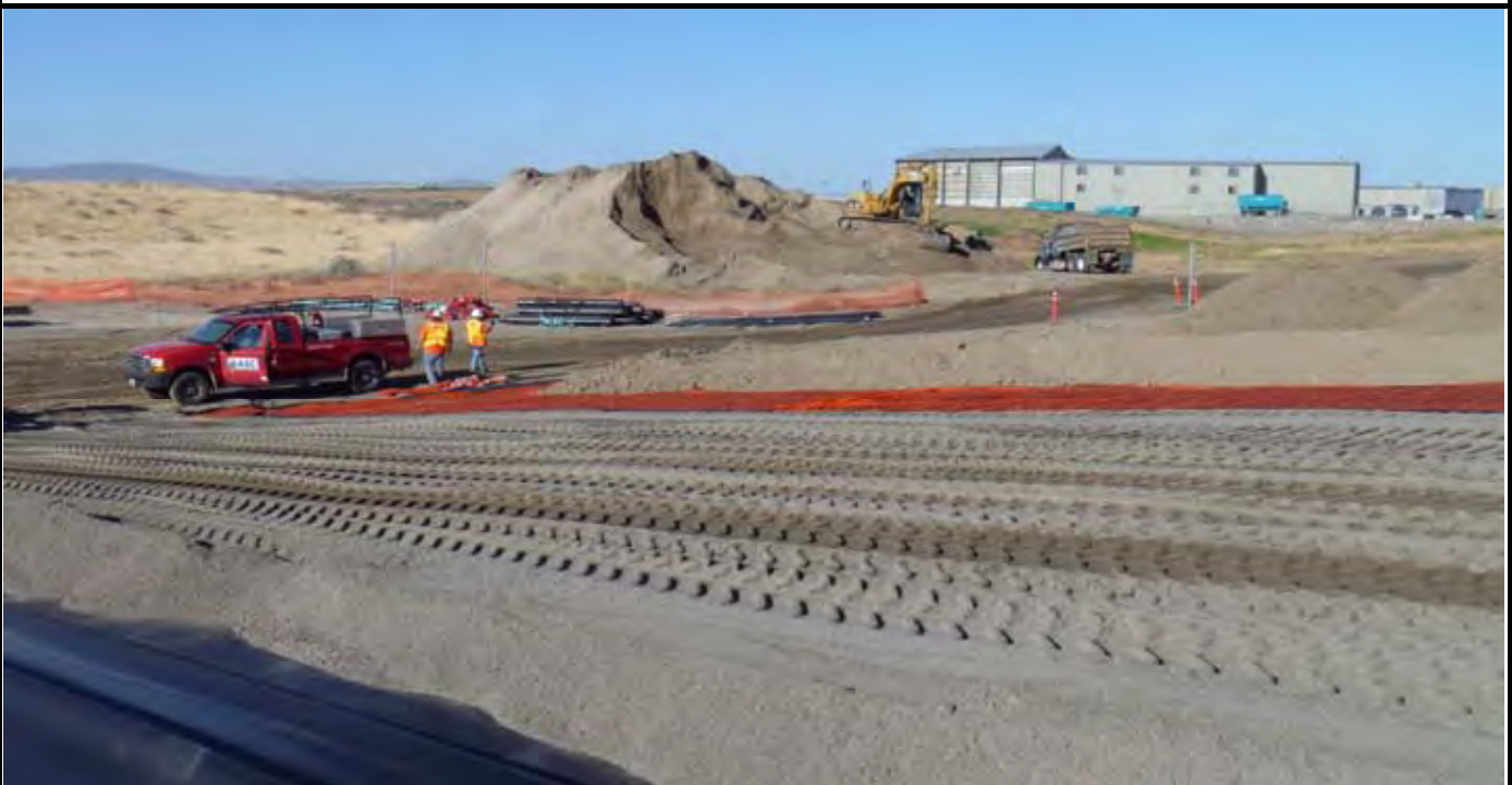
Photo 2: View of graded sand layer ready for Geo-Fabric and OCF installation before topsoil placement (see background of Geo-Fabric and OCF edge along eastern edge of topsoil layer. View looking SW from center of CAP.
