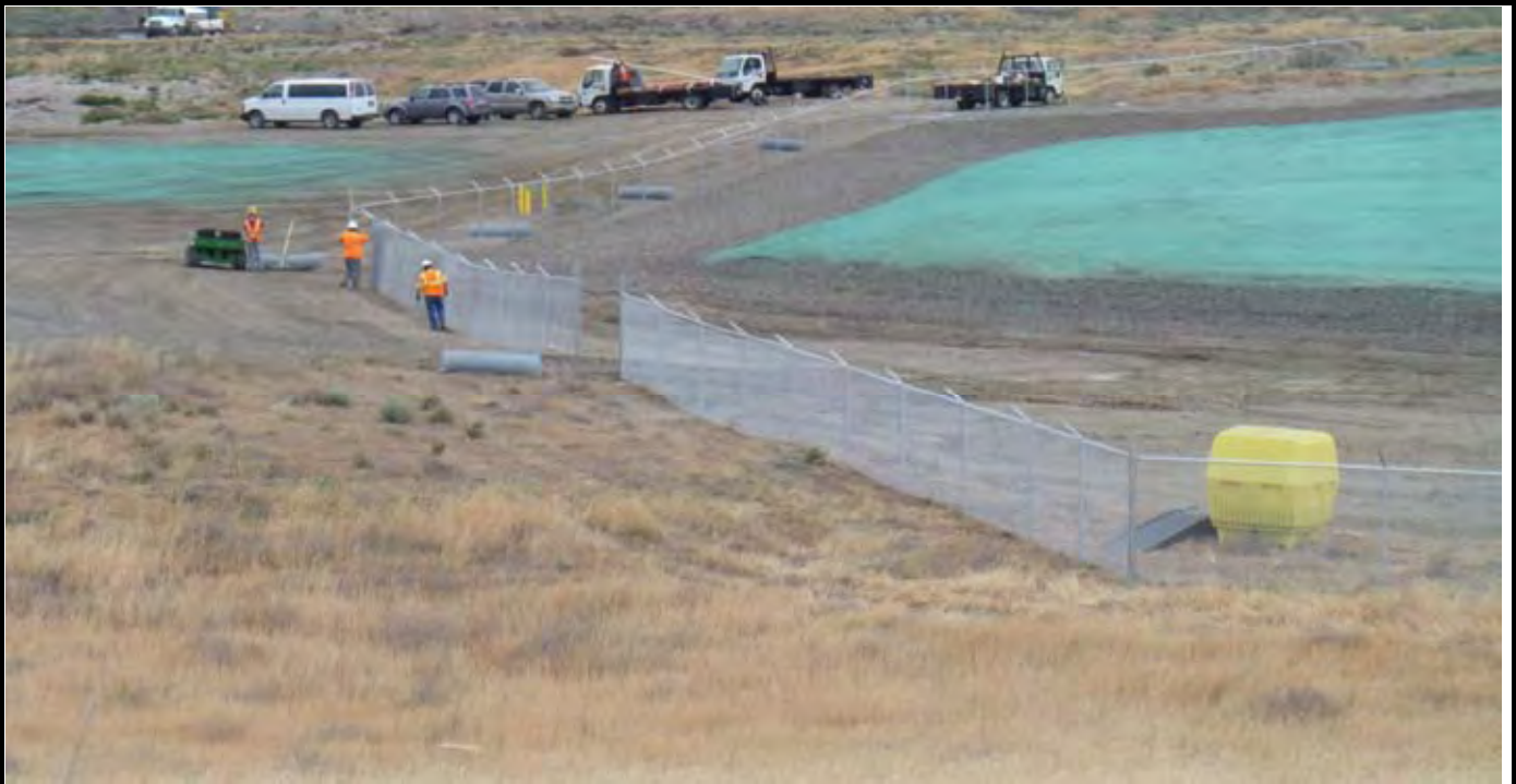
Photo 9: View of the west and southwestern side of the CAP where RCF is installing the fencing on the posts. View of the western side of the CAP from area south of the site.
