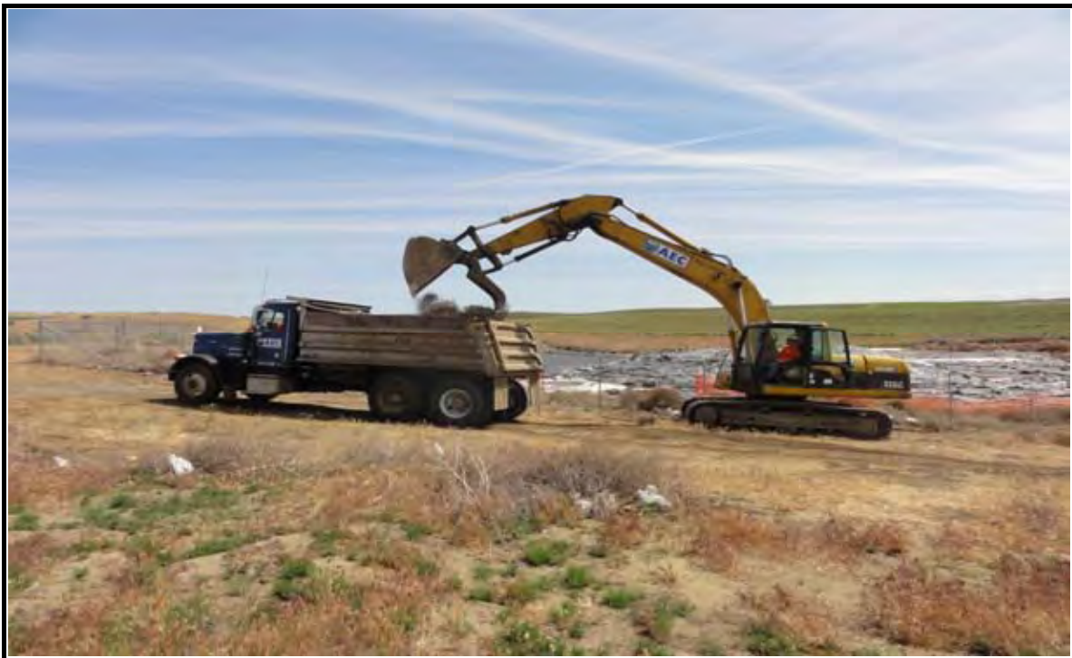
Photo 2: Loading tumbleweeds into dump truck along west side of the site (outside cyclone fence). View looking east.
