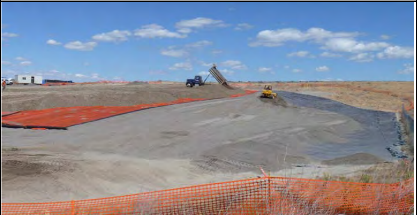
Photo 5: View of the eastern edge of the CAP during mid-day. Note bulldozer grading the sand layer over the geomembrane and AEC dump truck placing topsoil piles for later grading. Note Geo-Fabric and OCF between the sand and topsoil layers. View looking north from the SE corner of the site.
