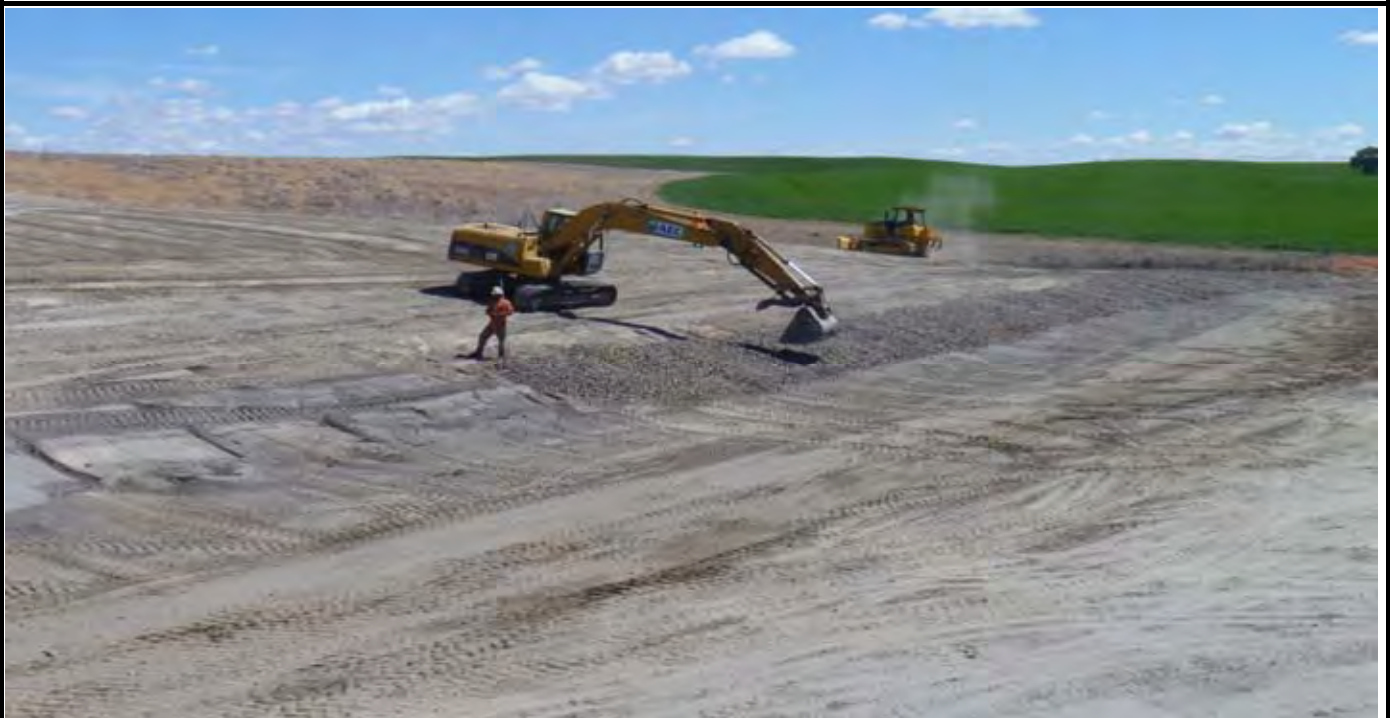
Photo 8: View of AEC trackhoe installing and grading the perimeter rock along the center of the southern EOC to EOL. View looking east/NE from rock pile located SW of the SW corner of the CAP.
