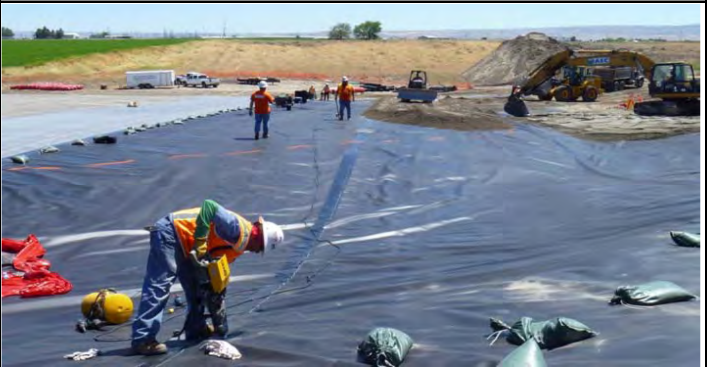
Photo 14: View of NWL worker patching the leak area on seam S-2. Note AEC in the background is beginning to cover the geomembrane with a 1-ft thick layer of sand. See orange dashed line that shows the EOC. View looking south from northwest corner of EOL.
