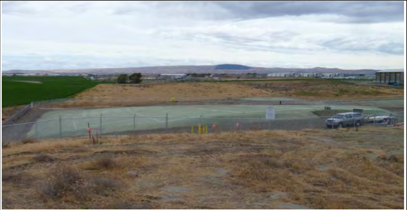
Photo 5: View of the completed CAP, perimeter fencing, hydroseeding, and irrigation system (currently installed in the picture). View of the CAP from area NE of the CAP.
