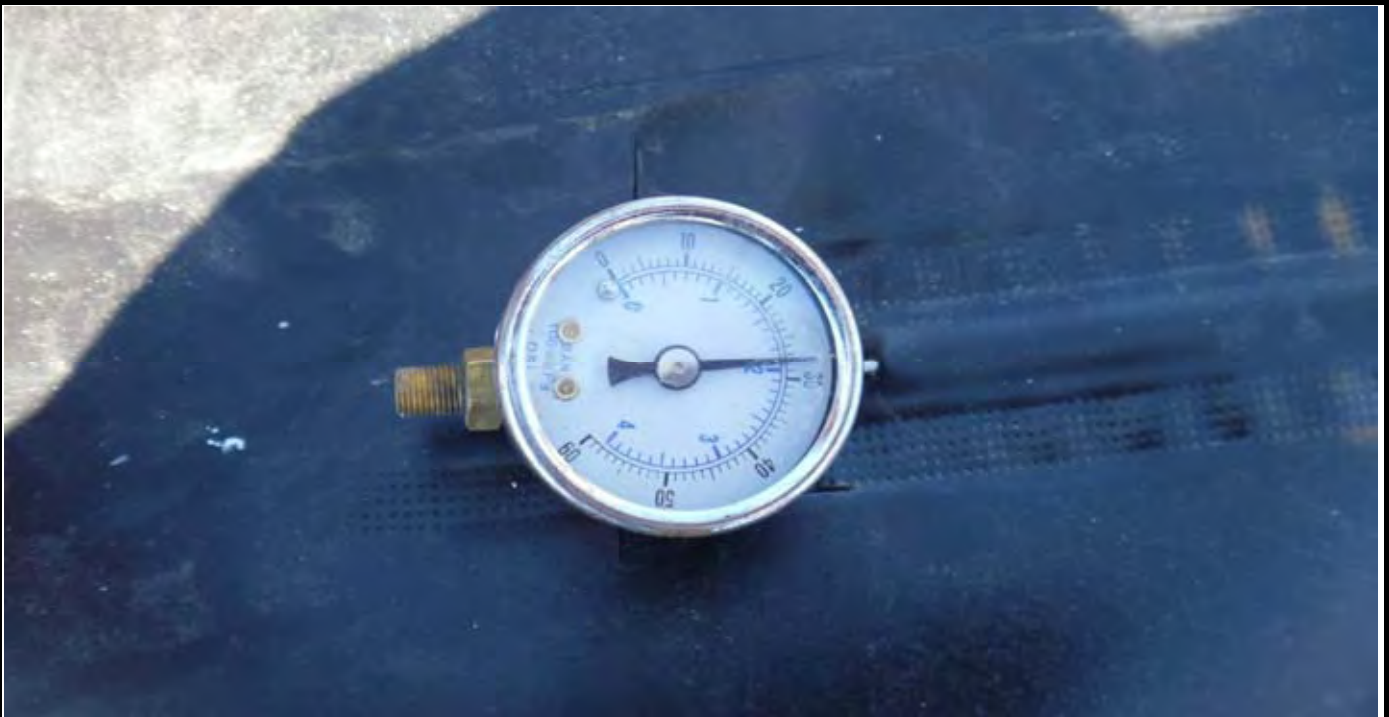
Photo 11: View of the pressure gauge monitoring the inflated welded seam between geomembrane pass P-1 and P-2. Note pressure is about 28 psi. This weld held pressure and was approved by AMEC. View looking down at pressure gauge assembly located new the SW corner of the EOL.
