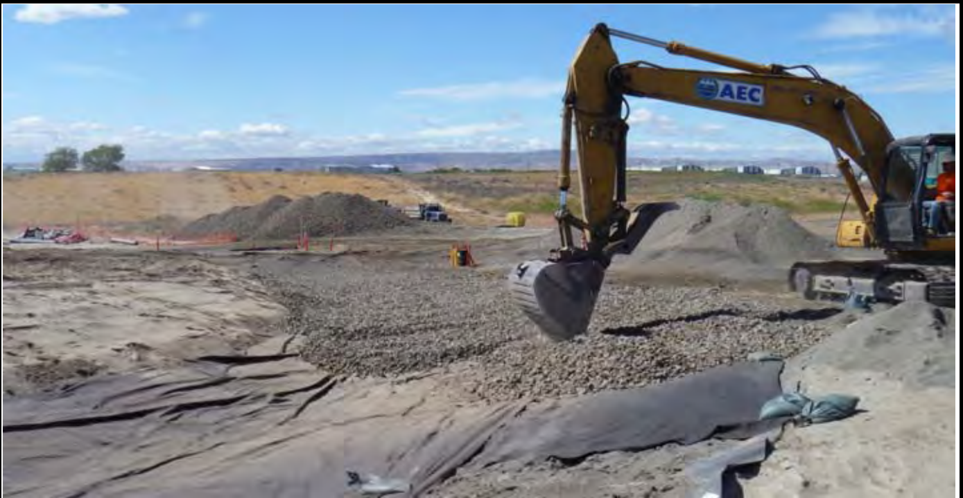
Photo 3: View of AEC installing perimeter rock over the Geo-Fabric (over the sand layer) along the northern end of the western swale area. View looking south from NW corner of the EOL.
