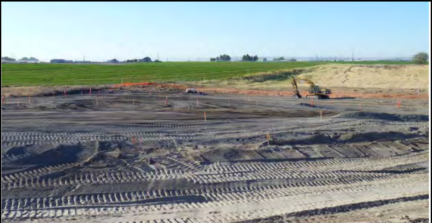
Photo 1: View of the site at the beginning of work for the day. View looking to the South / SE towards the trackhoe.
