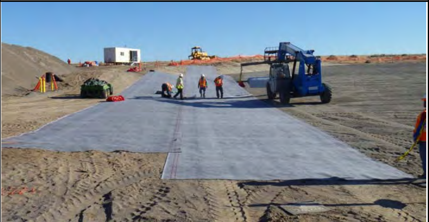
Photo 4: View of the first two GCL rolls laid out along the western side of the EOL and CAP area. Note remaining roll of GCL on telehandler is getting ready to install it along the northern EOL. View looking north from SW corner of EOL. Note that NWL will trim up the southern EOL later.
