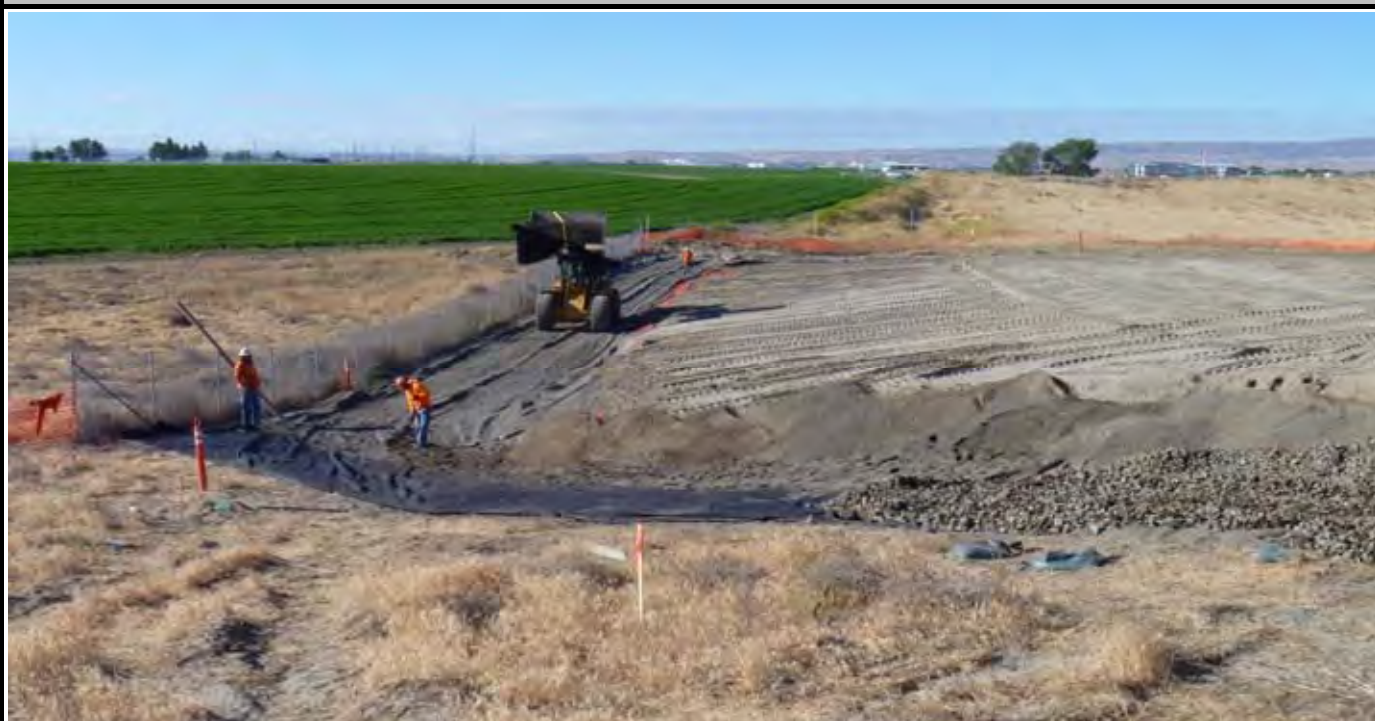
Photo 3: View of AEC working on the NE and eastern swales. Note loader bringing roll of Geo-Fabric to be installed over the sand layer on the eastern swale. View looking south from NE corner of the site.
