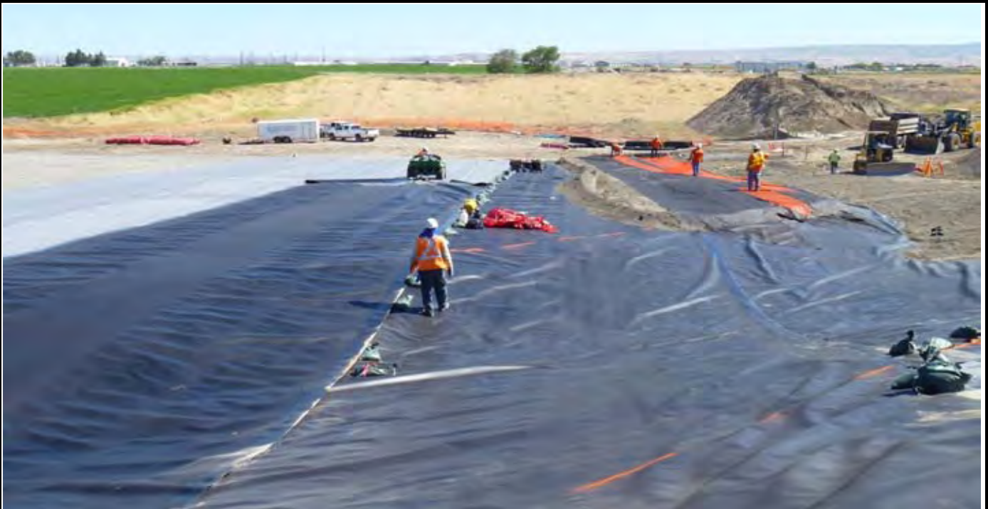
Photo 16: View of NWL installing 4th pass (P-4) of the geomembrane along the eastern edge of pass P-3. View looking south from northern EOL.
