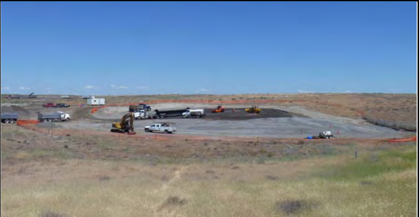
Photo 3: View of the Cap area during G-layer grading work. Note side dump truck, roller, bulldozer, and watering truck on cap. View looking north from area beyond south end of the site.
