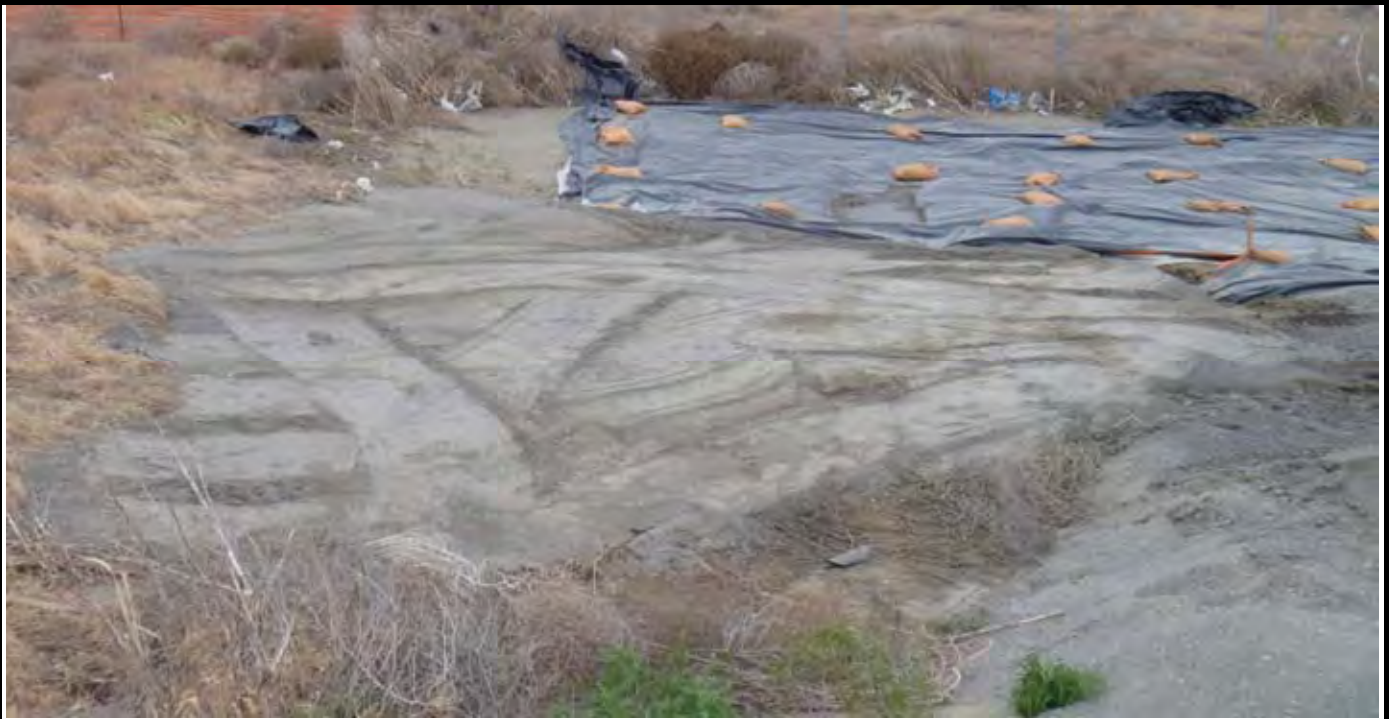
Photo 5: AE-3 backfilled and compacted to existing grade. View looking east from NW corner of AE-3 excavation.
