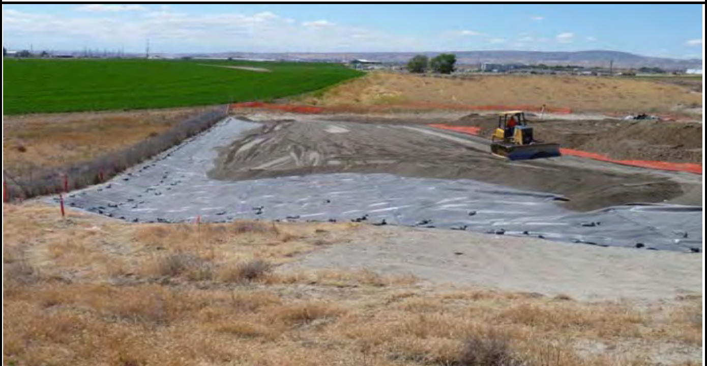
Photo 6: View of the eastern edge of the CAP showing the NE swale prior to sand and grading work. Note bulldozer grading sand layer. View looking south from NE corner of the site.
