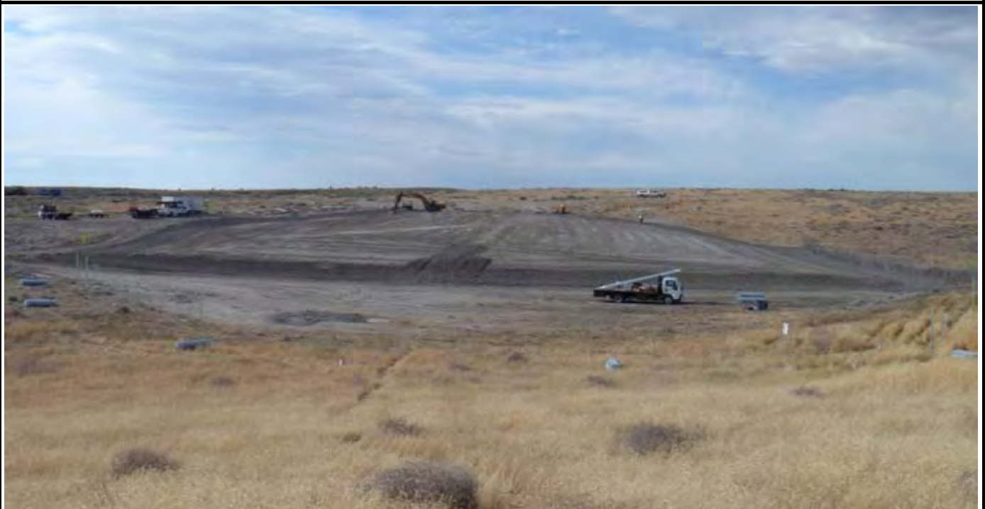
Photo 10: View of the site near the end of the work day. View looking north from area south of the site. Note Rick's Custom Fencing crew trucks, posts, and equipment.
