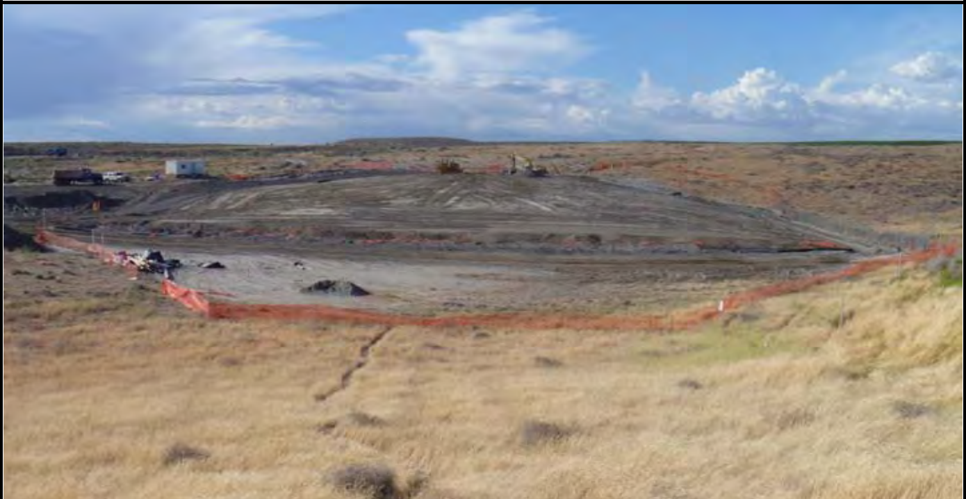
Photo 10: View of the site at the conclusion of work for the day. Note the change in the surface grade of the top of the CAP and the work completed on the SE corner of the CAP and western swale. View looking north from area south of the site.
