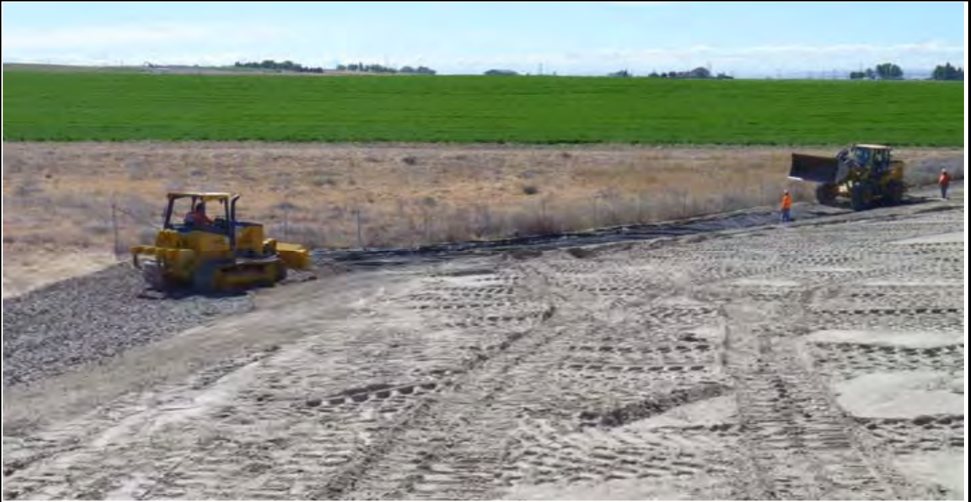
Photo 5: View of AEC grading perimeter rock over the Geo-Fabric in the eastern swale. View looking SE from the northern end of the CAP.
