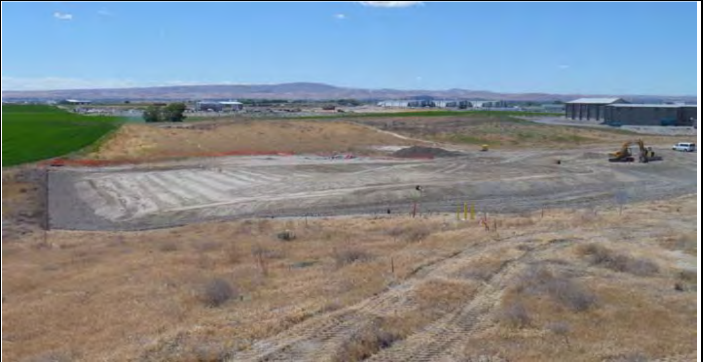
Photo 9: View of the site at the conclusion of the work day. Note the northern and eastern perimeter swales are completed and the top of the CAP is rough graded and ready for final grading on Monday. View looking south from area north of the site.
