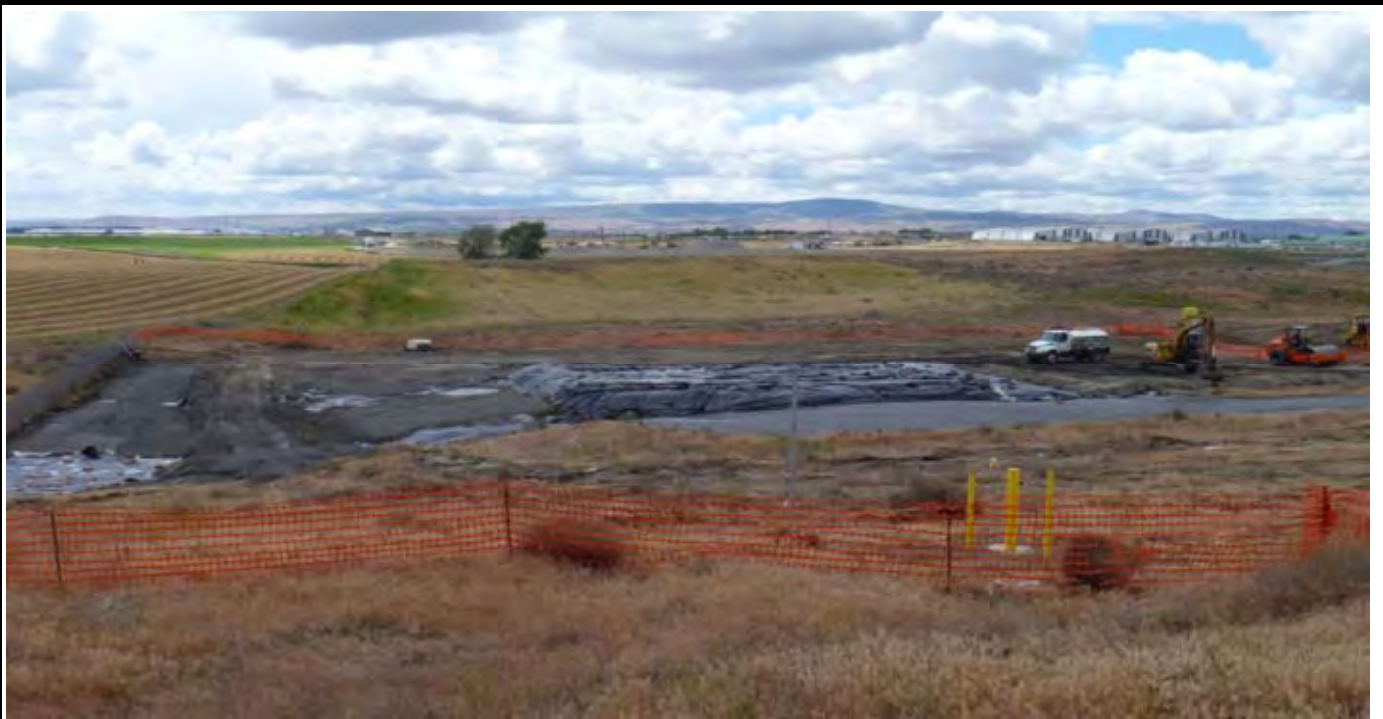
Photo 7: View of the site at the end of the work day from the NE corner. View looking south from NE corner.
