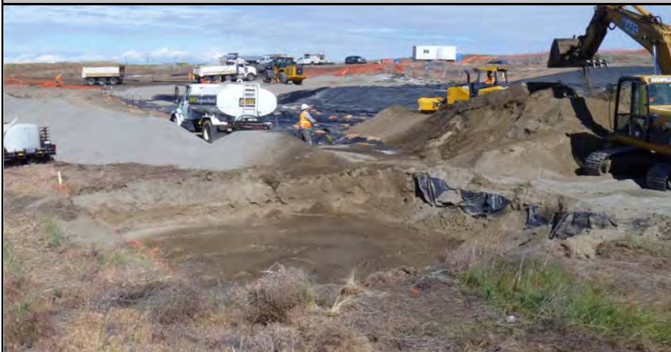
Photo 5: View of excavation AE-5 down to 4-ft bgs. Stockpiled soils from AE-5 shown on the right side of photo.
