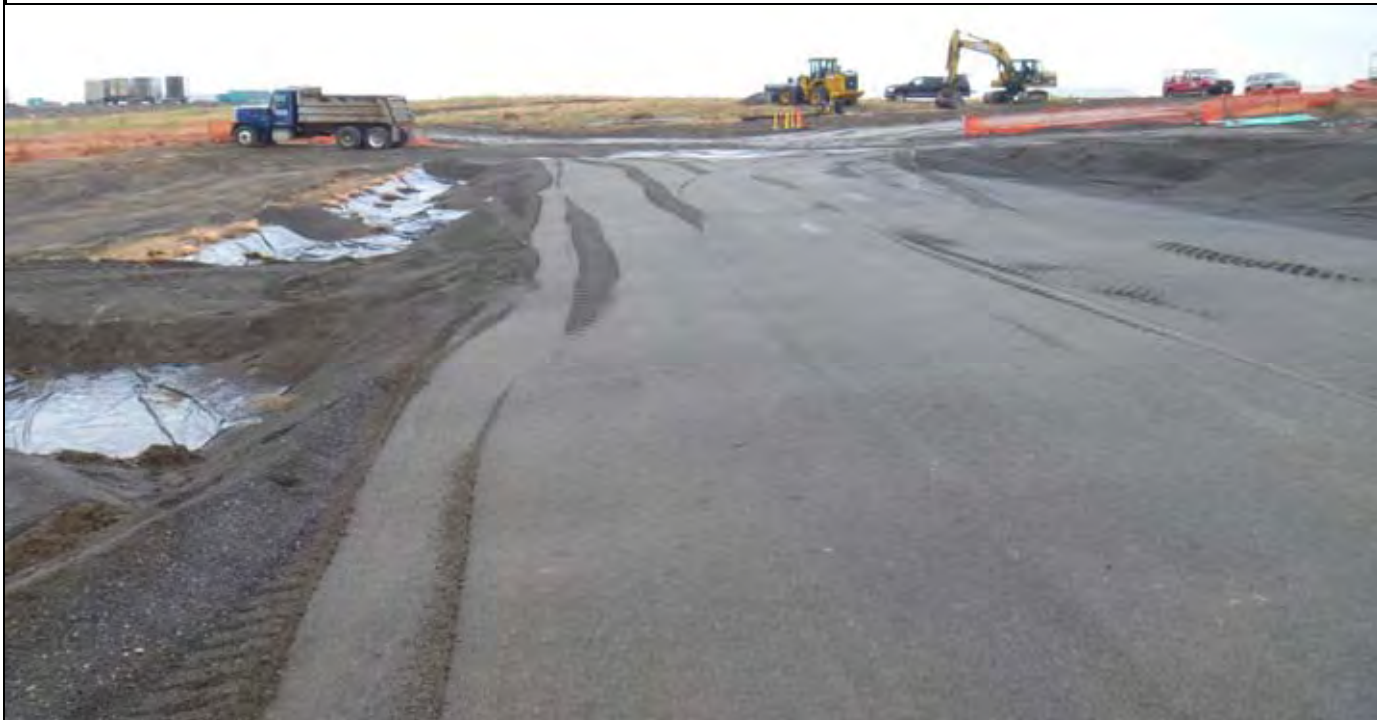
Photo 4: View of the southern edge of the G-layer. Note southern edge of shallow excavation on left site. View of site looking west from area near southern end of AE-4.
