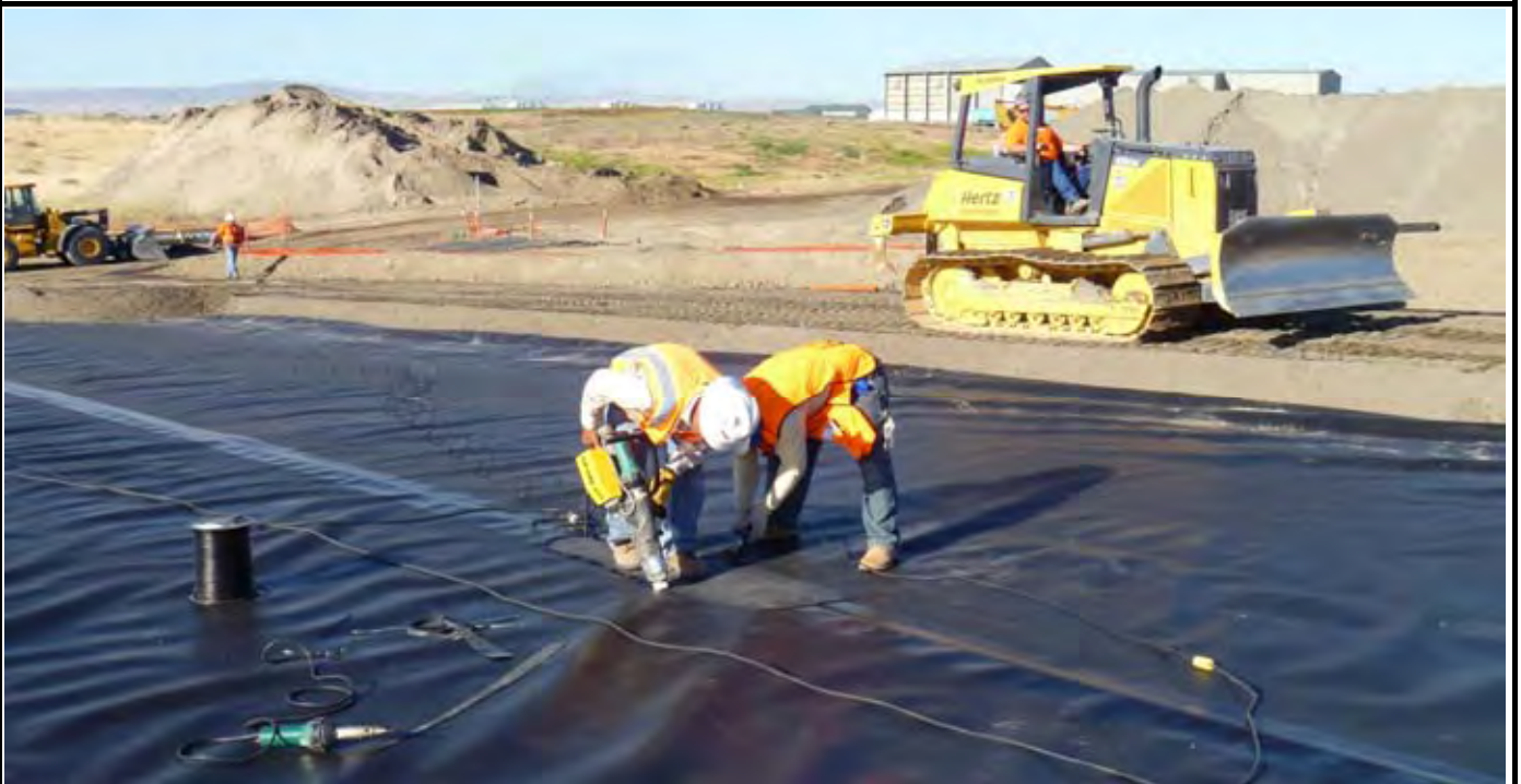
Photo 4: View of NWL crew sealing patch at location of DS-2 sample. Note AEC bulldozer laying out 1-ft thick sand layer on geomembrane panel 3. View looking SW from center of geomembrane panel 5.
