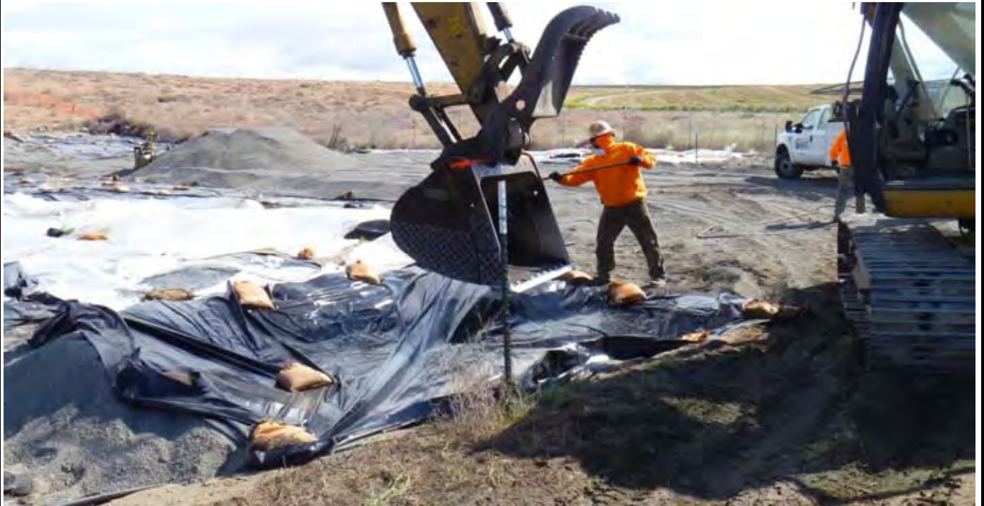
Photo 3: AEC decontaminating the trackhoe bucket over the lined wash sump (SE corner of the site) after excavating AE-3 to 4-ft bgs. View looking east from SE corner.
