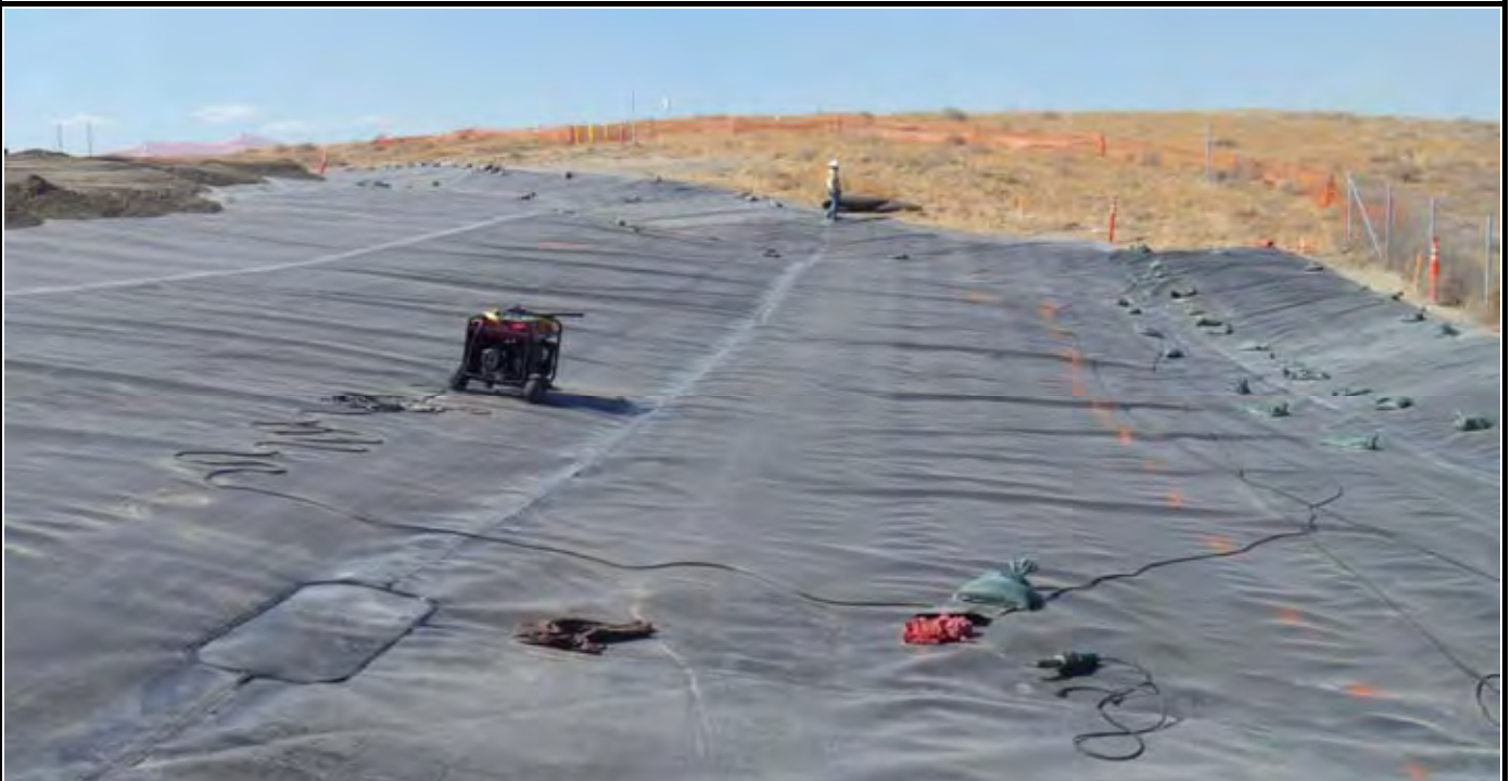
Photo 8: View of the NE corner of the completed geomembrane area (showing NE and east swale area between the EOC and EOL. Note patch for seam sample DS-6 between panels P-12 and P-13. Orange dashed line is the EOC. View looking north from center of the eastern side of the EOC.
