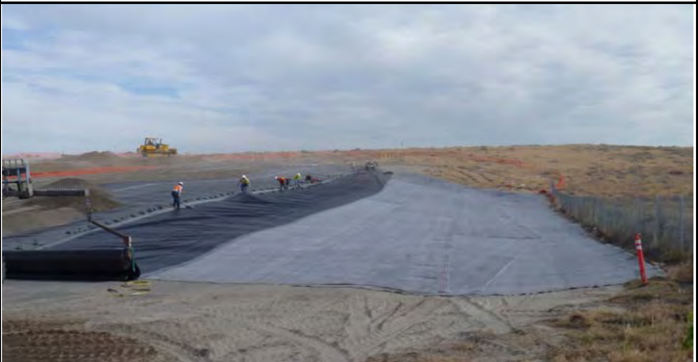
Photo 4: NWL begins rolling out the first geomembrane panel for the day (Panel 11). Note windy conditions and GCL construction along the eastern edge of the CAP. GCL has been installed all the way to the fence line. View looking north from area just south of the SE corner of the CAP.
