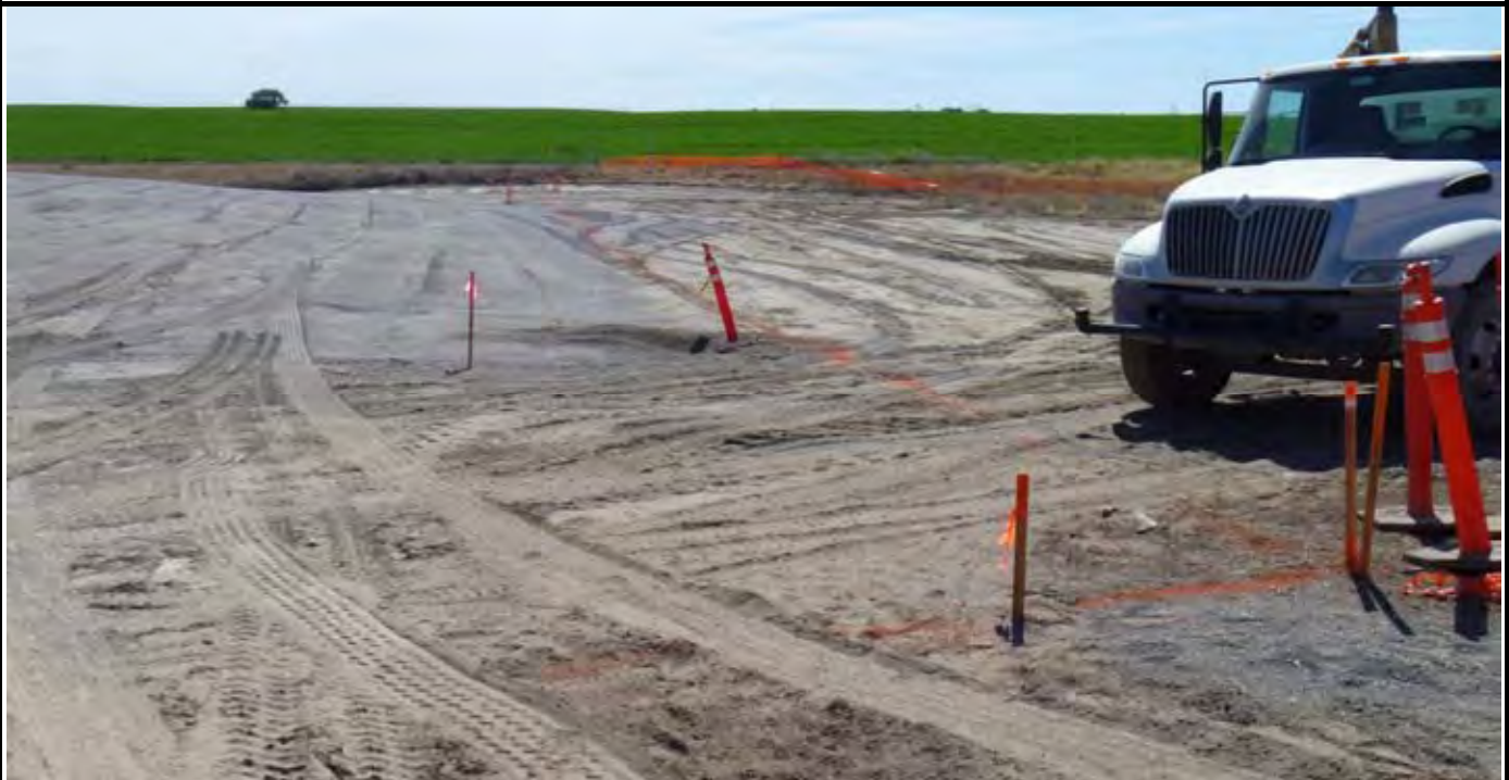
Photo 4: View of the SW corner and the stakes for the EOC and EOL corners and orange marking lines for the boundaries of the EOL. View looking east from SW corner of CAP.
