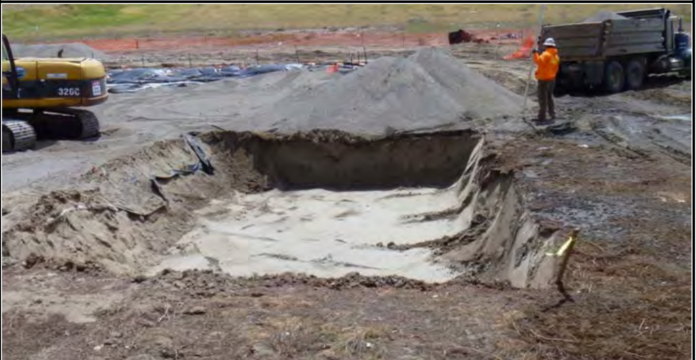
Photo 6: View of AE-2 after final 5-ft bgs excavation work. Note gravel stockpiles that will be used for backfilling AE-1 and AE-2. View looking south from north side of AE-2.
