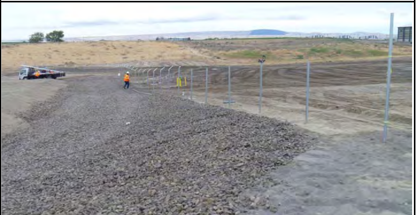
Photo 4: View of Rick's Custom Fencing installing the top bar and barb wire mounts along the western perimeter fence. View looking south from NW corner of the CAP.
