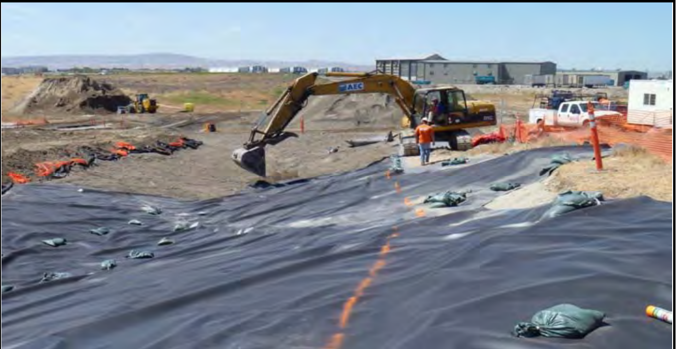
Photo 7: View of AEC laying out thin sand layer over geomembrane in the NW swale area. Note orange dashed line is the EOL for NW swale. View looking SW from northern/northwestern edge of the EOL.
