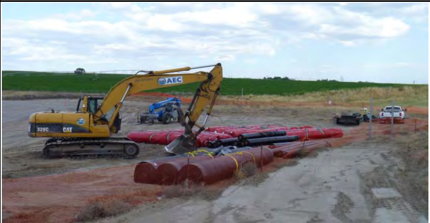
Photo 6: View of all 13 GCL rolls, 3 new geomembrane rolls (black) and 20 geosynthetic fabric rolls (small black rolls). Note NWL crew making sand bags on right side. View looking East from SW corner of the site.
