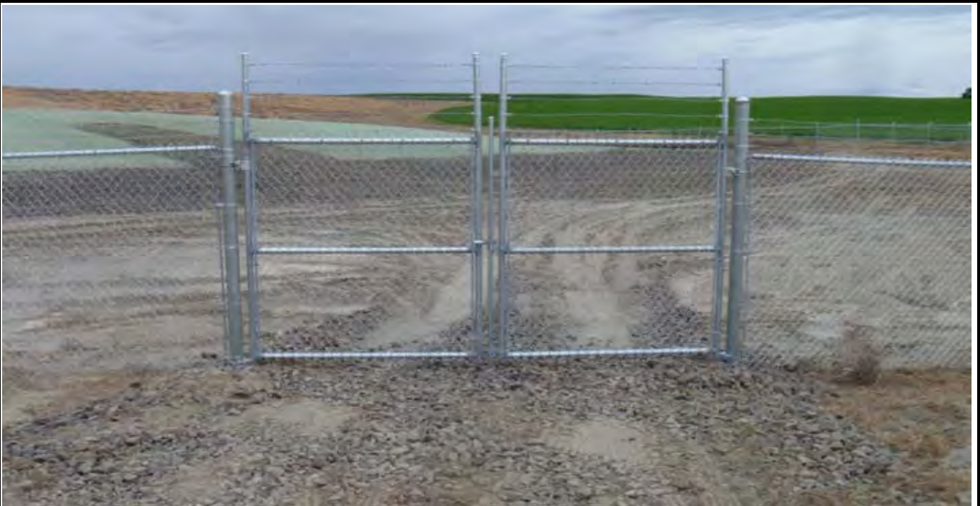
Photo 4: View of the completed perimeter fencing access double swing gate and roadway into the CAP. This work was completed by Rick's Custom Fencing. View looking NE from the SW corner of the CAP.
