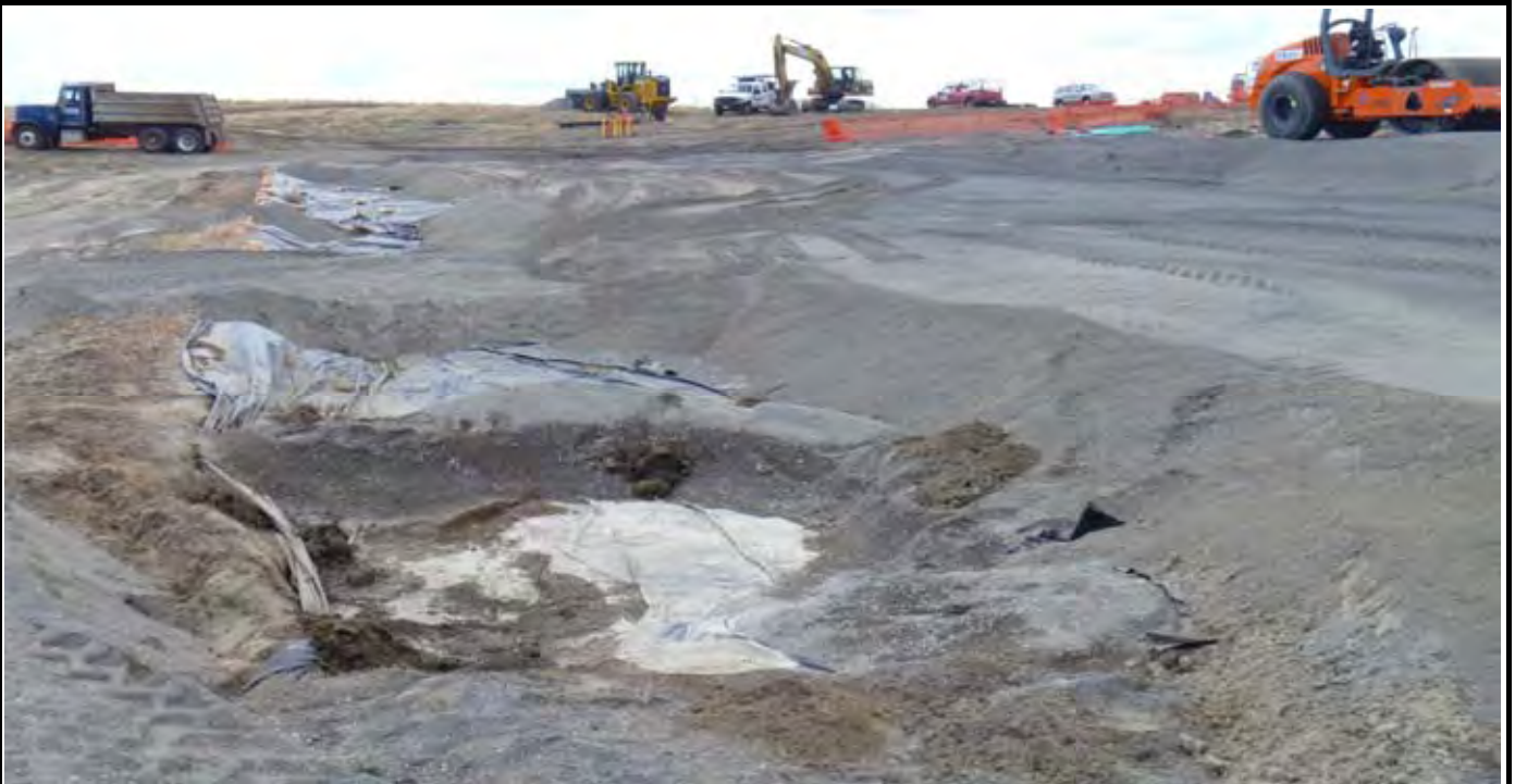
Photo 3: View of the decon pond after decon water has evaporated from the pond. AMEC authorizes burying the pond under the G layer material. View looking west from the SE corner of the CAP.
