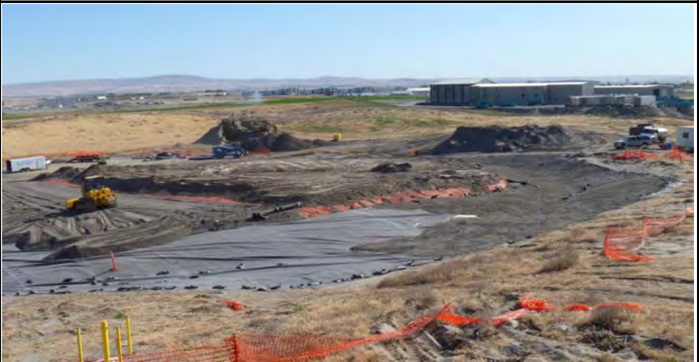
Photo 10: View of the northern and northwestern portions of the CAP. Note sand and topsoil layers (center and left) and the sand layer placed in the northern and northwestern sides of the north and northwestern swale area. View looking southwest to west from area north of the northern OCF.
