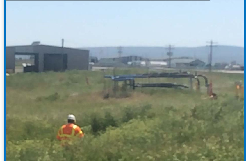
Soil vapor extraction system
