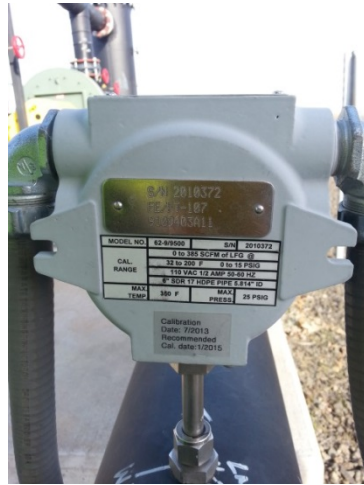
Main Flow Meter located at the Flare Station
