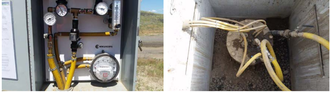
Sump Control Panel and Sump Vault
