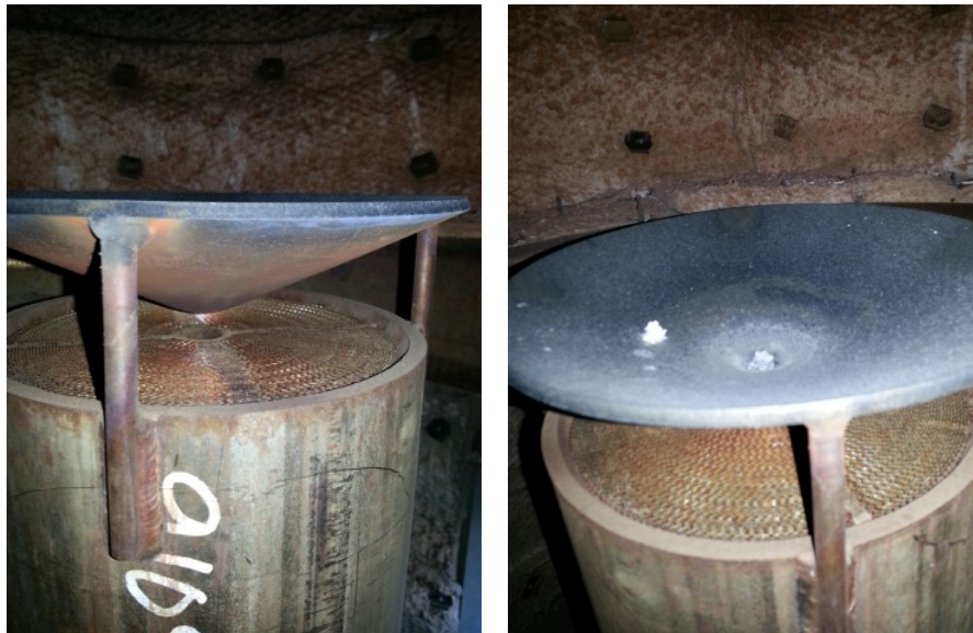
View of Flare Tip (View from Inside Flare)
