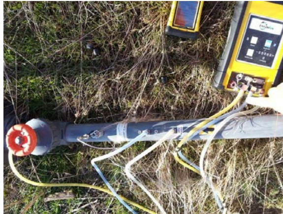
Example of Handheld LFG Analyzer and Wellhead
