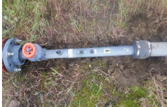
Example of Horizontal LFG Extraction Wellhead
