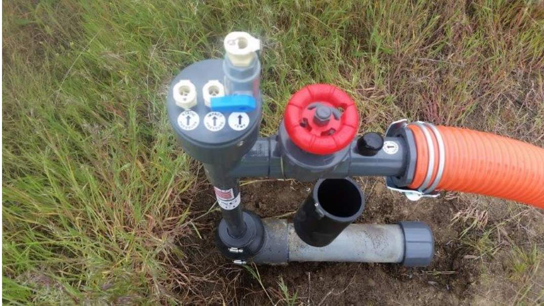
Example of Vertical LFG Extraction Wellhead
