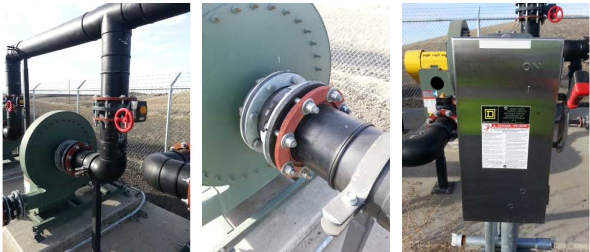
LFG Blower and LFG Power Breaker
