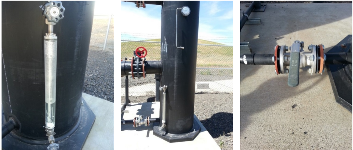
Condensate Knock-out Pot Sight Gauge and Drain Valve
