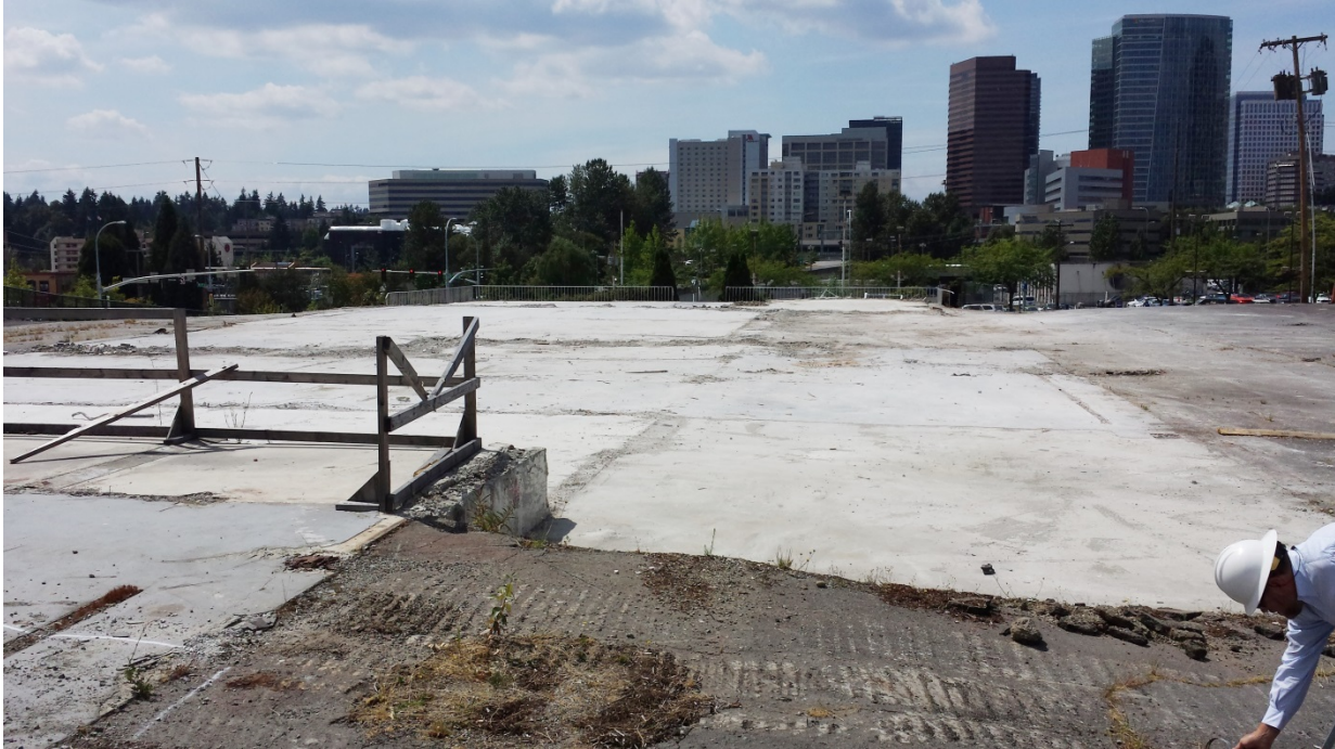
Photo 1: July 22, 2015. View looking west across the former DOB service bay area. Surviving surface features were helpful for locating the initial test pits installed during the supplemental RI.
