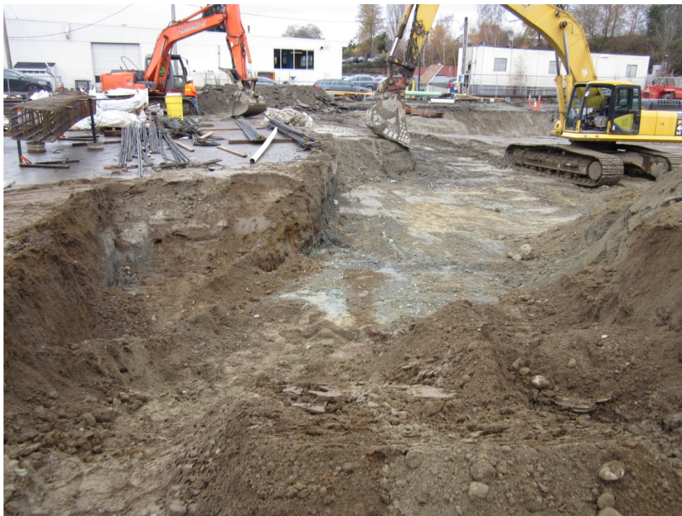
Photo 16: December 2, 2015. View looking north at the TP-16 excavation. The floor of the excavation was at 4 feet below the original grade and coincident with the construction grade.
