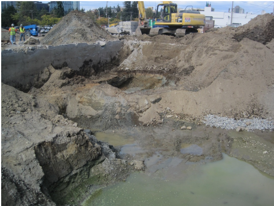
Photo 8: September 24, 2015. Another view of the same excavation later in the day, after the former lube pit area had been excavated (upper center).
