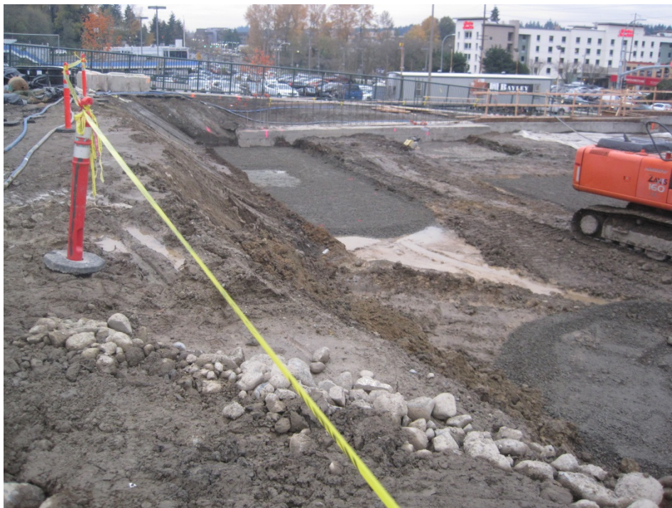
Photo 14: November 23, 2015. View looking south from near the location of the former lube pit. Water discharging from the toe of the slope contained no detectible diesel- or oil-range TPH.
