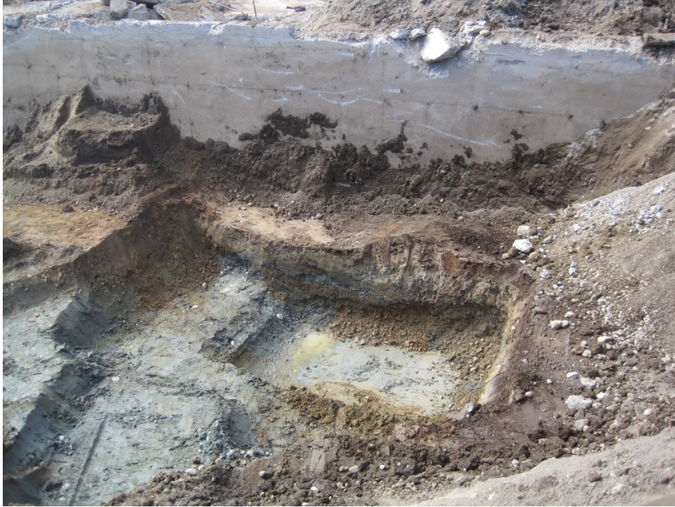
Photo 9: September 24, 2015. View looking west at the completed excavation at the former lube pit. The subsurface concrete wall was present along the west edge of the service bay area.
