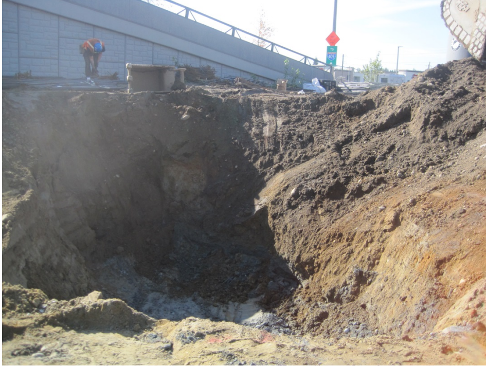
Photo 11: October 16, 2015. Excavation of the additional hydraulic lift vault. A limited volume of contaminated soil was identified on the west side of the vault footing.
