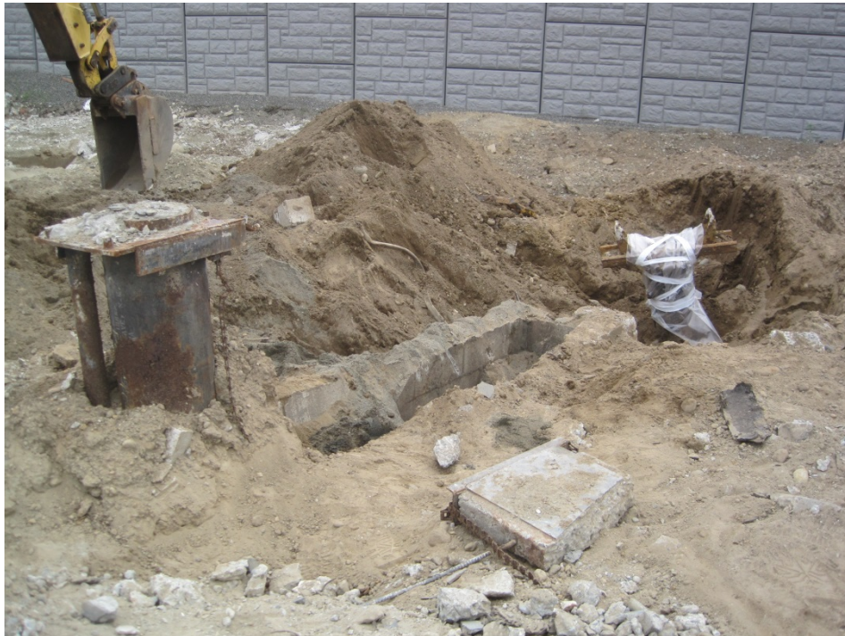
Photo 10: August 14, 2015. View looking southeast at the additional hydraulic lift vault. This lift assembly and vault were situated east of the other lifts. (See also Photo 11.)
