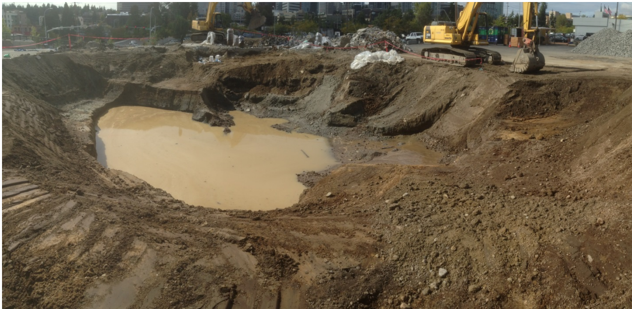
Photo 6: September 8, 2015. View looking west at the enlarged hydraulic lift excavation. Water was periodically pumped from the excavation and hauled for proper off-site disposal.
