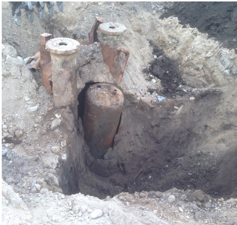
Photo 4: August 28, 2015. View one of the hydraulic lifts being removed. The two lift pistons and the hydraulic fluid reservoir are visible.
