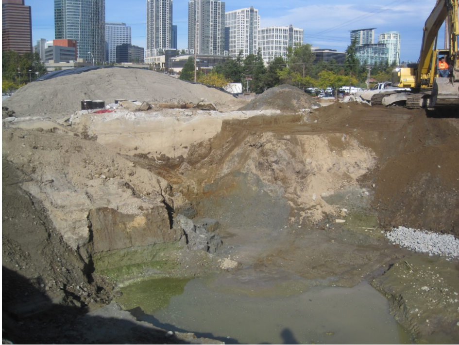
Photo 7: September 24, 2015. View looking northwest at the hydraulic lift excavation. The excavation water supported an algae bloom during the two weeks that the excavation was open and site activities were devoted to construction.
