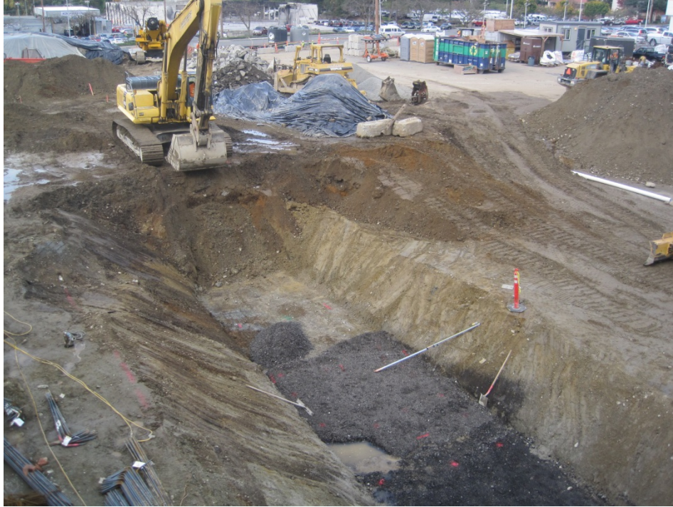
Photo 13: October 21, 2015. View looking northwest at a footing excavation being advanced into the area of the hydraulic lift remedial excavation. Note the difference in elevation between the original grade (left and top), the construction grade (right), and the footing grade (bottom center).
