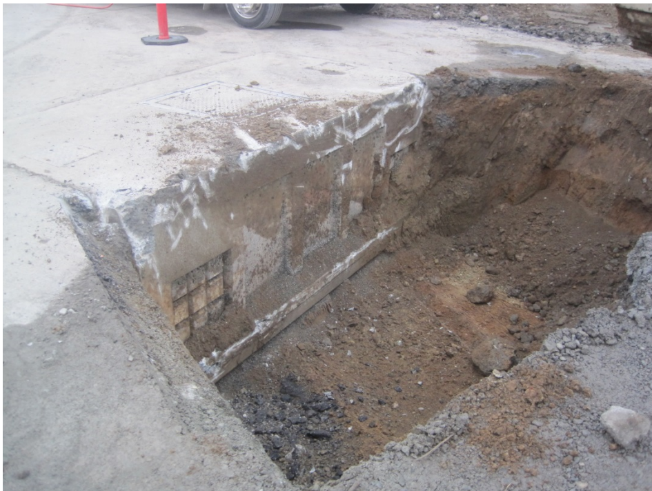
Photo 12: October 14, 2015. View of the removal of the north oil/water separator. Two smaller oil/water separators were removed on the same day. Field observations, PID readings, and the analytical results of confirmation soil samples indicated that the surrounding soils were clean.
