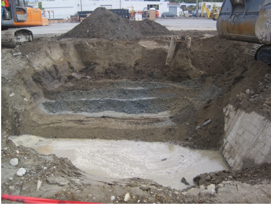
Photo 5: September 3, 2015. View looking north at the excavation being installed to remove PCS that was identified beneath the hydraulic lifts at approximately 4 to 8 feet bgs. Analytical chromatographs and on-site odors indicated that the contaminant was mineral spirits.
