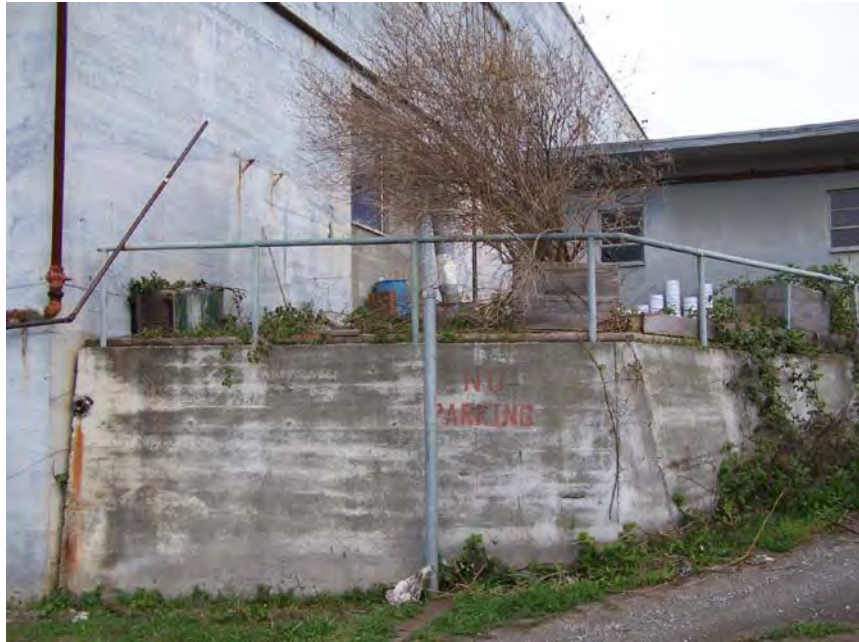
Figure 6. View of the retaining wall south of the southwestern portion of the building, looking east. The dry cleaning operations occurred within the main building in the left side of the photo and the building addition is visible in the background on the right hand side of the photo.
