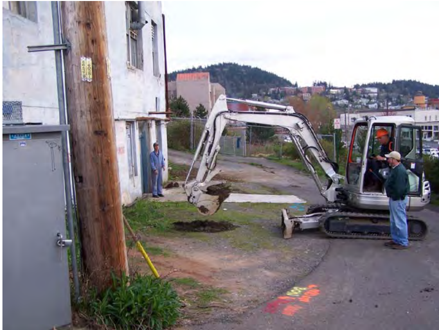
Figure 8. View of test pit #5 being excavated along the west side of the building, looking south. Disturbed material is visible in the back-central of the photo where test pit #3 was excavated. The closed-in-place underground gasoline tank is located just beyond the telephone pole in the forefront of the photo where the dirt looks reddish.
