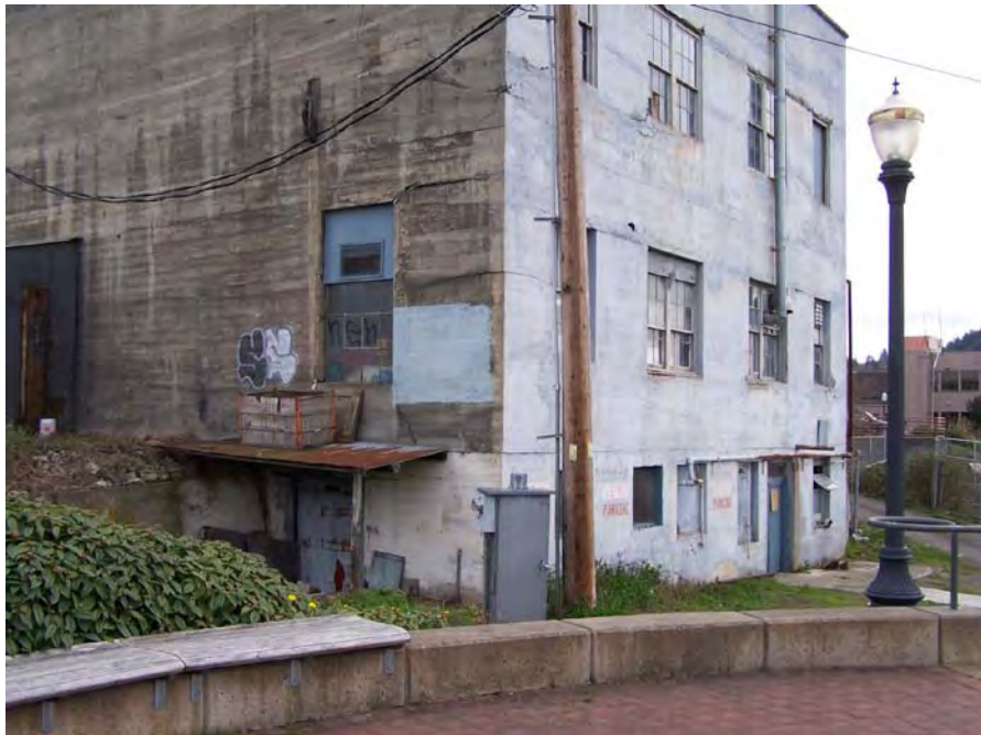
Figure 5. View of northwest corner of the Cascade Laundry building, looking southeast. Note the retaining wall and fill material on the left side of the photo. The underground storage tank used to hold fuel for the boiler is located near the building within the fill material.
