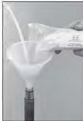
Figure 3. Glass Beads create a permeable layer around vapor sample implants.
