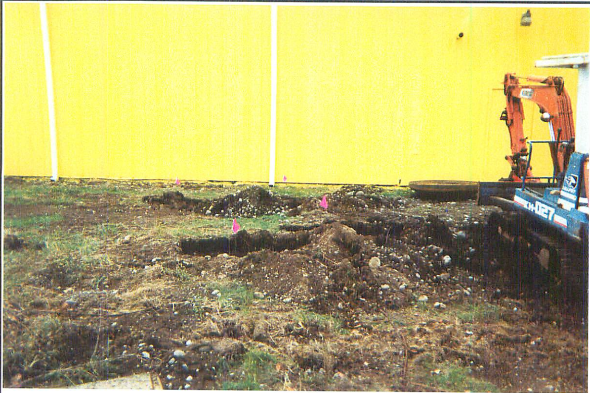
Photo #11: Photograph depicting the depressional area in the lower left corner, facing west. Excavated trenches indicate where soil samples were collected. Photo taken on 11/15/02.
