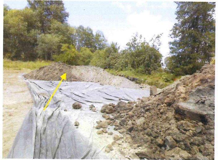
Presumed contaminated stockpile
