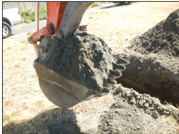
Test Pit TP-6: View of Beach Deposit soils from test pit excavation.
