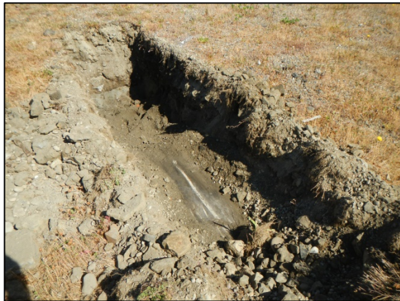
Test Pit TP-6: Top of intact concrete slab encountered at 1½ feet below grade. Test pit was moved 10 feet to the northwest.
