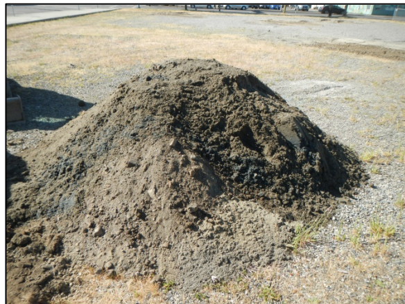
Test Pit TP-5: View of spoils pile after completion of test pit.
