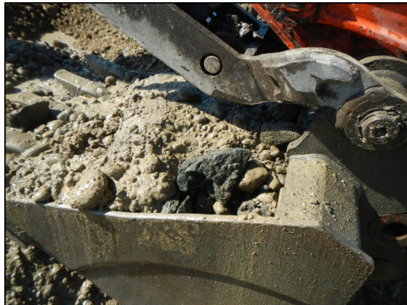
Test Pit TP-4: Soils in excavator bucket from bottom of test pit. Mixture of quarry spalls and gravel borrow fill.
