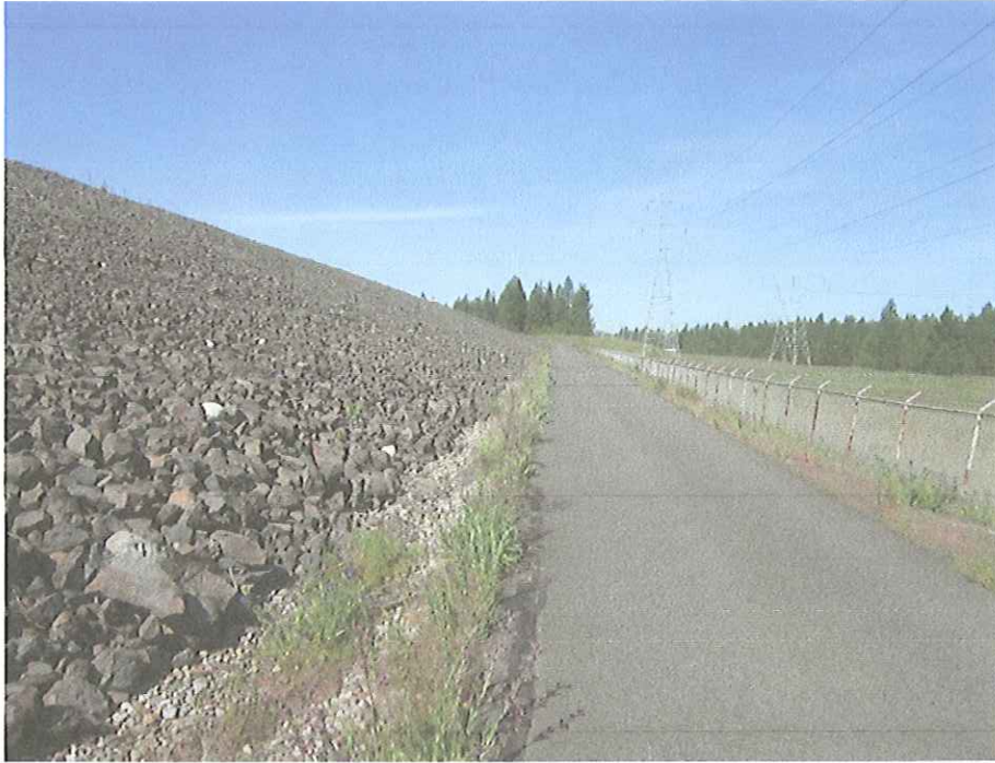
Photo 3: Photograph showing SPL Pile perimeter ditch along north perimeter road looking west.
