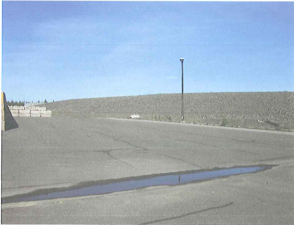
Photo 1: Photograph of asphalt area southeast of SPL Pile showing ponding.
