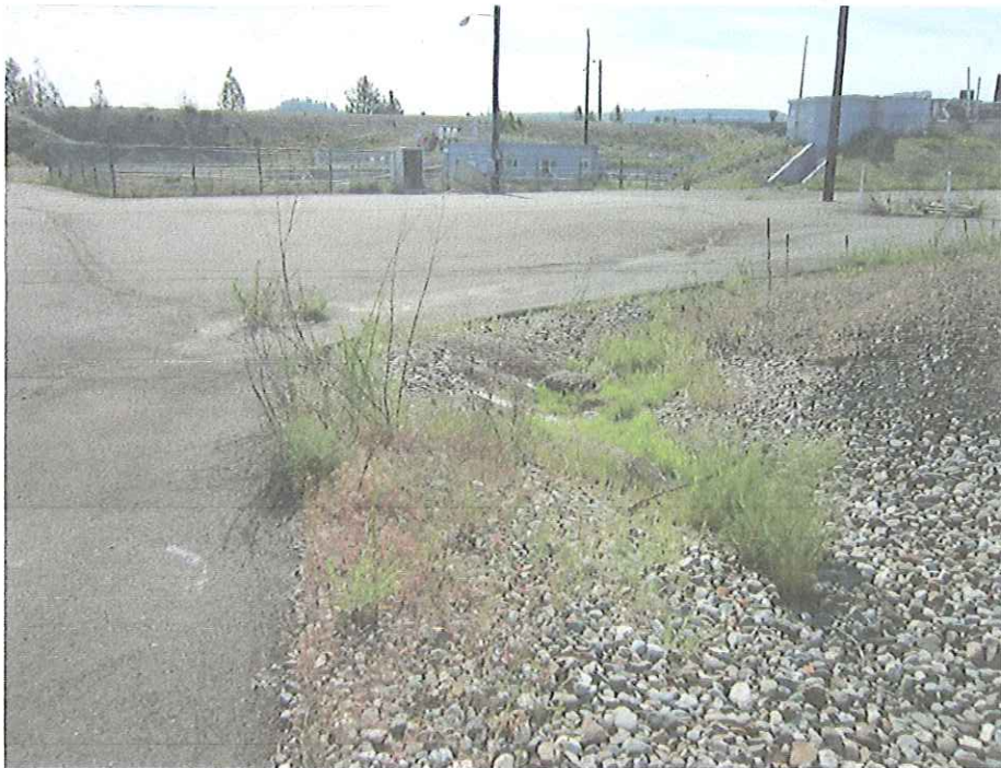
Photo 2: Photograph of perimeter ditch drainage into northeast storm water drain looking east. Vegetation is not impeding flow.
