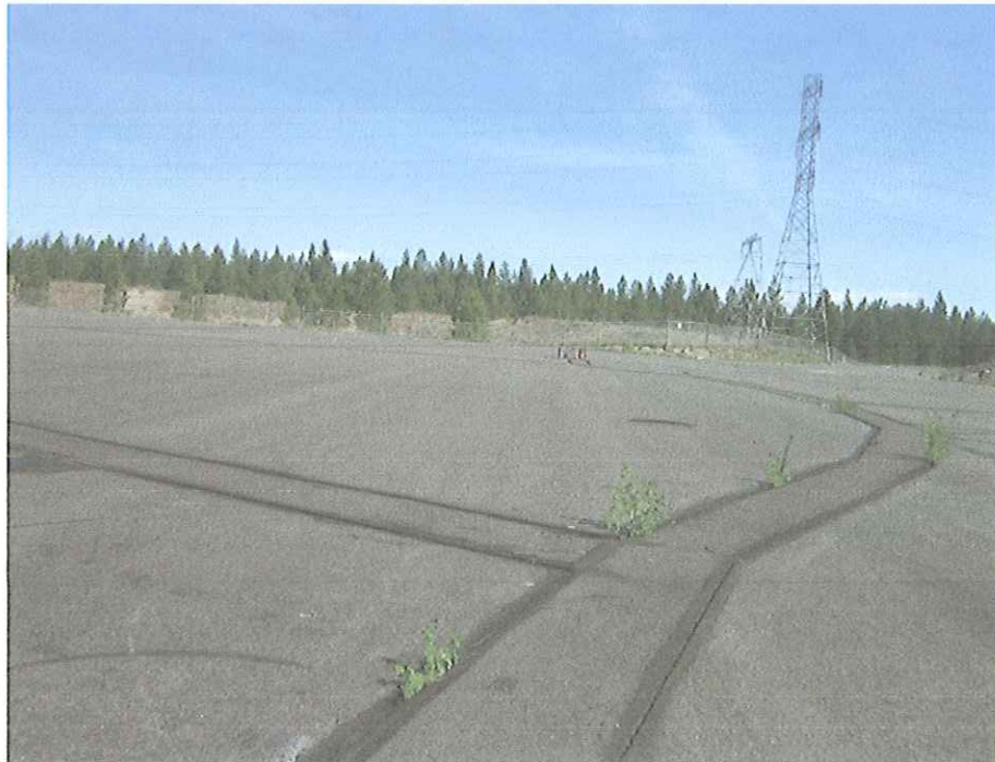
Photo 8: Showing asphalt cracks west of SPL Pile cap looking north.
