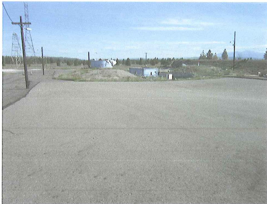
Photo 2: Photograph of asphalt area east of SPL Pile (Area 2) looking north showing good condition.
