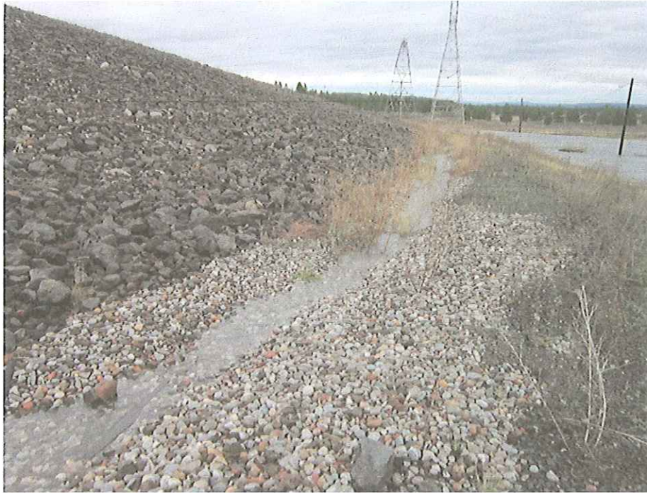
Photo 1: Photograph showing flowing ditch along southeast corner of SPL Pile looking north.
