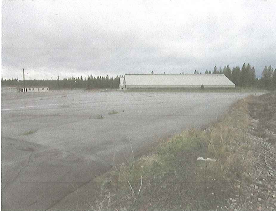
Photo 3: Photograph of asphalt area west of SPL Pile looking west showing some cracks.
