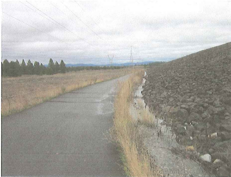
Photo 3: Photograph showing SPL Pile perimeter ditch flowing along north perimeter road looking east.
