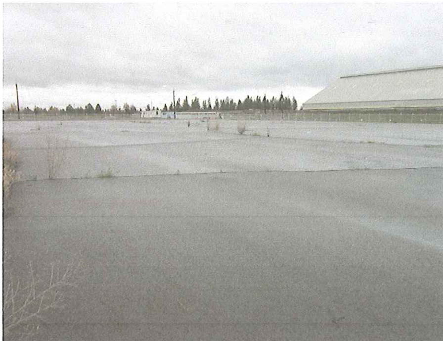
Photo 4: Photograph showing asphalt west of SPL pile looking southwest, showing cracks.
