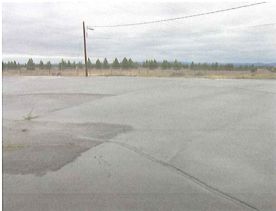
Photo 2: Photograph of asphalt area northeast of SPL Pile looking northeast showing good condition.
