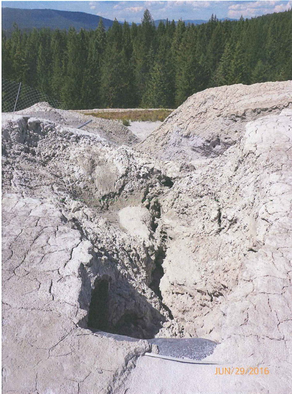
7. West Cell north side dam crest, looking downstream. Erosion damage above PVC liner.
