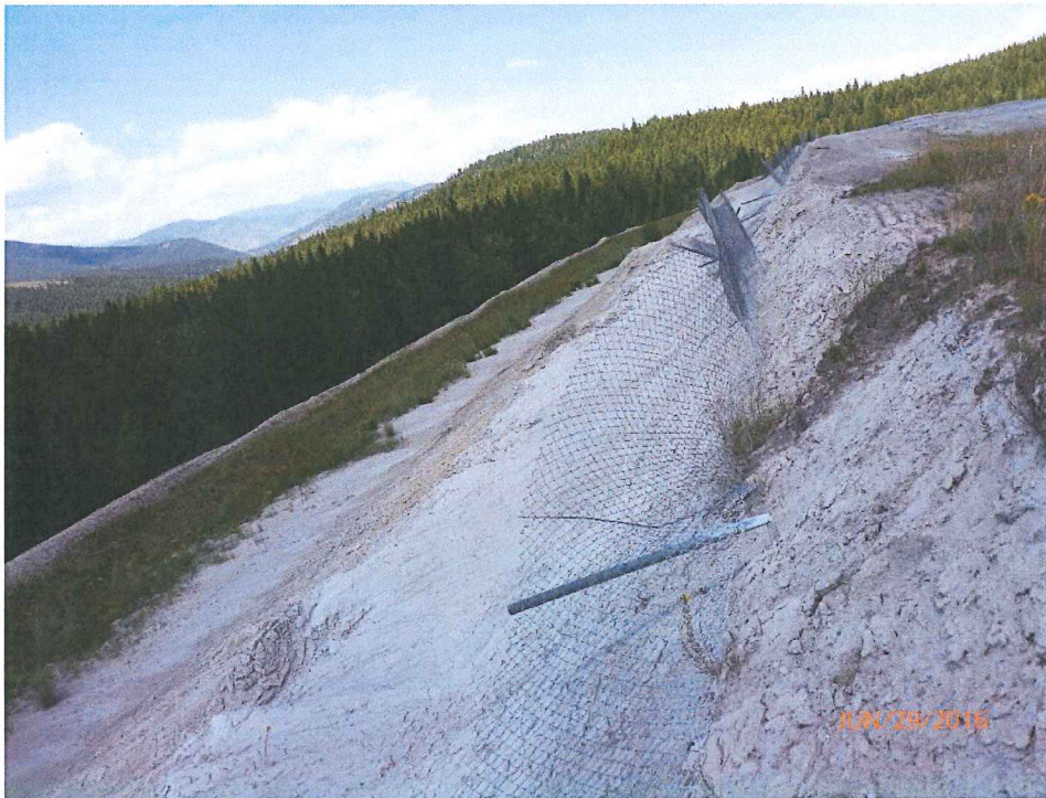
9. West Cell west side downstream face, looking right. Soil movement (slumping).
