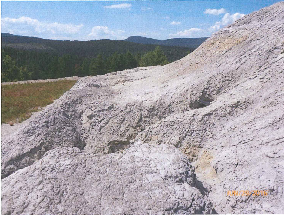
12. West Cell south side downstream face, looking right. Erosion.
