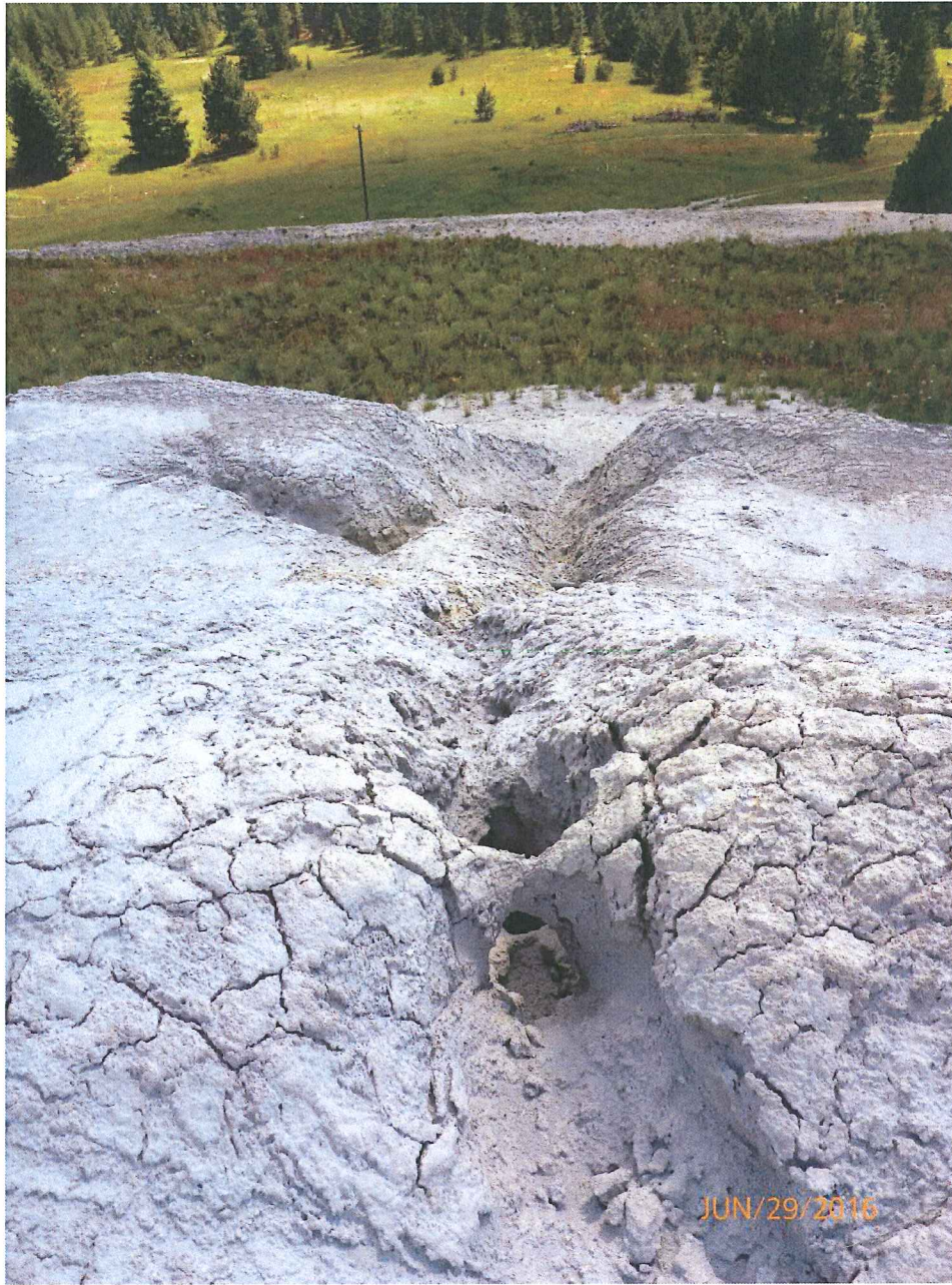
10. West Cell south side downstream face, looking downstream. Erosion damage includes piping.
