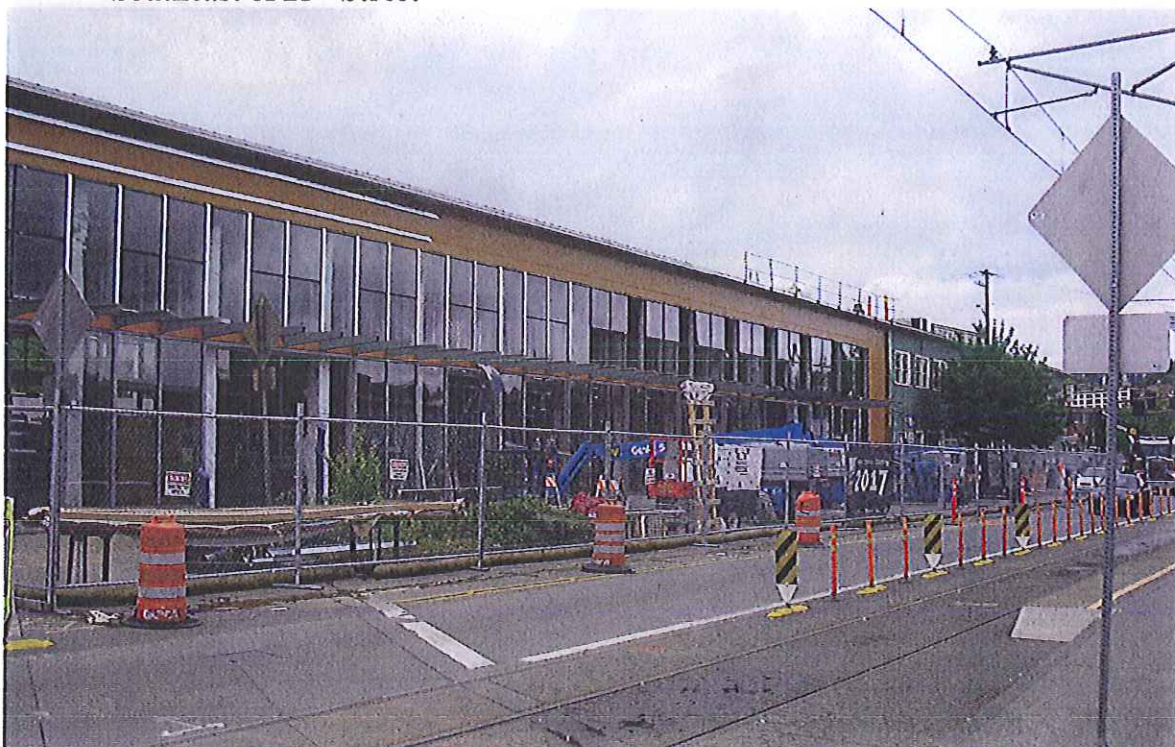
Photo 6: North Side of Building, New Amtrak Train Station Construction—from the Southeast of 25 th Street
