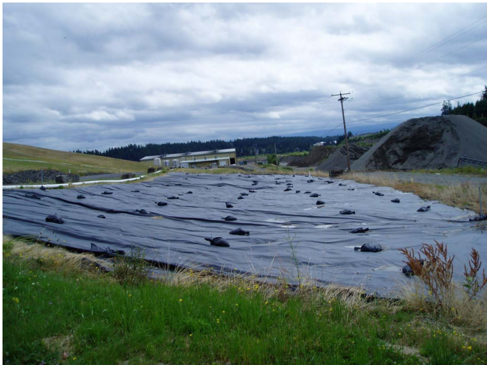
Sink Hole Repair Area – Facing west toward transfer station
