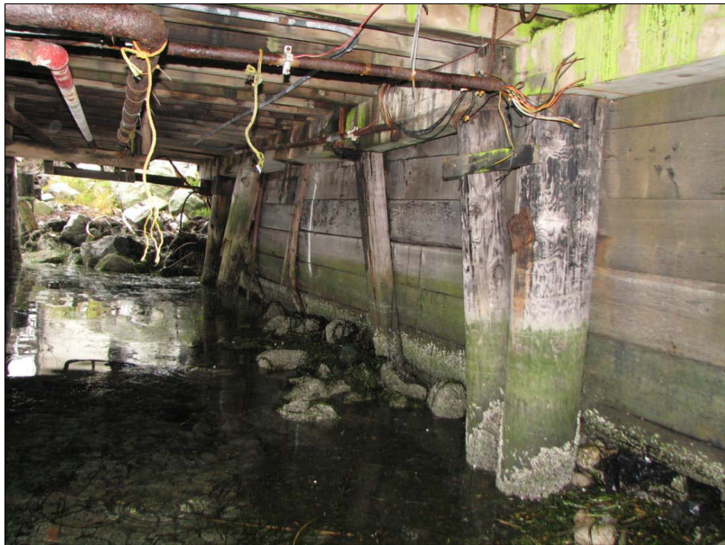
Photograph 2: Aging timber soldier pile bulkhead beneath fuel office, November 7, 2011.
