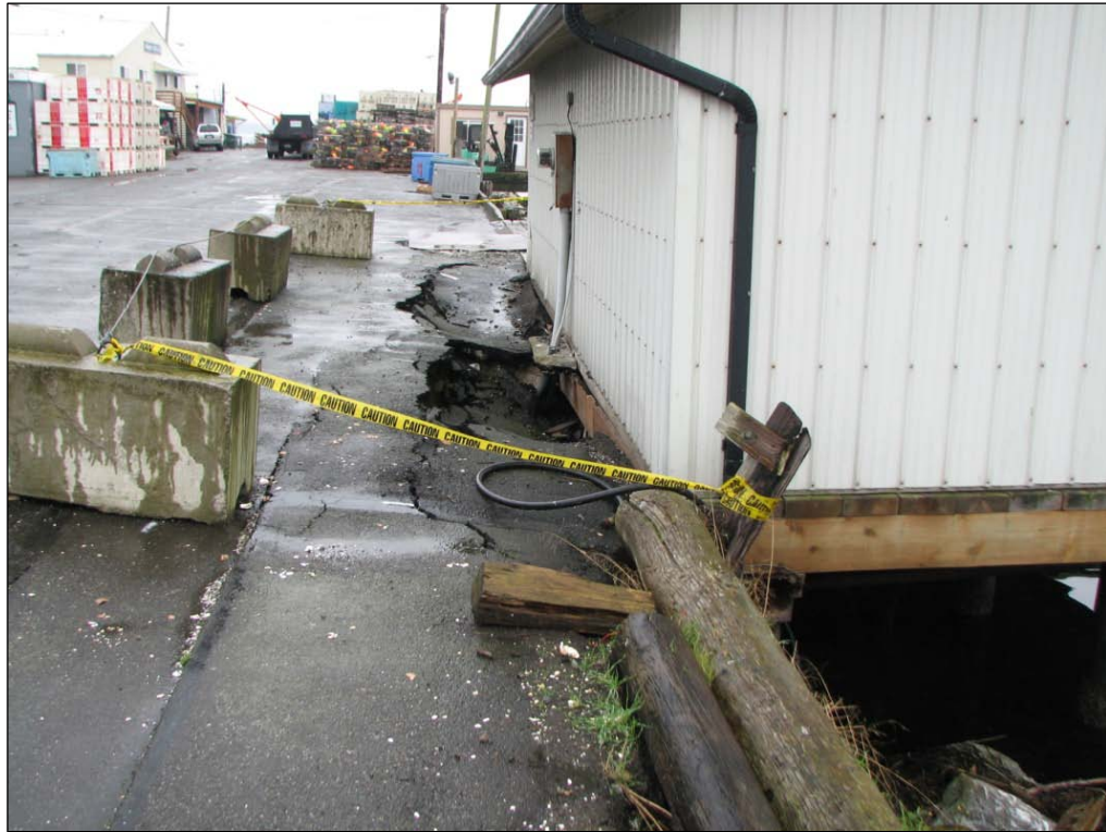
Photograph 1: Collapsing pavement at bulkhead near fuel office, November 7, 2011
