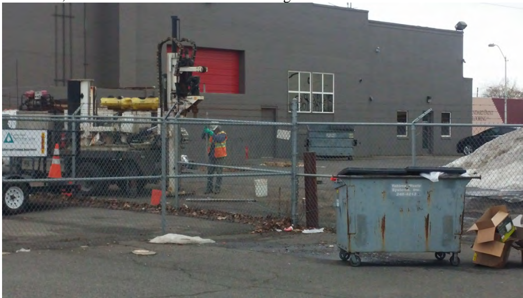
Drilling at location B-5. For reference, monitoring well CNGMW-9 is the white flush mount monument in the foreground approximately 10 feet left of the dumpster.
