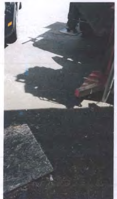
View of the AMS Powerprobe set up to drill boring B5E located near the eastern side of the building.
