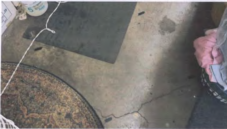
View of the floor inside the All Star Cleaners near the pretreatment area. Darker gray area appears to be a patch from a previously completed boring. No report of this investigation was available.
